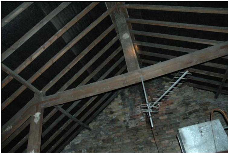
Figure 17 The roof truss near the north end of the building. The truncated principal rafters, queen posts and collar beam are connected by iron straps: N
