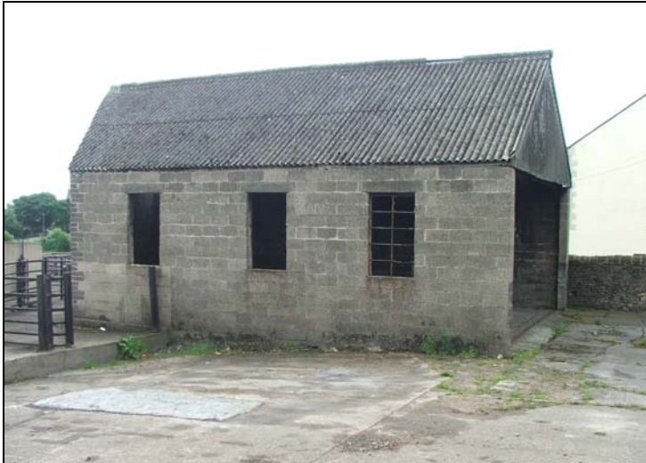
Figure 7 Former coal depot building at the north end of the site: S
