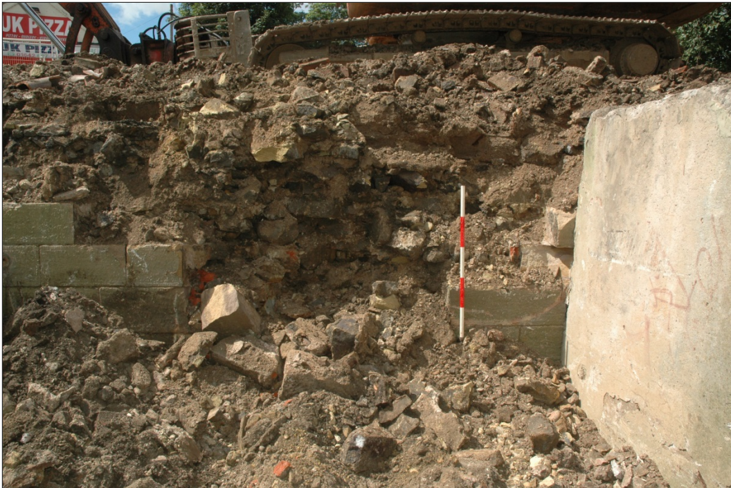
Figure 37: View of the backfill in the span between piers 2 and 3, looking south-west
