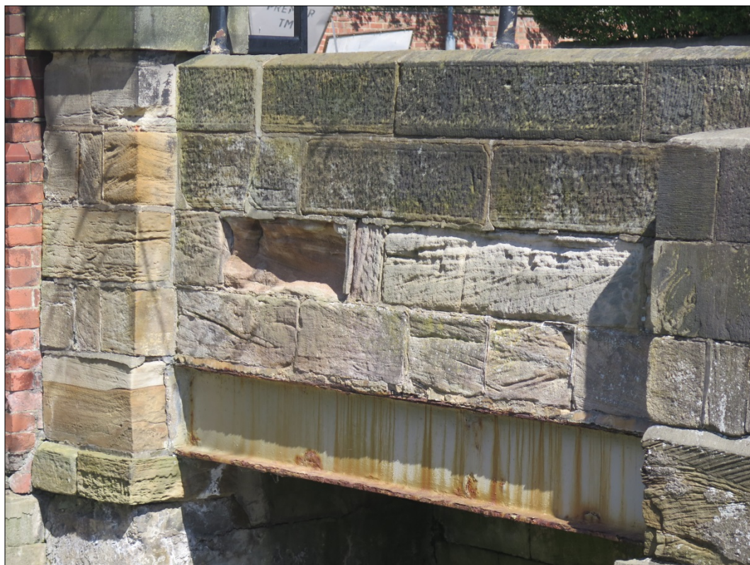
Figure 17: South-western elevation, detail of eroded blocks in the parapet, looking north
