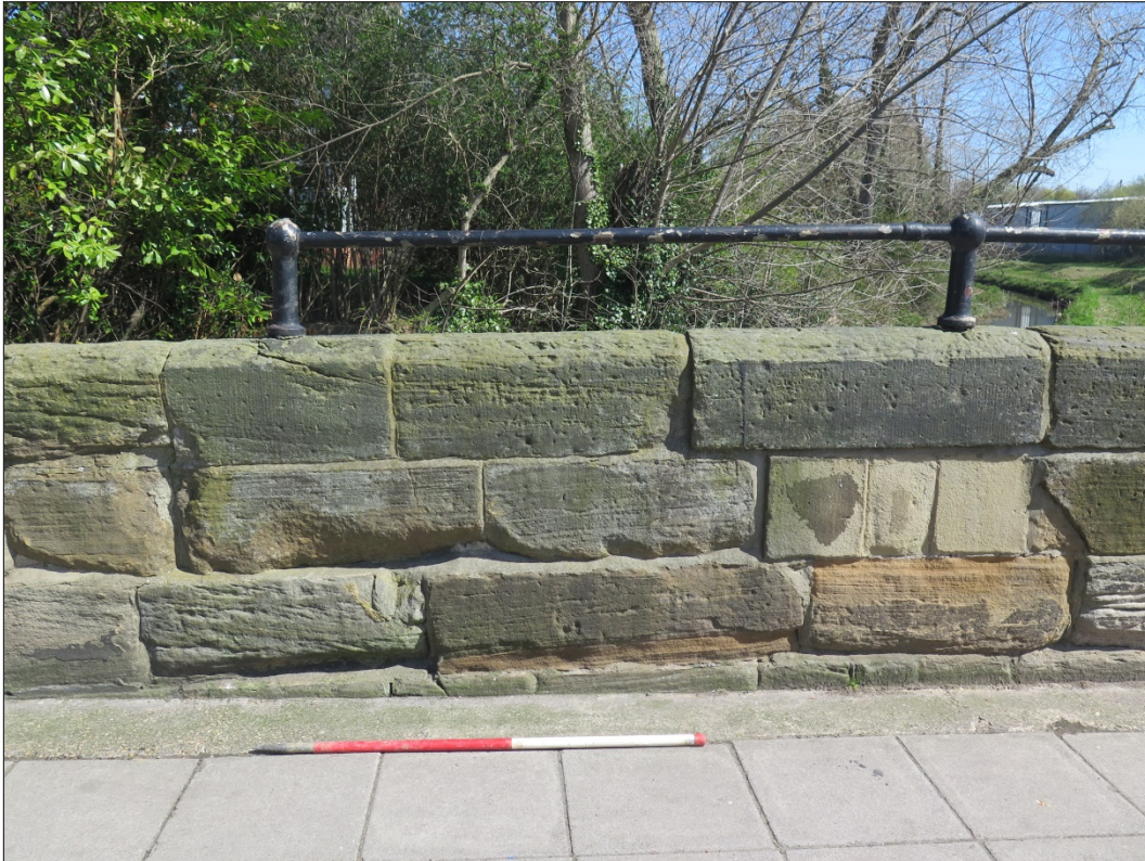
Figure 24: North-eastern inner parapet, showing eroded and replaced blocks, looking north-east
