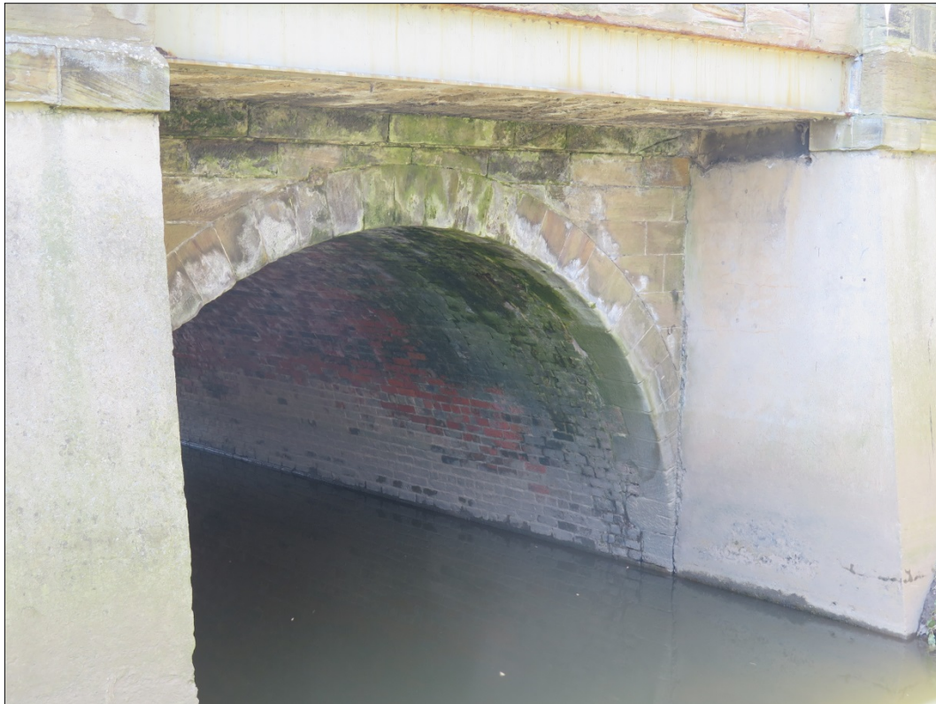
Figure 14: North-eastern elevation, detail of main channel showing internal brickwork of the barrel arch, looking west
