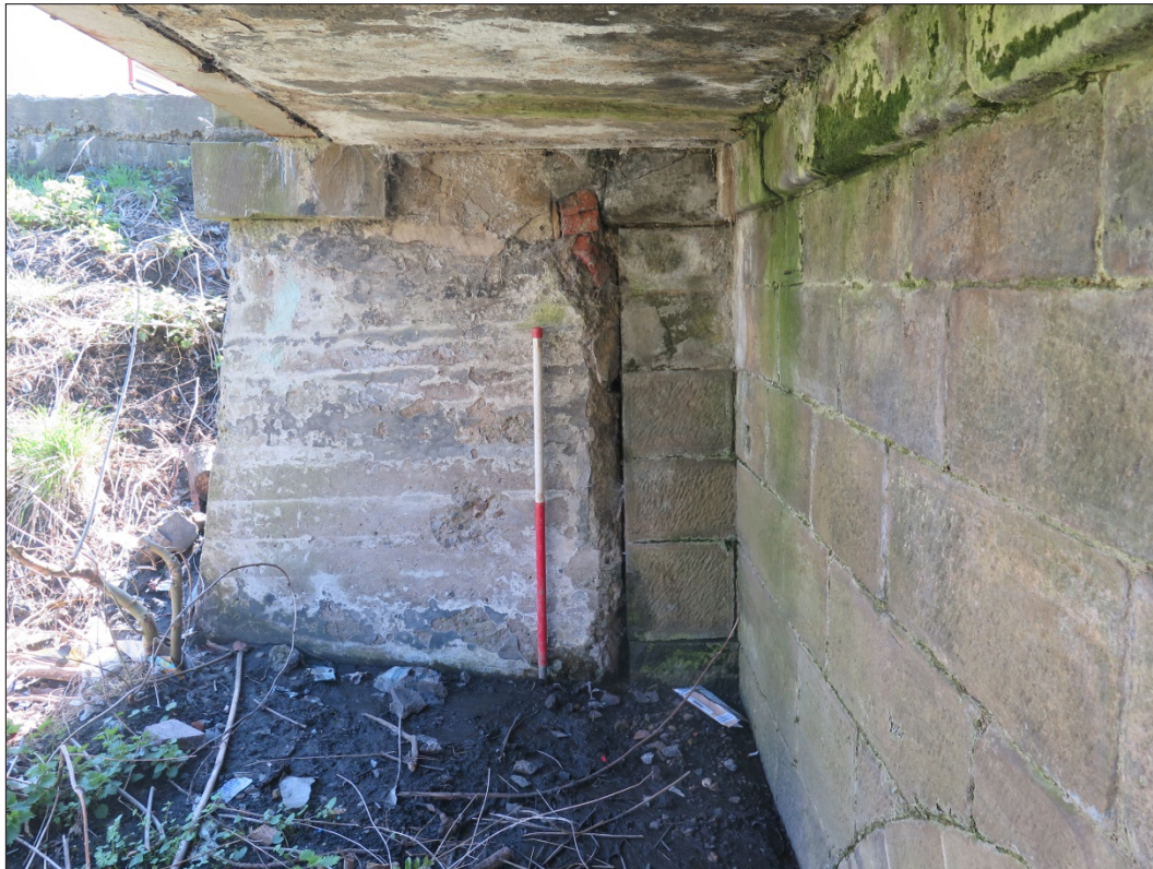
Figure 28: North-eastern elevation, detail of pier 1 showing original stone pier and concrete addition, looking south-east
