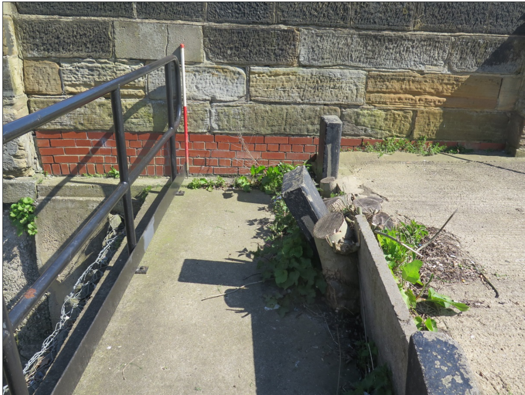
Figure 16: South-western elevation, detail of modern brick repair below parapet between piers 2 and 3, looking north-east
