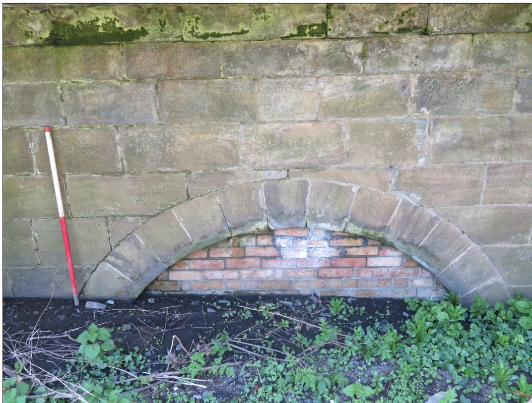
Figure 27: North-eastern elevation, detail of infilled flood channel between piers 1 and 2, looking south-west
