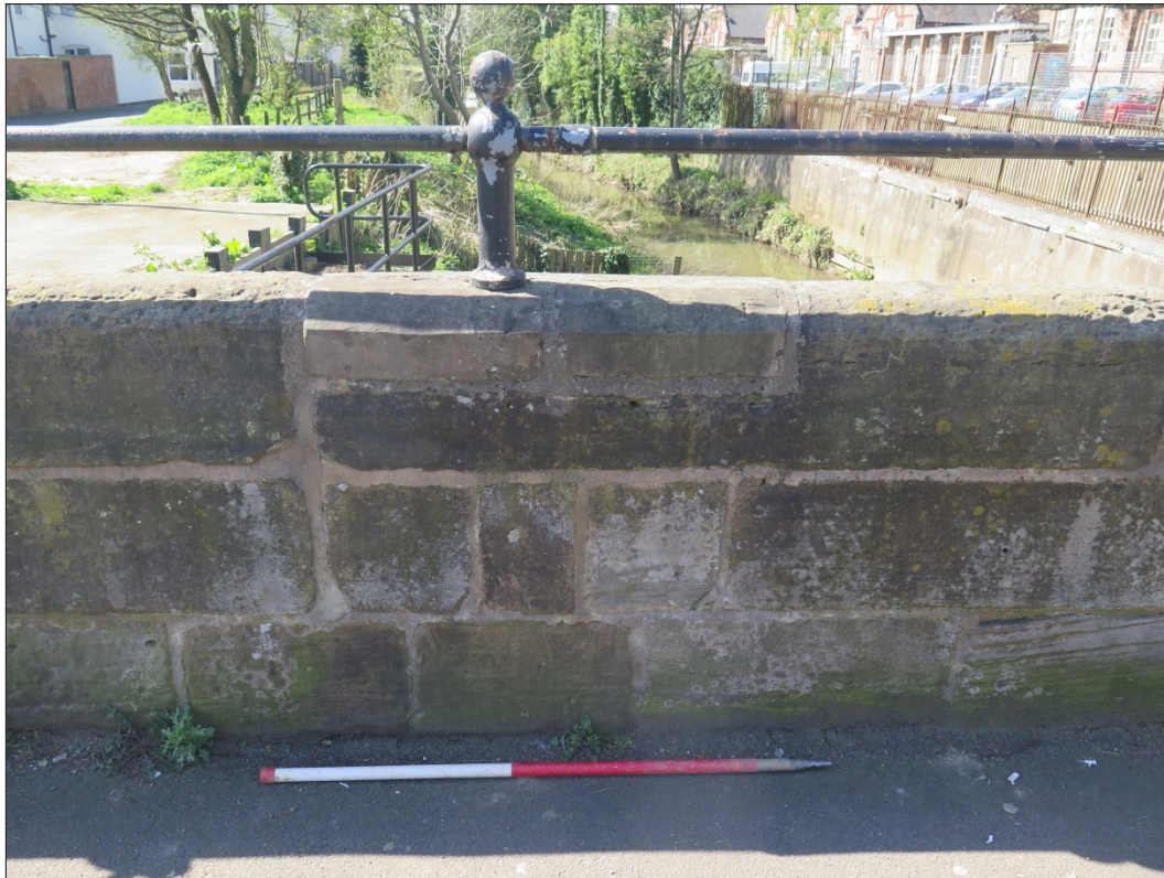
Figure 18: Internal view of the south-west parapet showing finials and a handrail, looking south-west
