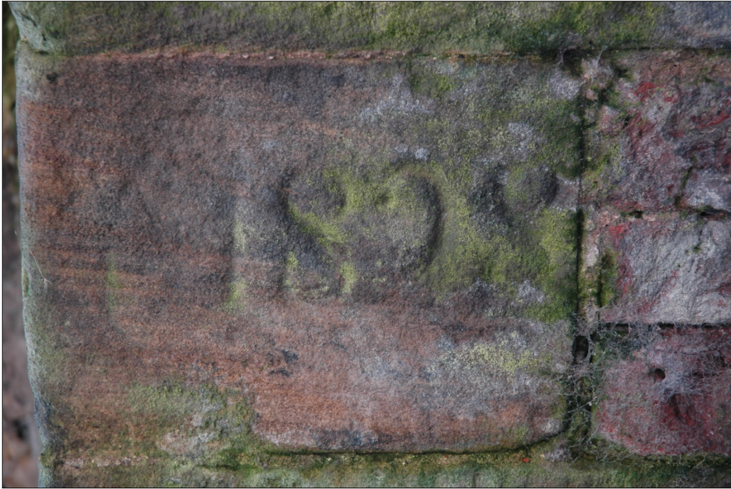
Figure 36: Detail of the keystone in the north-eastern arch of the main channel
