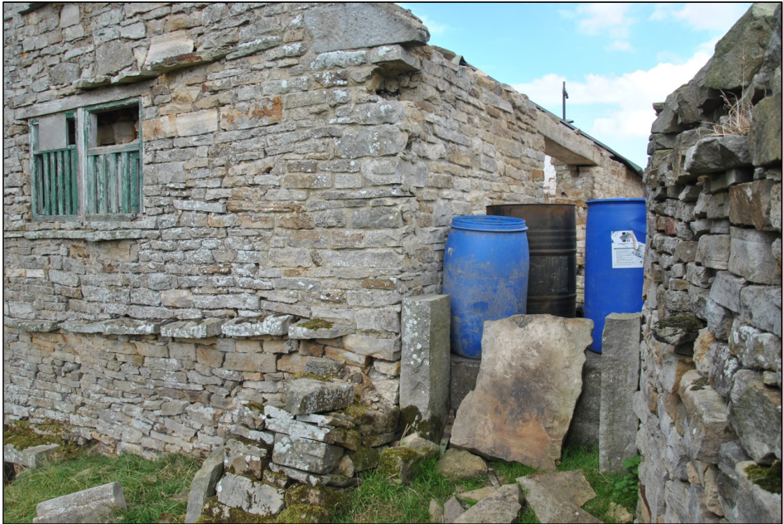
Photograph 11: The south corner of the building. This is another area of recent rebuilding. Note the cut-down gateposts at the right, beside the former fuel store
