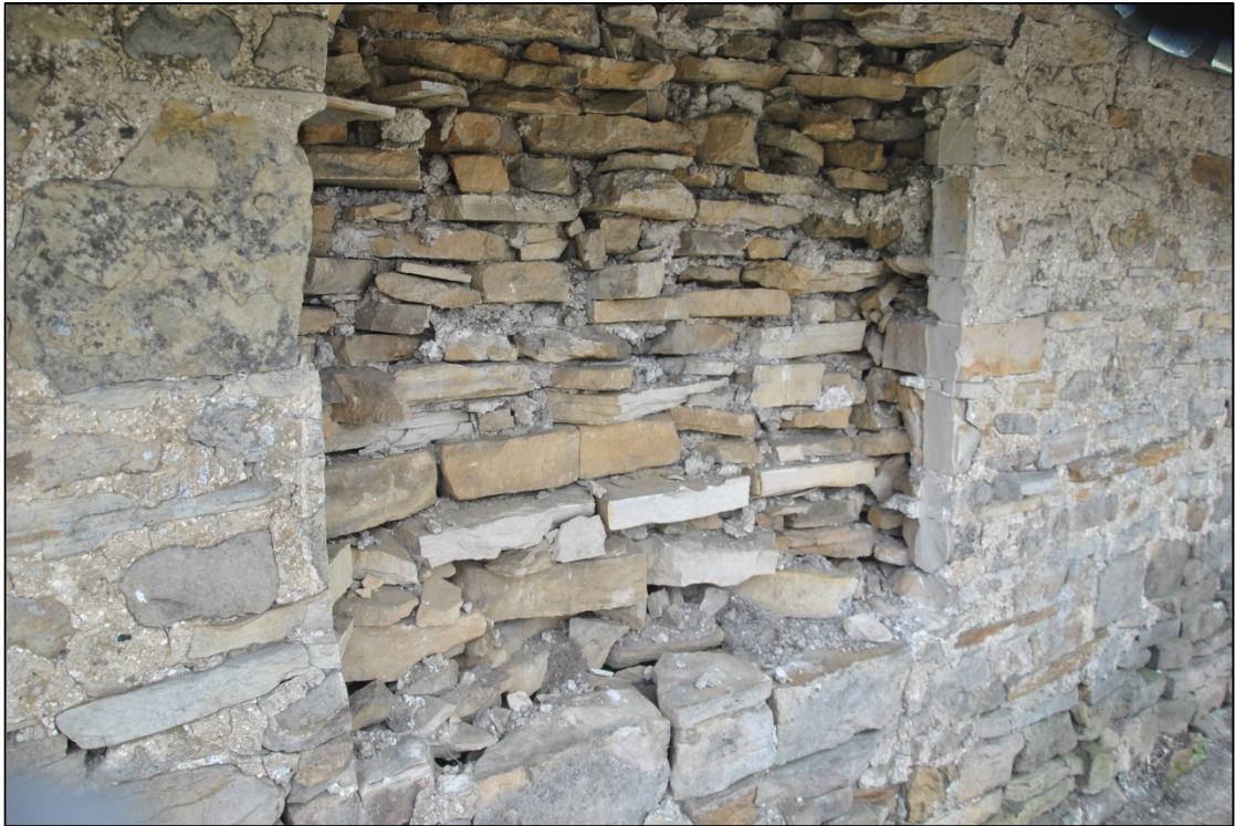
Photograph 21: The incomplete modern window opening at the north end of the north-west face
