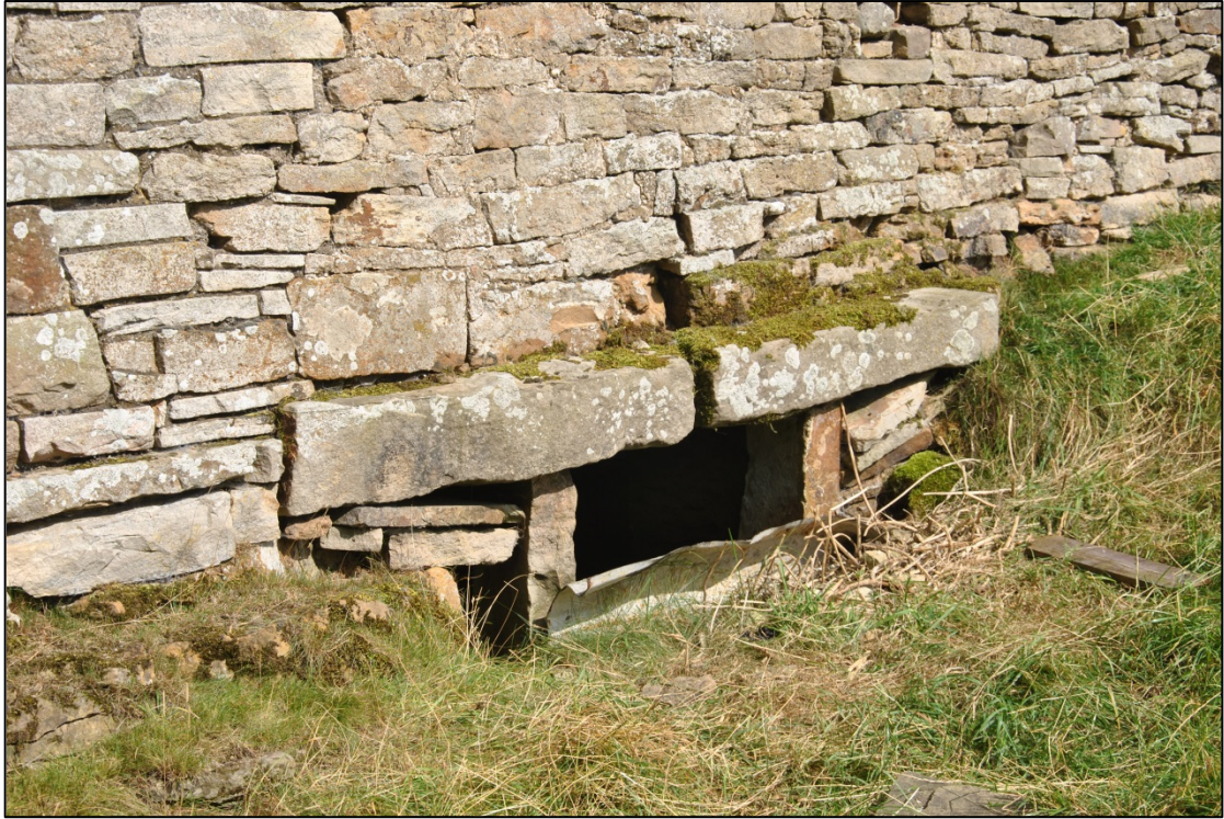
Photograph 15: The opening to the under-floor room, at the foot of the south-west wall
