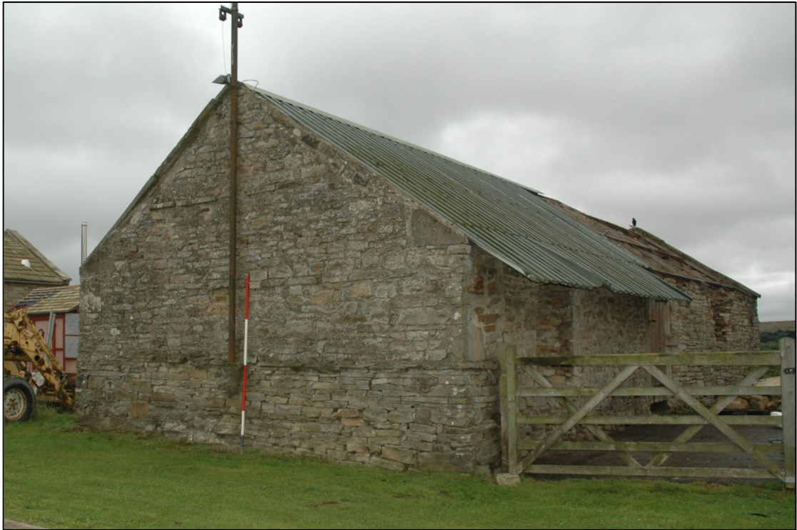
Photograph 5: The north-east end of the building with the attached electricity supply pole. Note the additional course of stones on each slope of the gable
