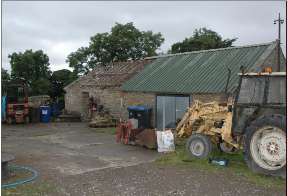
Photograph 3: The yard and the south-east face of the building. Stubs of steel posts for the enclosures can be seen in places in the concrete yard
