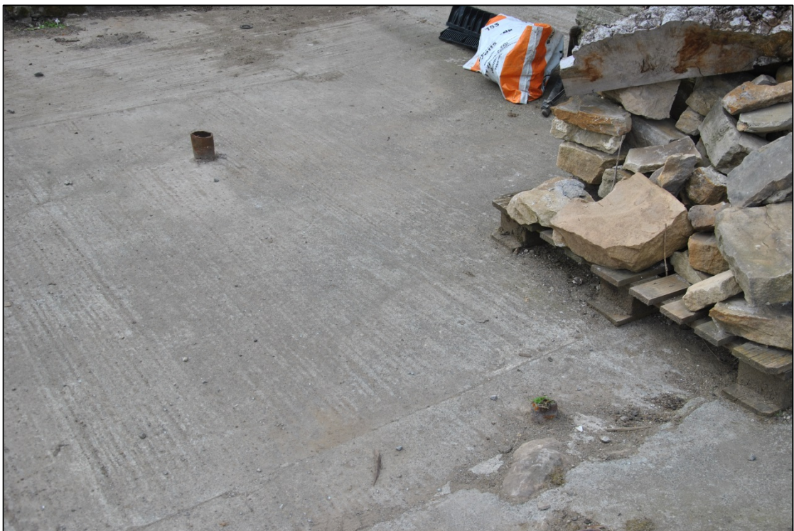
Photograph 4: Detail of two of the cut-off steel fence posts seen near the far door in the picture above
