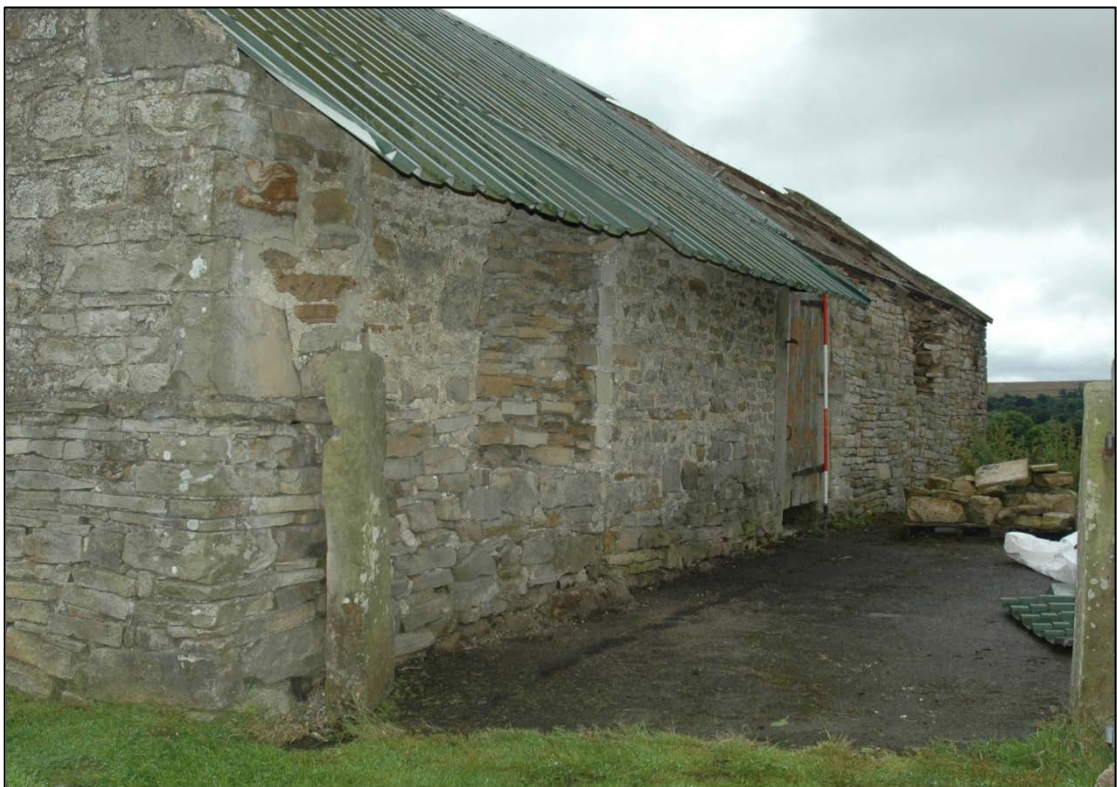
Photograph 18: The north-west face. Note the central door beside the scale and the recent window in the foreground
