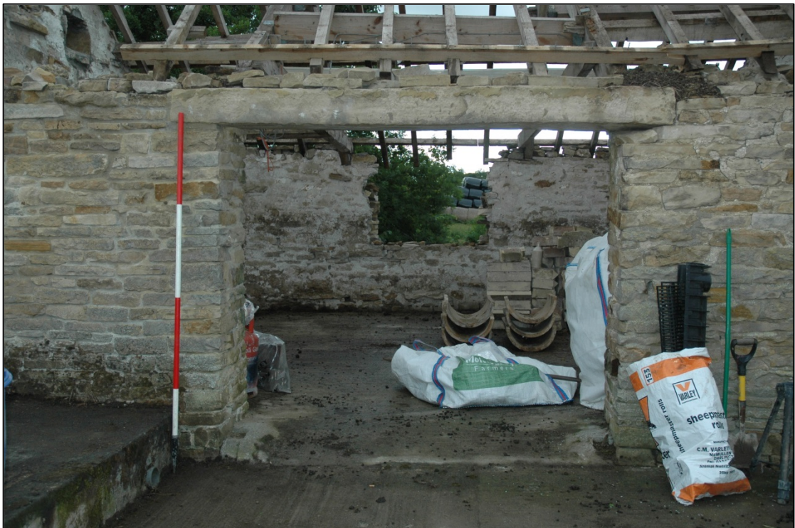
Photograph 8: The south door in the south-east wall. The masonry to the left of the door has been rebuilt relatively recently
