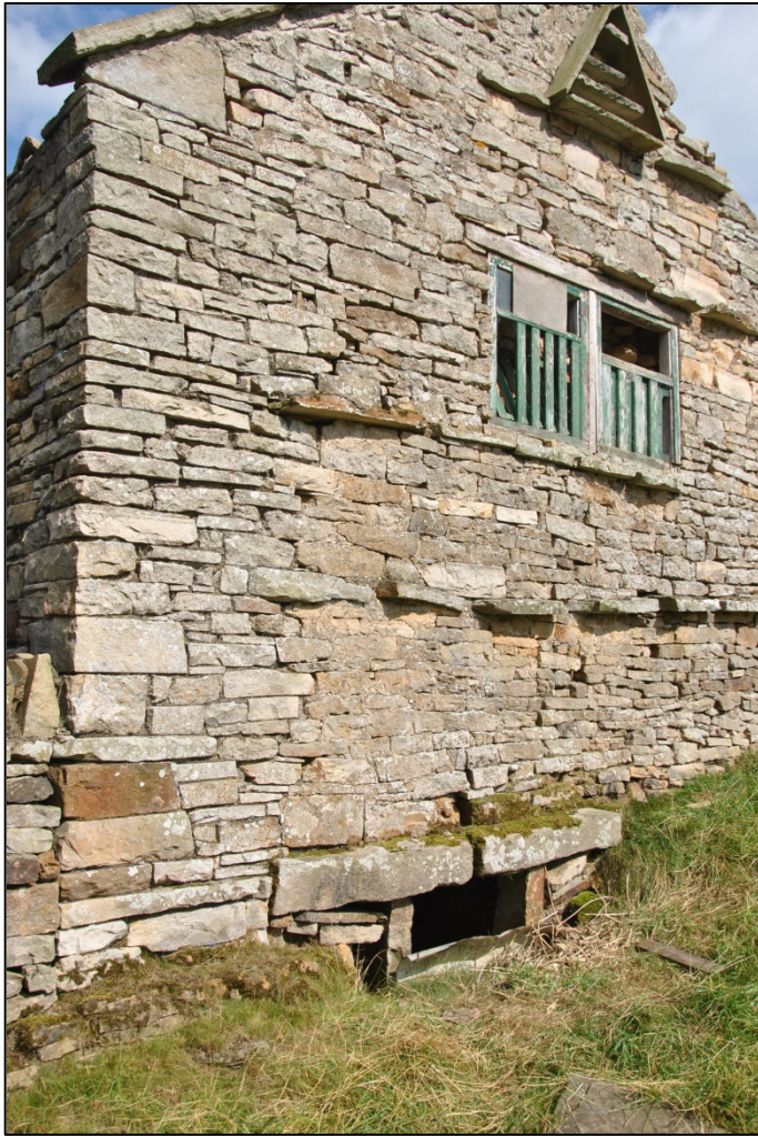
Photograph 13 (left): Detail of the south-west end, showing the courses of through stones, the pigeon holes above the recent window, and a large area of rebuilt masonry at the left-hand corner
