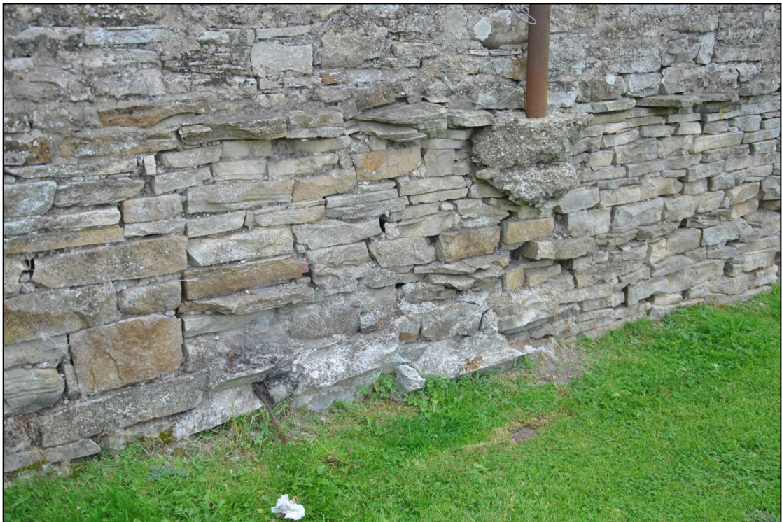
Photograph 6: Detail of the foot of the north-east wall. Note the concrete at ground level and around the bottom of the timber pole
