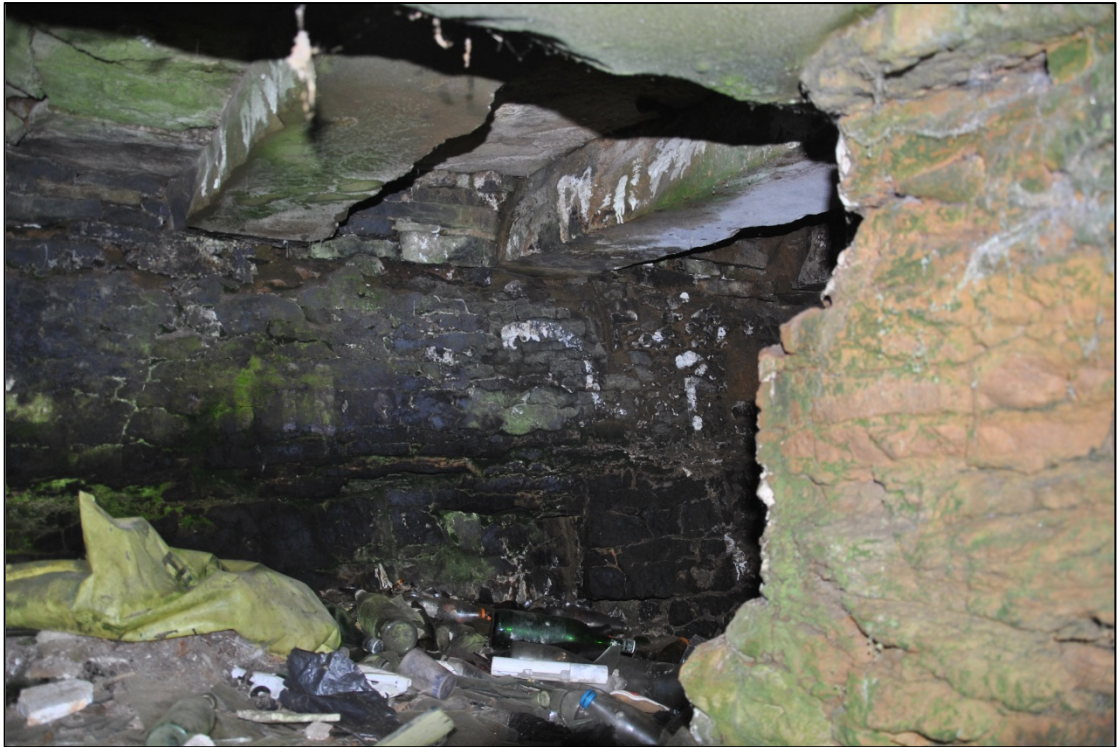
Photograph 17: Looking around the corner from the entrance of the under-floor room. Note the heavy stone lintels in the ceiling
