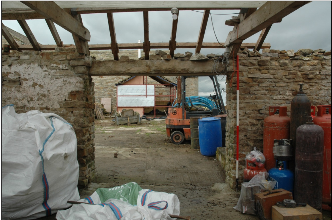
Photograph 23: The door of the south room. The rebuilt wall at the right has been slightly thickened at its head to support the roof truss.
