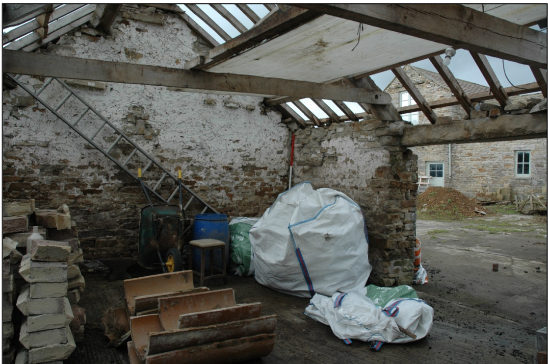
Photograph 22: Looking east in the south room. The half-pipes in the foreground formed a feeding trough against the far wall
