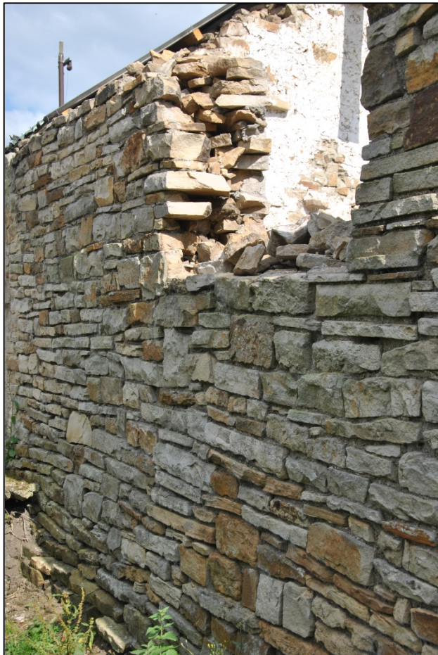
Photograph 20: The north-west face. A detail of the re-faced wall and the ragged window opening south of the door
