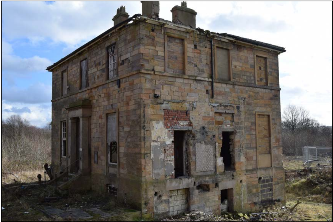
Photograph 7: The house from the north-west, showing the paved area at the front
