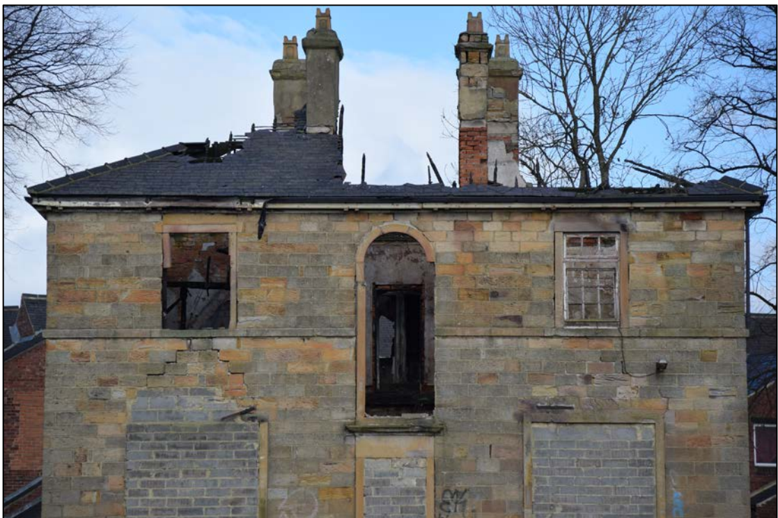
Photograph 4: The upper floor and the stair window on the south face. Paired timber gutter brackets can just be seen. Note the settlement cracks between the left-hand windows
