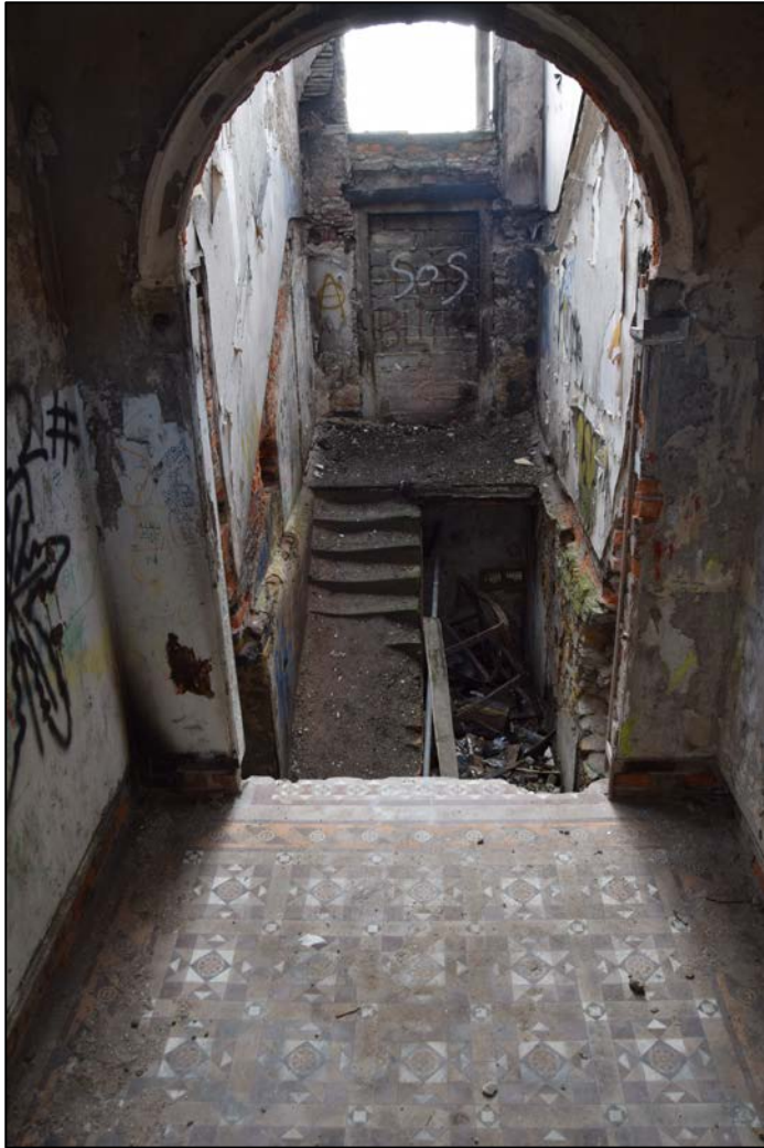
Photograph 9 (left): The staircase hall seen from the fanlight of the north door. The worn stone steps rise from the service quarters in the basement. Marks in the plaster of the side walls show the position of the lost stone staircase mentioned in the listing description. Note the remaining decoration of the arch from the lobby
