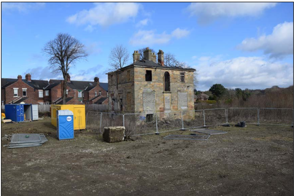
Photograph 2: The house from the south-west. The ground level seen here is well above the former garden, which was below the lowest point visible on the south wall of the building.
