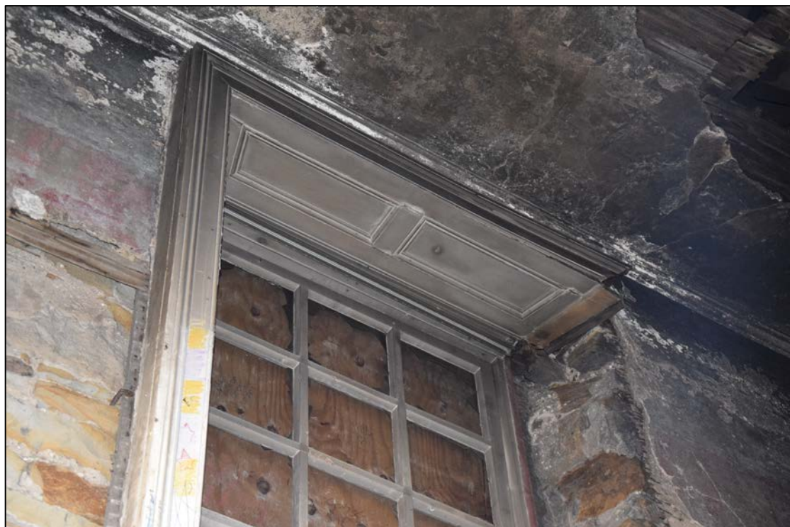
Photograph 18 (below): The surviving woodwork of a window in the north-west room on the ground floor
