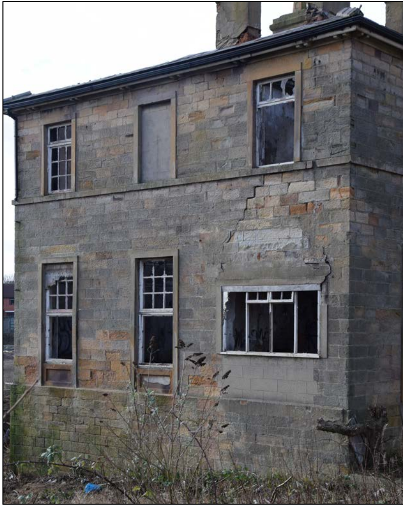
Photograph 5 (left): The east face, showing the large alteration to the ground-floor window at the north-east corner
