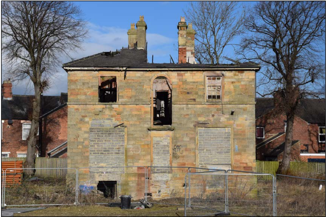
Photograph 3: The south or garden front. Note the wide ground-floor windows and the scar of the steps below the central door
