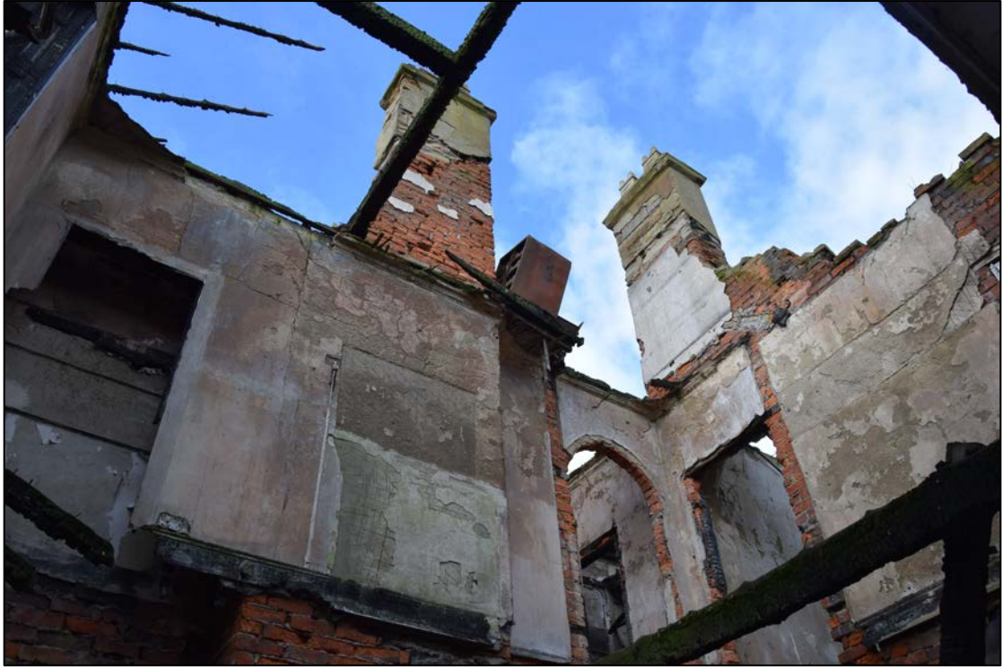
Photograph 21: The south-east room on the first floor. The mark of the partition wall can be seen at the left of the arched brick doorway on the former landing
