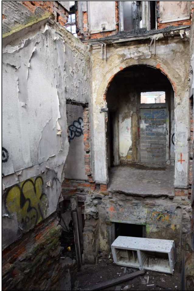
Photograph 17 (left): The staircase hall seen from the south-east. The service rooms in the basement are choked with rubbish and debris
