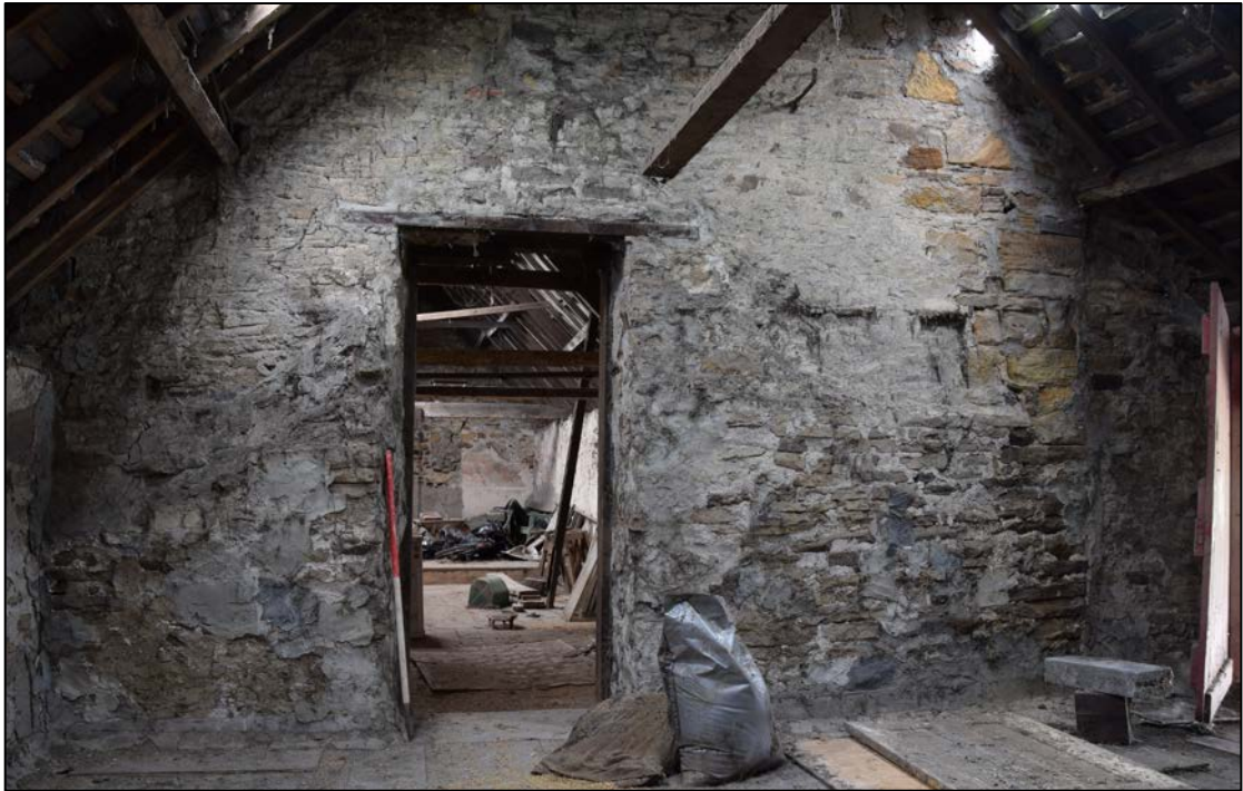
Photograph 49: The west end of the granary. The outline of the gable of an older and lower building can be seen at either side of the door. At the right-hand side, a straight joint shows where the present building was widened
