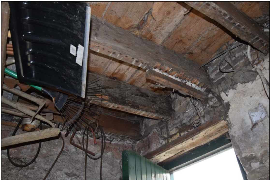
Photograph 20: The marks of a lath and plaster ceiling on the joists just inside the door
