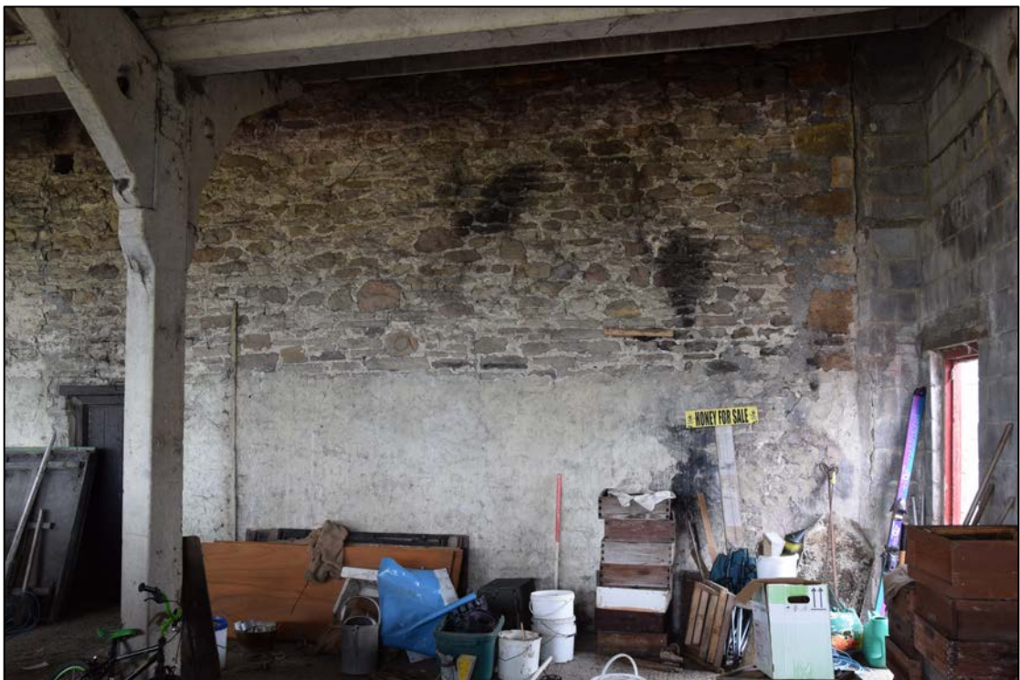
Photograph 12: North face of the old house; the west end. Old angle quoins abut the concrete block wall at the right-hand side. The soot marks are the relic of a fire in the yard, not evidence of flues
