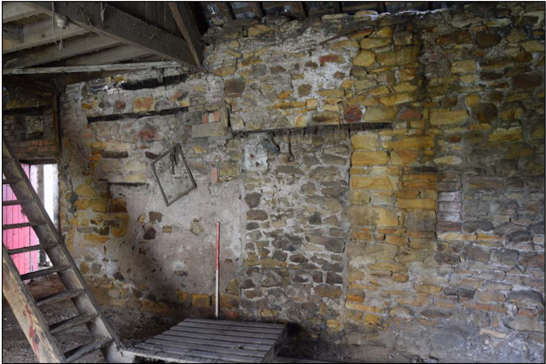
Photograph 61: The blocked east door is at the centre of this view, with the shaft holes above and to the left. A vertical line of bricks just to the right of the band of yellow stones block a breather slit
