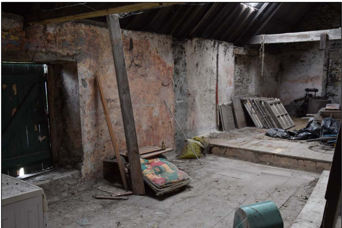
Photograph 28: The south wall, showing the loading door, the grey scar of the internal wall and the change in floor level just beyond the old division
