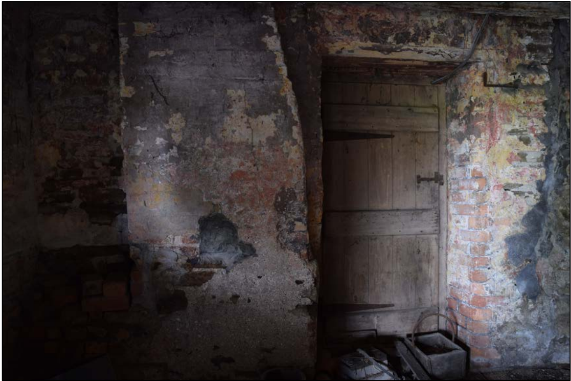
Photograph 43: The brick and stone chimney and the door inside the brick building shown in Photo 42. This is the east end of the old house and the west end of the cart shed
