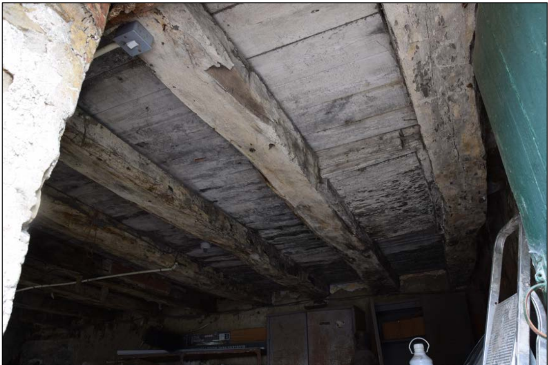
Photograph 26: Detail of the old joists, seen from the doorway at the east end of the room
