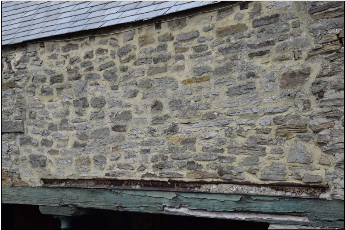
Photograph 37: Detail of the blocked opening at the east end of the granary. The masonry rests on a length of railway line
