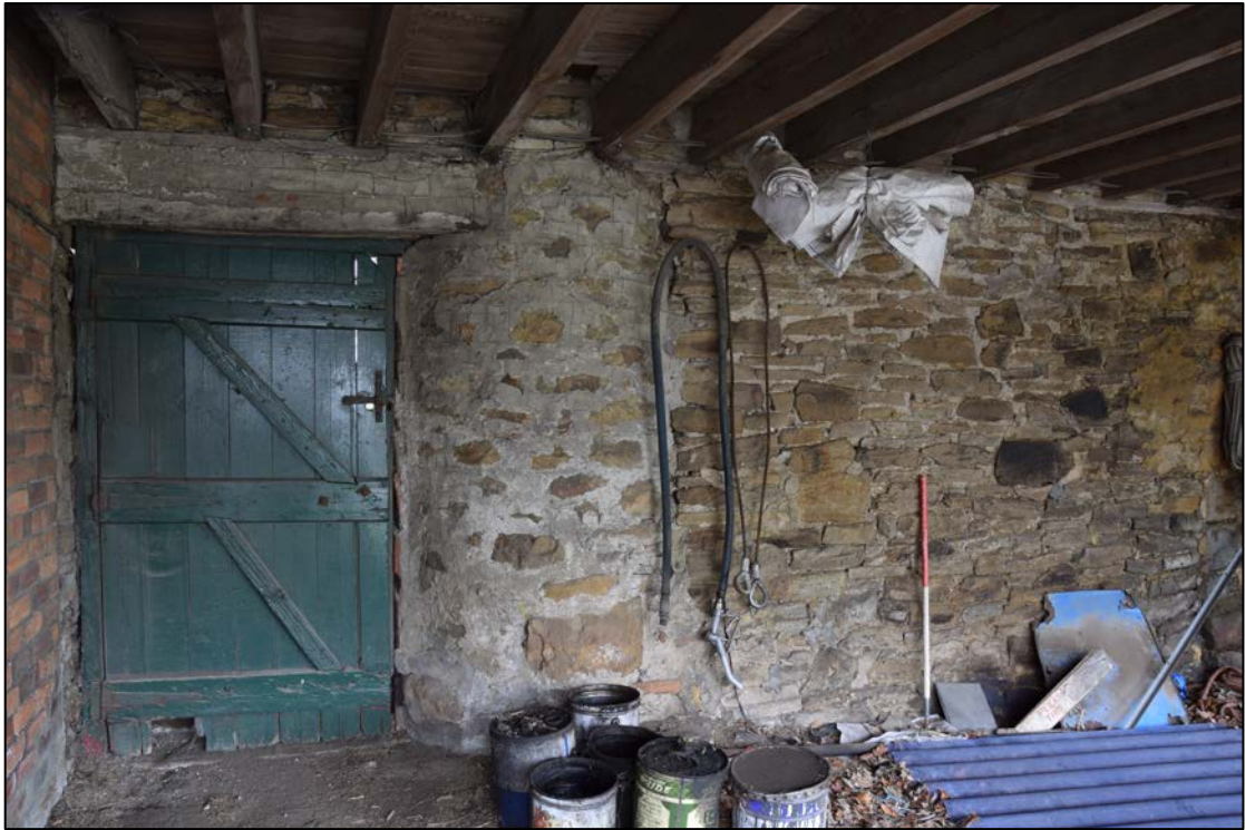
Photograph 45: Detail of the north wall. The stonework in the curved face of the gin-gang pier beside the door is different from the later wall to its right. The straight joint at the corner of building C is just visible at the right-hand side of this picture
