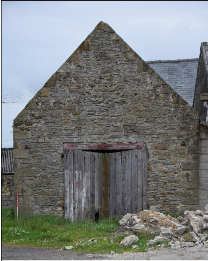
Photograph 55 (left): The north end of the barn, with a blocked loading door above the lintel
