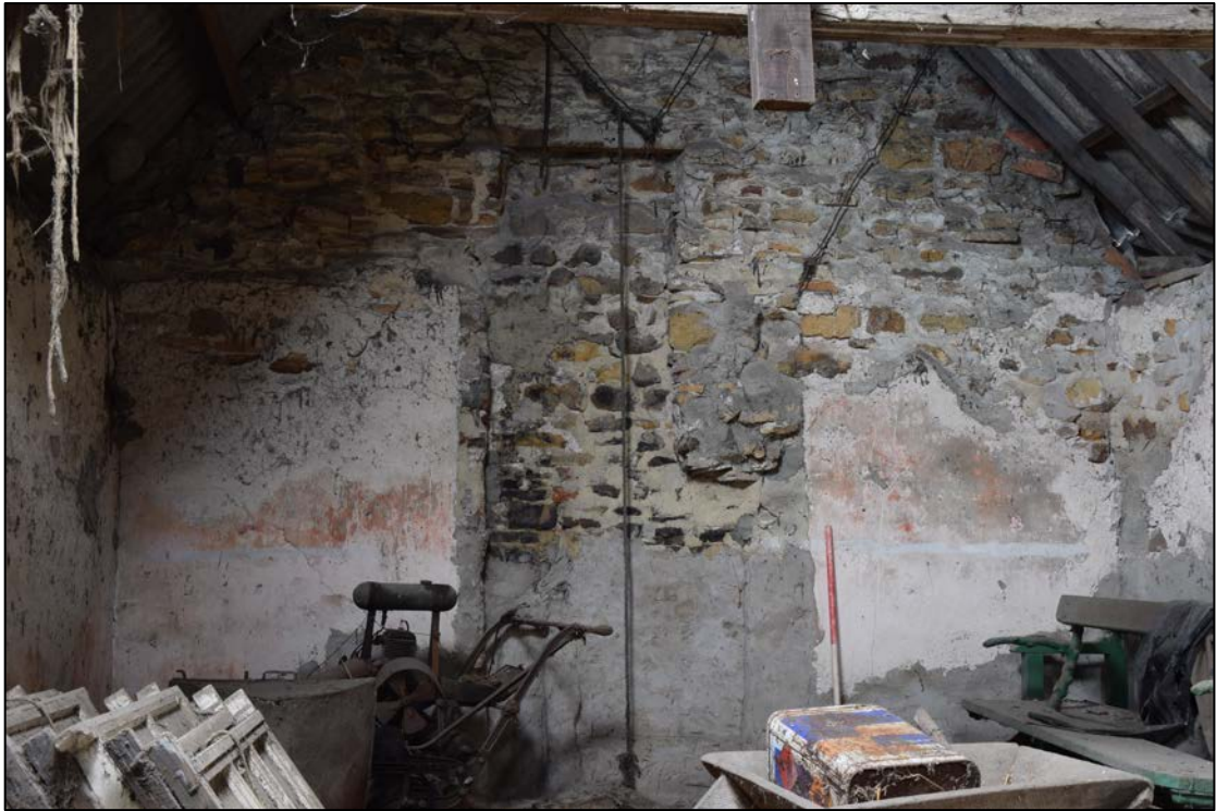
Photograph 31: The marks of the demolished chimney breast at the west end of the first floor
