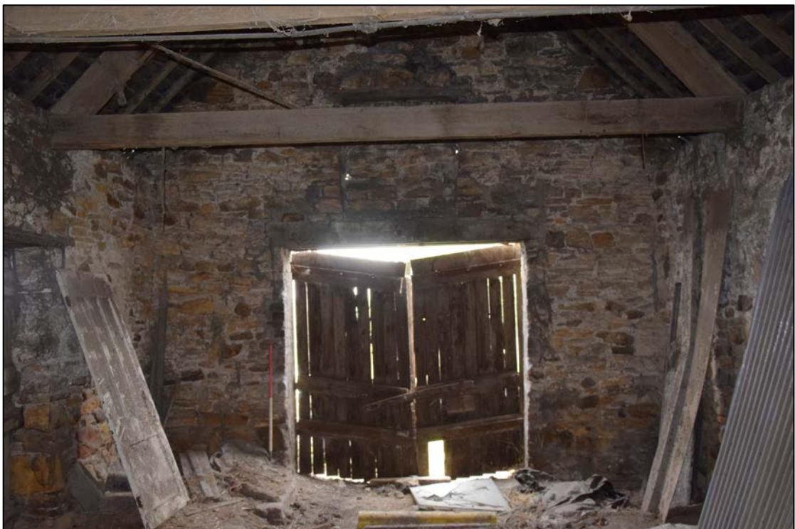
Photograph 62: The north end of the barn, with the blocked opening above the doors
