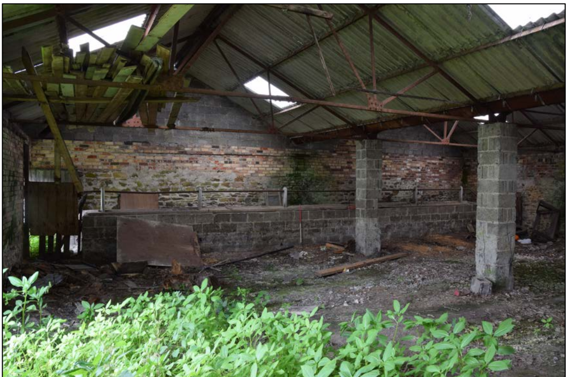
Photograph 68: Looking south-east inside the old hemmel. The old stone wall has been raised with brick and blockwork. A concrete trough runs the length of the east wall here
