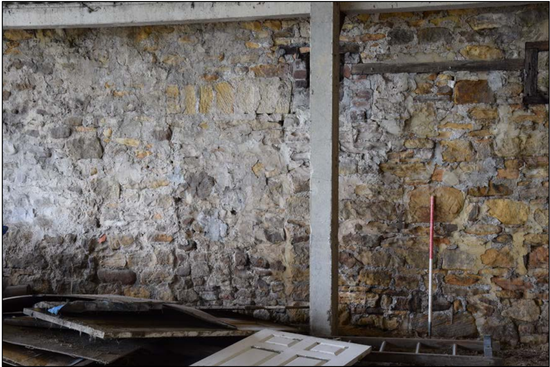
Photograph 57: The blocked door at the middle of the wall shown above can be seen just left of the concrete column. The horizontal timber links two of three holes in the upper part of the wall here
