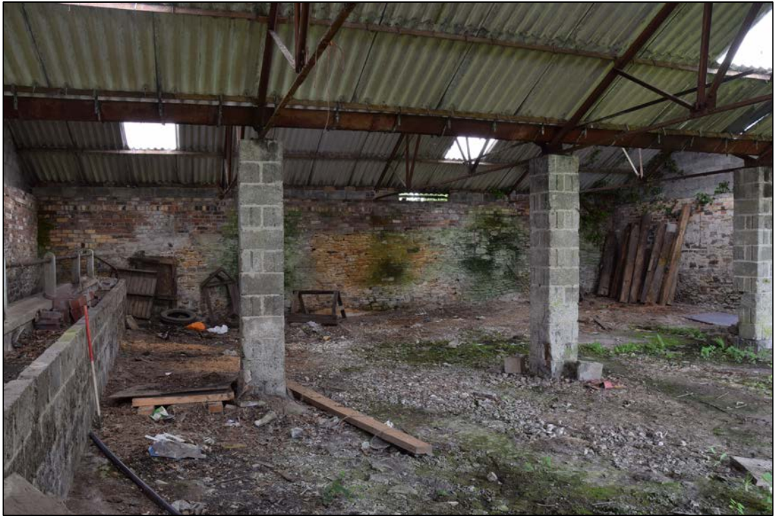
Photograph 69: The south side of the old hemmel. The blockwork piers have steel columns inside them
