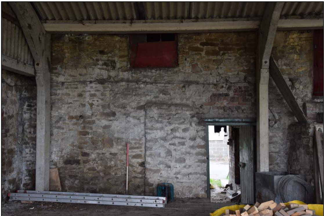
Photograph 40: The centre of the north wall. The projecting masonry between the scale and the door is the inside face of a gin-gang pier
