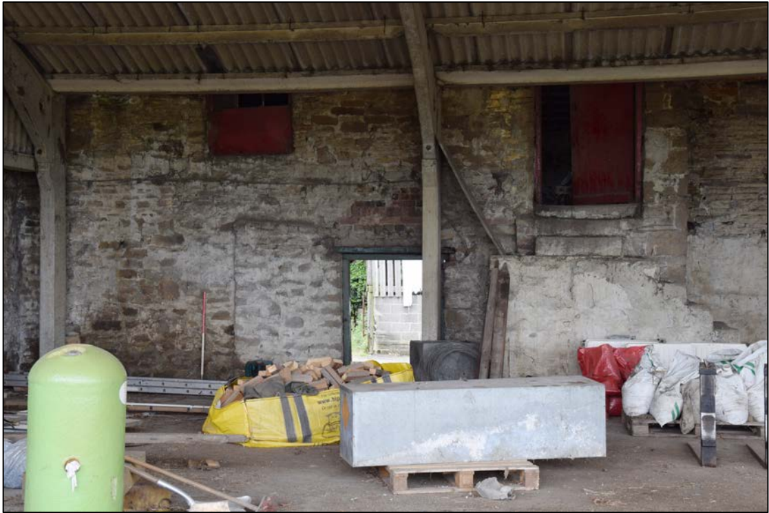
Photograph 41: The north wall of building B, showing the stone stairs seen in Photo 39, the two doors and the window to the granary
