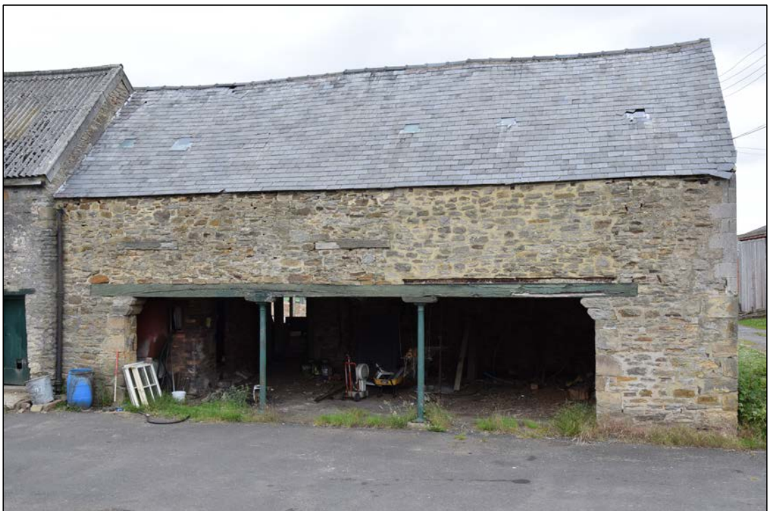
Photograph 36: The south face of the cart shed / granary, building B. Note the sills of blocked windows, left and centre, which project slightly from the wall face. A matching window at the right has been replaced by a larger blocked opening
