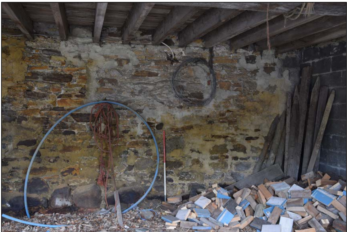
Photograph 46: The south end of building C, inside the cart shed. Note the large rough stones of the footing course
