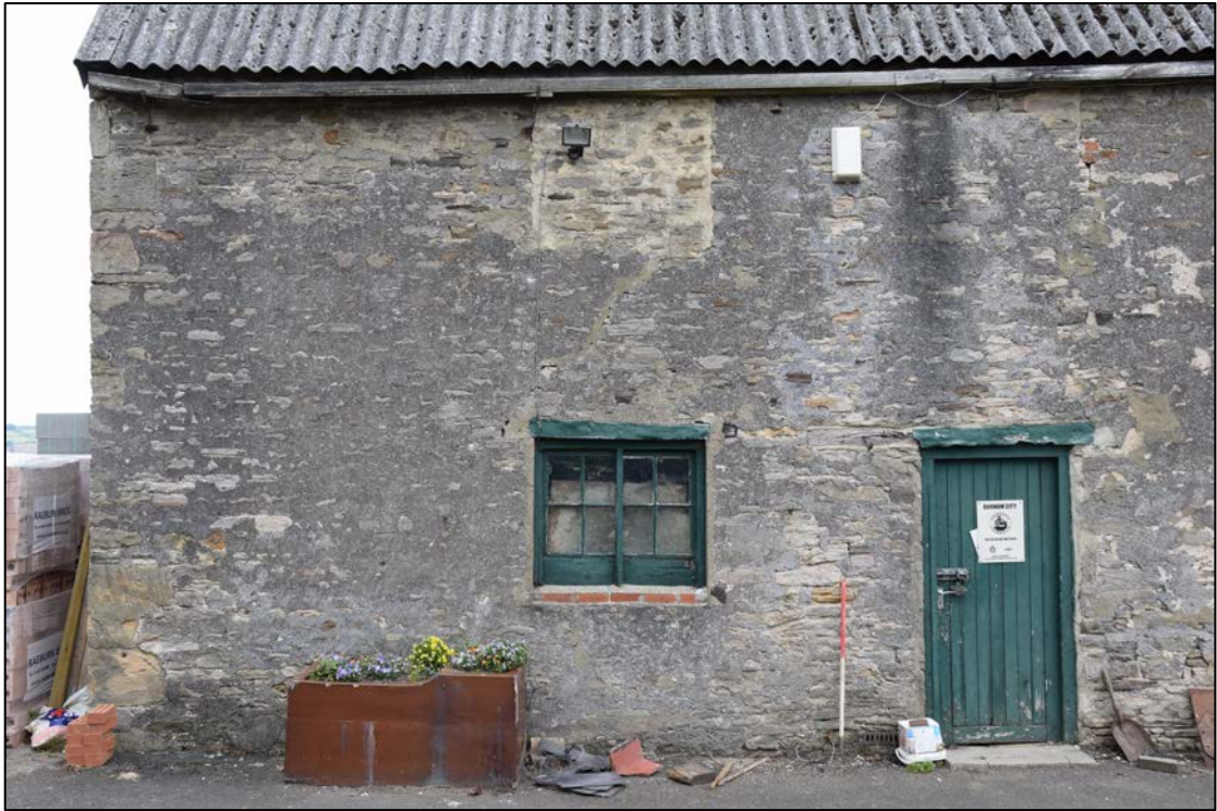
Photograph 7: South face of the old house; the west end. Although much of the masonry is concealed by mortar, the thinness of the courses can be made out. Note the straight joint, top left, and how the door lintel extends well past the left-hand jamb of the door
