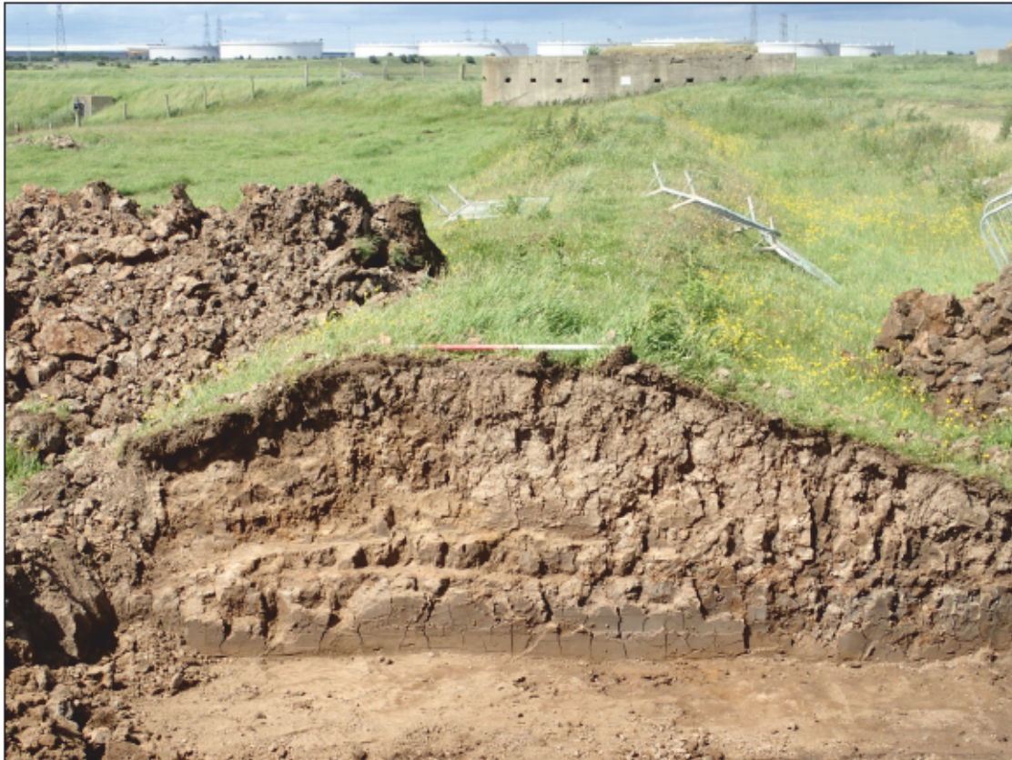
Photograph 7: The old sea wall, looking north, with the WWII section post in the distance
