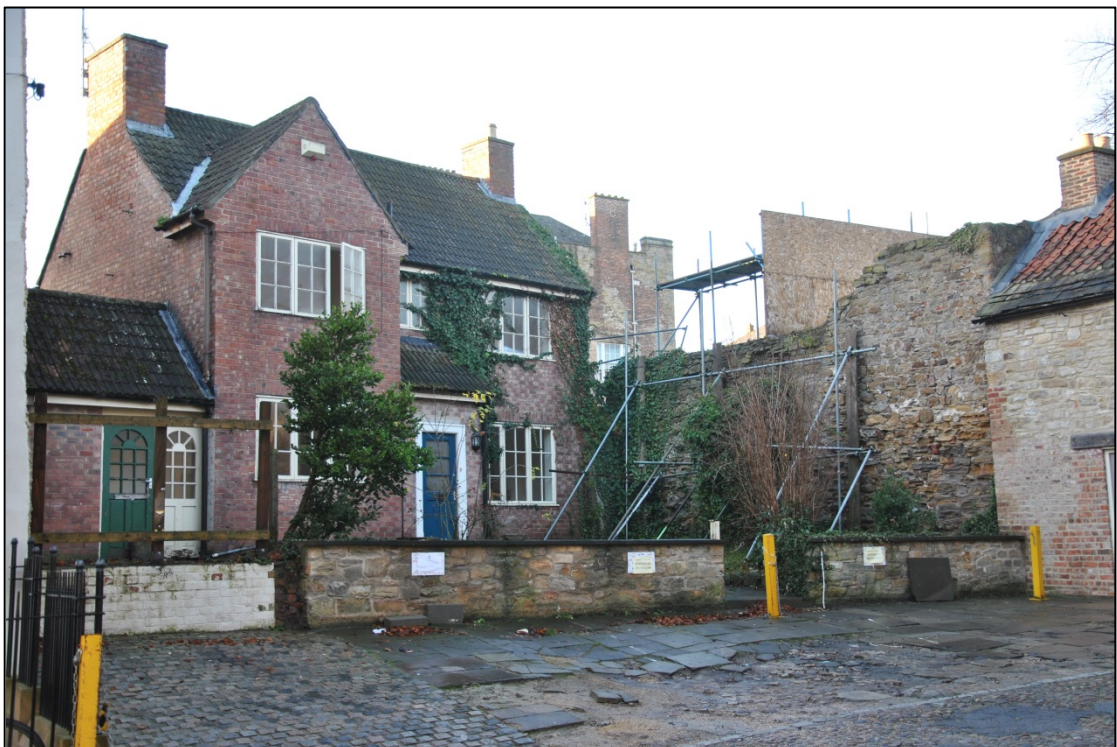
Photograph 2: A view from the south-east, showing the old retaining wall / gable end of the earlier rectory supported by scaffolding
