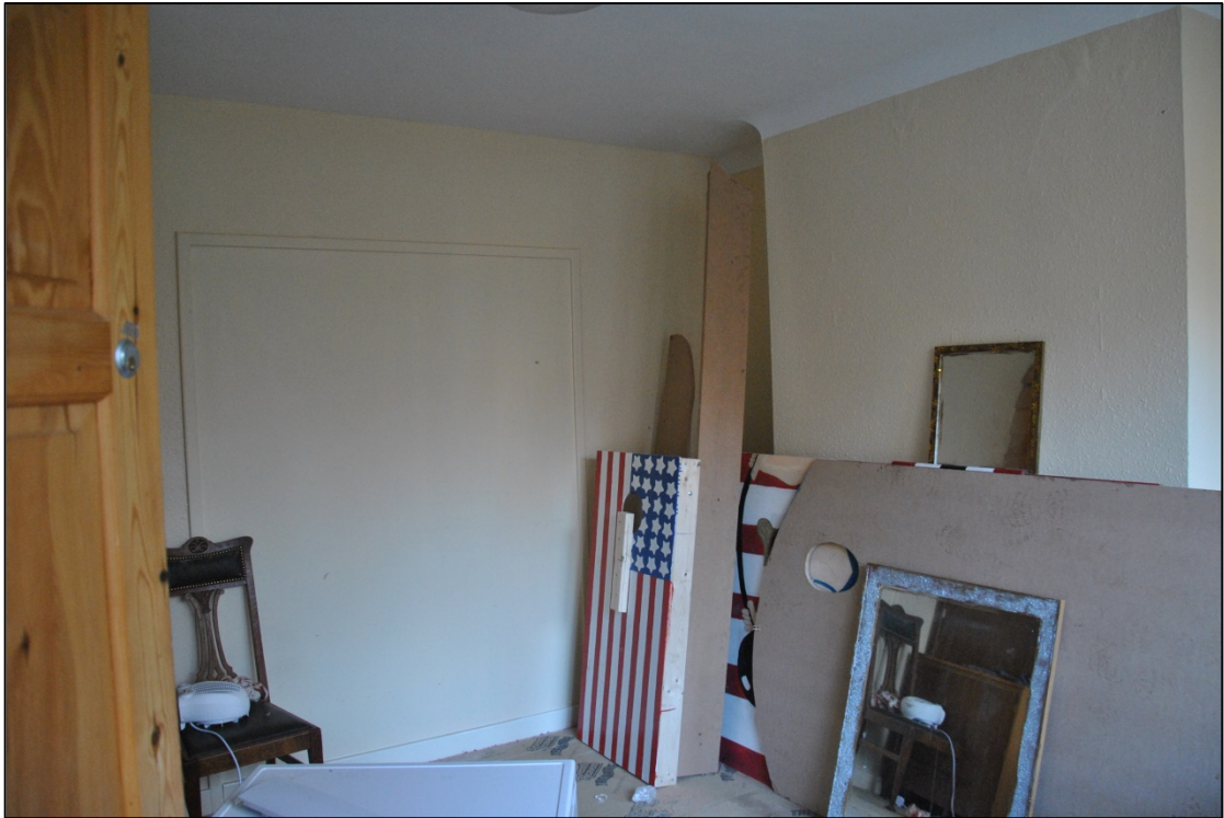
Photograph 11: The north-eastern reception room 6. The far wall is a recent insertion that reduces the size of the room
