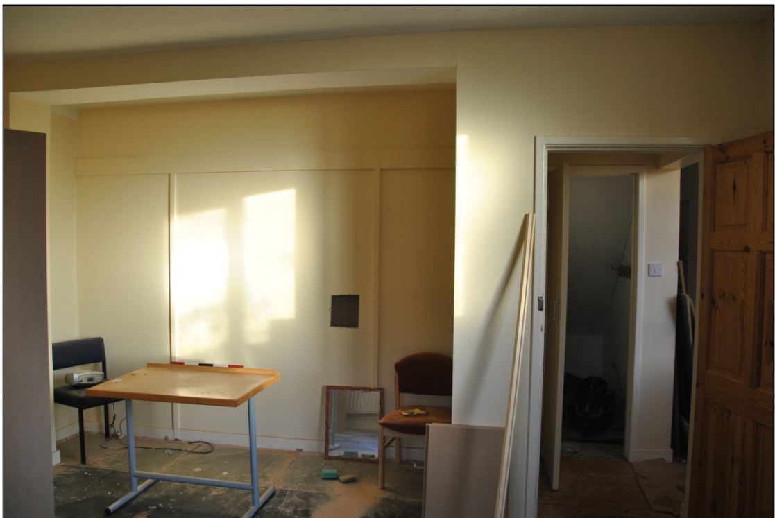
Photograph 12: The same inserted wall, seen from the south-west in the common room 7. The door at the right looks into the hall and the under-stair cupboard
