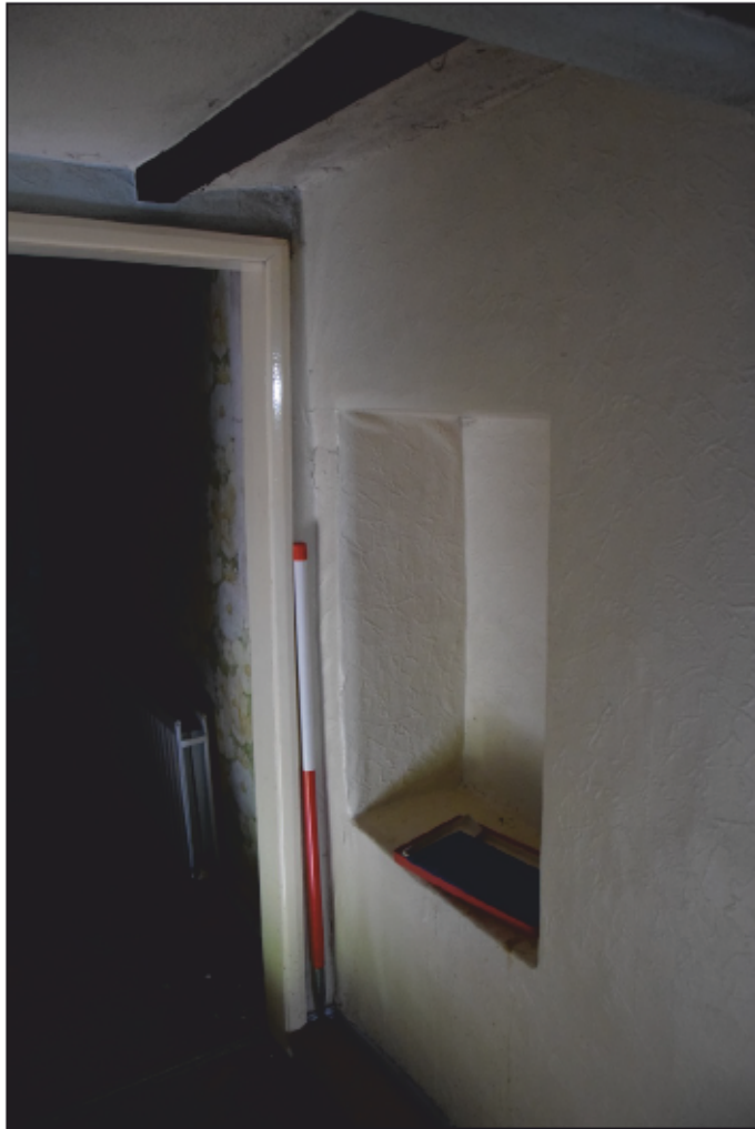
Photograph 33 (left): A blocked widow at the head of the staircase
