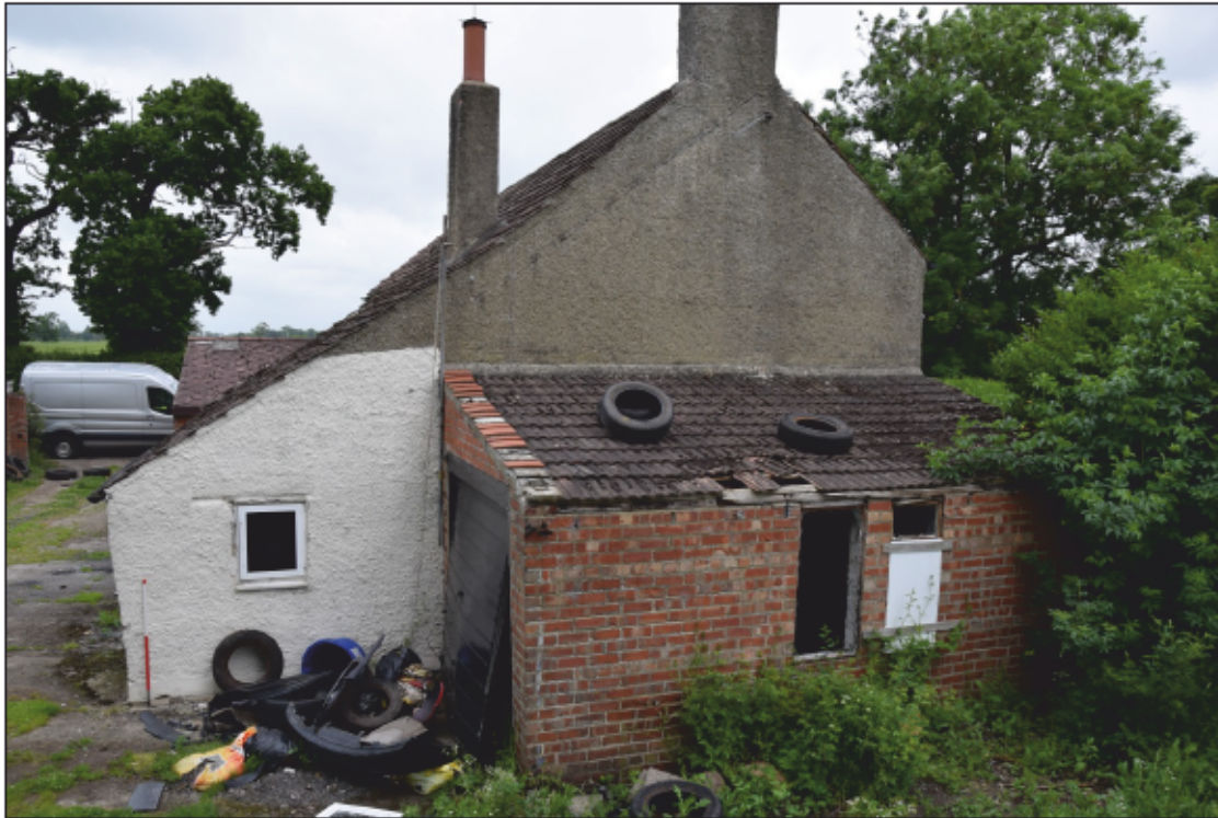
Photograph 11: The south-west end and the brick garage. What appears to be an old roof line is the mark of a later fixture on the gable
