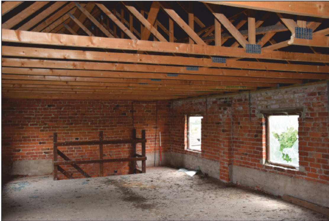
Photograph 59: The first floor seen from the north-west corner. Note the strip of cement render around the lower walls
