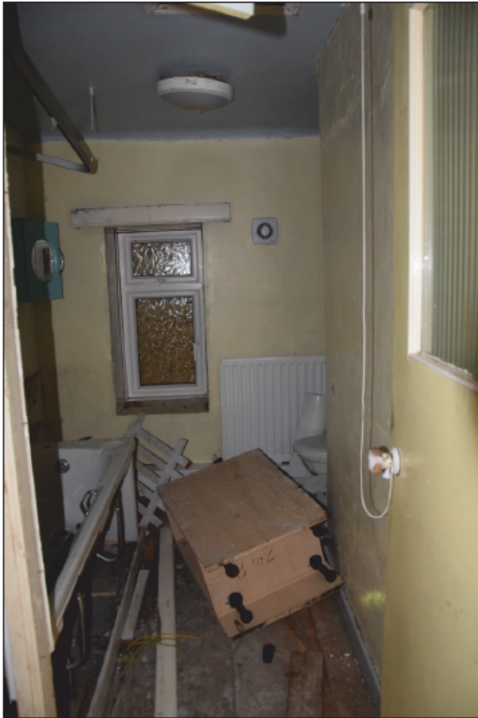
Photograph 35 (left): The bathroom, damaged by thieves
