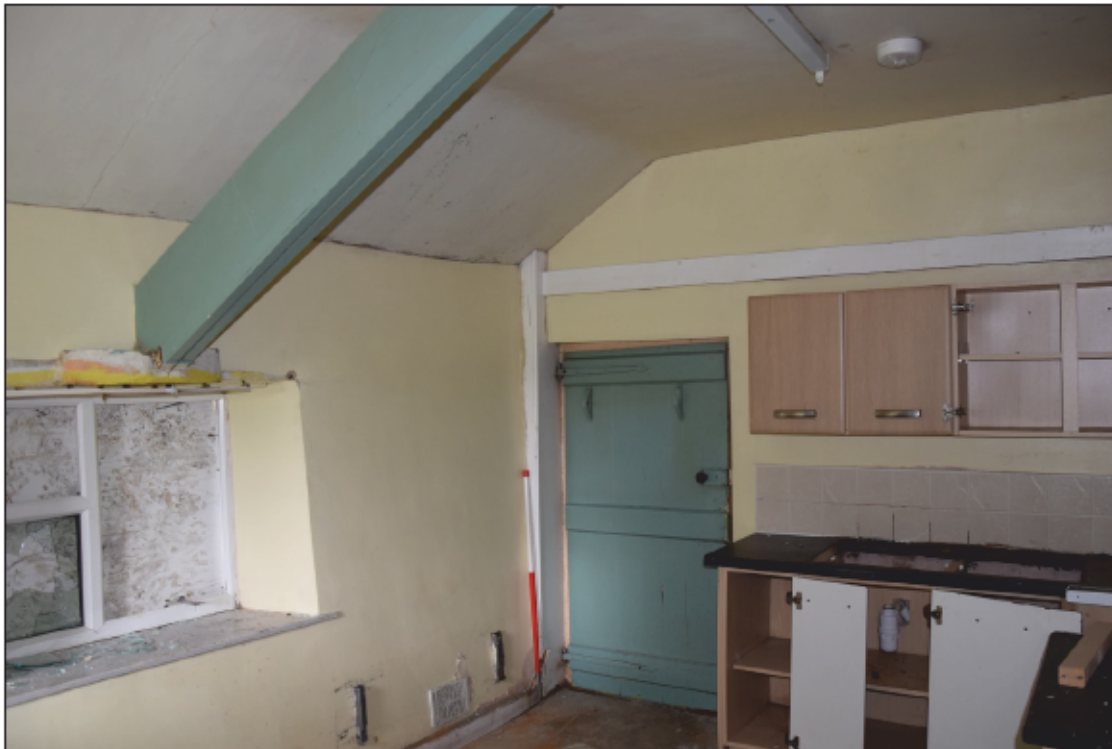
Photograph 18: The outshut kitchen, with the exposed roof truss carried on a projecting slab above the window
