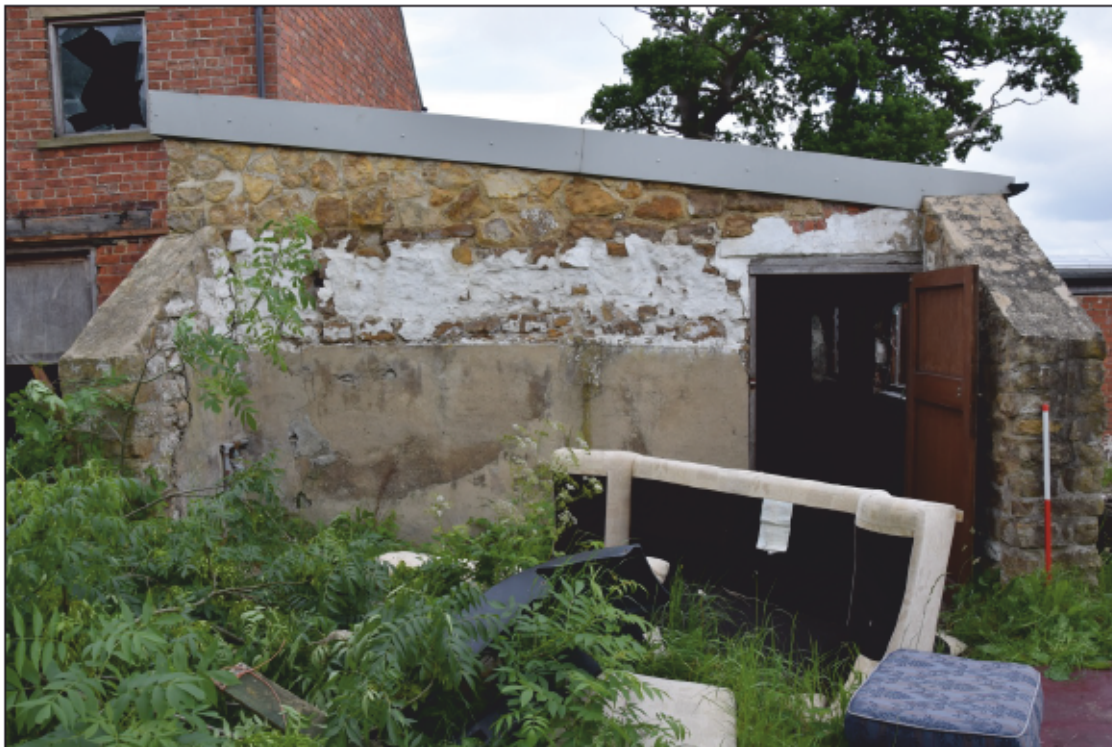
Photograph 44: The stump of the old stone building. Note the cement render beside the modern door to the byre
