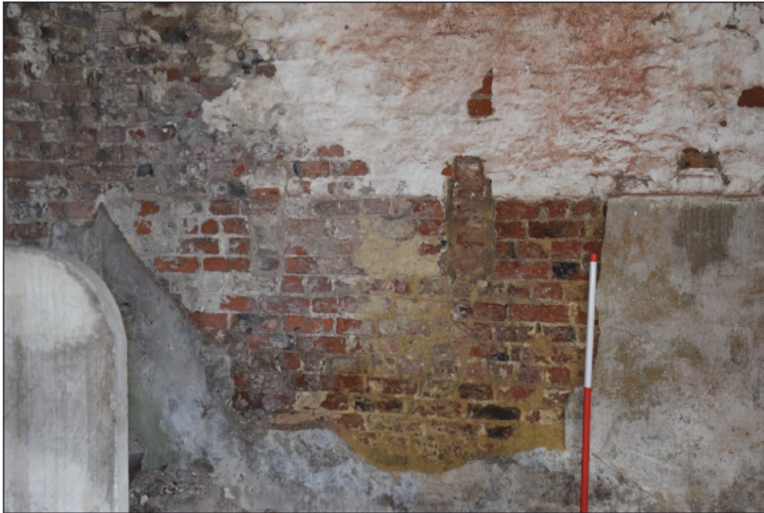
Photograph 49: Breather slits covered by 1960s cement render
