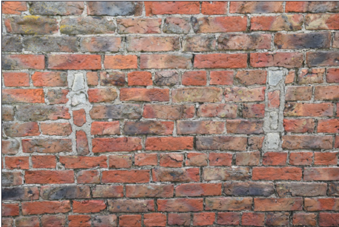
Photograph 43: Blocked breather slits in the north-east end of the brick byre
