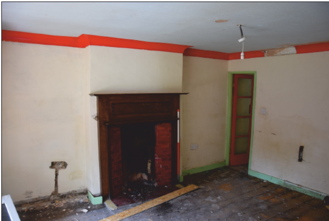
Photograph 14: The dining room, with the surviving fireplace and the narrow door to the kitchen
