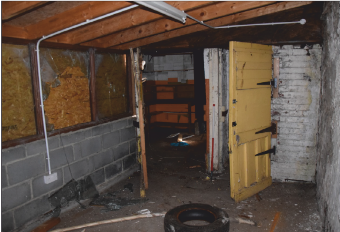
Photograph 27: Doors to the older workshop sheds seen from the later concrete structure. A view looking north
