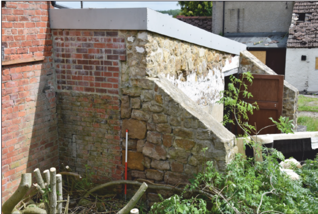
Photograph 45: The end of the stone building and the south corner of the brick byre; note the ventilator slit and the modern brickwork above
