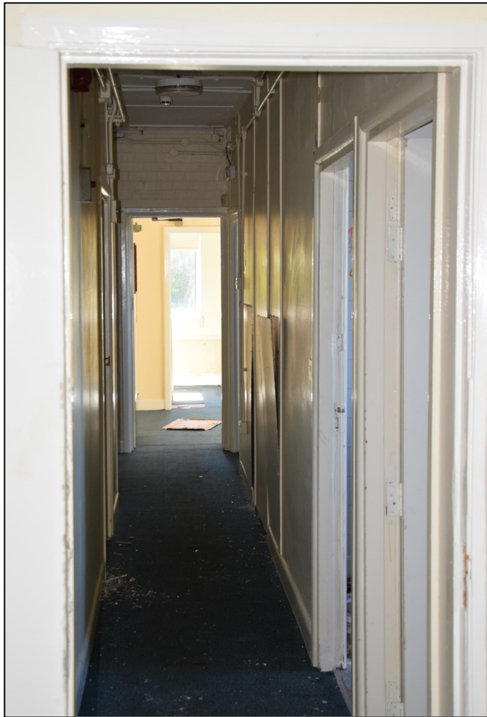
Photograph 69 (left): A typically Spartan corridor for staff and service rooms 41-46 in the 1936 extension
