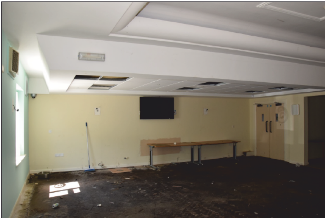
Photograph 32: The north end of the former dining room 9, latterly used as a gym
