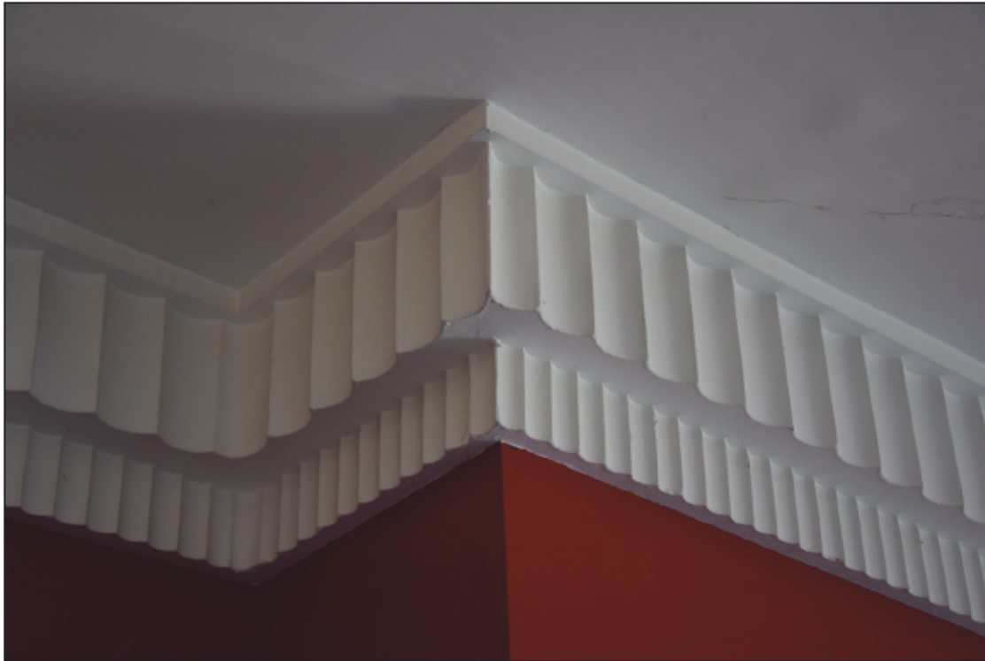
Photograph 43: Detail of the fluted concrete decoration on the chimney breast in the lounge
