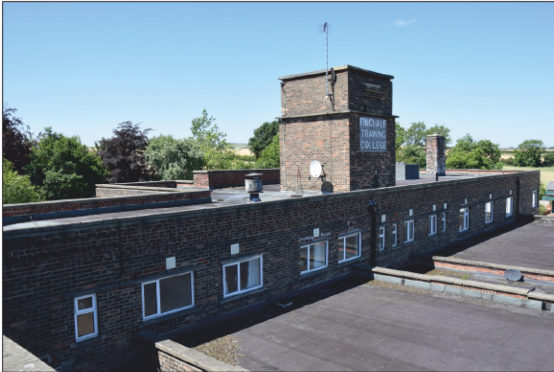
Photograph 19: Windows to the first-floor rooms 20-25 and 36-38, with the water tower and boiler flue. A view from the south-east
