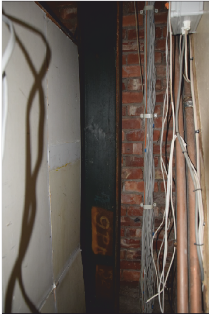
Photograph 27 (left): A steel column and bare brickwork in a cupboard near the main staircase
