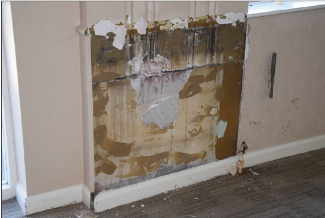
Photograph 45: The lower part of the pilaster shown above, covered up when the window sill was raised
