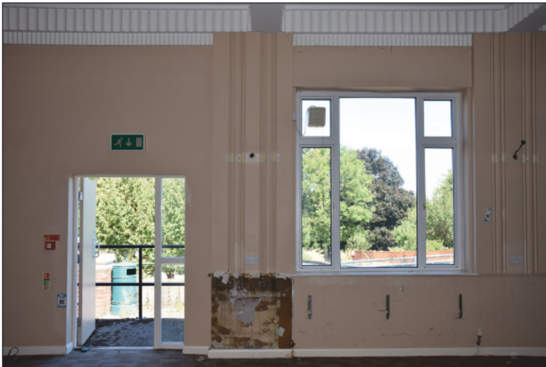
Photograph 44: A door and window between the lounge and the terrace, with decorative pilasters between the openings
