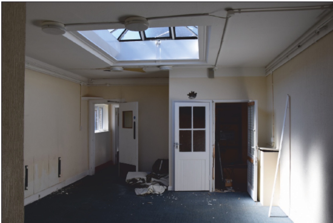
Photograph 68: Looking north-west across the old kitchen 40. The cupboards are on the site of the dumb-waiter lifts
