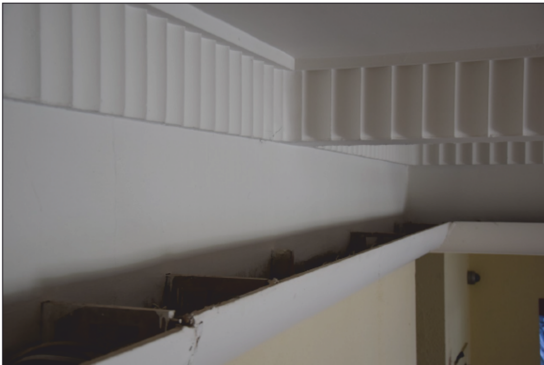
Photograph 48: Detail of the concrete ceiling beams and the plaster coving in the centre of the ballroom 15
