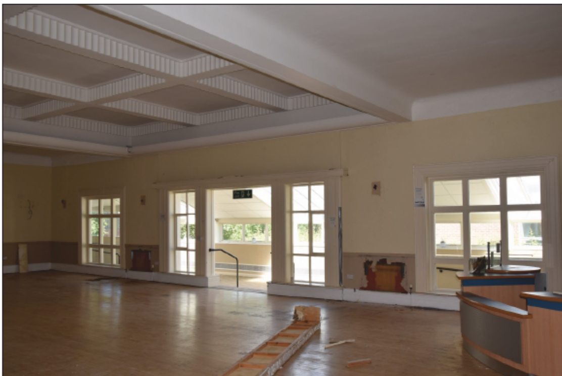
Photograph 50: The windows in the east wall of the ballroom, with the modern conservatory beyond
