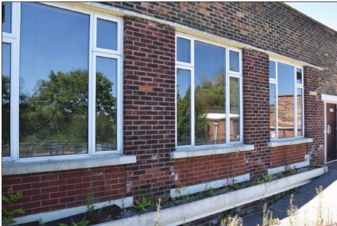
Photograph 18: The lounge windows have been reduced in size and re-glazed; the old sills are below the redder brickwork
