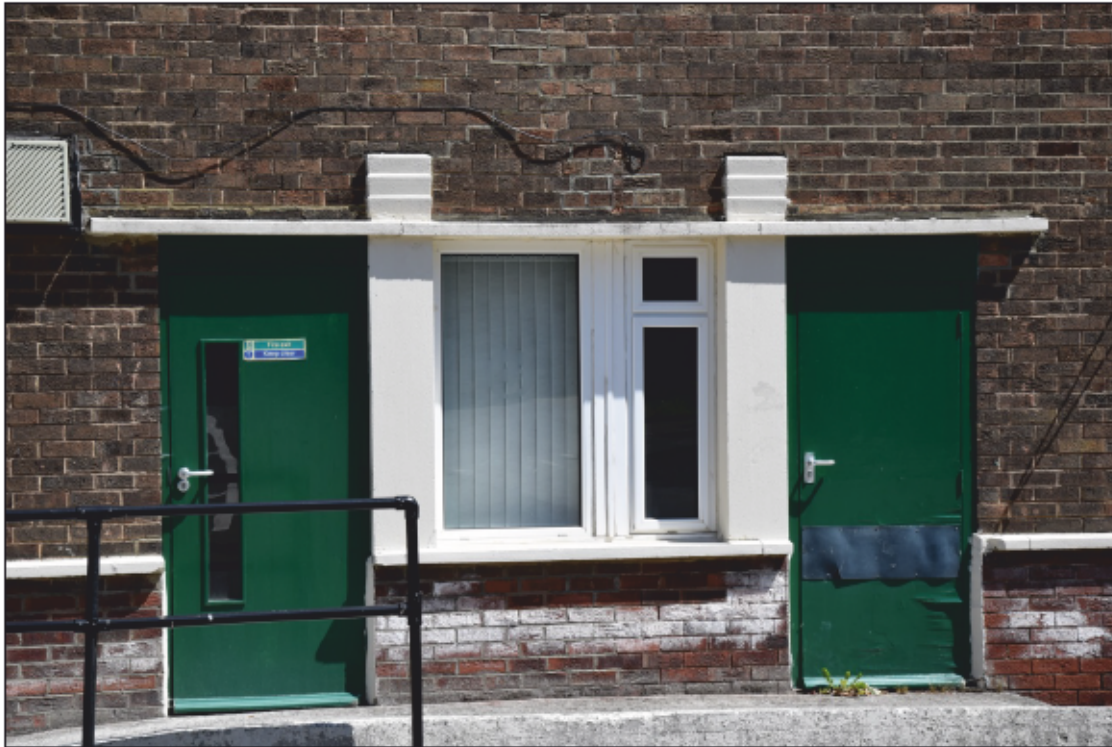
Photograph 13: The matching window in the south wing has been altered to create two doors
