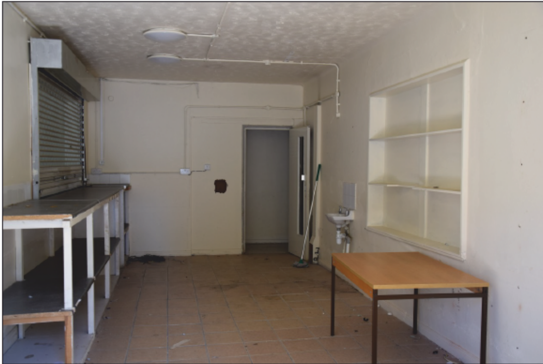
Photograph 35: The small room 10 contains the old south window of the dining room, now closed up and fitted with shelves
