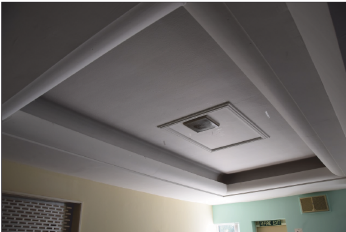
Photograph 34: The recessed centre of the ceiling in room 9; compare this with Photos 48 and 49
