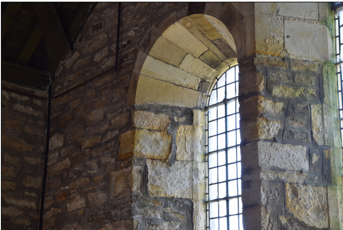
Photograph 28: Detail of the east window, showing damage to the surface of the stonework. The grey cement mortar can be seen clearly here
