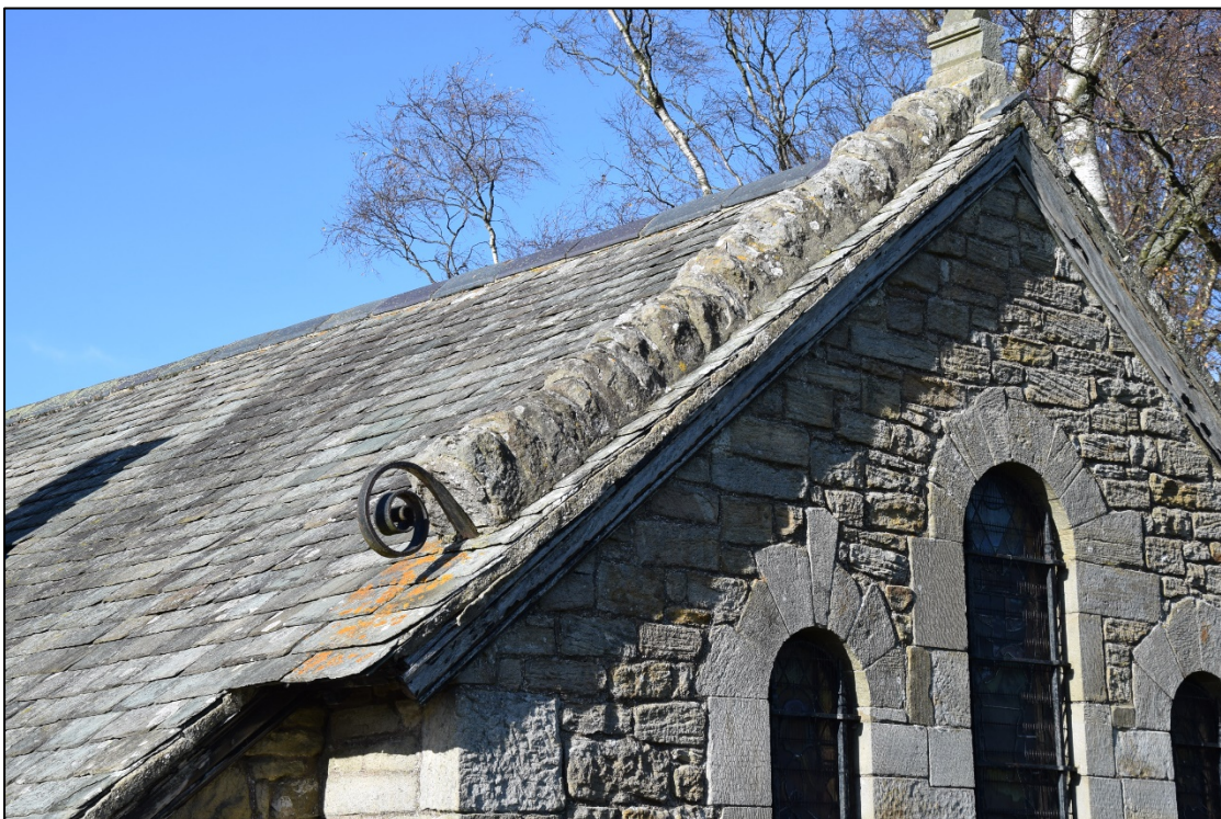
Photograph 10: Detail of the rustic coping on the east gable. Note the random lengths of the dressed quoins in the three-light east window
