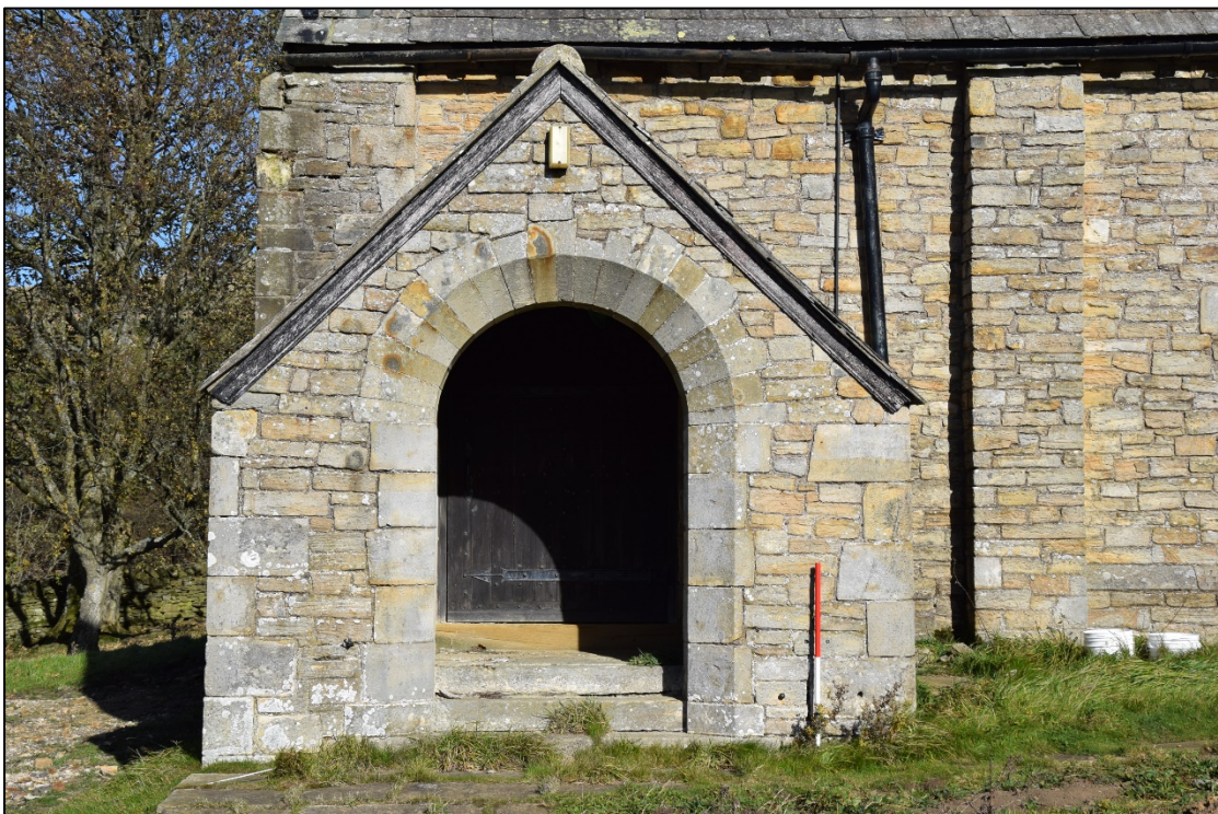
Photograph 4: The porch, with some sloping stone paving outside it. The scale is 1m long
