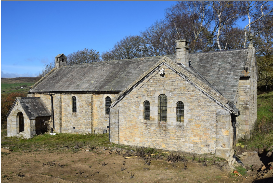
Photograph 3: The south face of the church. Note the recently-disturbed ground in the foreground. A bag at the peak of the gable covers recently-disconnected electric cables
