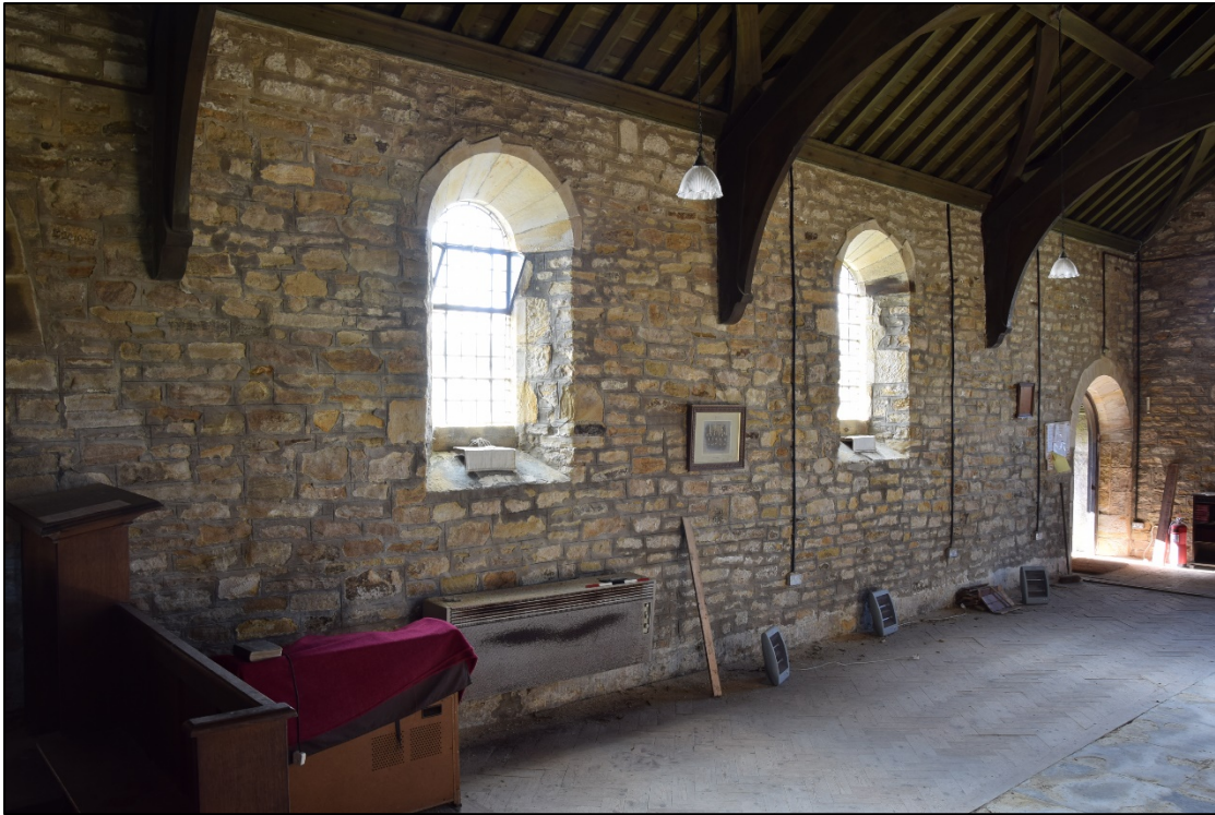
Photograph 25: The south wall of the nave, with one of the modern gas heaters
