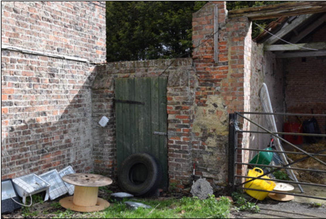
Photograph 63: The north face of the screen wall between the house and the barn
