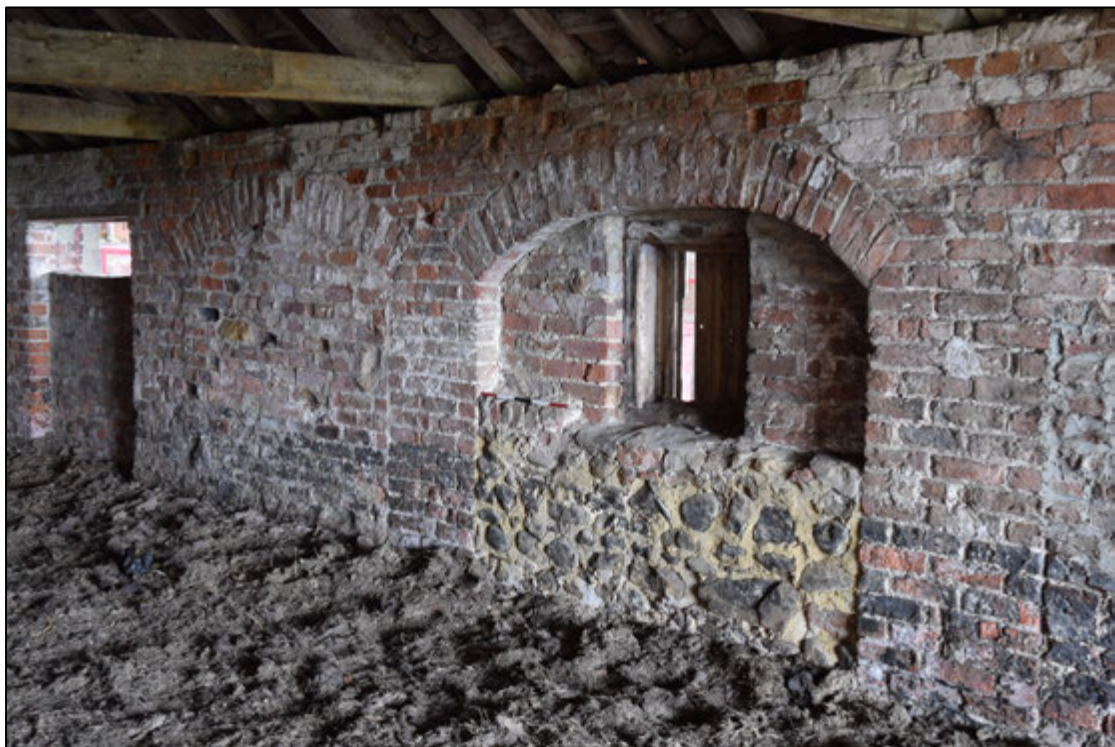
Photograph 80: The twin arched openings in the south wall of the byre. A view looking south-east
