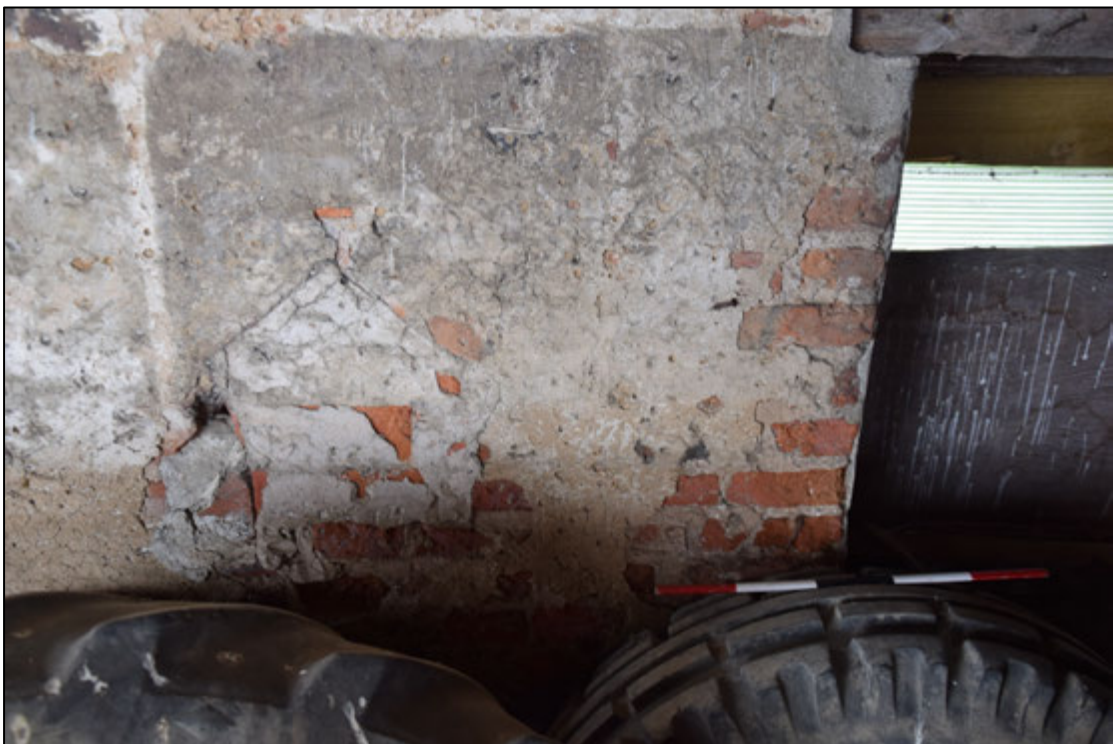
Photograph 58: Detail of the blocked niche, which would have been used for equipment or a lantern
