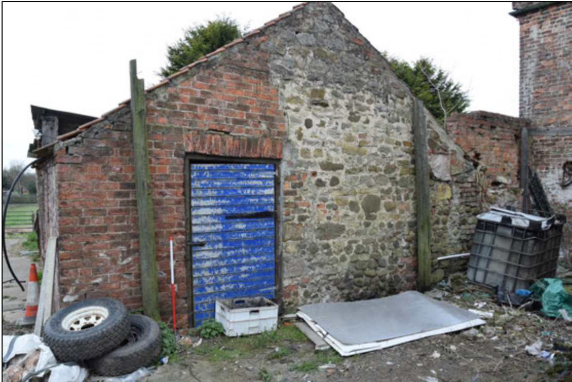
Photograph 45: By contrast, the north wall includes some older stone masonry of a character like that in the house and the workshop
