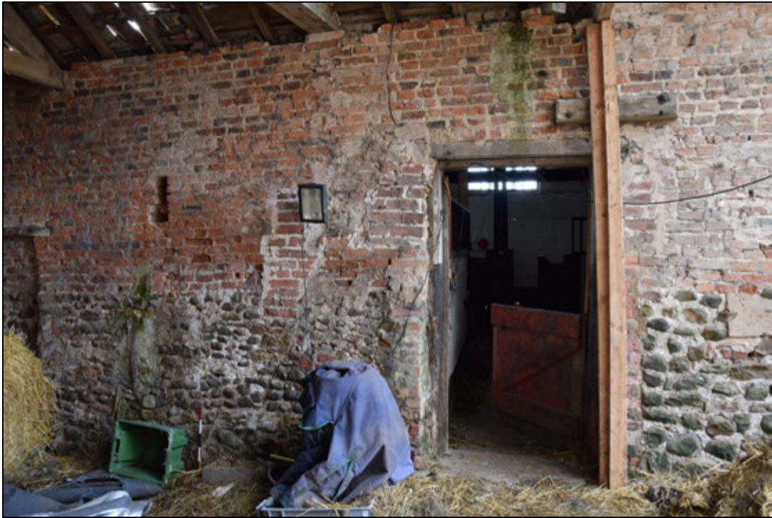
Photograph 69: Old stone and irregular brickwork, with extensive repairs, around the door to the stable building H
