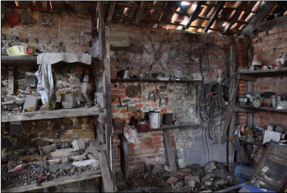
Photograph 39: The brick rebuild in the south wall of the workshop, with the blocked door seen in the previous photograph at the right
