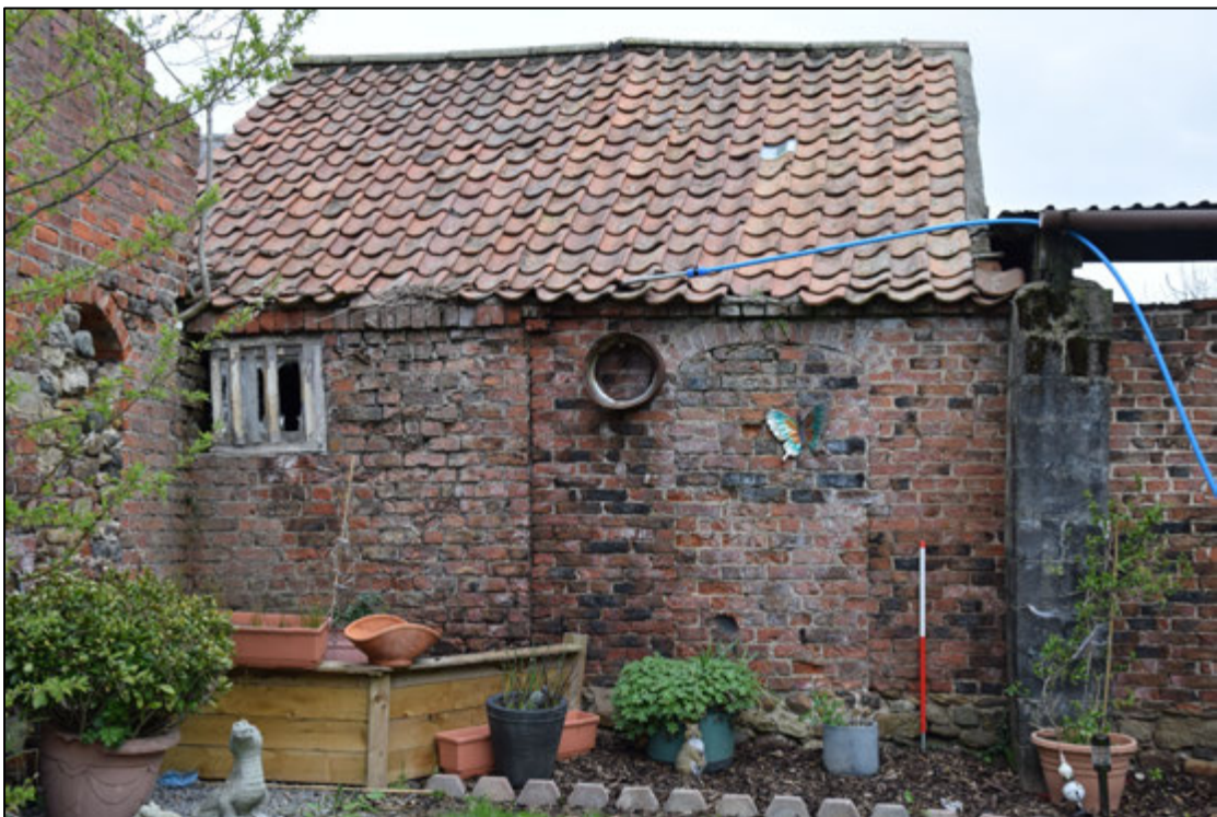
Photograph 48: The west face of the surviving section of the stable. The central straight joint shows that the northernmost bay, at the left, was formerly open on this side. The arch over the blocked door is the same shape as those further south and similar doors in the workshop and the screen walls
