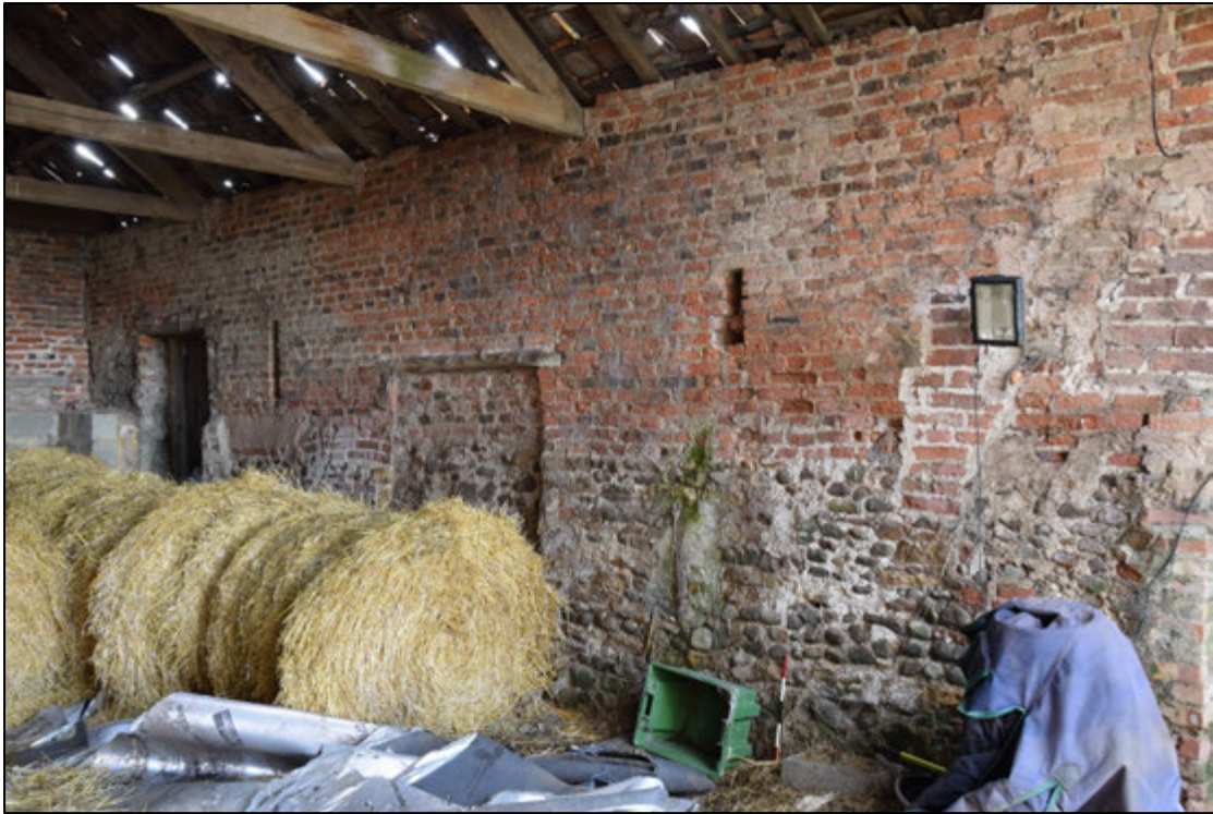
Photograph 67: The south end of the west wall in the barn. The mixture of brick and older stone can be seen here as elsewhere. The blocked door is now covered by the byre, building E
