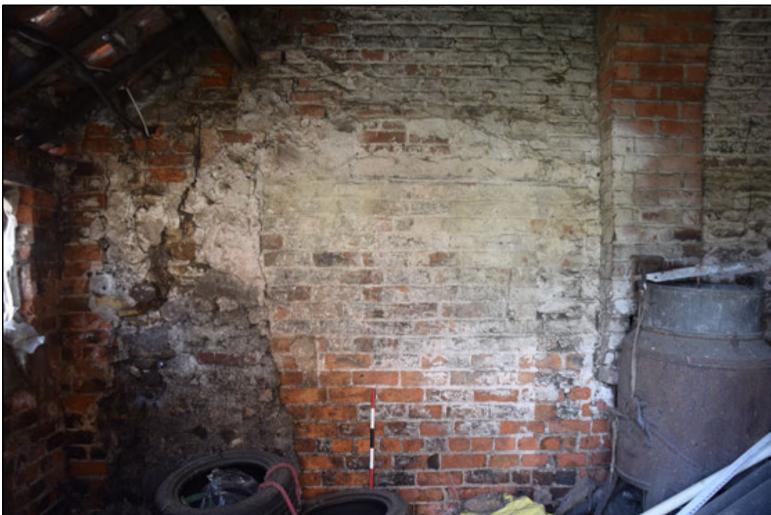
Photograph 52: A blocked opening in the south wall of the shed, with old stone masonry at its left side
