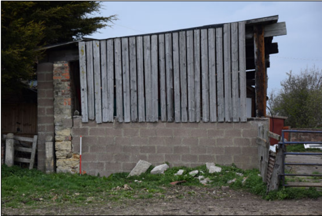
Photograph 47: The south end of the former stable. The only old masonry is the end of the wall beside the concrete pier at the left, which is built of brick over stone
