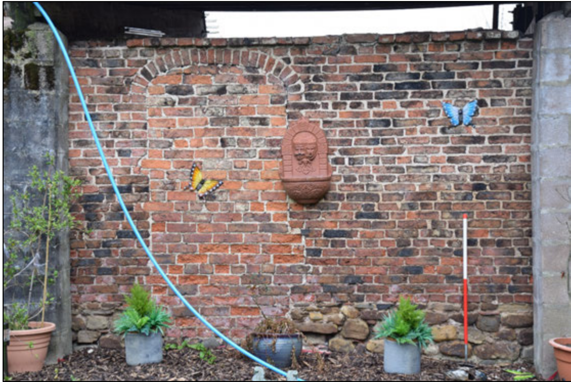
Photograph 49: Another blocked opening in the second bay from the north end of the stable
