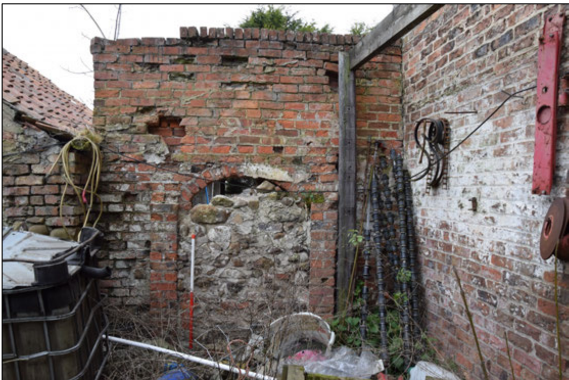
Photograph 46: The screen wall between the stable (left) and the house. A view looking south
