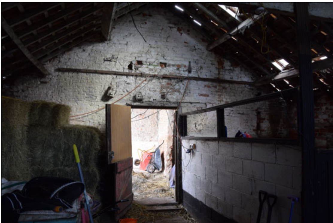
Photograph 72: The west face of the stable seen from the stable. No evidence of openings or fittings connected with a gin-gang can be seen here
