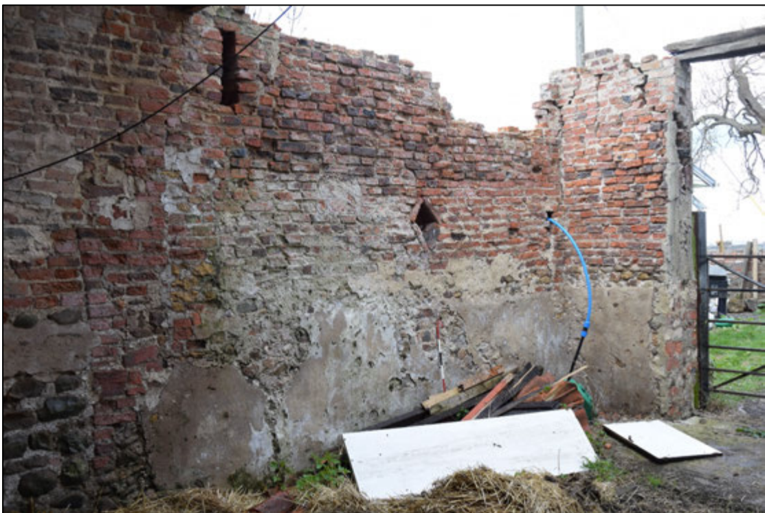
Photograph 70: Irregular brickwork and the diamond-shaped ventilator at the north-west corner of the barn
