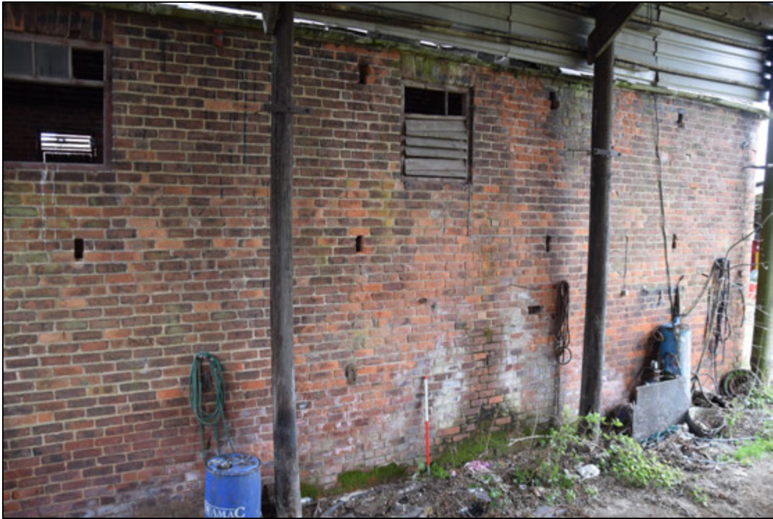
Photograph 97: The east wall of the building has only two louvred windows. The smaller holes are the marks of a later shed built against this face
