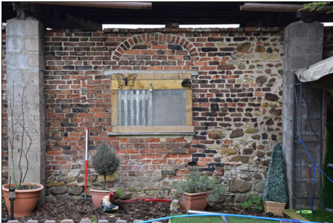
Photograph 50: A third blocked door in the west face of the stable. There is a small breather slit to its left, above the scale. Note the change to old rough stone masonry at the right
