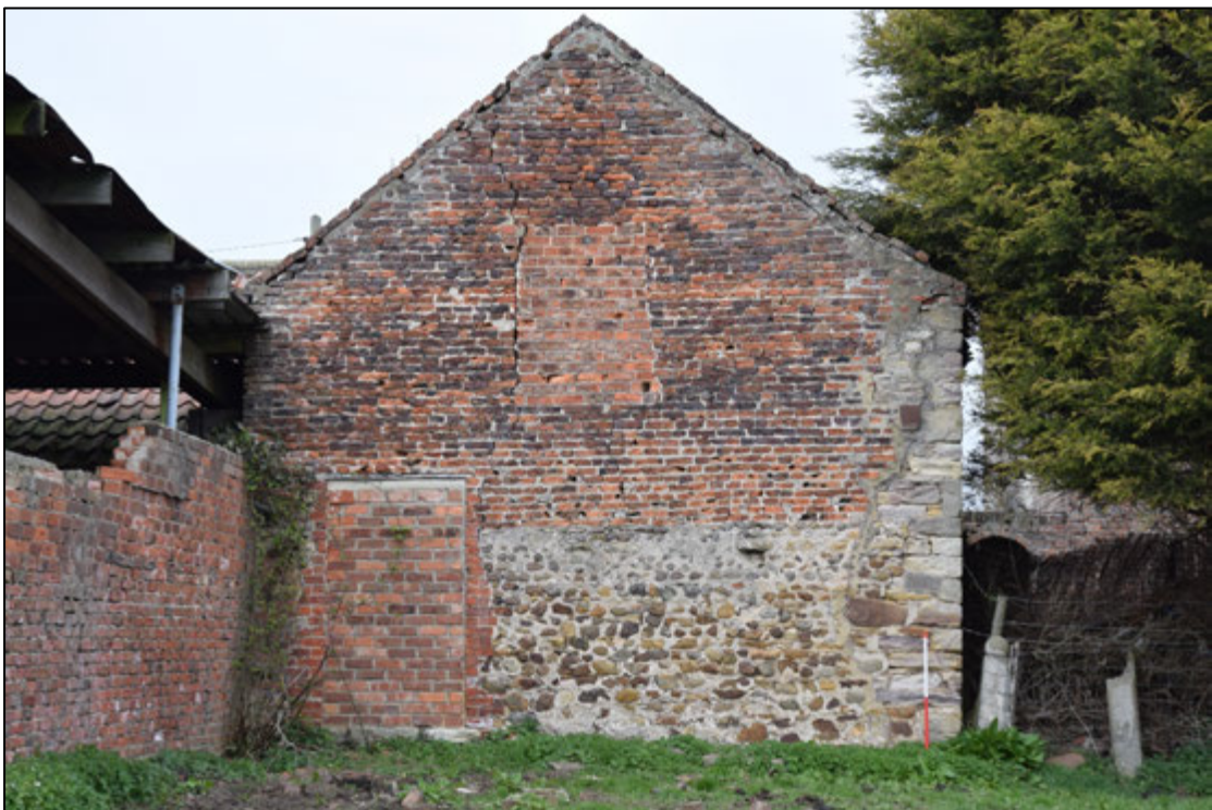
Photograph 60: Rougher stonework can be seen in the lower part of the barn's south end. The door at the left is clearly a later addition but the pitching door in the gable is contemporary with the surrounding brickwork
