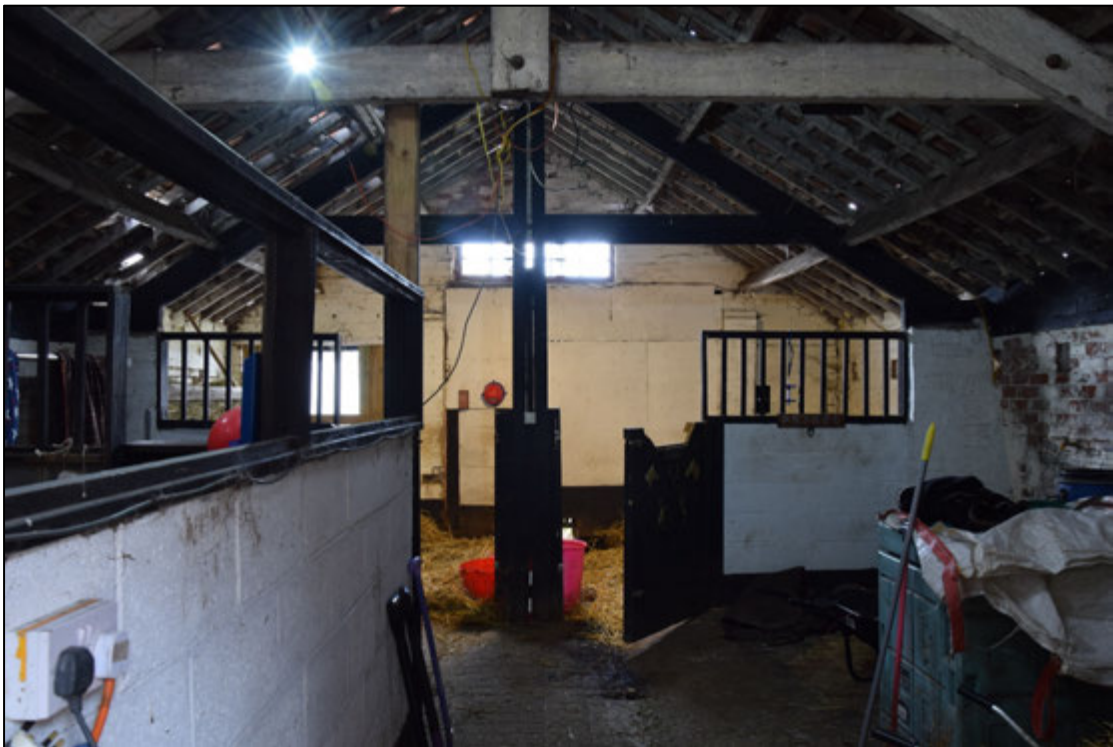
Photograph 92: A view looking west in the stable. The concrete loose-box partitions were built within the past five years
