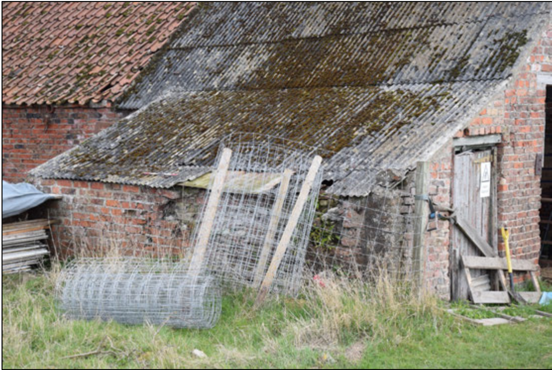
Photograph 83: The small shed F is all that remains of a west range shown on the 1857 Ordnance Survey map
