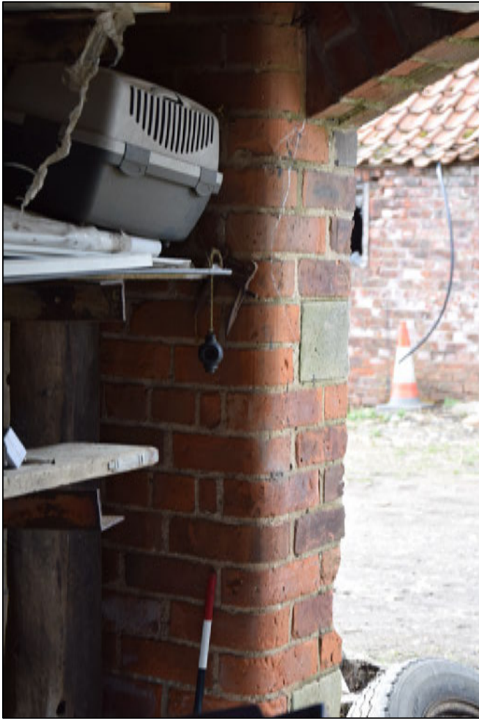
Photograph 99 (left): Detail of the rounded corner of one of the piers at the front of the cart shed
