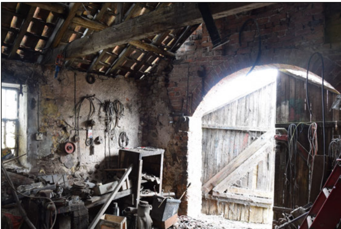
Photograph 40: Mixed brick and stone in the north-east corner of the workshop, with some plaster on the walls
