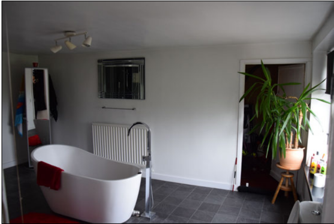
Photograph 27: The modern bathroom 10 has no historic features but the far wall is an old plank-built partition
