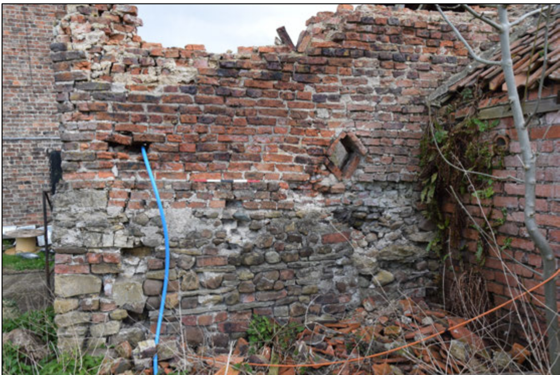
Photograph 62: Brickwork over older rough stone at the north-west corner of the barn. The wall at the right is the later stable, building H
