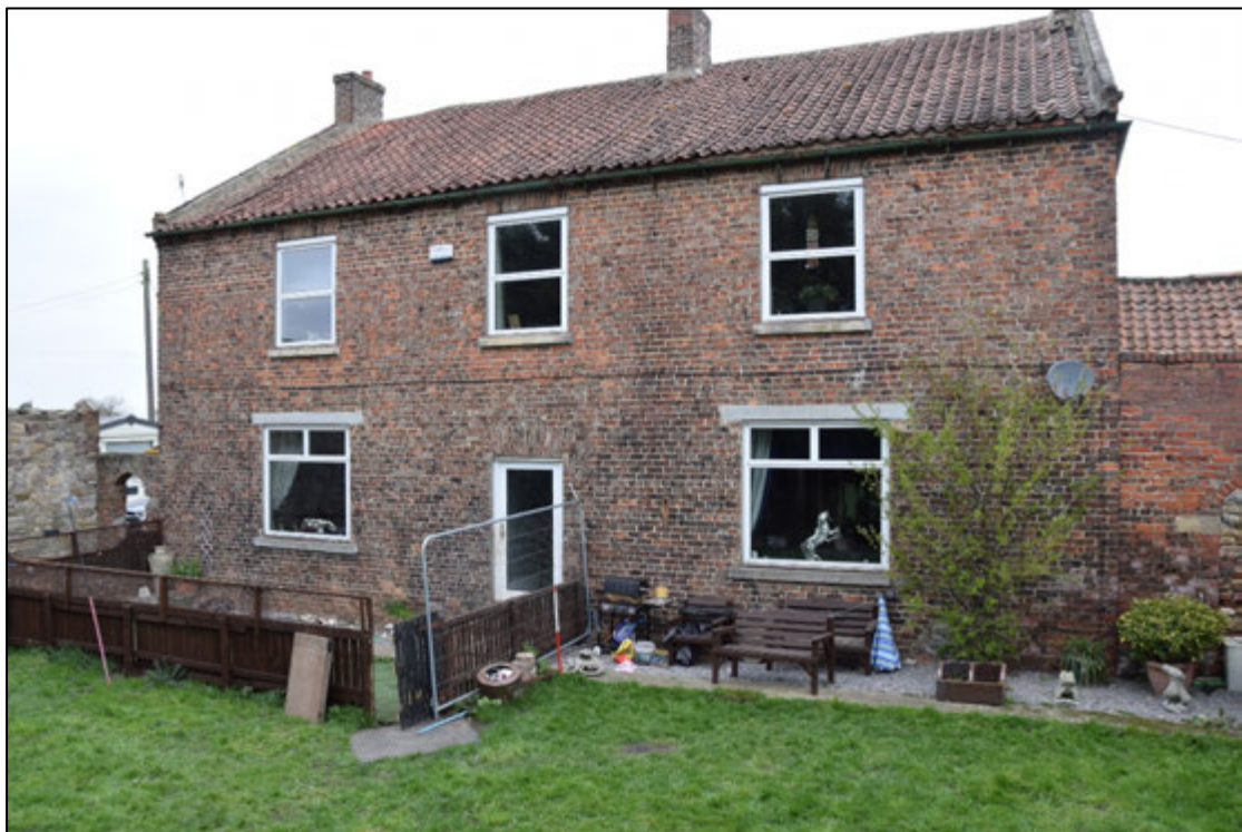
Photograph 6: An oblique view of the front of the house. Short sections of wall at either end separate the garden from the rest of the steading
