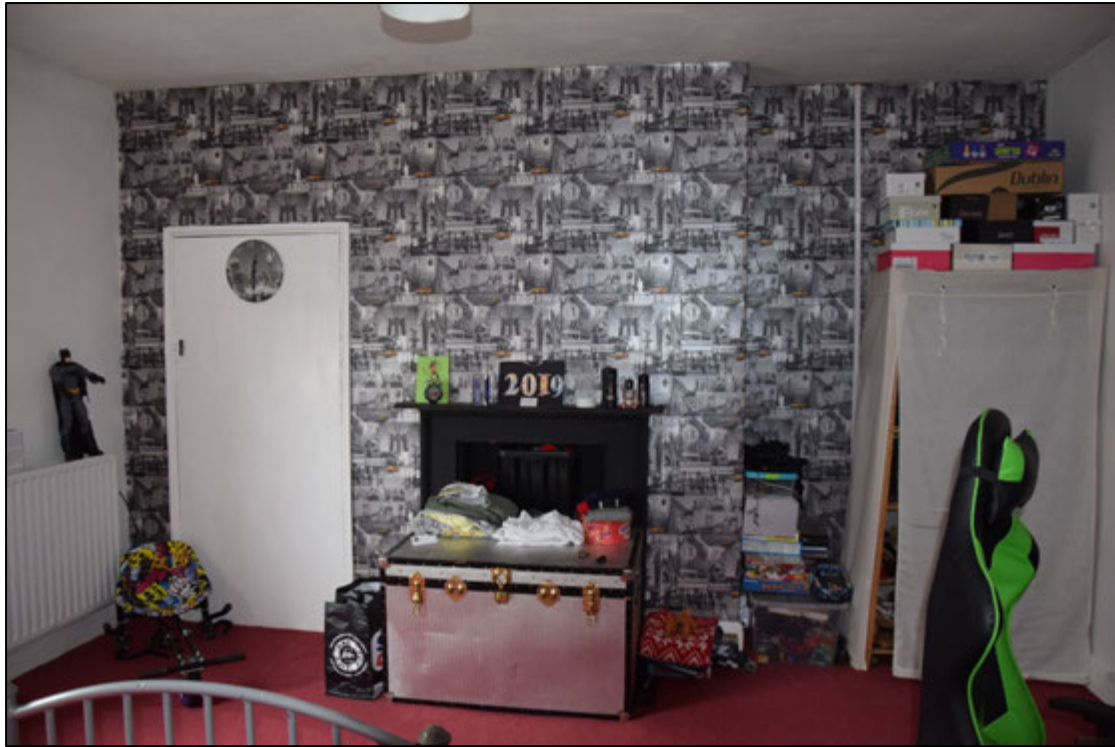
Photograph 33: A chimney breast and flanking cupboard in room 14, at the south-west corner of the house
