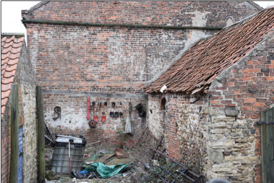
Photograph 9: The outline of the old building projects slightly from the east gable, above the roof of the adjoining workshop
