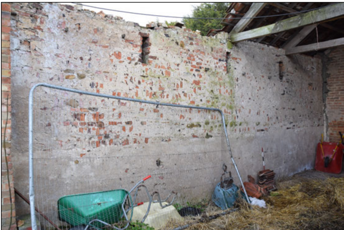
Photograph 66: The inner face of the east wall, with brickwork, cement render and small timber stubs below the level of the breather slits
