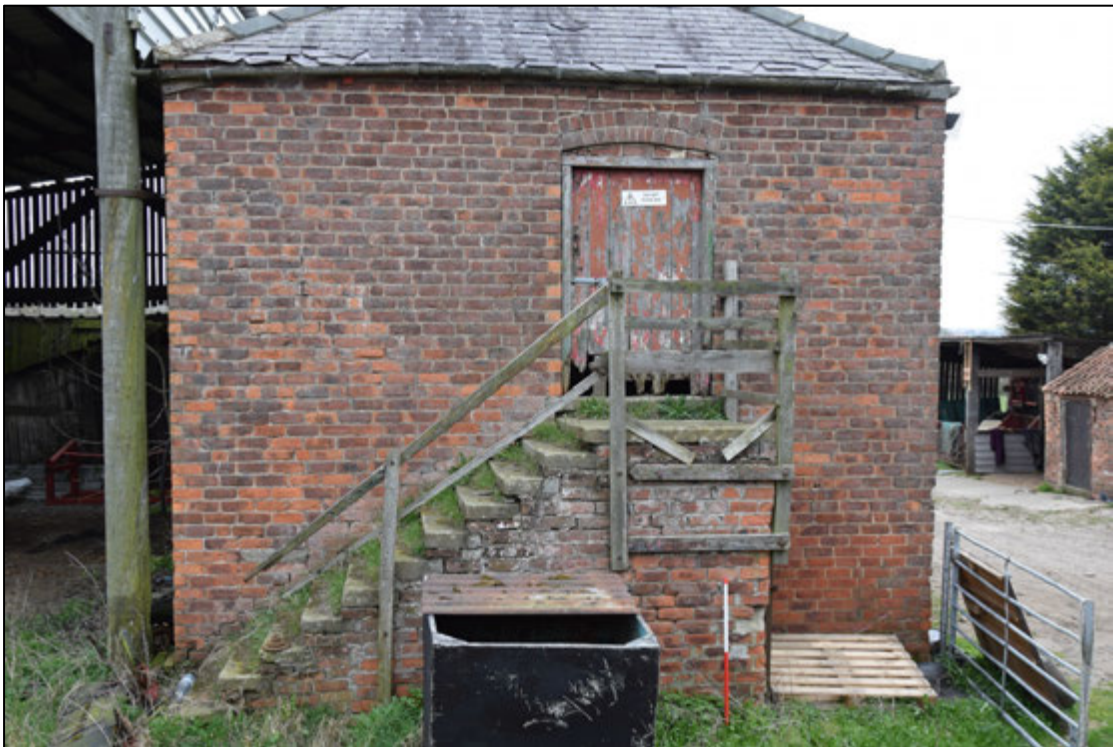
Photograph 94: The wide external stair at the north end is a typical feature of buildings of this kind
