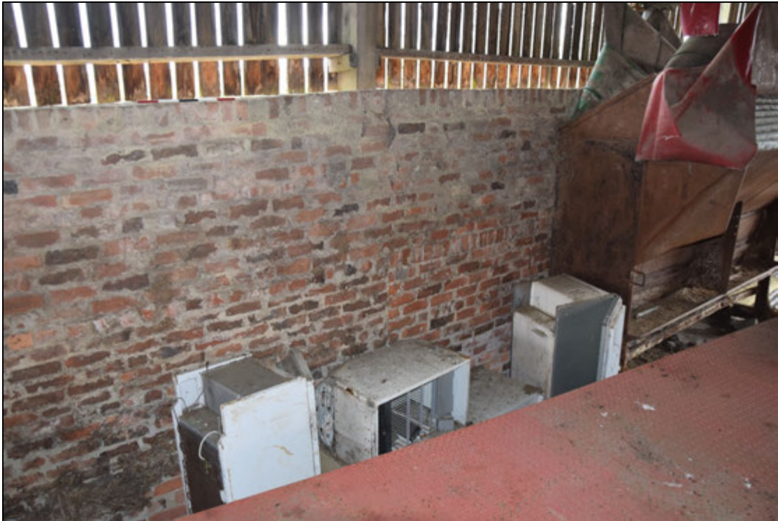
Photograph 89: A straight joint and coping marks part of the south end of the western building that has been absorbed into building G. A view looking south-west
