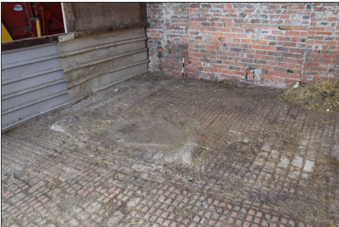
Photograph 56: Concrete surrounds the sockets for heel posts and the floor drain at the rear of the former stalls can still be seen
