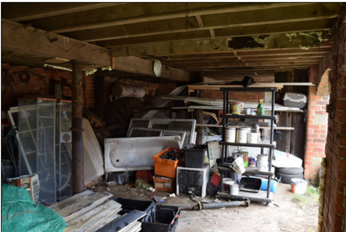
Photograph 98: The interior of the cart shed, seen from the north-west corner. The heavy central beam and the cast-iron columns can be seen here
