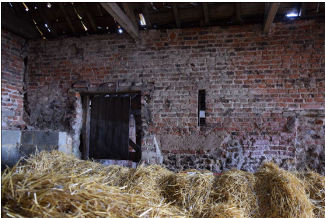
Photograph 68: Most of the brickwork at the south-west corner of the barn is more even than that in the lower part of this wall, or at the north end (Photo 62)
