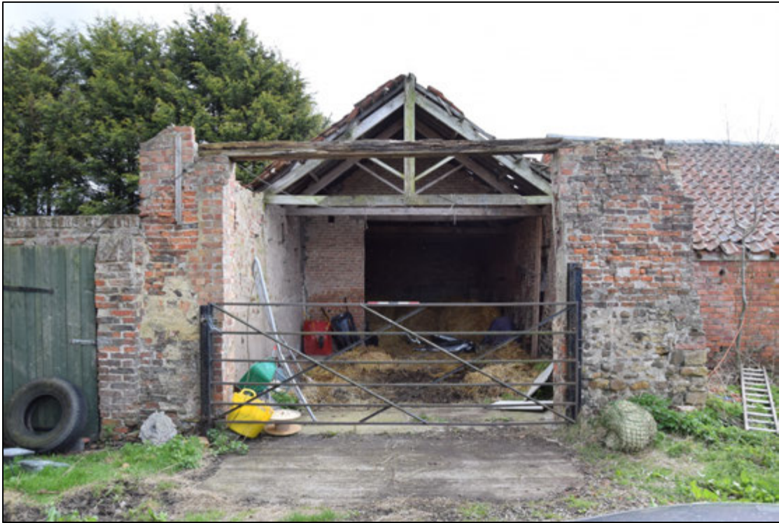
Photograph 61: The north end of the barn is largely gone. The simple agricultural roof trusses can be seen here
