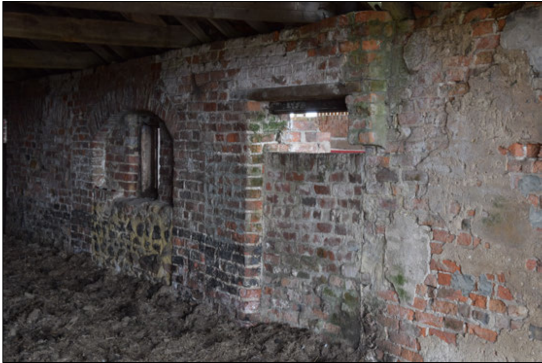
Photograph 79: The west end of the south wall. The thicker section, centre and right is part of the original building
