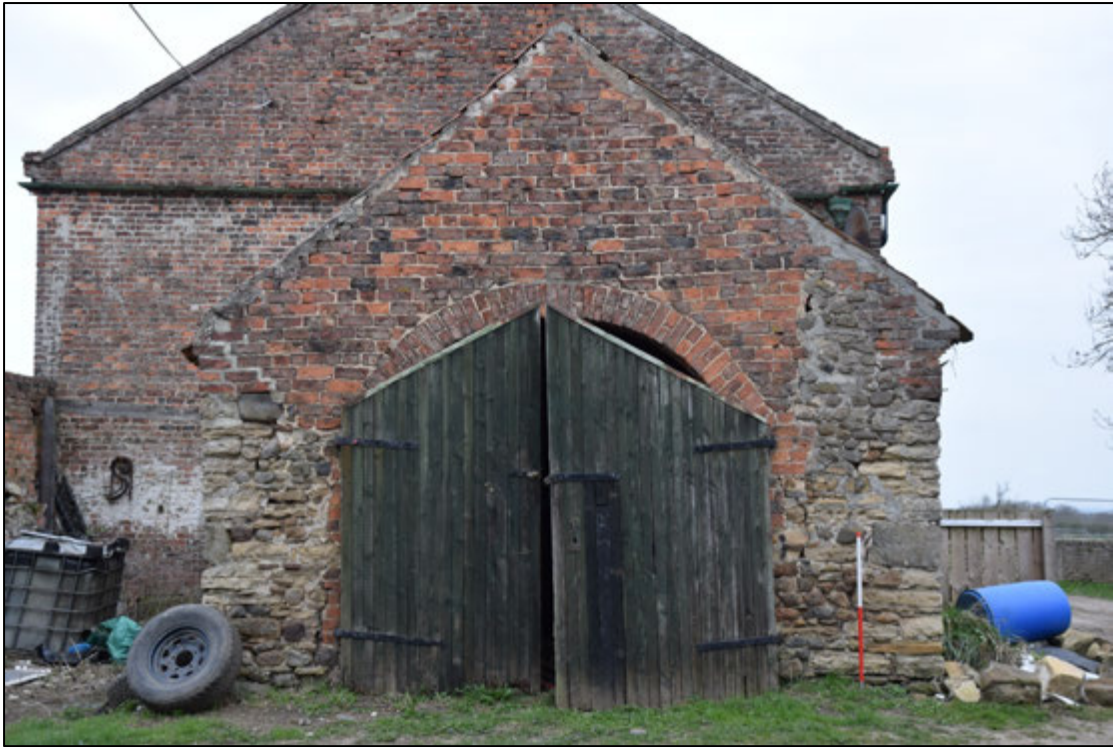
Photograph 37: The east end of the workshop was substantially rebuilt to accommodate the large double door. Note the occasional large stone blocks at the corners of the old walls
