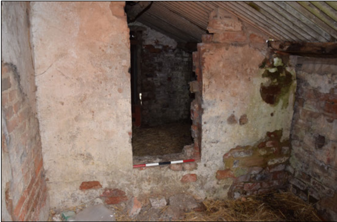
Photograph 85: A modern opening in an internal wall; the building is now a dog kennel
