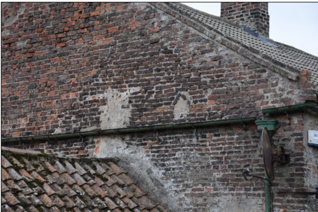
Photograph 10: The old gable visible above the roof of the workshop. Note the scar of a chimney rising from the lower roof, and the small blocked opening with a triangular head to its right
