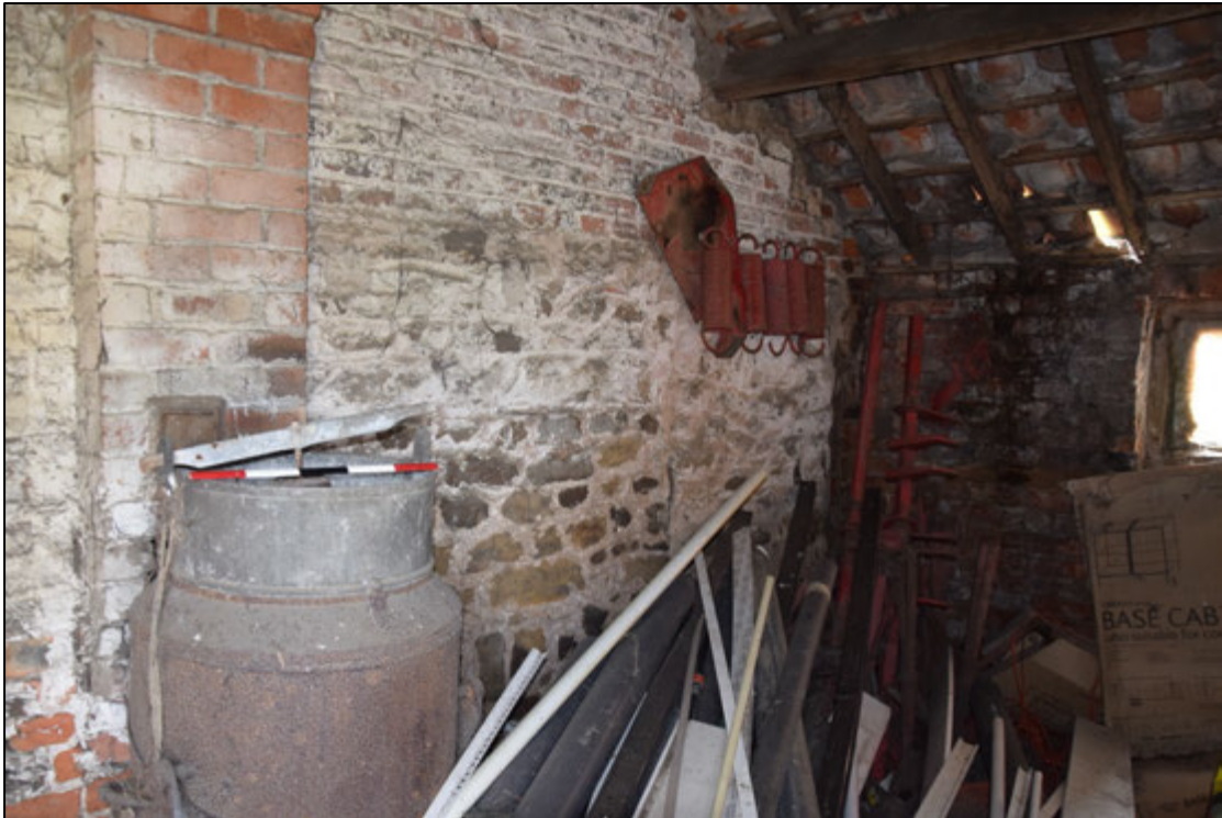
Photograph 51: A view looking south-west inside the north room of the stable block. The brick at the left is the later flue for a stove
