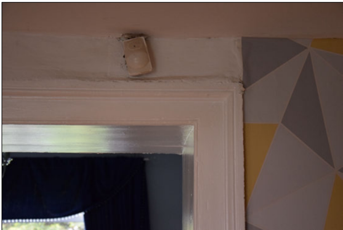
Photograph 14: The architrave on the kitchen side of the door seen in Photo 13
