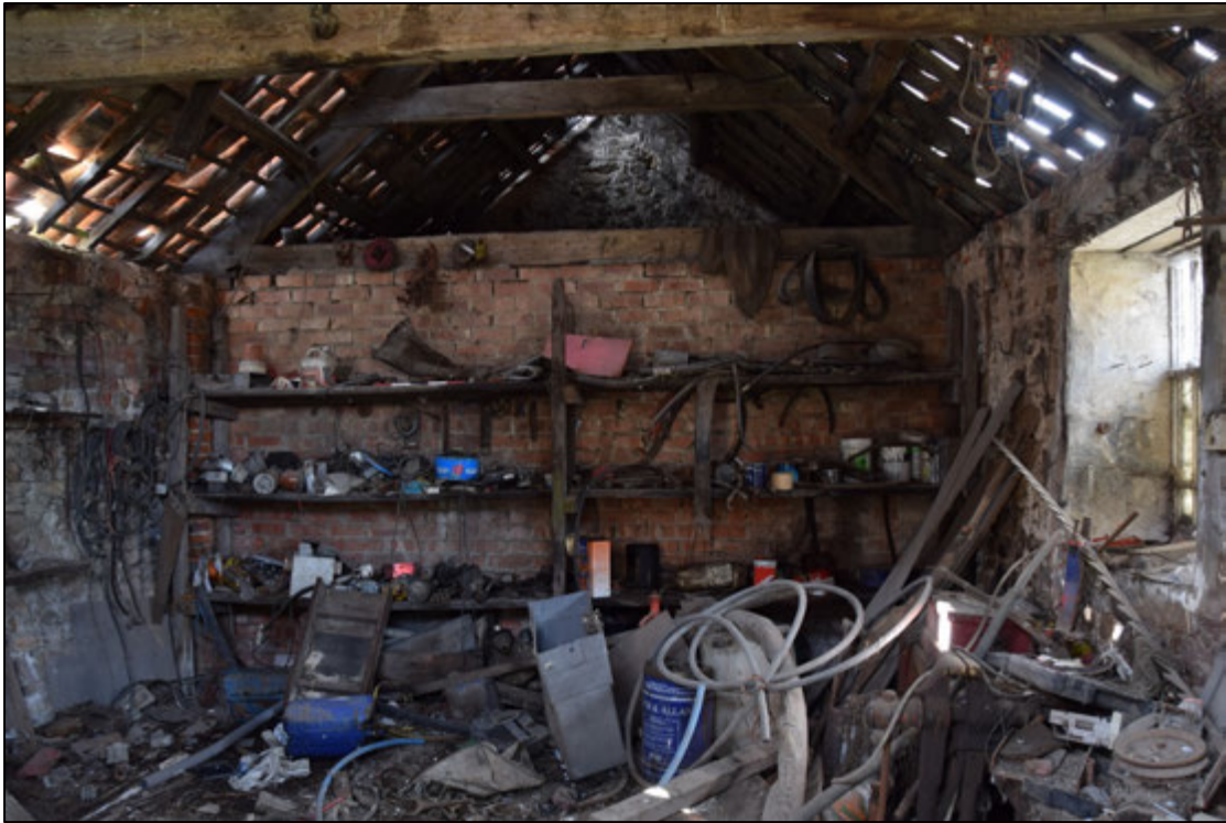
Photograph 41: The modern wall that divides the workshop only reaches the bottom of the simple roof truss
