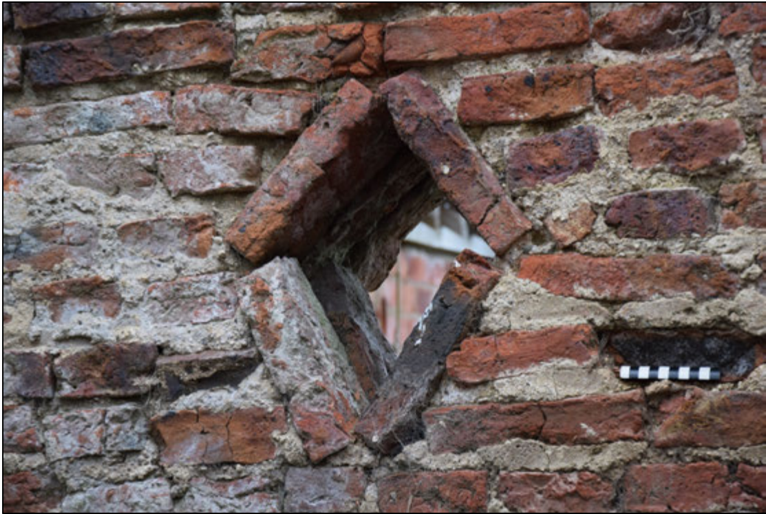
Photograph 71: Detail of the ventilator seen in the previous photograph. The scale is 10cm long
