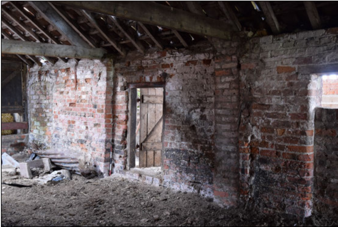
Photograph 77: The east end of the byre's south wall. Ragged brickwork right of the pier that carries the near roof truss marks the old east wall of the building. The door leads out onto a modern feeding gangway in building G
