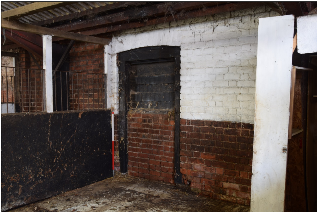
Photograph 58: One of the blocked doors in the east wall of the central range, with part of the steel frame of the covered yard [17]
