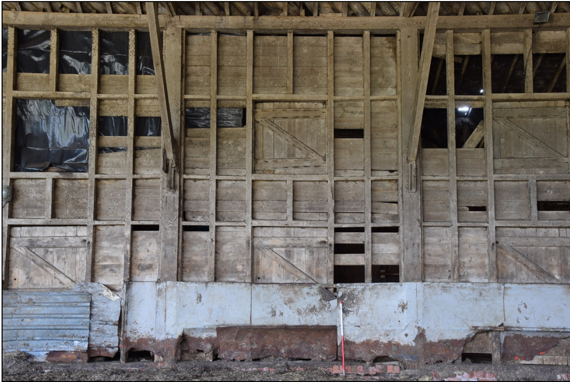
Photograph 43: A typical bay in the south wall, with upper and lower feeding doors. Steel sheets, installed when the building was used as a cow-house, cover the lower section of the face. The brick sleeper wall can be seen in the middle of this picture
