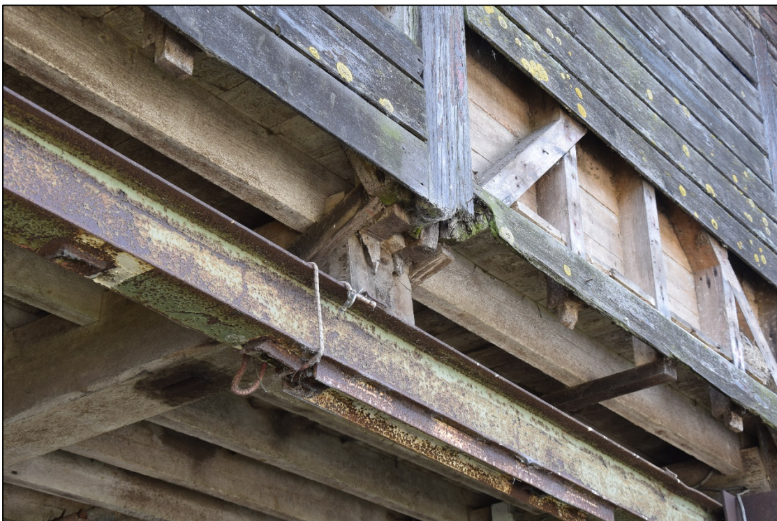
Photograph 32: Detail of the crude alteration made to create a wide opening at the east side of the shed [7]. The form of the double-skinned timber wall of the granary is clearly seen here. A view looking south-west
