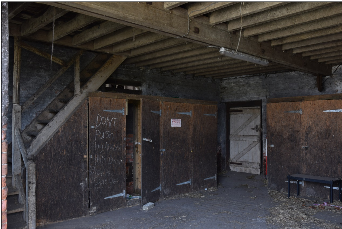
Photograph 14: The ground floor room [4] in the west block, showing the stairs and the door to the feeding passage [10]
