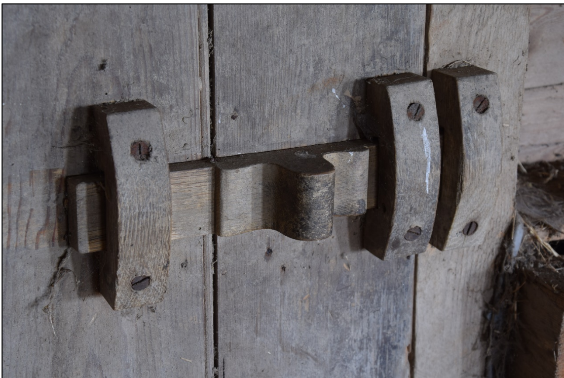
Photograph 26: High-quality joinery in the bolt of the door from [6] to the feeding passage
