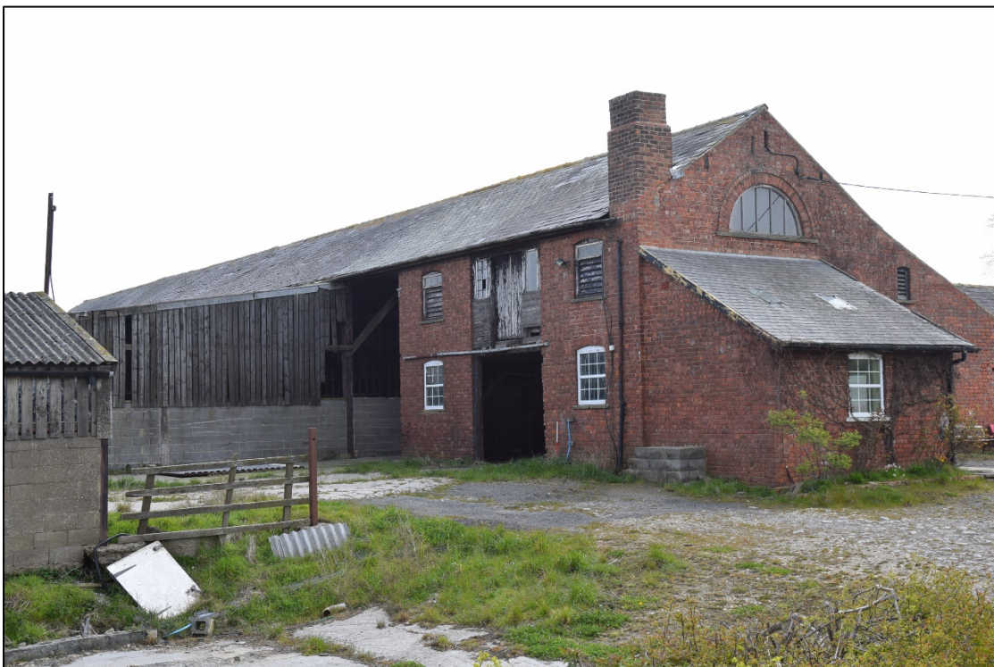
Photograph 4: The north-west corner of the main building, with the later pole barn left of centre
