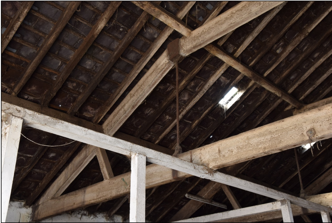
Photograph 57: Detail of one of the timber and iron roof trusses in the central range [13]
