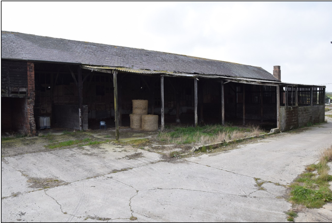
Photograph 5: The dilapidated pole barn [1], seen from the north-east
