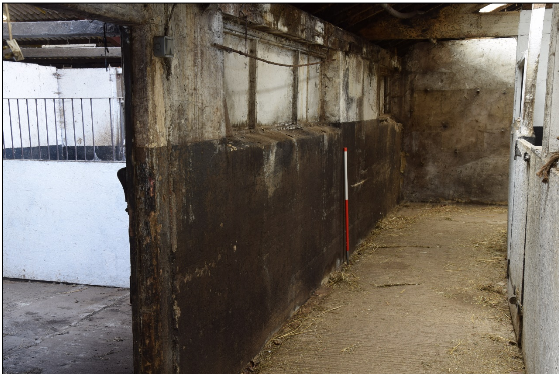
Photograph 50: A view looking south-west at the old north end of the west yard
