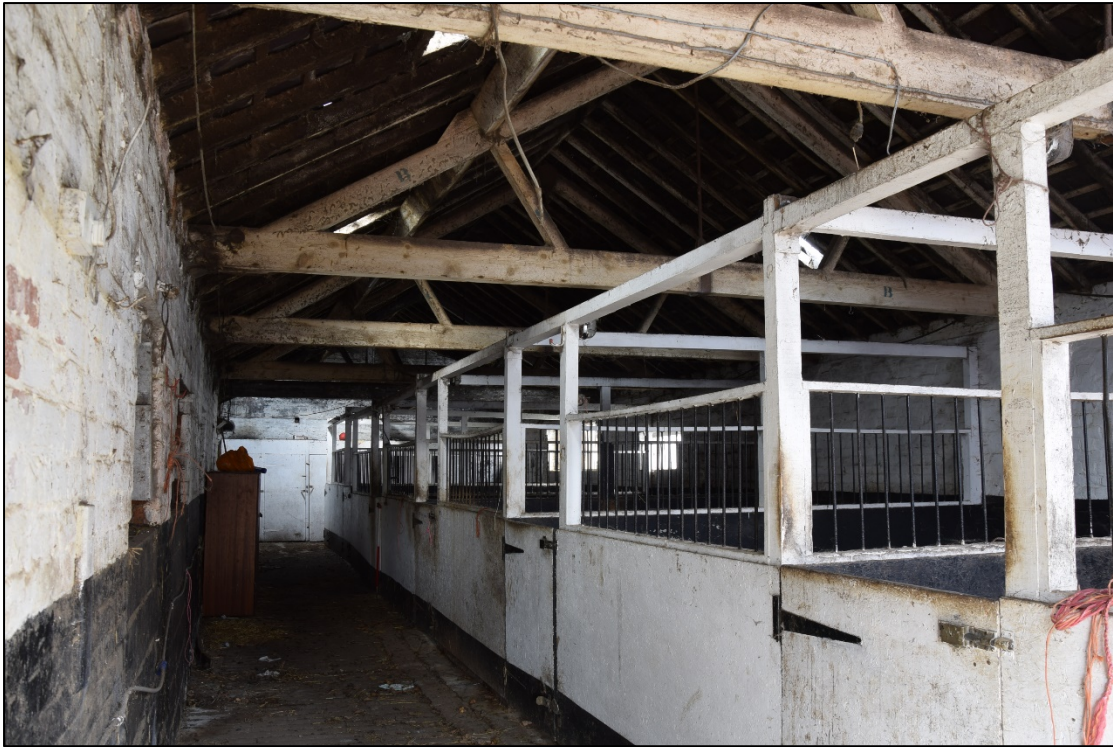
Photograph 61: The interior of the east range, with the wall of the granary block at the far end. Note the stencilled letters painted on the roof trusses
