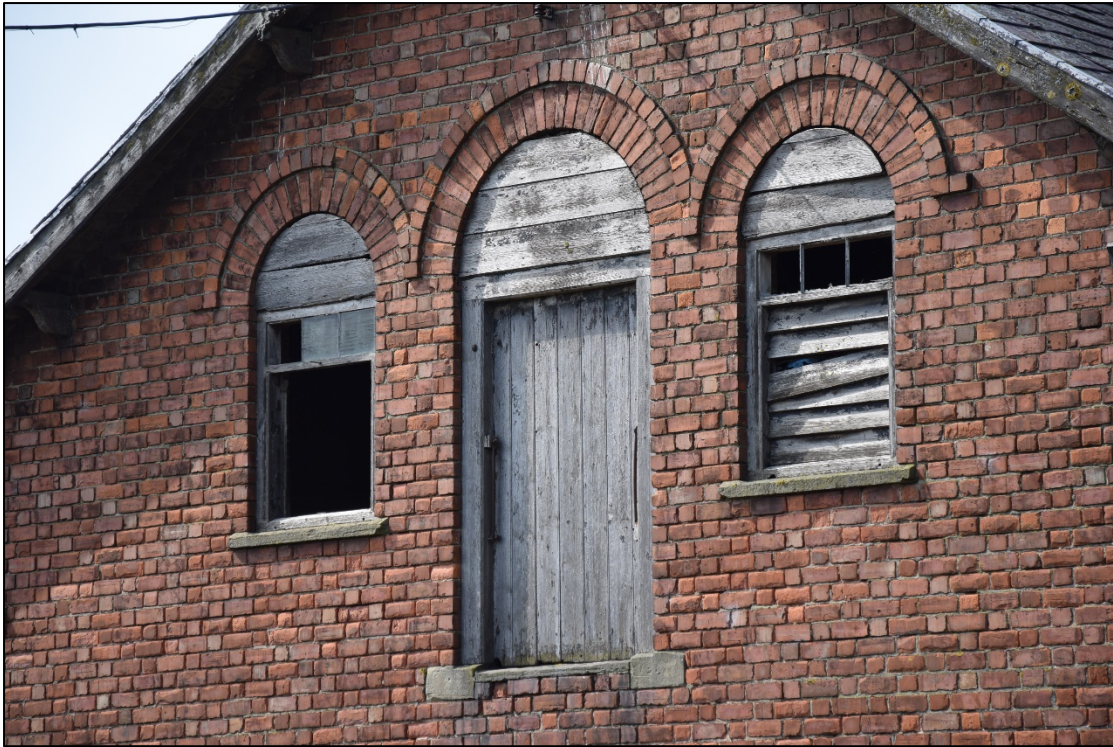
Photograph 35: The loading door and louvred windows at the east end of the granary [8]
