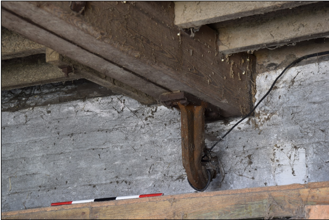
Photograph 17: An iron bracket at the south end of the ceiling beam in room [4]. This supported a bearing for a shaft that ran parallel with the wall
