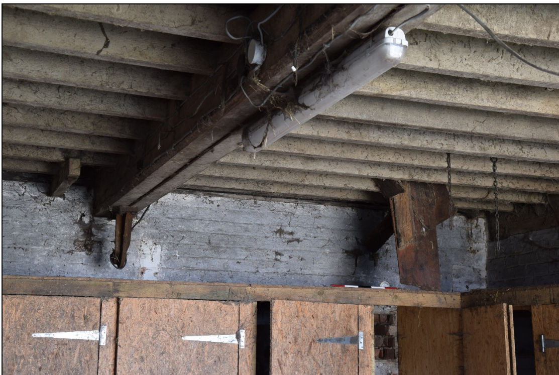
Photograph 18: The south-west corner of room [4], showing the beam, bracket and wooden chute from a first-floor hopper
