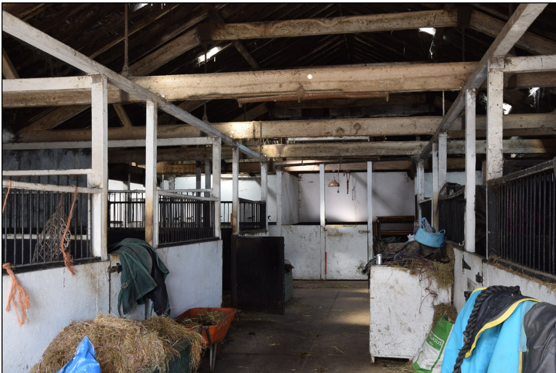
Photograph 56: The junction of the centre range [14] and the east-west stable [12]. A view looking north-west
