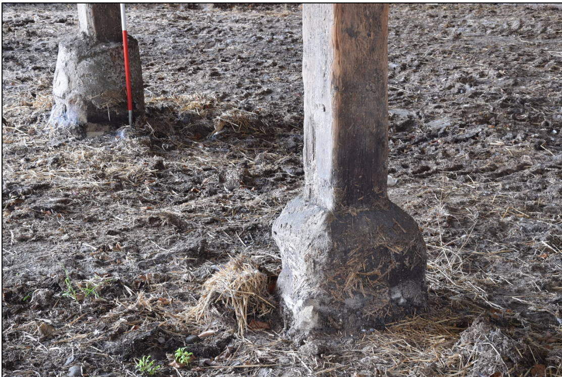
Photograph 42: The stone blocks supporting the timber columns on the north side of the barn; note the crude cement repair on the left
