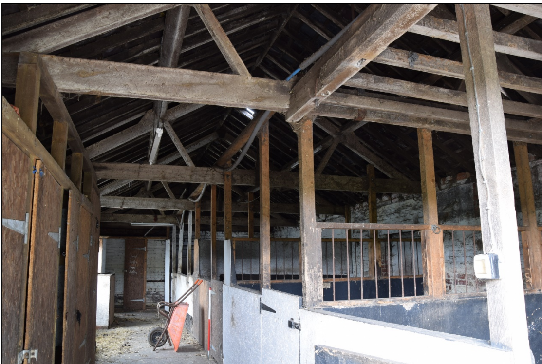
Photograph 52: The interior of the west range [13]. The scar of the lower part of the chimney is covered by one of the lockers at the left
