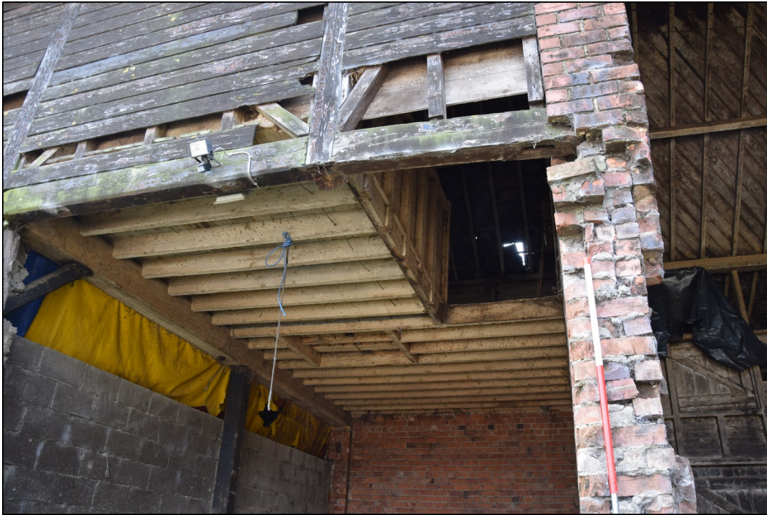
Photograph 33: A trapdoor and the opening for the original granary staircase in the west bay
