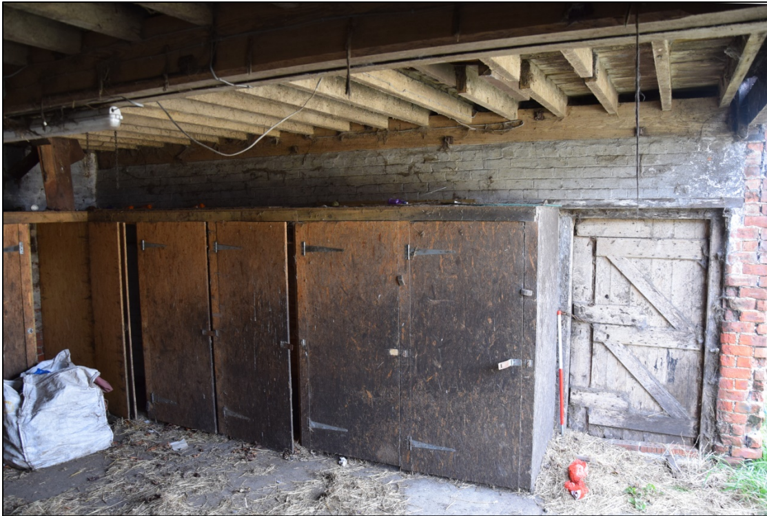
Photograph 15: Most of the west wall in [4] is concealed by lockers; the door leads to the small store room [5]
