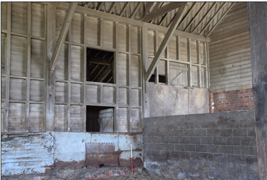
Photograph 44: Open feeding doors at the south-west corner of the hay barn. The brick and timber wall at the right is the end of the west block
