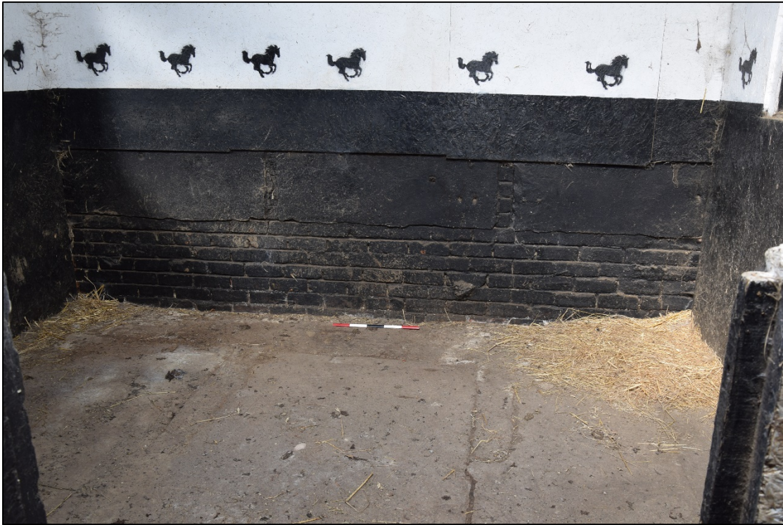
Photograph 49: The marks of old stall partitions can be seen in the floor and north wall of one of the loose boxes in [12]
