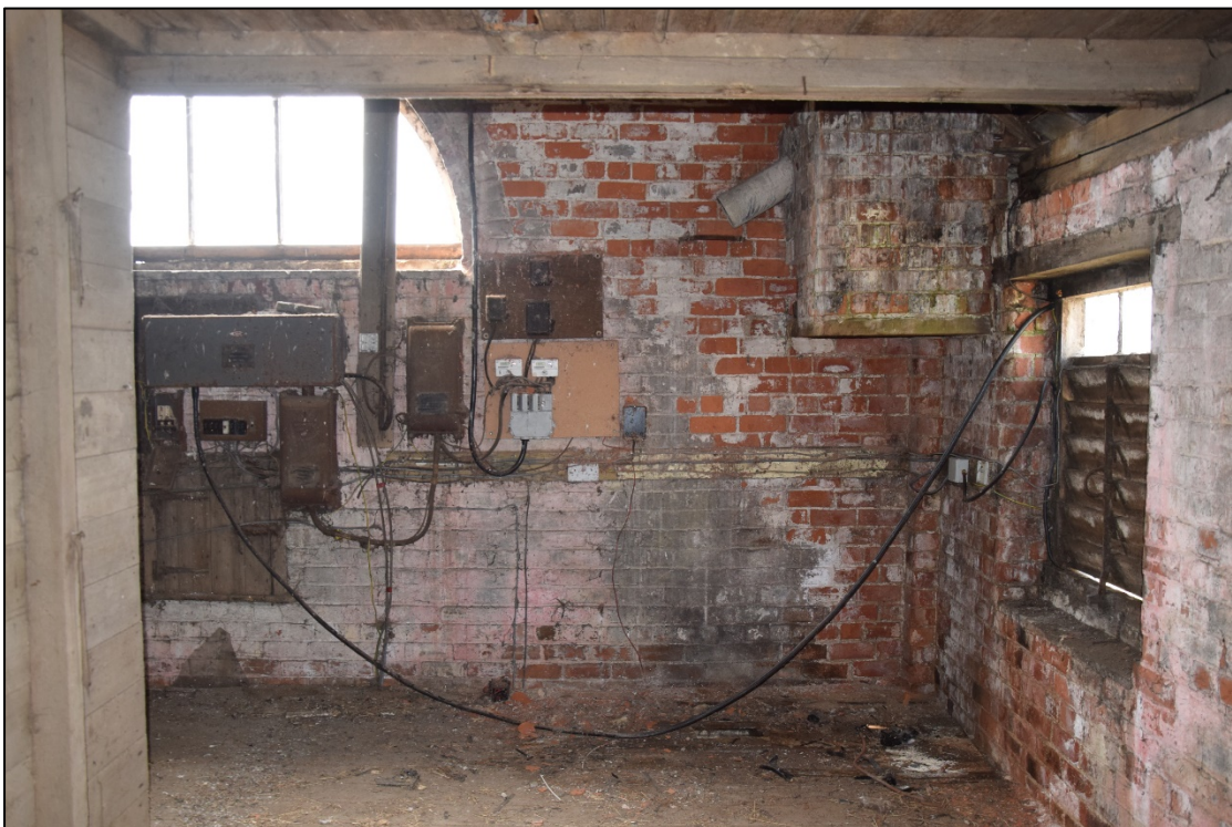
Photograph 22: The chimney and later electrical equipment at the north-west corner of room [6]
