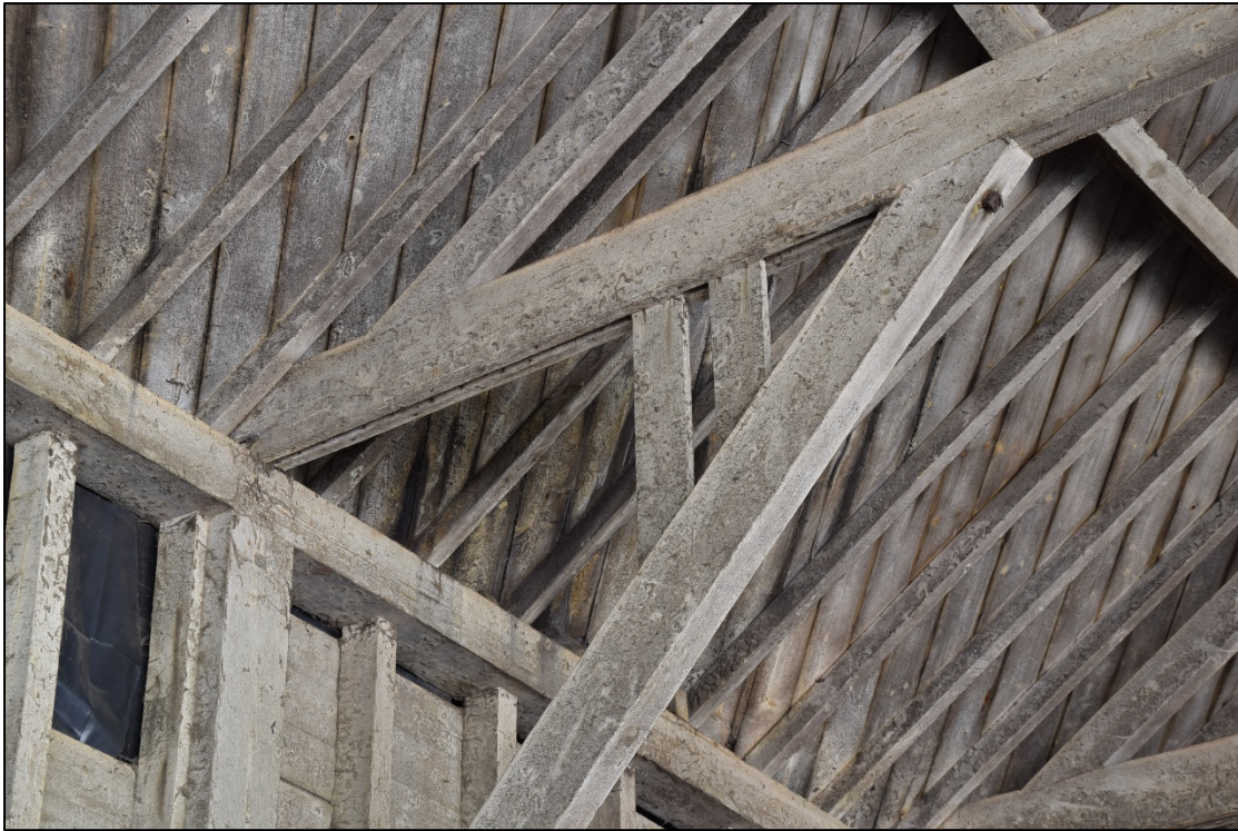
Photograph 41: Detail of the slots and plank partition below one of the tie beams in the barn
