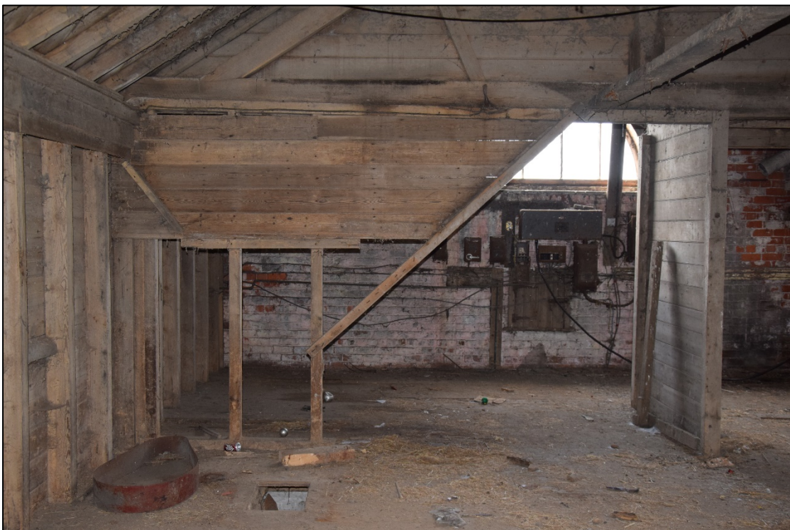
Photograph 24: A view looking west at the remains of the hopper in room [6]
