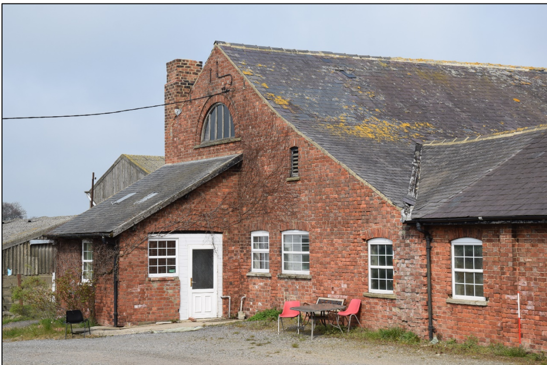
Photograph 10: The lean-to formerly had a wide door that filled most of its south wall. A view looking north-east
