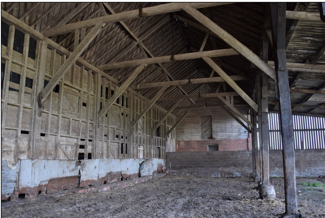
Photograph 38: The whole of the hay barn's south wall is timber and the opposite side was originally open to the yard
