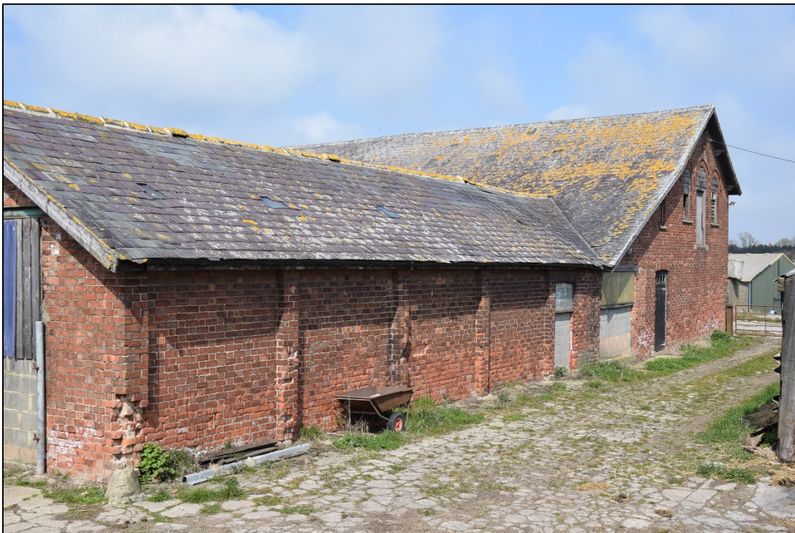
Photograph 6: The east end of the building, showing the first-floor door to the granary at the far end
