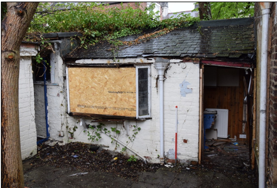
Photograph 14: The lean-to kitchen on the west side of the yard butts up against a smaller shed at the left, now the bathroom
