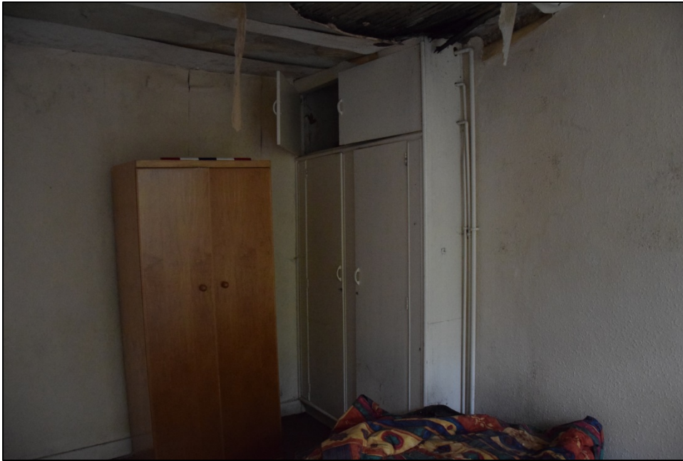
Photograph 33: The cupboard on the north side of the chimney breast covers the site of the blocked window seen in Photo 12
