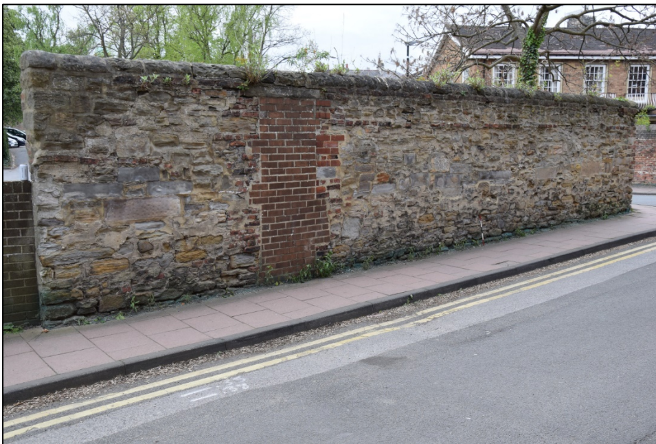
Photograph 50: The north face of wall A. The bricked-up door is shown on the 1861 map
