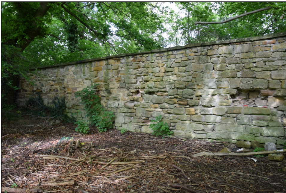
Photograph 126: Wall K, west face. The masonry here, near the middle of the wooded area, is better than that in the wall further north
