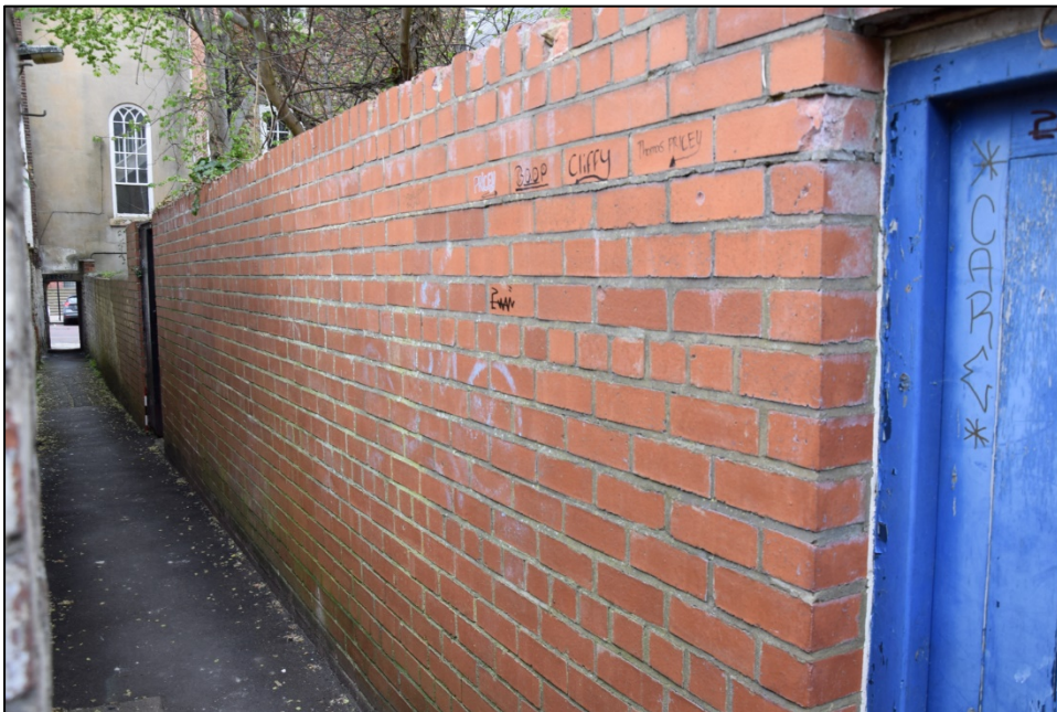
Photograph 72: Wall B, east face. Recent brickwork south of the gate to the Cottage
