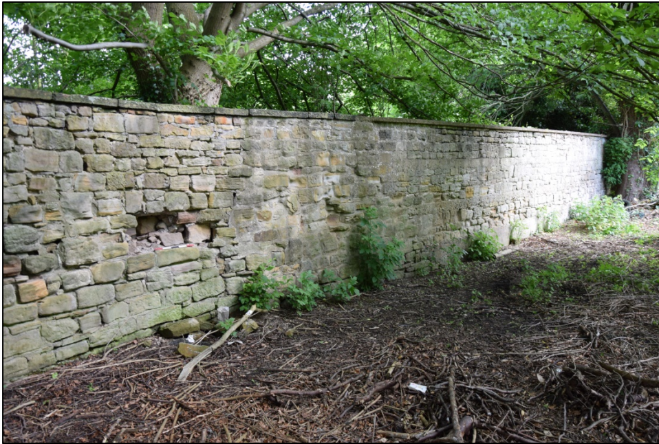
Photograph 127: Wall K, west face. The tree at the far end of this view marks the beginning of the overgrown section
