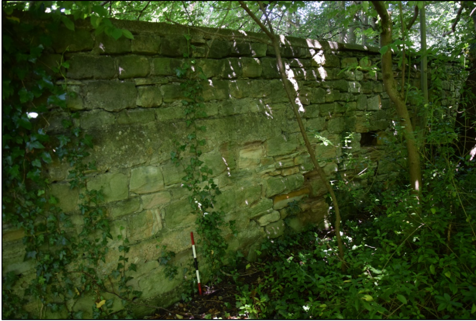
Photograph 133: Wall K, east face. Substantial concrete slabs in the wall match those on the other side (Photo 128)
