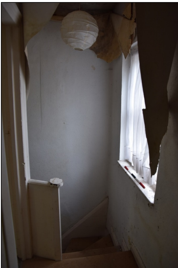
Photograph 28: The winders at the head of the stairs cut into the landing [5] outside the door to bedroom [6]
