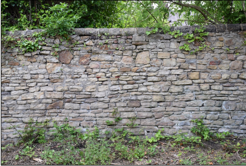
Photograph 89: Wall D, north face. Detail of the masonry, which is more irregular in the upper part of the face
