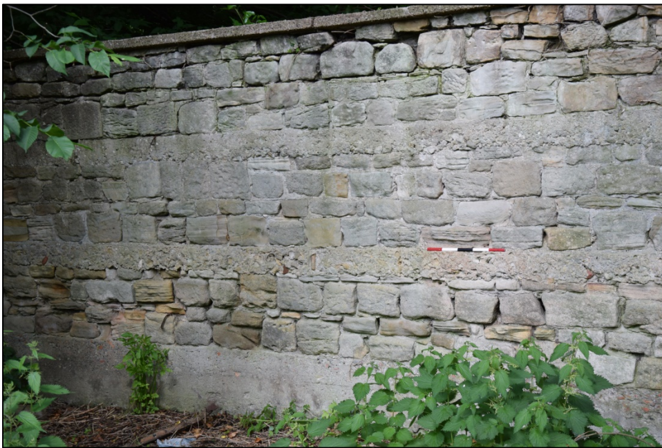
Photograph 128: Wall K, west face. This section has a deep concrete footing course and bands of concrete higher up; these are also visible in the opposite face
