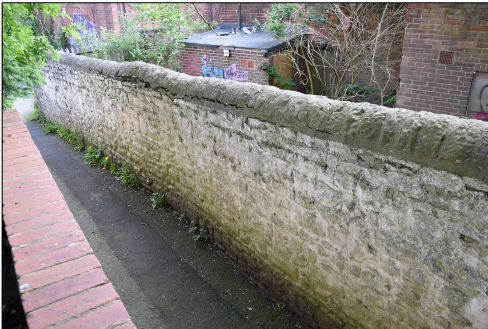
Photograph 74: Wall C, west face. This painted rubble masonry with rounded copings runs almost as far south as Vennel Cottage
