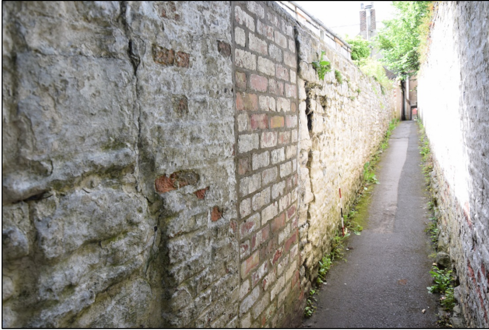
Photograph 77: Wall C, west face. The older middle gate near the north end of the temporary building. The masonry beyond the gate is the same as that seen in Photos 73-76
