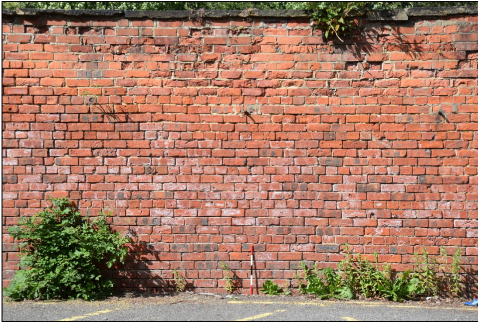
Photograph 121: Wall J, south face. Detail of the brickwork. Two small iron pegs, a little over halfway up, are the only trace of a glasshouse that stood here in the early 20th century
