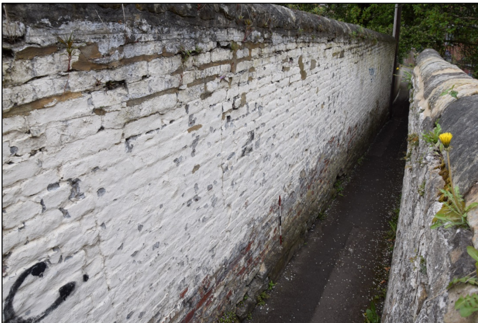
Photograph 68: Wall B, east face. The centre and north of the old building. A blocked window shows as two straight joints, left of centre
