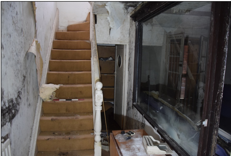
Photograph 22: The staircase hall 2, seen from the south. The thinness of the glazed partition can be seen here
