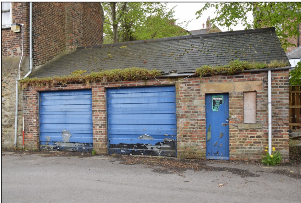
Photograph 34: The north face of the garage block. Modern brickwork can be seen above and between the steel doors
