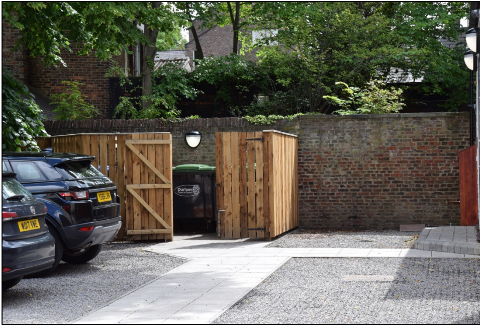
Photograph 107: Wall F, west face. This is the retaining wall for the garden outside Vennel Cottage
