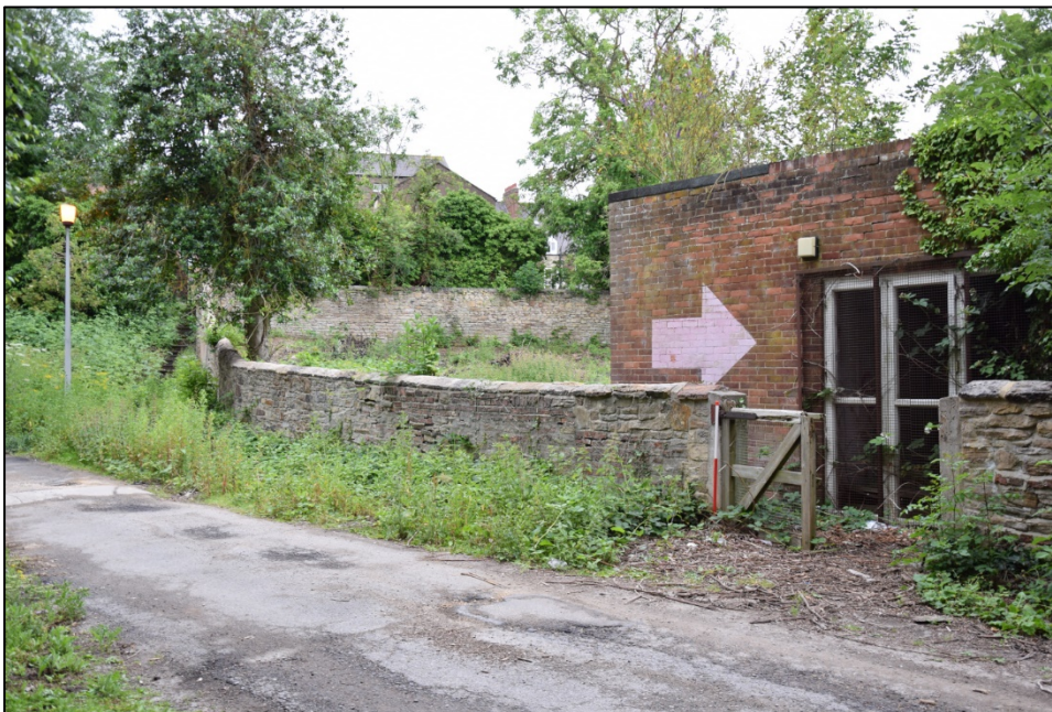
Photograph 44: The east end of the nursery building and walls D and E. A view looking south-west
