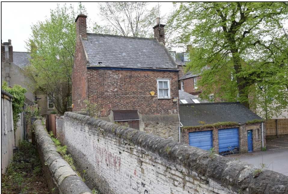
Photograph 70: Wall B, east face. The centre and south end of the old building, with Vennel Cottage behind
