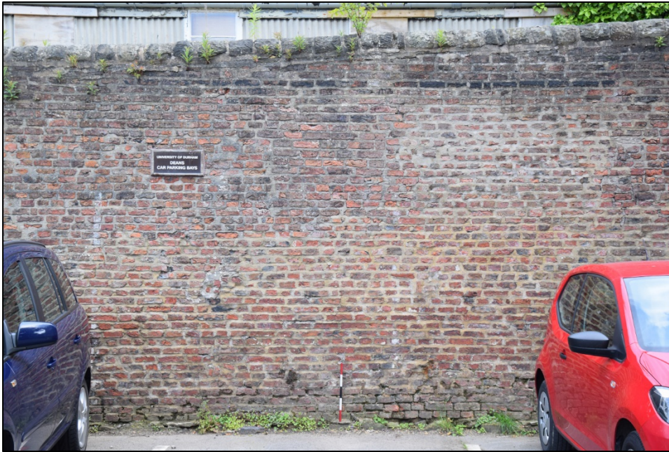
Photograph 61: Wall B, west face. Another blocked window is visible in the middle of this view
