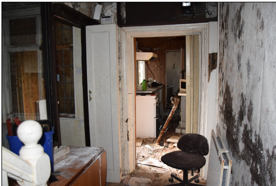
Photograph 24 (below): A view from the staircase into the kitchen [3]. The central opening, which was the original entrance to the building, has been fitted with a plastic concertina door
