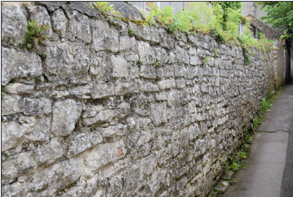
Photograph 78: Wall C, west face. The south end of the wall has a pronounced lean to the east
