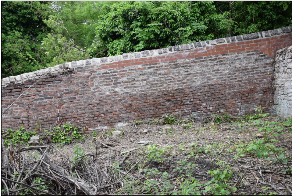
Photograph 97: Wall E, west face. Old and modern brick near the junction with wall D
