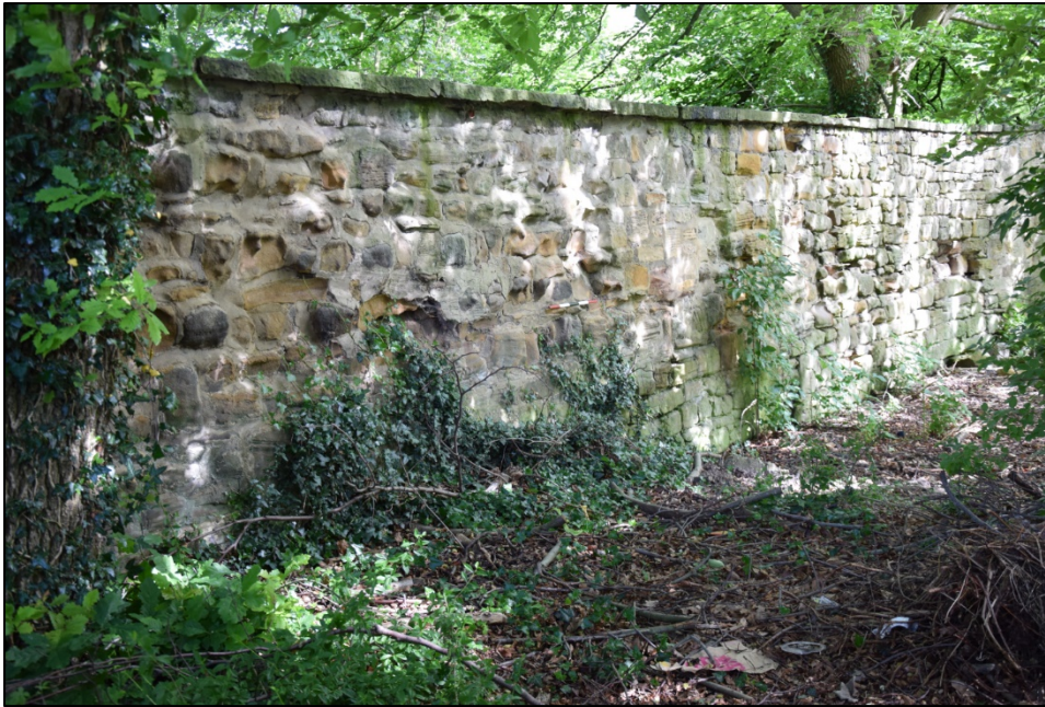
Photograph 125: Wall K, west face. The wooded area south of the car park
