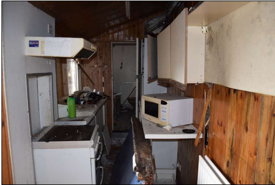
Photograph 25: The kitchen [3] seen from the north end. Because of the narrowness of the lean-to, the cooker is recessed into the wall and the sink extends into the projecting window. The far door leads up into the bathroom [4]
