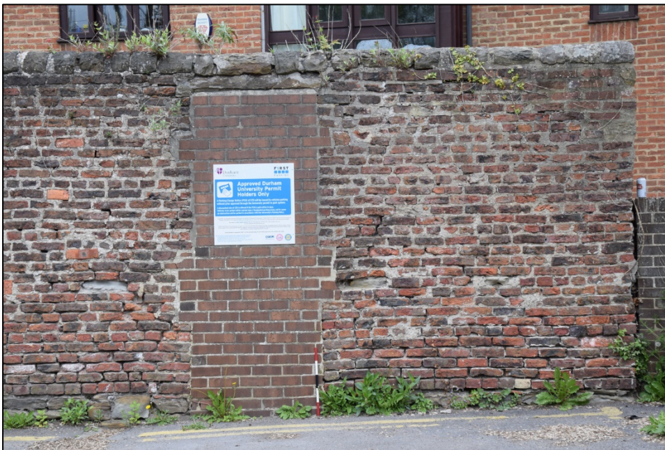
Photograph 54: Detail of the masonry on the south side of wall A, with modern bricks in the blocked door
