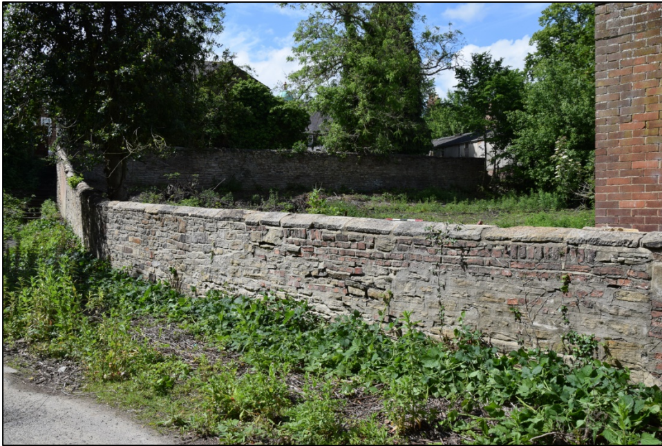
Photograph 99: Wall E, east face. This general view looking south-west shows the change in alignment near the bottom of the slope
