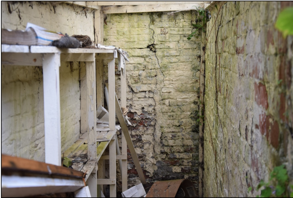
Photograph 17: Looking north along the gap between the cottage and the vennel wall. The straight joint in the far wall can also be seen in Photo 10, above
