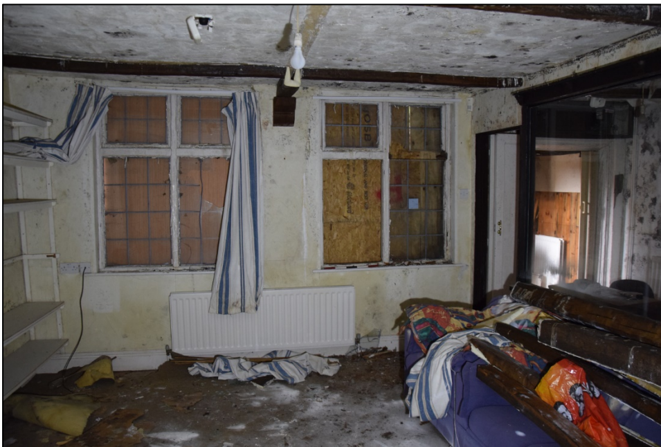
Photograph 18: A view looking south-west across the ground floor room 1 in Vennel Cottage. The partition at the right and the expanded polystyrene ceiling beams are modern additions
