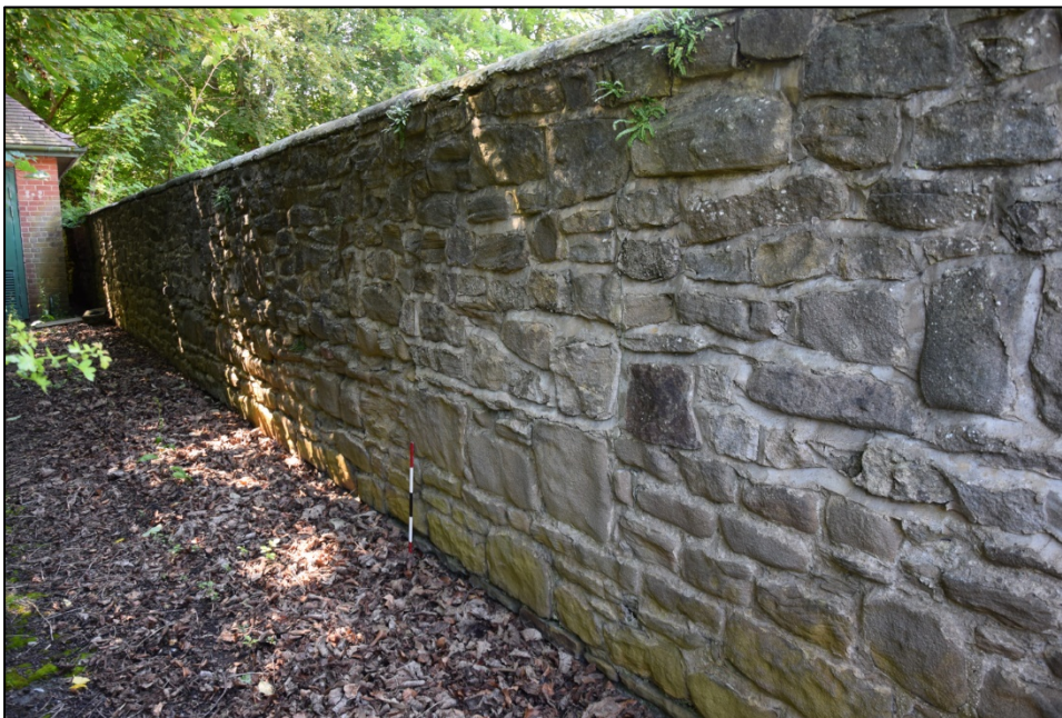
Photograph 130: Wall K, east face. Once again, there is a stone face on the outside of a wall seen as brick from inside the former garden
