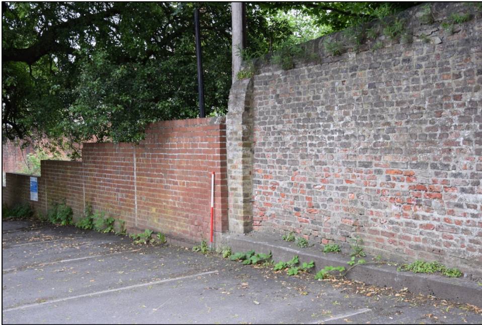
Photograph 58: Wall B, west face. A step and the stub of a wall separate modern fabric from the older brickwork of the building shown on the 1861 map. The concrete plinth course is at about the same level as the visible stone foundation on the opposite face (Photo 67, below)
