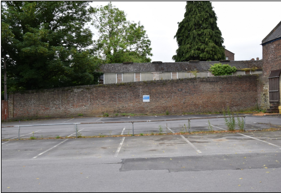
Photograph 59: Wall B, west face. This is what remains of the east face of the early 19th-century building
