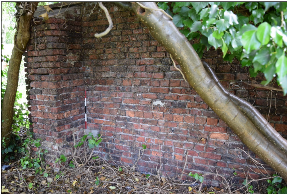
Photograph 112: Wall H, north face. The slightly larger buttress at the east end was originally beside a gate to the lower garden
