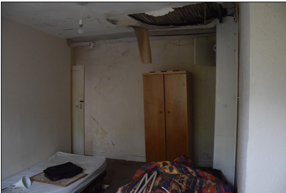
Photograph 32: The north end of bedroom [7], showing ceiling damage caused by a leaky roof. Plaster behind the wardrobe covers the site of the blocked window shown in Photo 11
