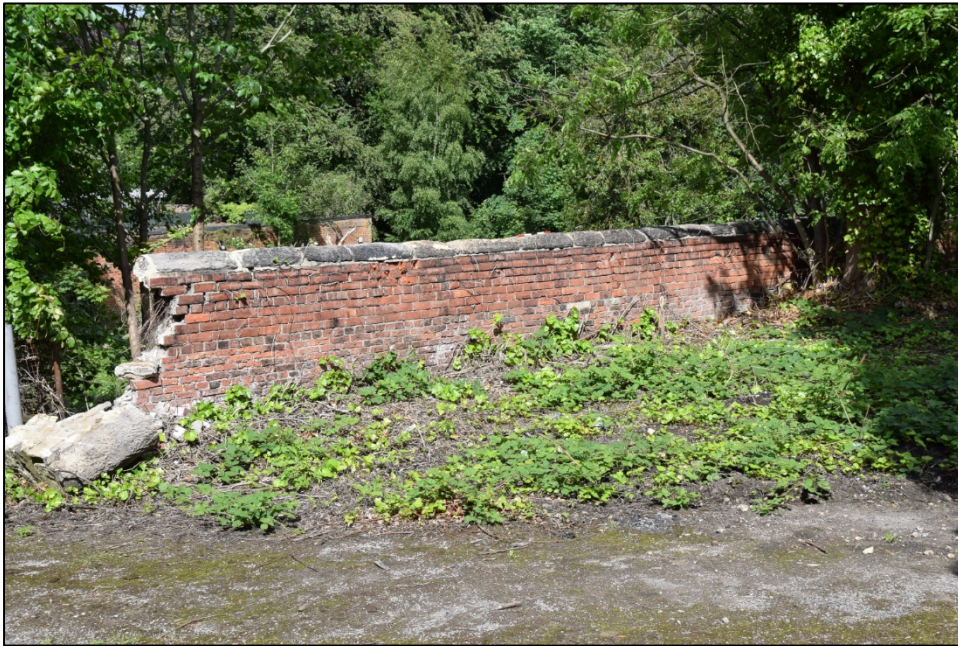
Photograph 90: Wall D, south face. As elsewhere, the inner face is brick. The damaged west end adjoins a later gateway cut through the wall at the north-east corner of the temporary building
