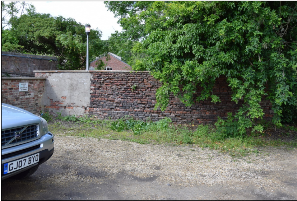
Photograph 113: Wall H, south face. The 1816 map shows a structure at the left-hand end, but no sign of it can be seen
