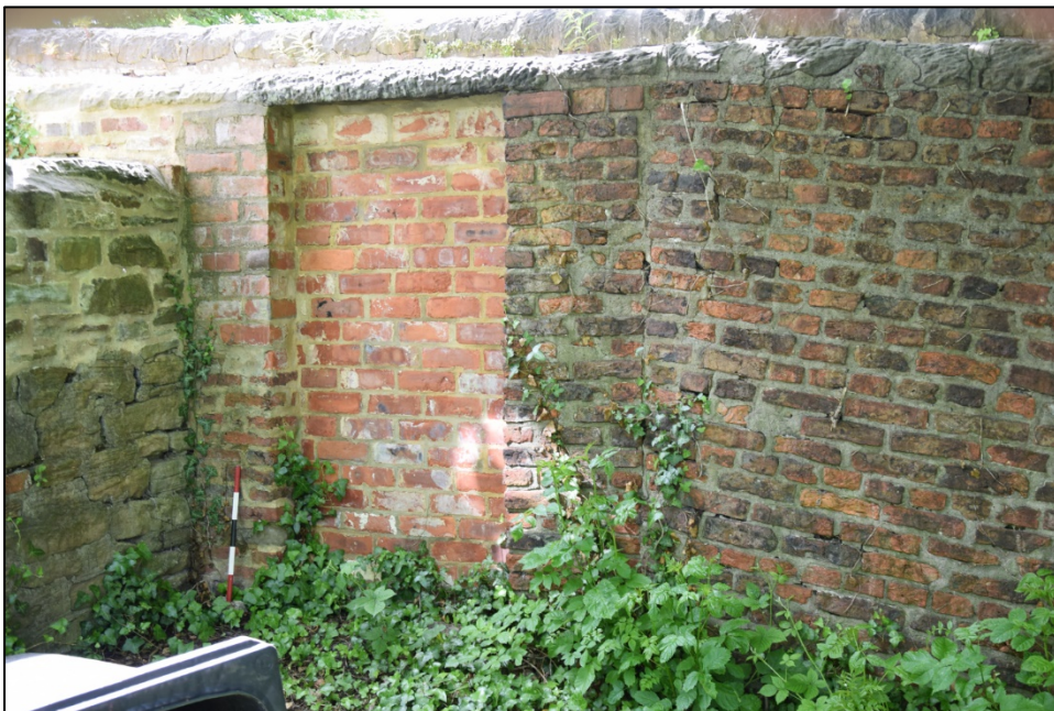
Photograph 84: Wall C, east face. The middle gate and the east end of wall D
