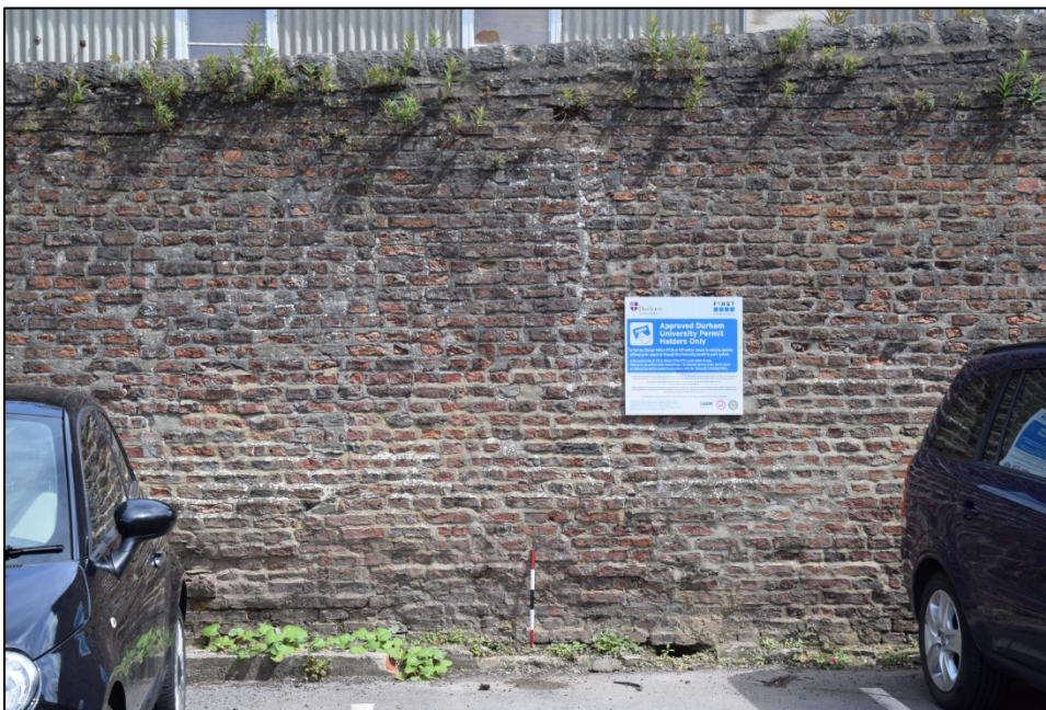
Photograph 60: Wall B, west face. A blocked opening can be seen to the left of the notice
