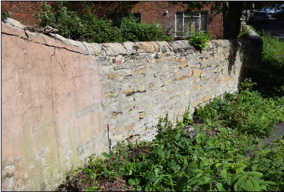
Photograph 103: Wall E, east face. The wall on the slope has an area of pink plaster
