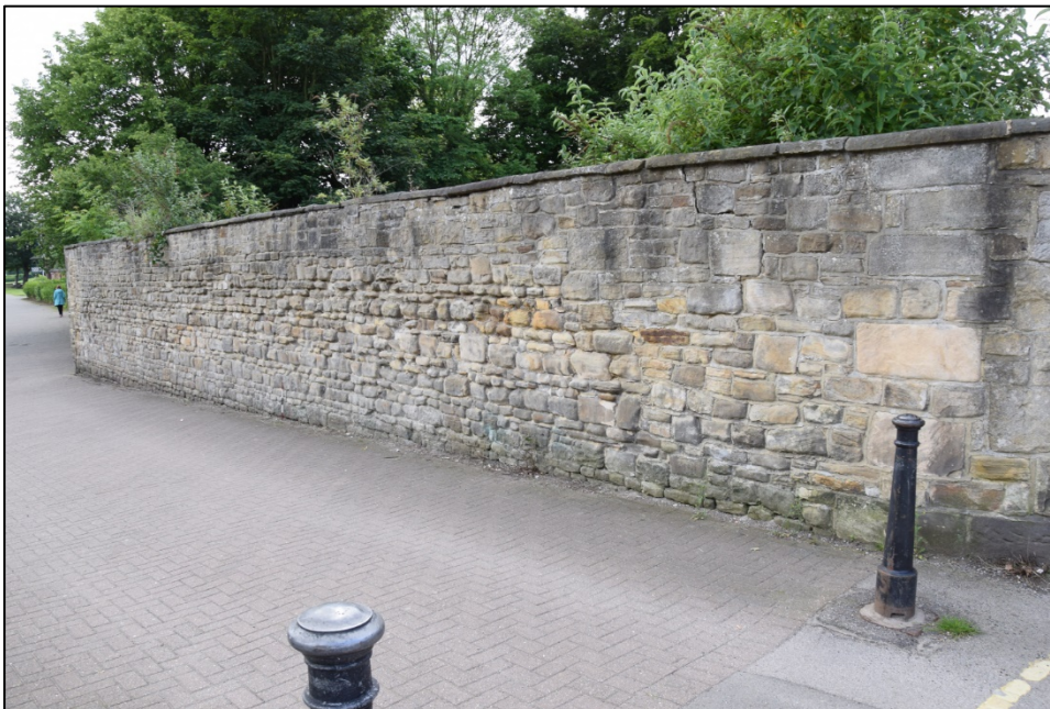
Photograph 118: Wall J, north face. Note the difference between the upper courses and the rest of the face
