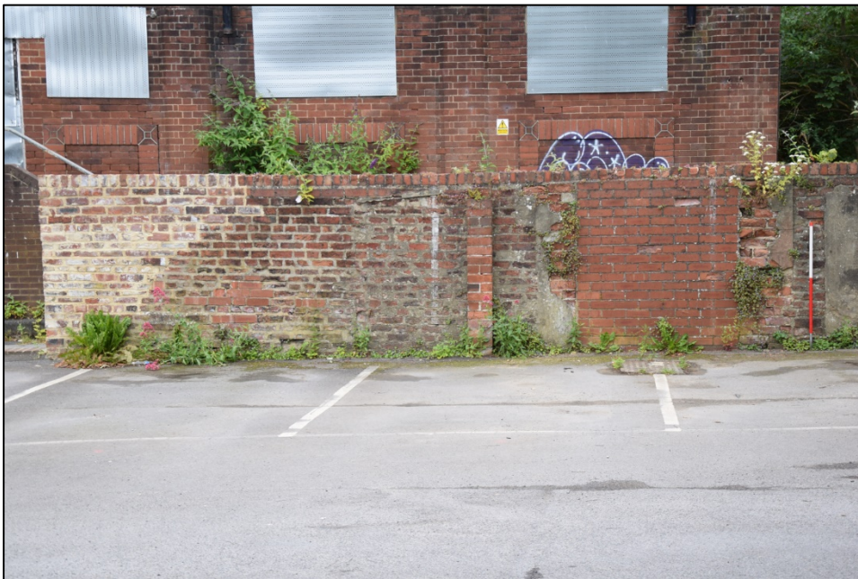
Photograph 56: Wall B, west face. Recent repairs and a blocked gate at the north end
