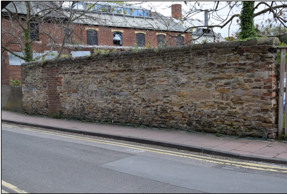
Photograph 51: Wall A from the north-west. Note the discontinuous line of bricks about 0.6m from the top of the face
