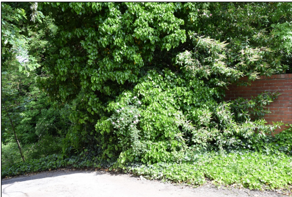
Photograph 116: Wall I, south face. The old wall is completely hidden; the adjoining section is all modern brickwork
