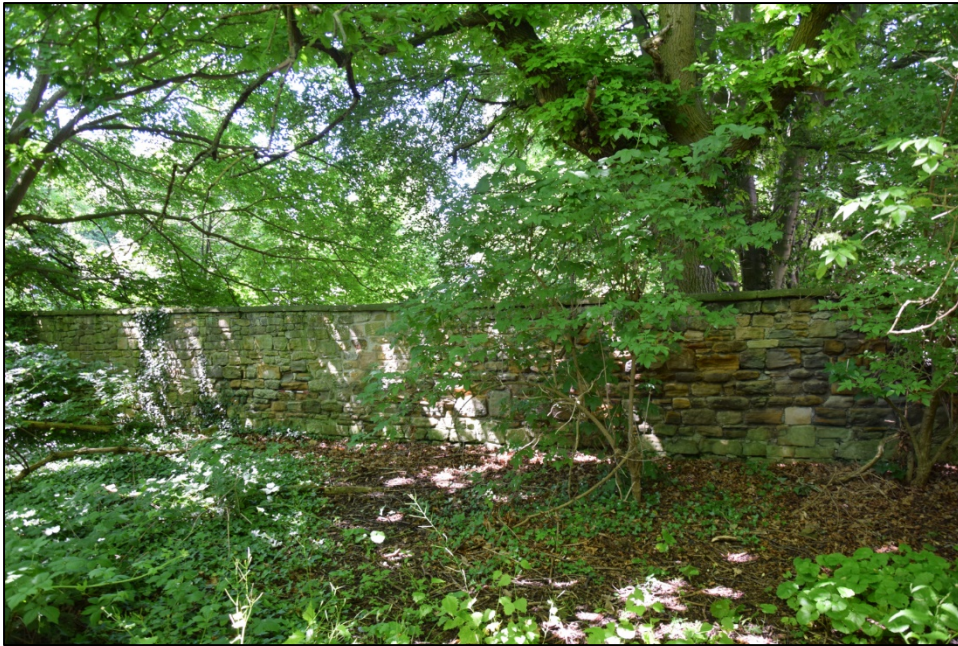
Photograph 131: Wall K, east face. The masonry near the centre of the wooded area at the foot of the slope is similar to that on the opposite face, seen in Photo 126
