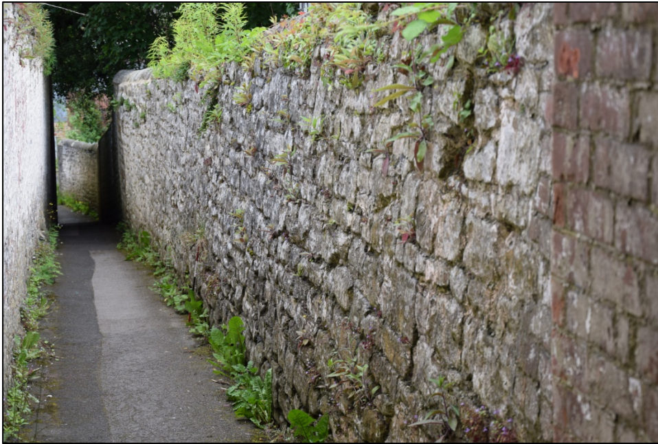
Photograph 79: Wall C, west face. The junction of the leaning stone wall and later brick
