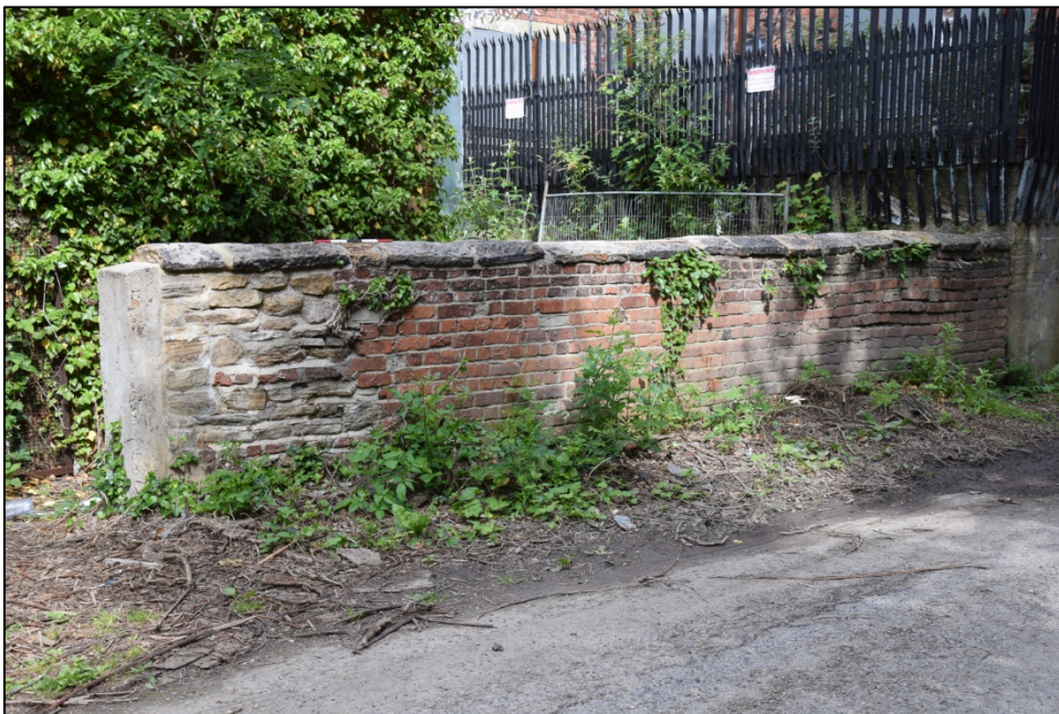
Photograph 100: Wall E, east face. A short section between the gate to the former nursery and the corner of the baths
