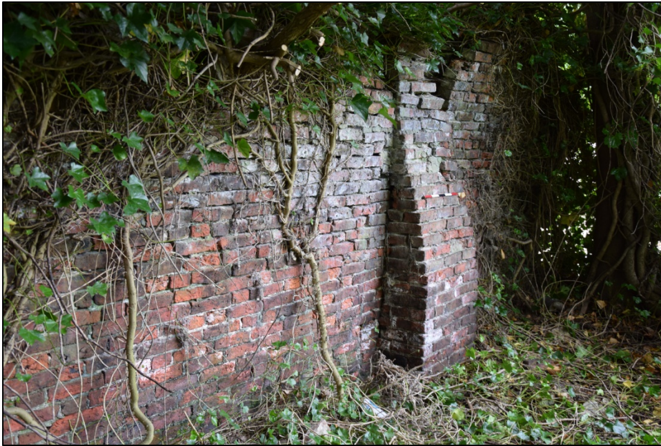
Photograph 115: Wall I, north face. This buttress is different from those on the other side of the old gate. The outer face of brickwork beside it is in a dangerous state
