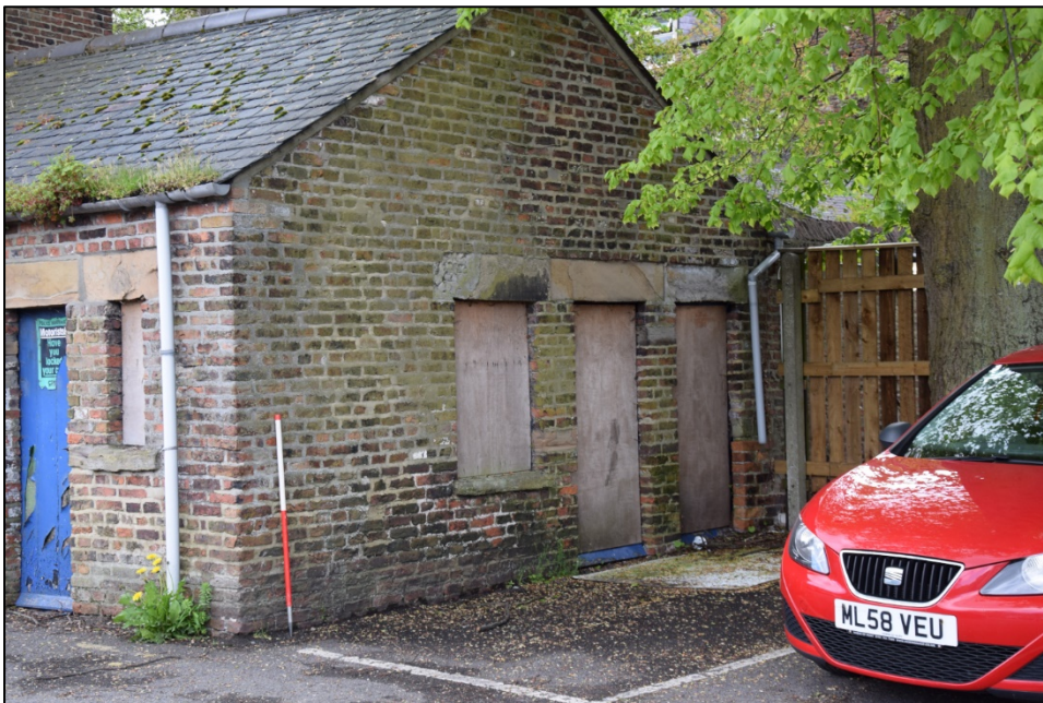
Photograph 36: The west end of the building was inaccessible for this survey. The door at the far left once opened into a small toilet
