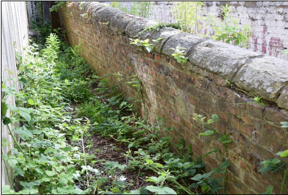
Photograph 85: Wall C, east face. Looking south-west along a narrow gap between the vennel and the temporary building. The ground level south of wall D is higher than that to the north and in the vennel
