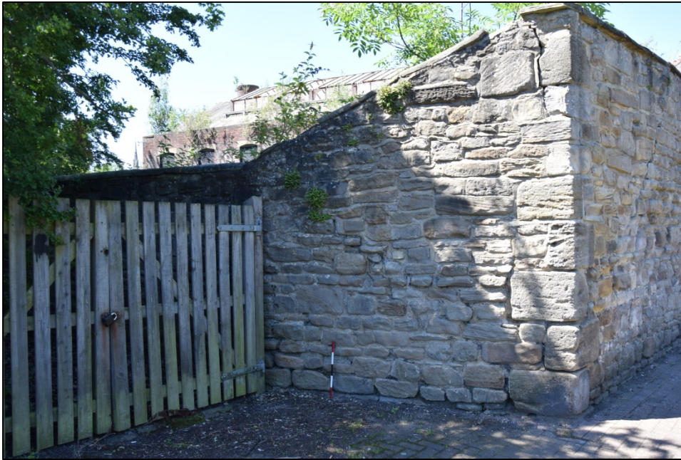
Photograph 129: Wall K, east face. The fence is the compound for the electricity substation
