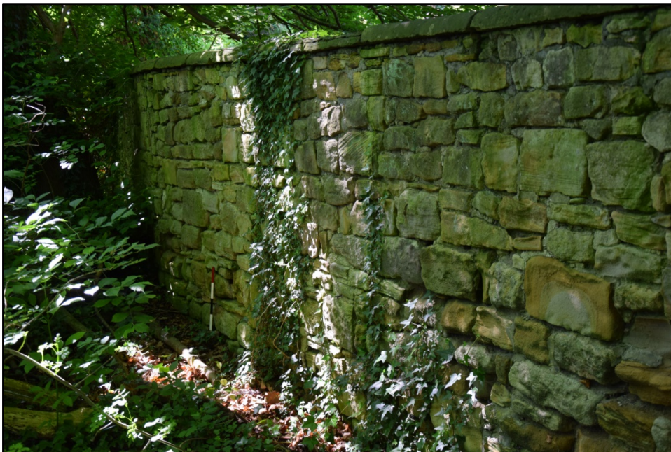
Photograph 132: Wall K, east face. A view looking south-west near the end of the unobscured wall
