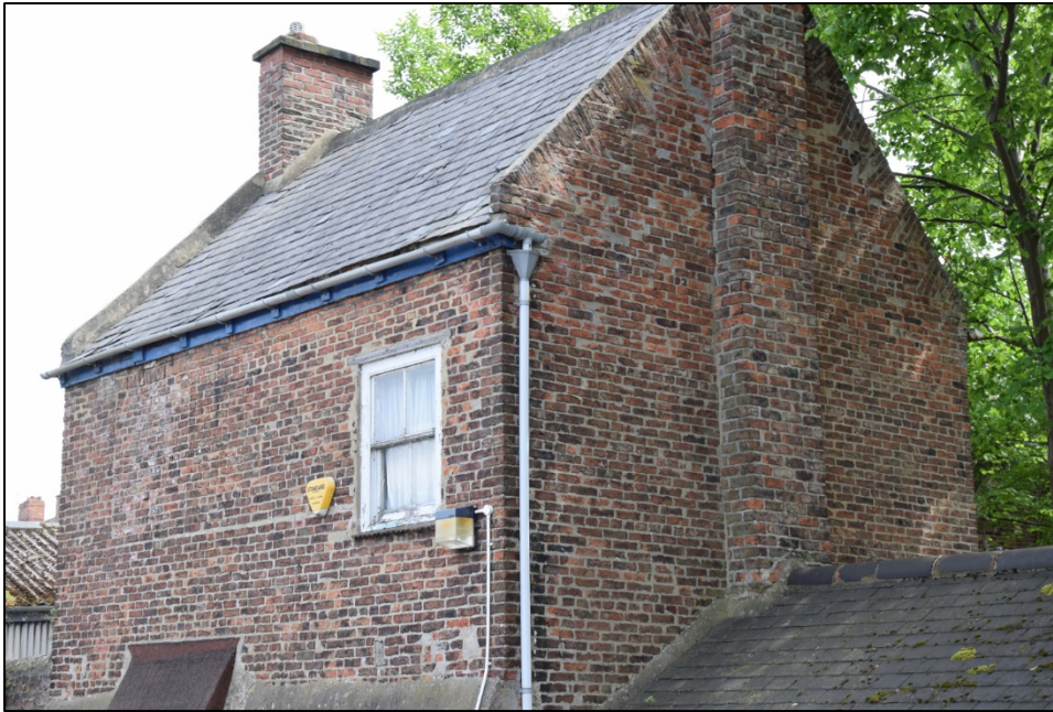
Photograph 13: The west gable has similar tumbled-in brickwork, but here the chimney projects from the wall
