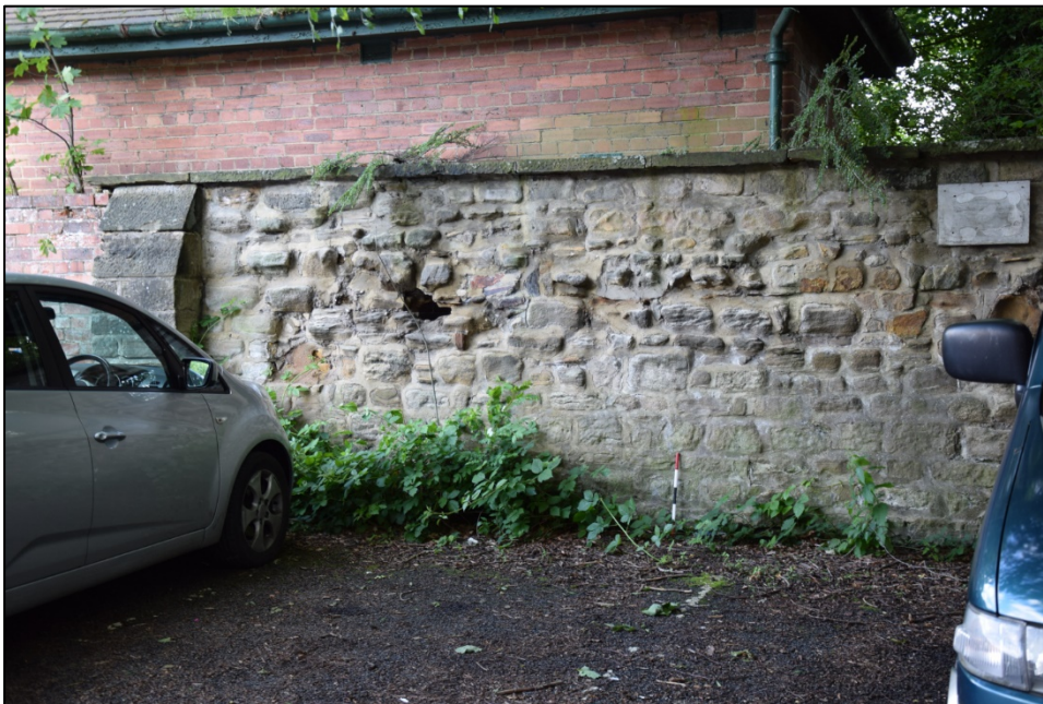
Photograph 124: Wall K, west face. The stone wall with the electricity substation behind it. The stone has decayed to the point that there is a hole through the wall, just right of the grey car
