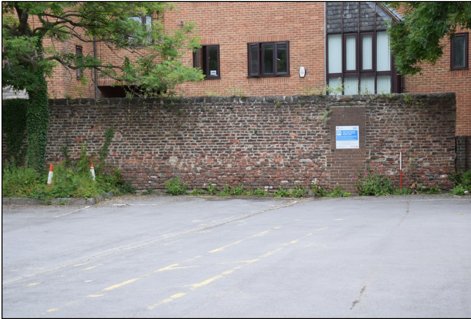
Photograph 53: The south face of wall A is all brick and formerly faced onto a large garden
