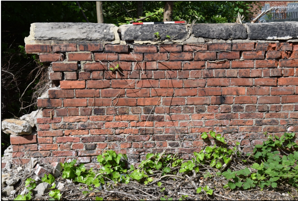
Photograph 91: Wall D, north face. Detail showing the two different types of brickwork. Both use common or English Garden Wall bond, with three courses of stretchers to one of headers
