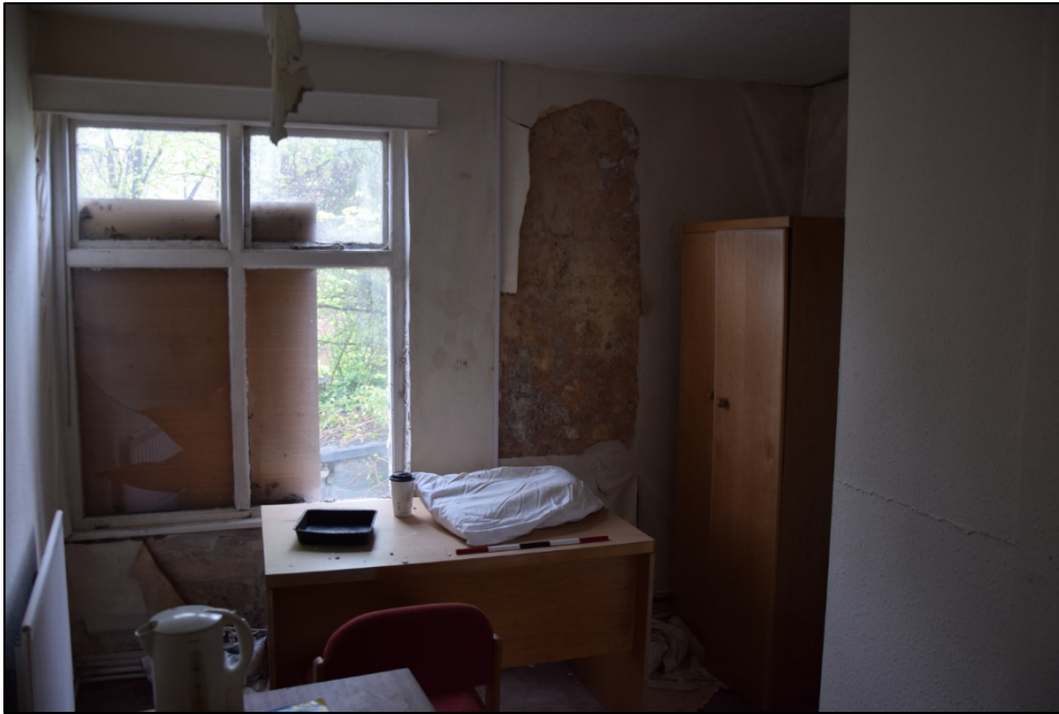
Photograph 29: A view looking south into the west bedroom [6]. The simple windows are the same as those on the ground floor
