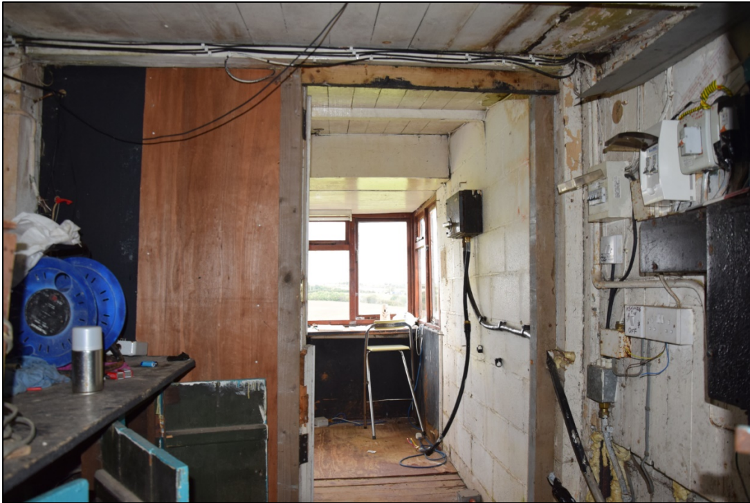
Photograph 47: A view looking west from store room [21] into the control room. A ladder to the upper room is out of shot on the right-hand wall
