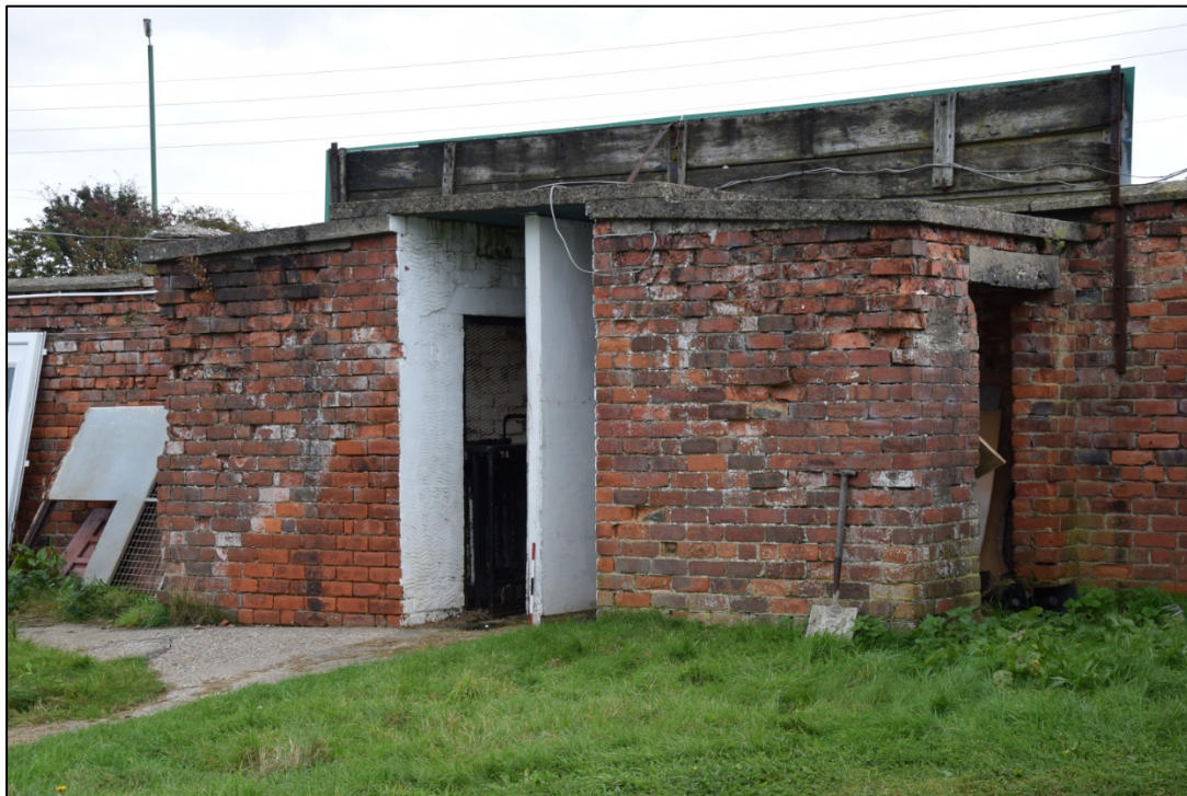
Photograph 62: The turnstile blocks [31, 32] at either side of the old entrance. The white internal wall is a recent addition
