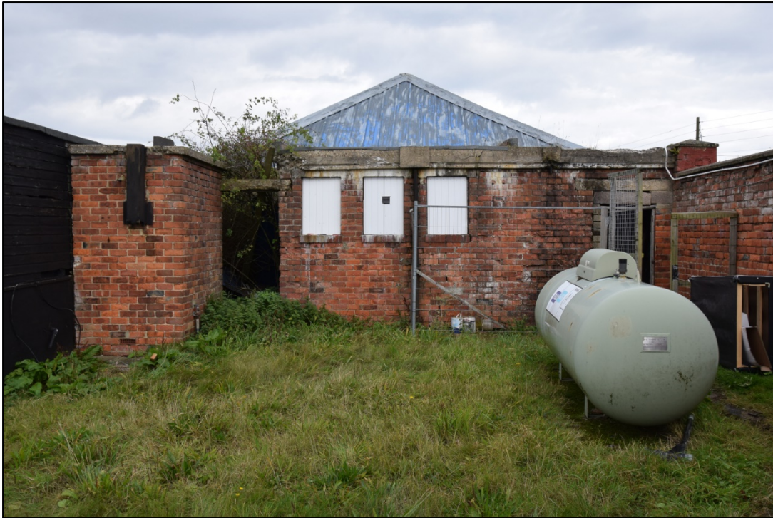
Photograph 67: The south end of the building. Boiler house [29] is at the left, with windows to toilets [7] in the middle and the store room [30] to the right
