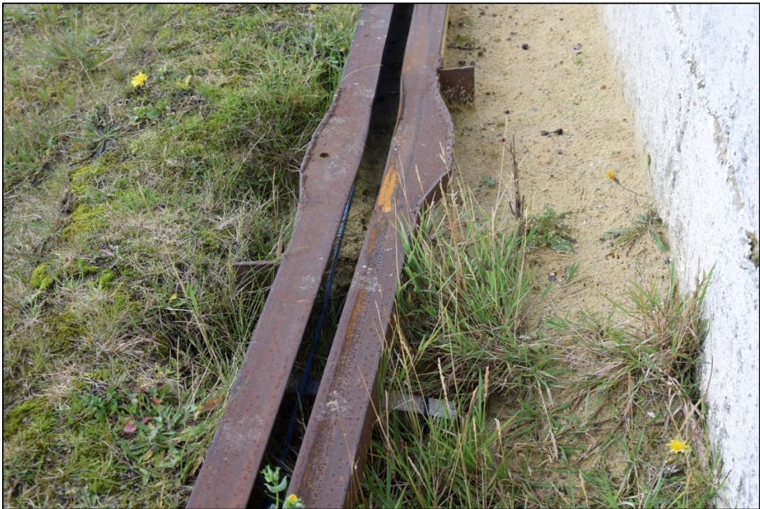
Photograph 10: Detail of the hare track showing a typical welded joint between straight sections and evidence of wear. The blue cable (centre) draws the hare along
