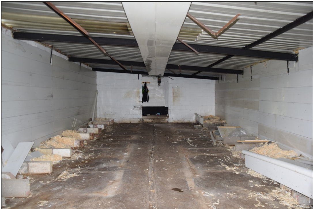
Photograph 16: Interior of the kennel building, with the bases of the boxes at either side
