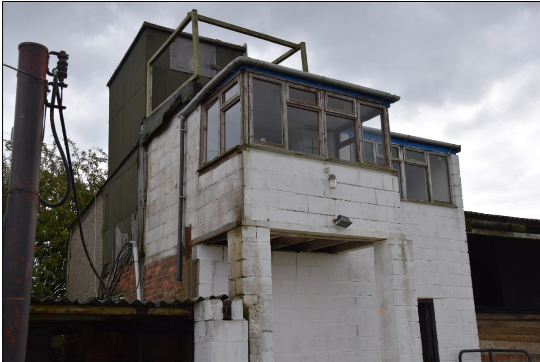
Photograph 49: The windows of the control room [20] and vet's room [19], with the felt-covered upper room and the open platform above
