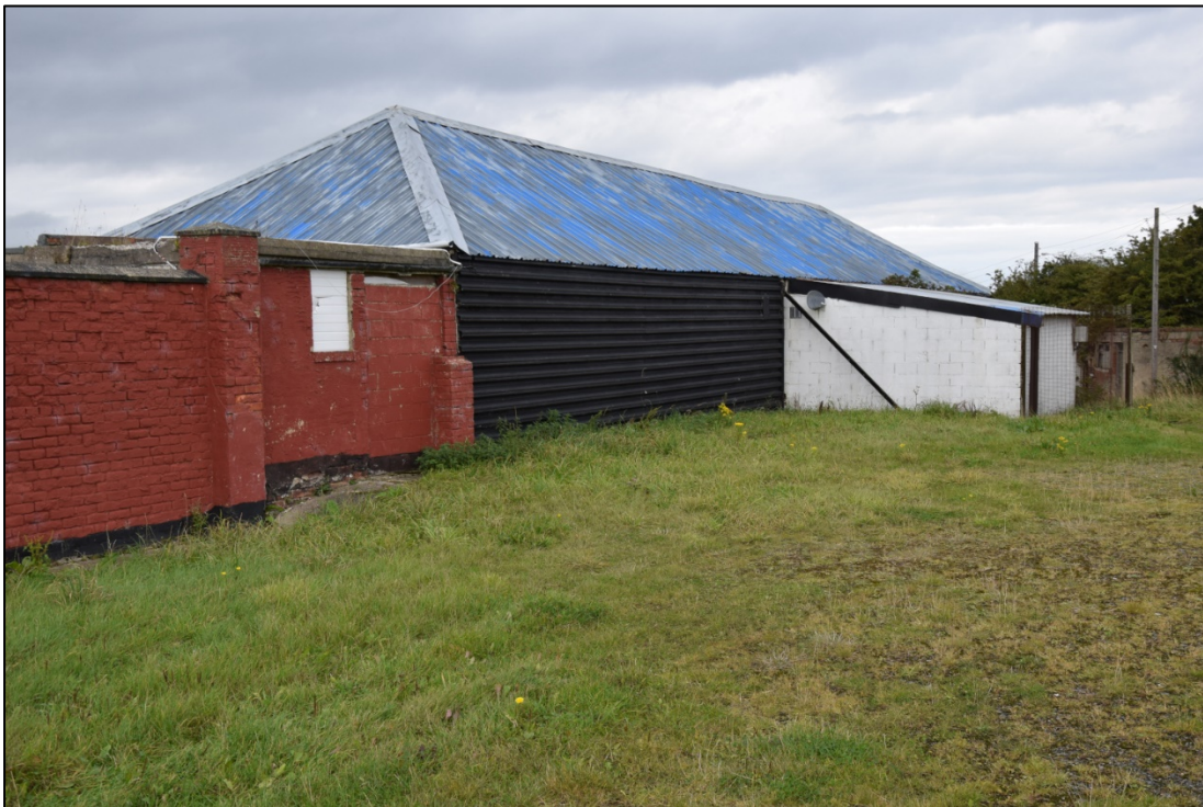
Photograph 68: The east face of the building, with blocked openings to store [30] left of centre and the white-painted cellar [9] at the right
