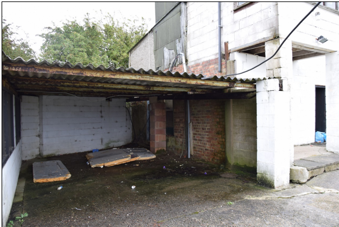
Photograph 50: The open shed [22]. Doors partly hidden by the central pillar lead to the old betting kiosk [25] and the rear store [26]
