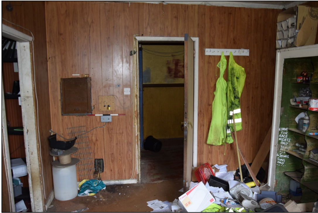
Photograph 39: The west wall of the workshop, with the blocked hatch from lobby [12]
