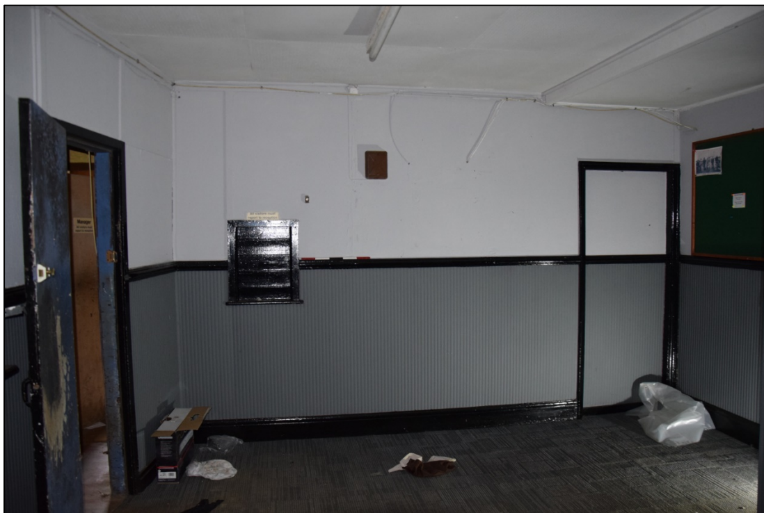
Photograph 36: The entrance lobby [12] that opens onto the terraces has a blocked door and hatch in its east wall
