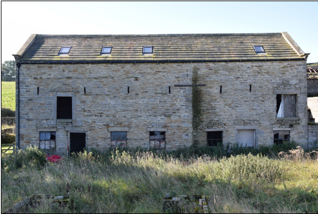
Photograph 9: The division between the two parts of building 1 is very clear in this view of the north face. The open stonework above the openings is the result of repair of the door and window lintels
