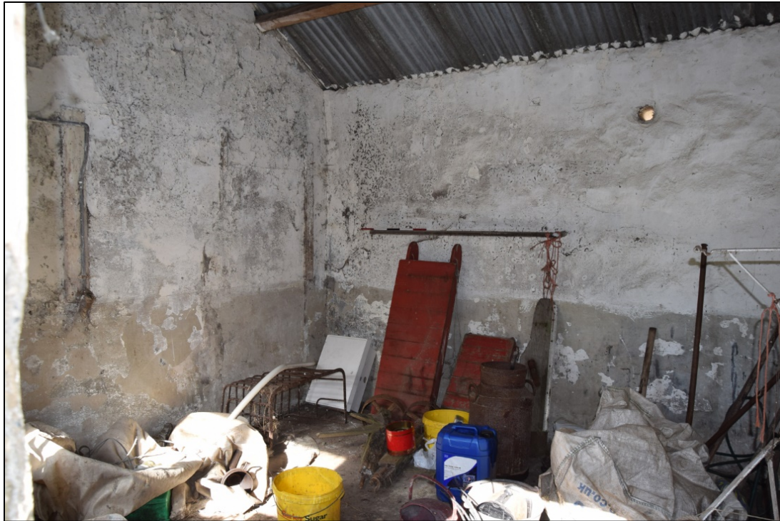
Photograph 67: The interior of the west room has traces of the old door near the far corner
