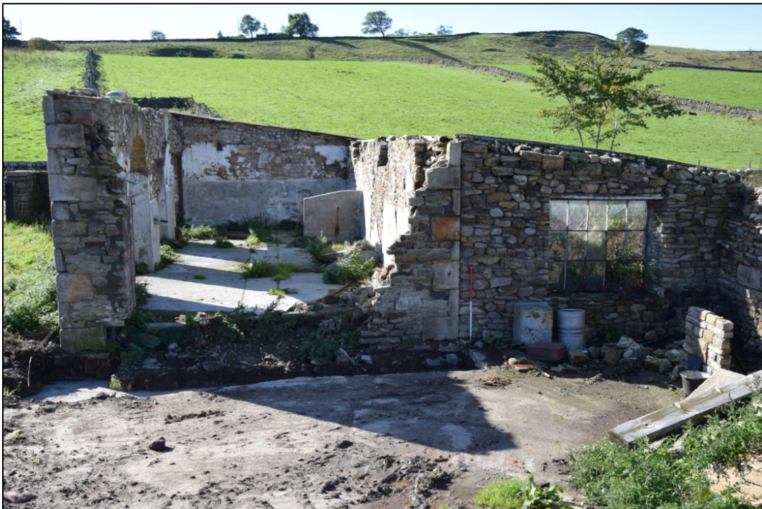
Photograph 50: Most of the north end of the building has been demolished. The wall with the window is what remains of an adjoining single-storey building
