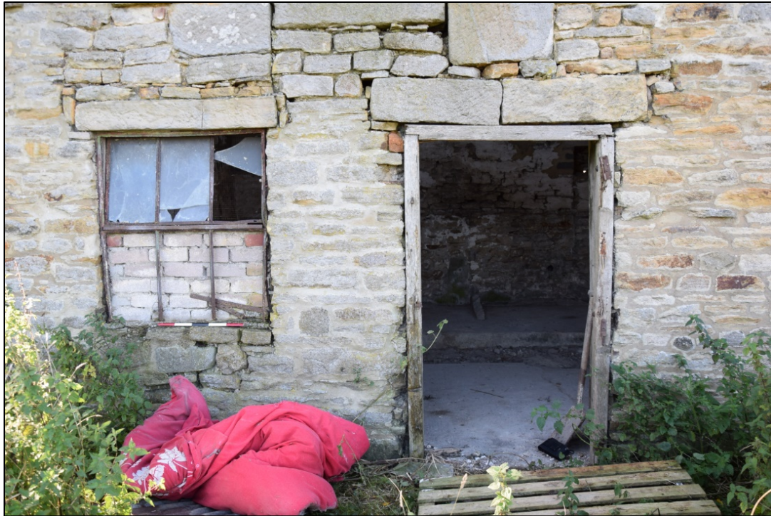
Photograph 11: Detail of the door and window at the east end of the north face. The loading door above has been altered
