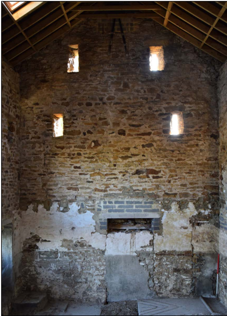
Photograph 17 (left): The east end of building 1, showing the wall finishes restricted to the byre. There is no sign of a loft; the roof is new
