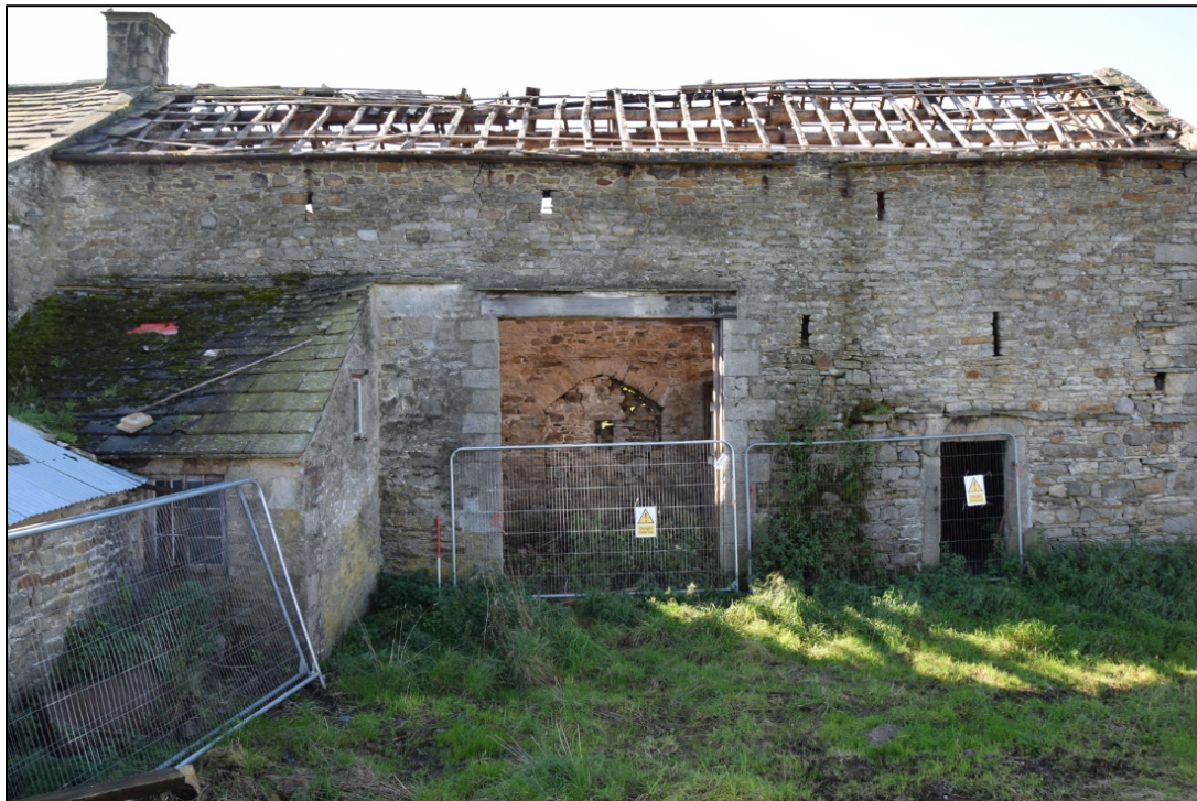
Photograph 28: The north face of building 2. Note the row of projecting throughs above the small door
