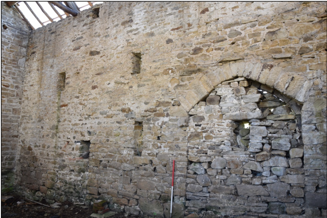
Photograph 40: The rebuilt south wall on the eastern part of the building. Note the change of masonry low down at the far corner
