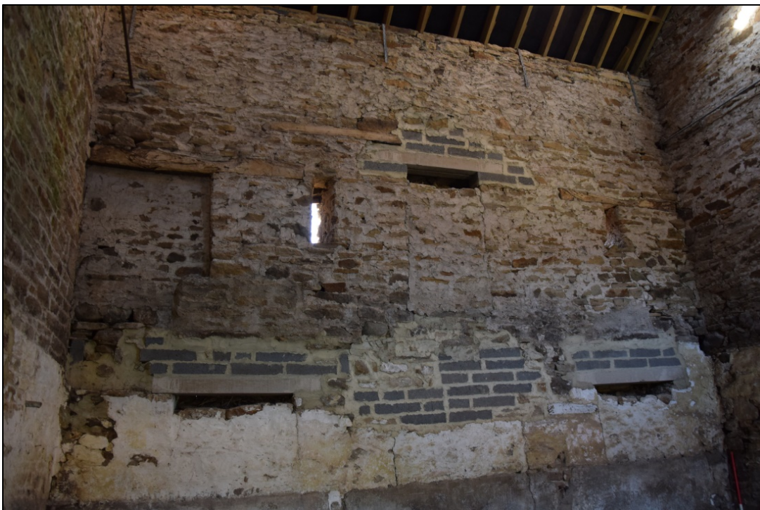
Photograph 22: Blocked openings, breathers and repairs in the upper floor of the south wall
