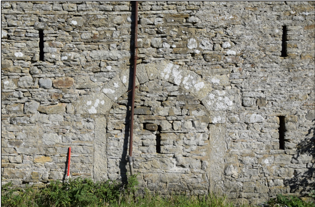
Photograph 33: Detail of the central door, with its unusual pointed arch. The break in the masonry runs diagonally above the right-hand side of the arch
