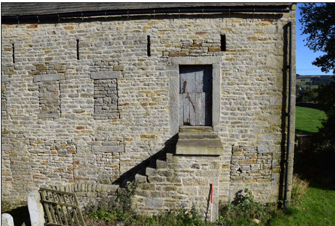
Photograph 6: The hay loft entrance near the south-east corner of building 1. Blocked doors can be seen to the right of the staircase and above the wooden gate
