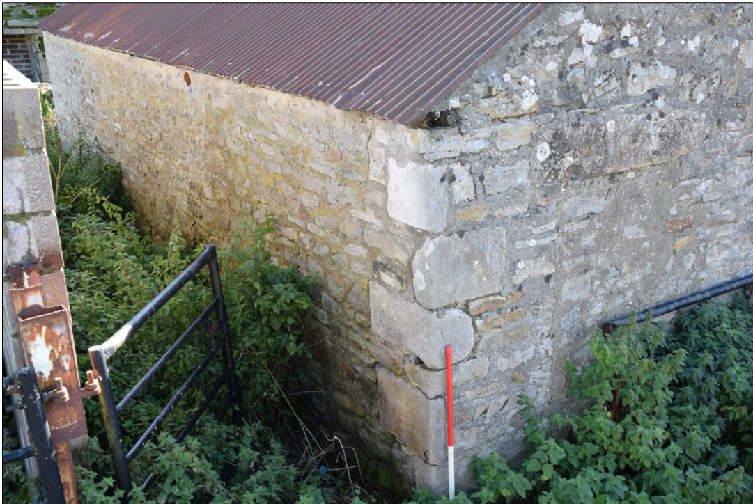
Photograph 66: The north-west corner of the shed, showing the blocked door (right of the scale) and the windowless north face
