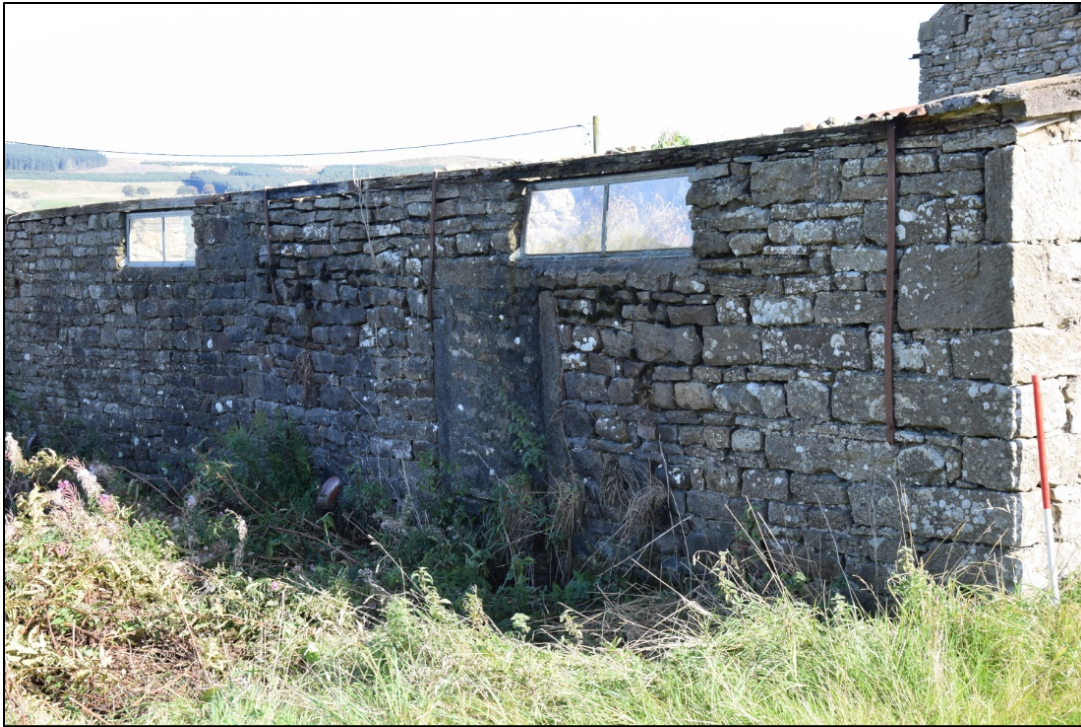
Photograph 51: The west face of building 4, with recent high windows above a blocked door
