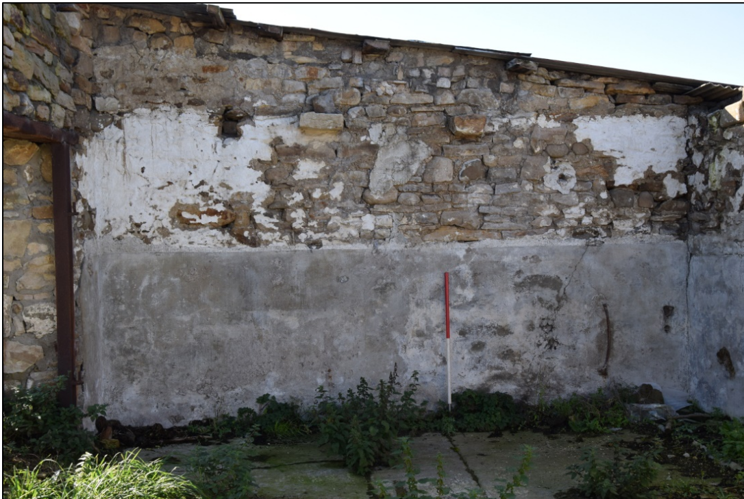
Photograph 62: Cement render on the south wall. The whitewash above indicates the line of the old ceiling
