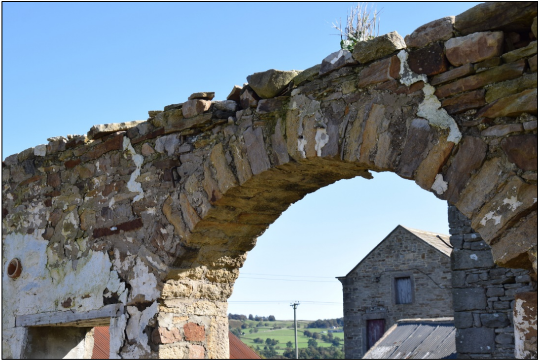
Photograph 61: The arched door is also a recent alteration. There are no traces of similar arches on the rest of the wall
