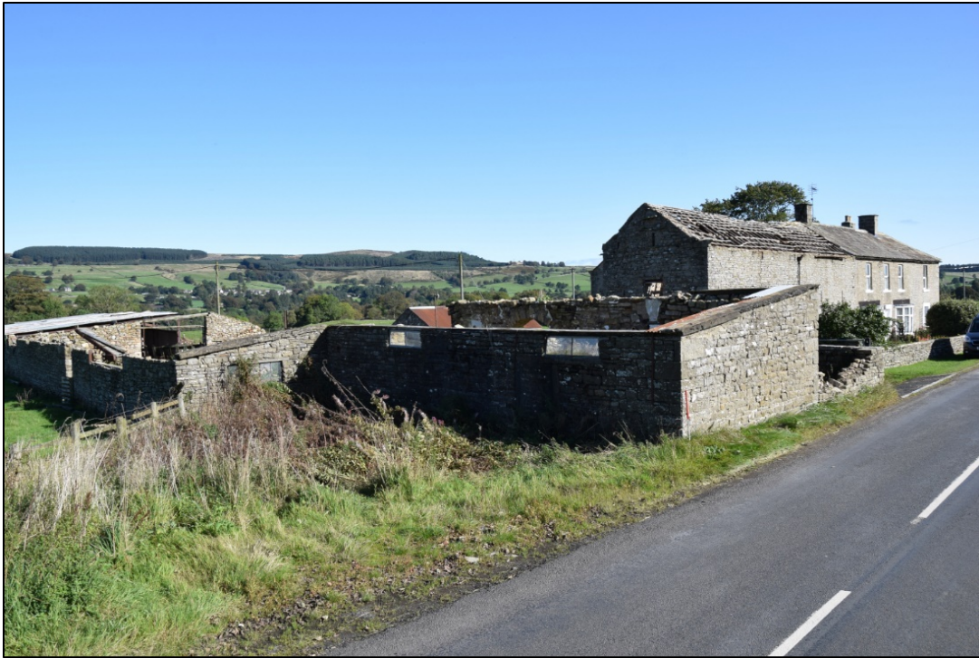
Photograph 3: The site from the south-west, with the truncated building 4 in the foreground
