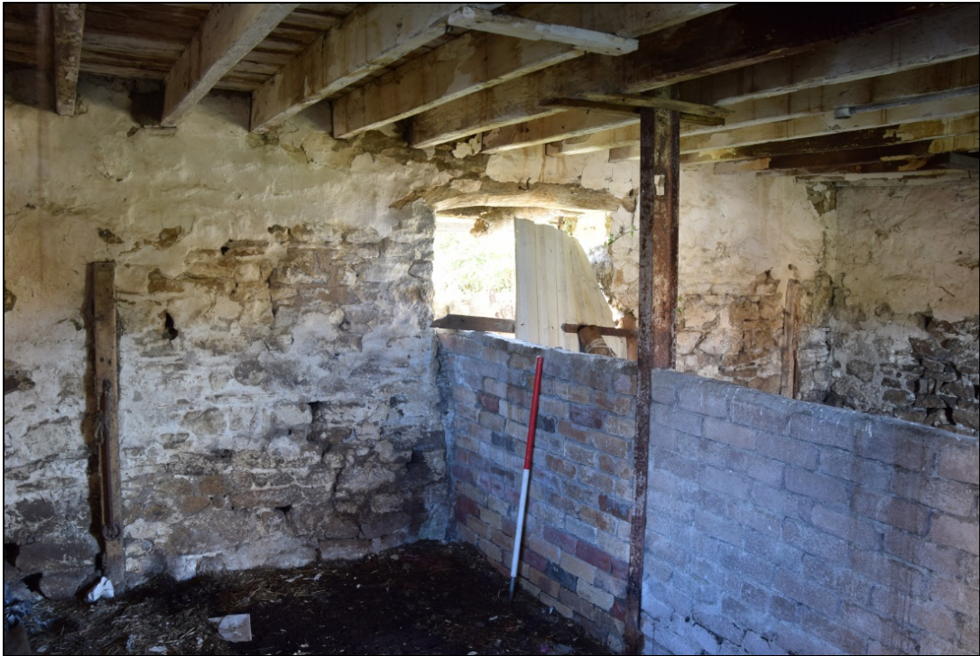
Photograph 39: This view, looking south-west across the byre, shows the old south door and a pair of tethering posts
