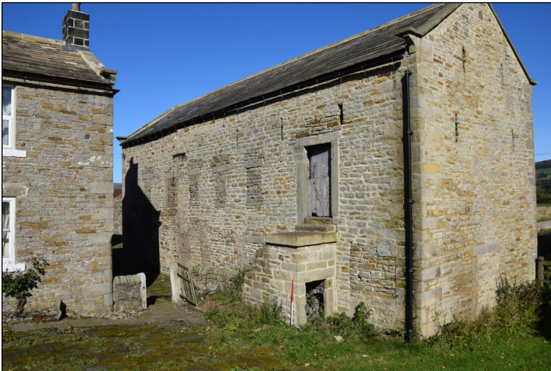
Photograph 4: Building 1. Note the placement of the blocked windows with reference to the floor height shown by the door. A dark line below the eaves, left of centre, is the iron strap that reinforces the junction between the older block and the extension at the far end
