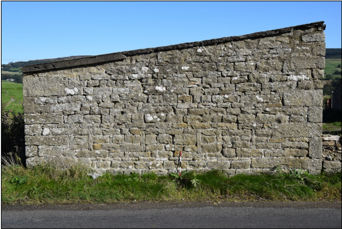
Photograph 53: Three blocked breather slits can be seen in the south end of the truncated building 4
