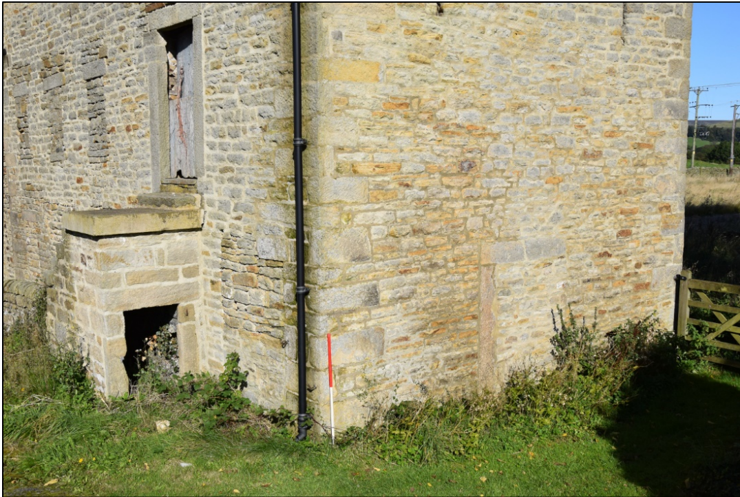
Photograph 5: The blocked opening at the east end of building 1. Recent repointing is apparent, as is the rebuilding of the stone staircase
