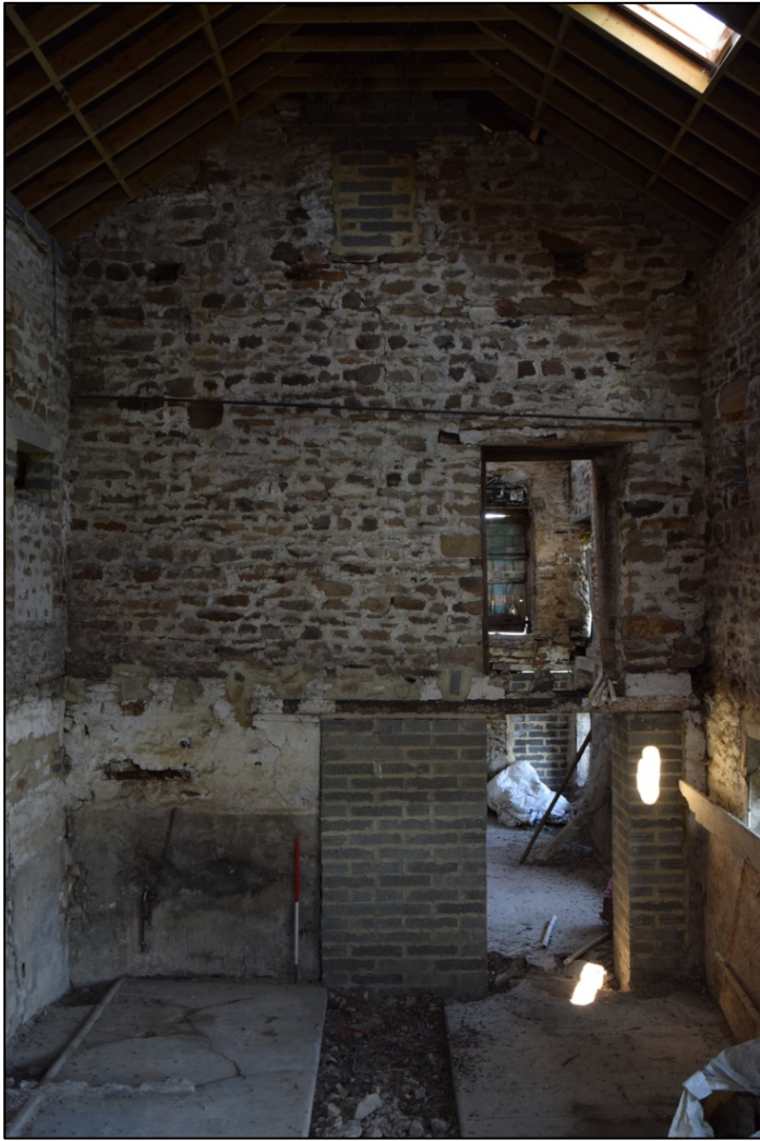
Photograph 19 (left): The old west end, now an internal wall, has been rebuilt at the base. The open door above would have been used for loading hay
