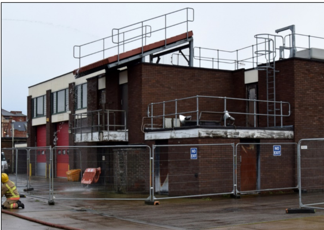
Photograph 4: Training rooms and roof at the south end of the ambulance building. Water can be seen running from the tiled roof; the ground-floor room right of centre is for smoke training
