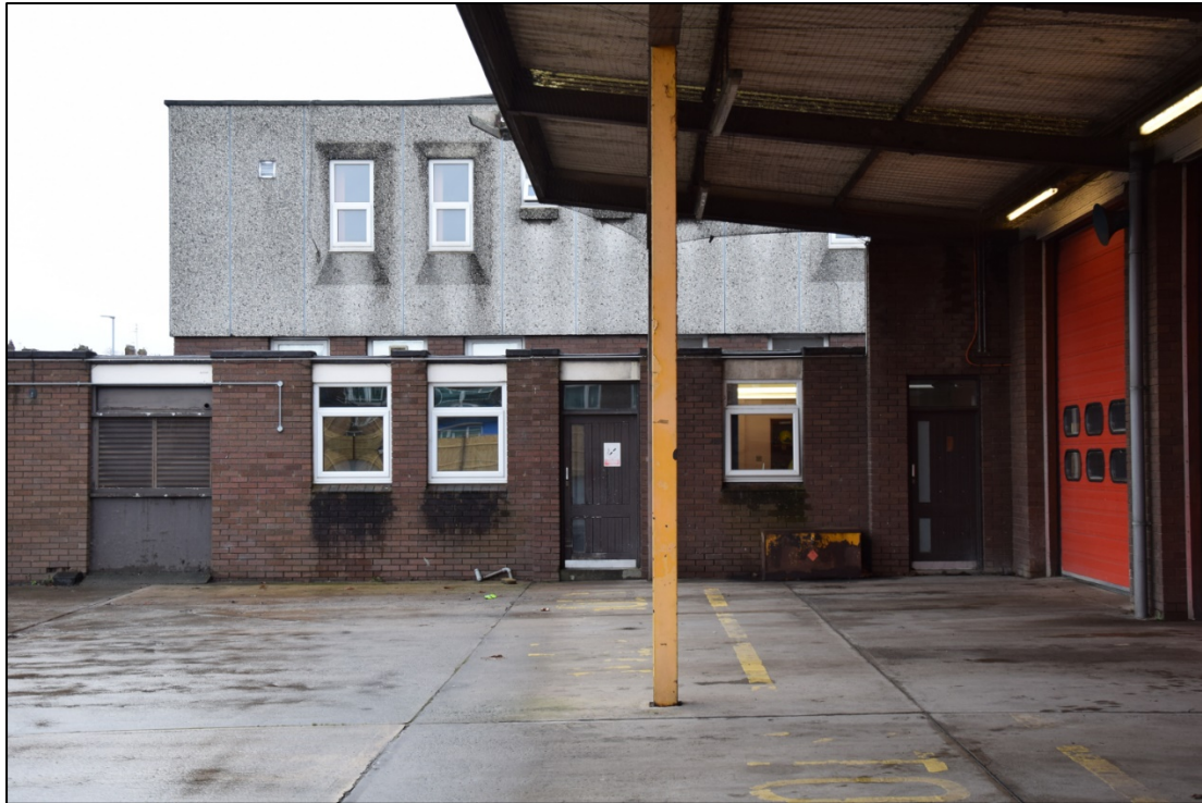
Photograph 13: The north face of the building seen from the canopied area at the back of the garage
