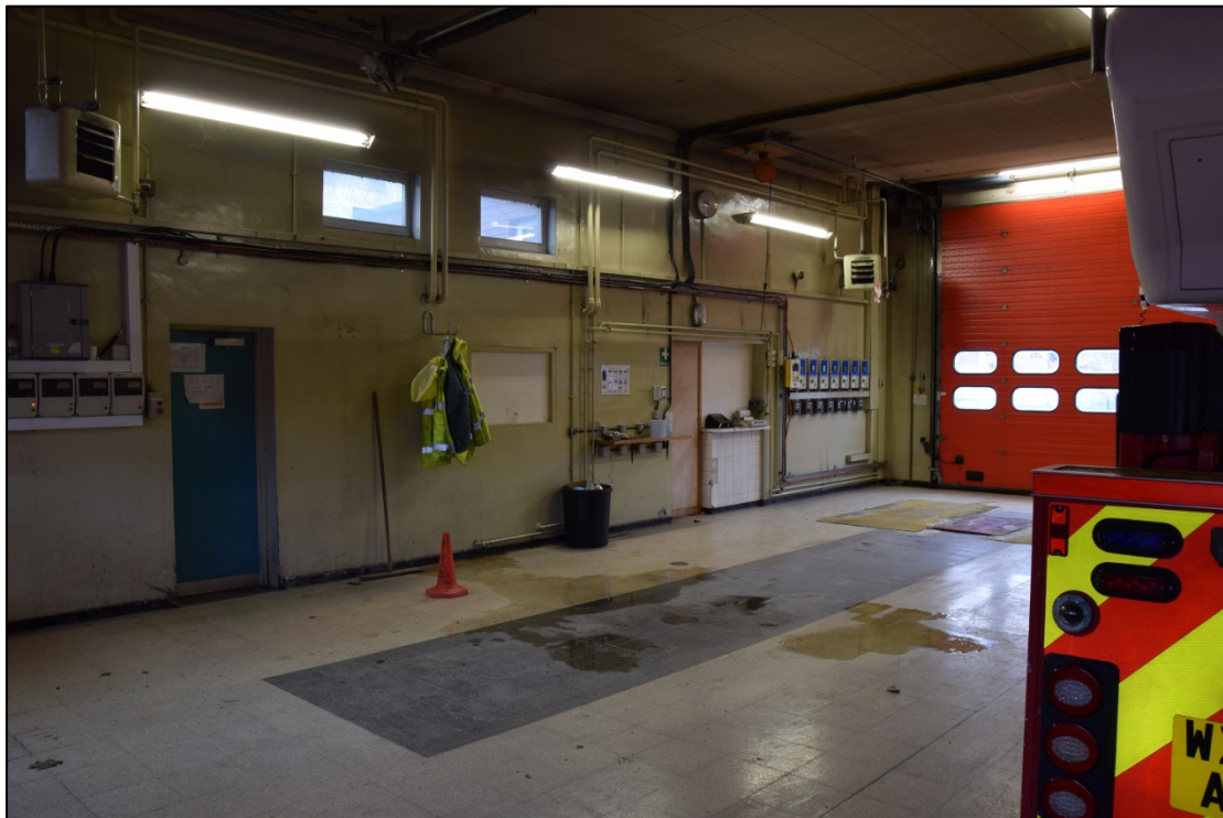
Photograph 48: The south end of the garage 35, showing blocked openings to rooms 15 and 16
