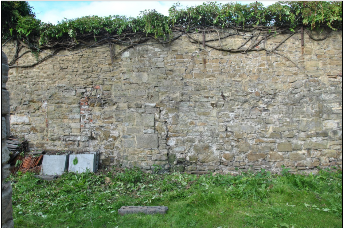
Photograph 11: Blocked openings [8] and [9] flank an anomalous vertical section of dressed stone [13], just left of centre. There is a ragged straight joint [14] just to the right. Note the yellowish stonework in the upper part of the wall here
