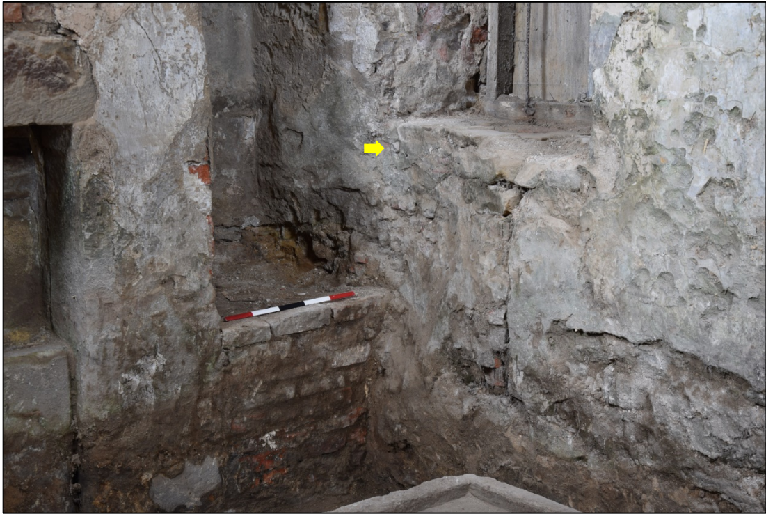
Photograph 39: In the south-east corner, a straight joint runs through the sill of the splayed window. To the left, arrowed, is the lead water pipe shown on the 1830s plan
