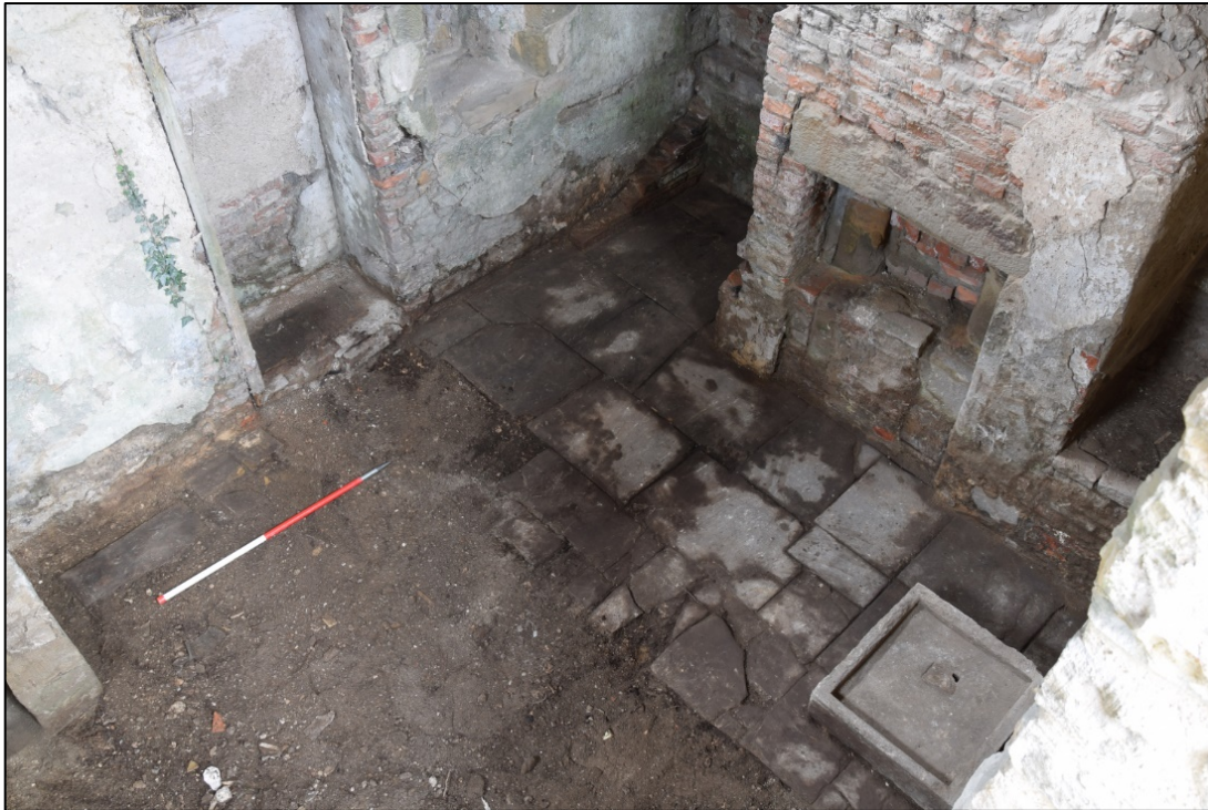
Photograph 47: Flagstones survived at the east end of the tower, at the north-west corner and in the small south block
