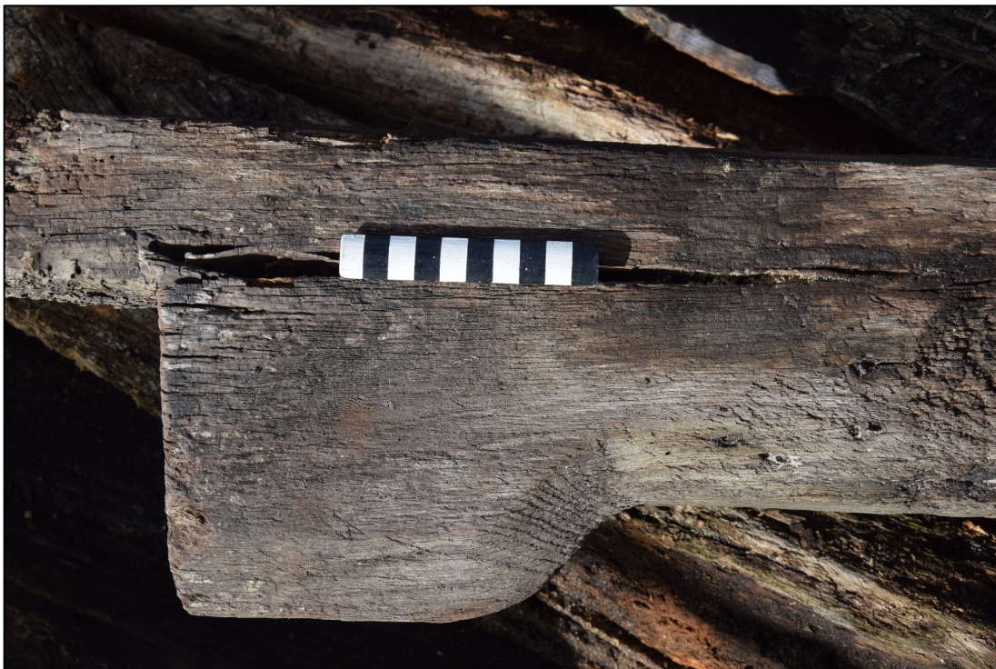
Photograph 20: Detail of the jowl at the end of a purlin, photographed in the yard after removal from the floor of the tower
