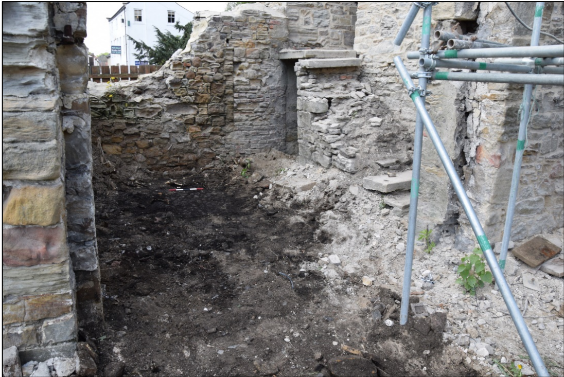
Photograph 51: The yard and external stair after the gate was re-opened. The straight joint marking the north side of the outer gate can be seen in the far wall. A view looking north-west
