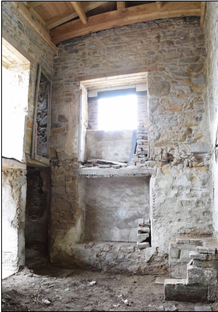
Photograph 45 (left): The west wall and the new roof timbers. There is no masonry between the embrasures of the upper and lower windows
