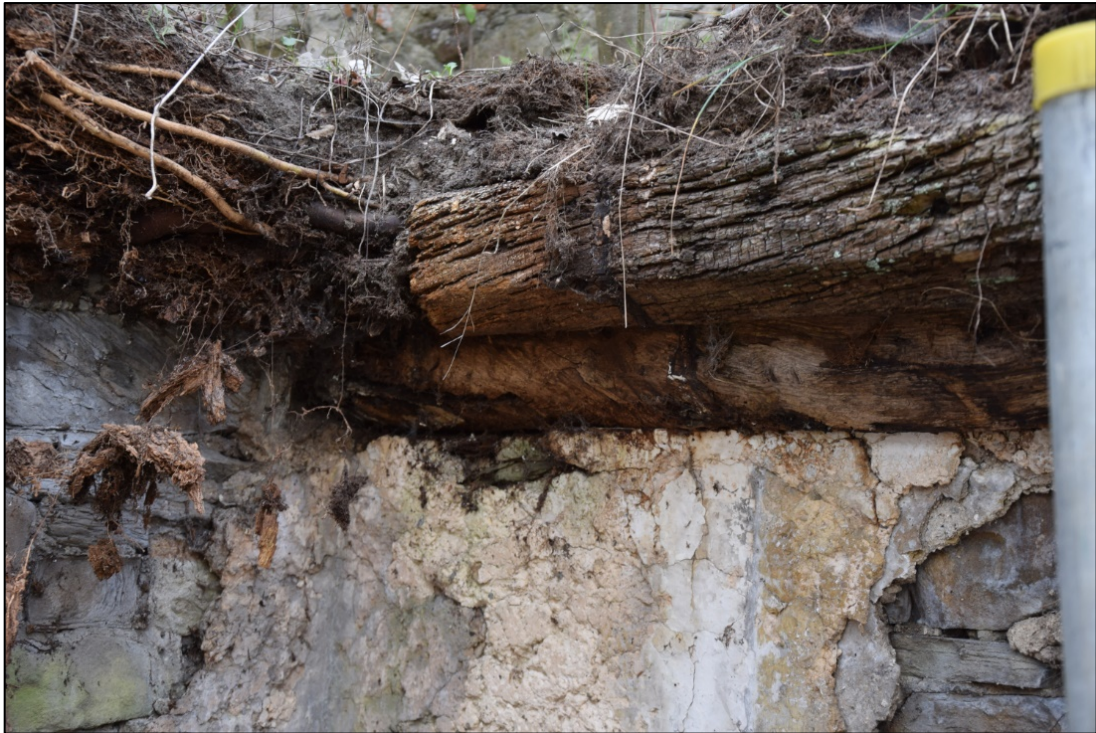
Photograph 25: Detail of the wall plate and closer at the south-east corner of the tower. Note the gap for the eastern tie beam, removed when the chimney was added to the building
