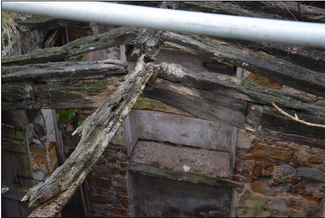
Photograph 23: Side view of the central tie beam, showing the tapered packing pieces that separated the beams from the rafters. The housings for the purlins and the joint at the end of the tie beam can be seen here. A view looking south-west
