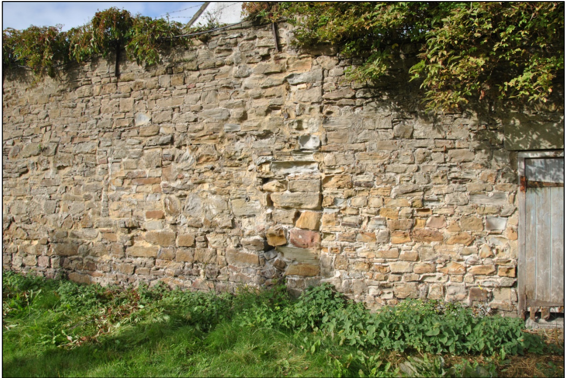
Photograph 13: The northern blocked window [12] and the wall [17] that filled the gate beside the tower
