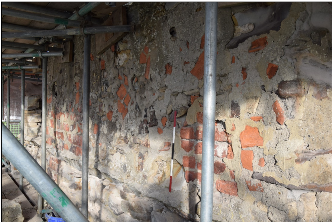
Photograph 26: Typical low-quality repair work in the upper part of the west face of the tower, with broken pantiles set in thick smears of mortar
