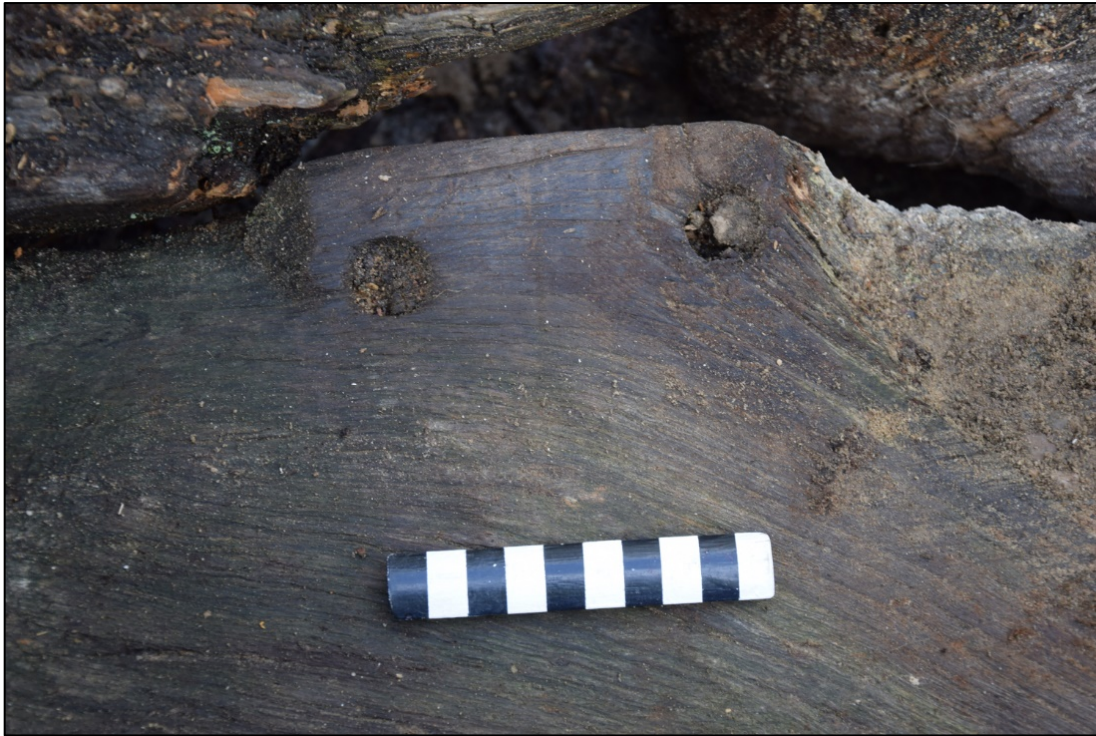
Photograph 21: Detail showing the side face at the centre of a tie beam. The two holes were for pegs that fixed a tenon at the bottom of the muntin that served as a tiny king post. At either side, plain chamfers sweep upwards to be continued on the angles of the muntin
