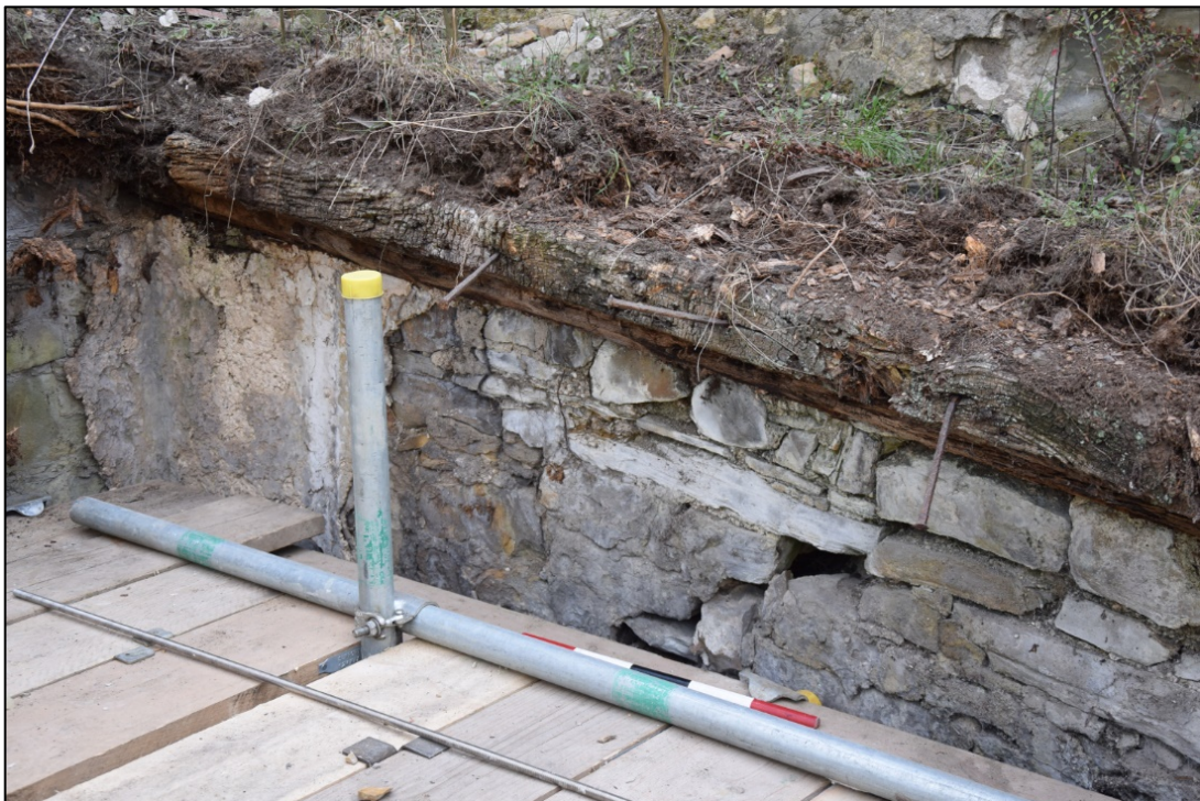
Photograph 24: The heavy overhanging wall plate and the closer beam with its large square nails. A view looking south-east
