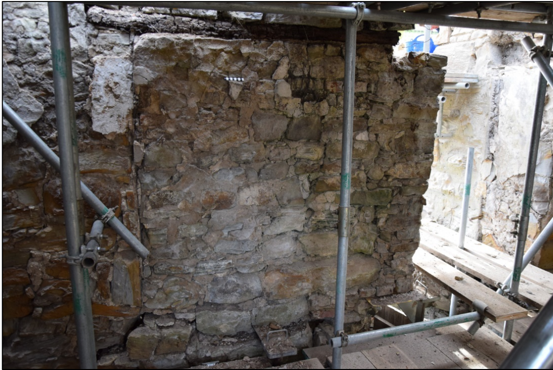
Photograph 43: First floor, south wall; the large blocked window at the centre of the wall. Note the plaster on the splay at the left. Above this, the blocking stonework has slipped forward. The right-hand side of the opening was lost when the doorway was created
