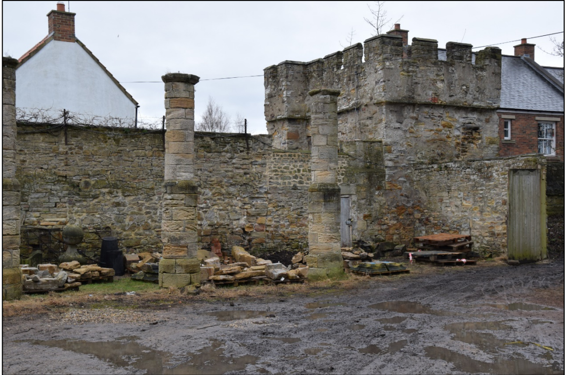
Photograph 15: The west mural tower before the start of work and after removal of the ball finials. Note the door and recent pointing in the blocking wall [17] near the centre of the view
