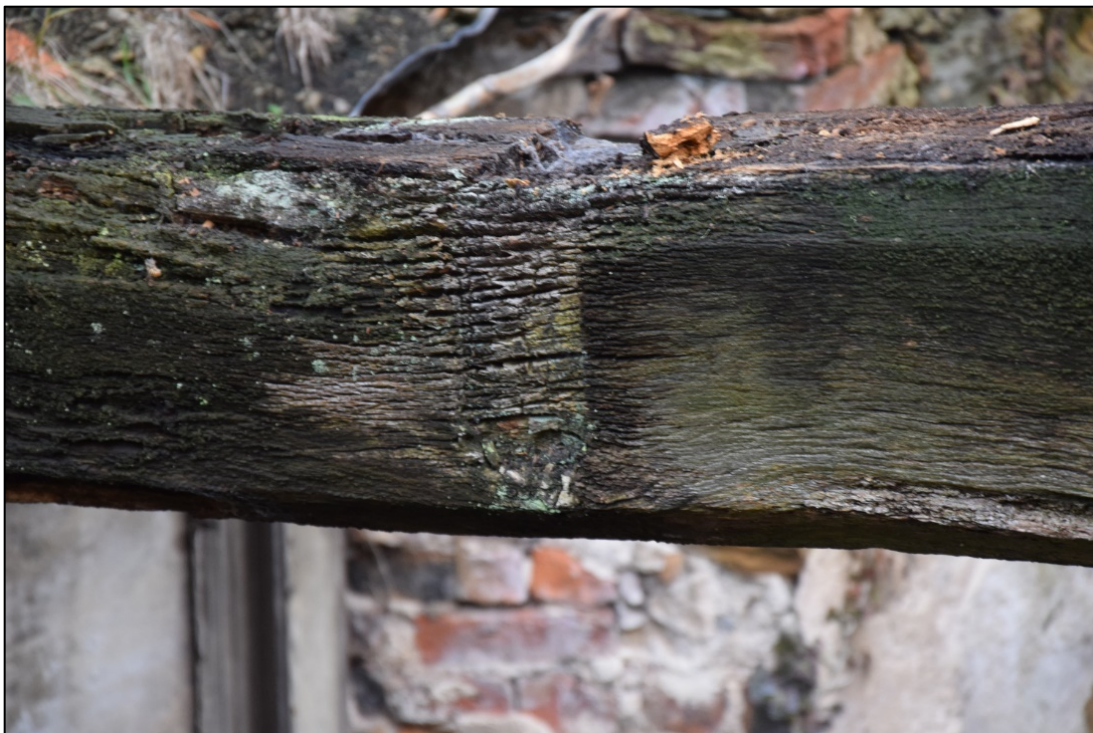
Photograph 18: The housing for the south purlin, cut into the west face of the middle tie beam
