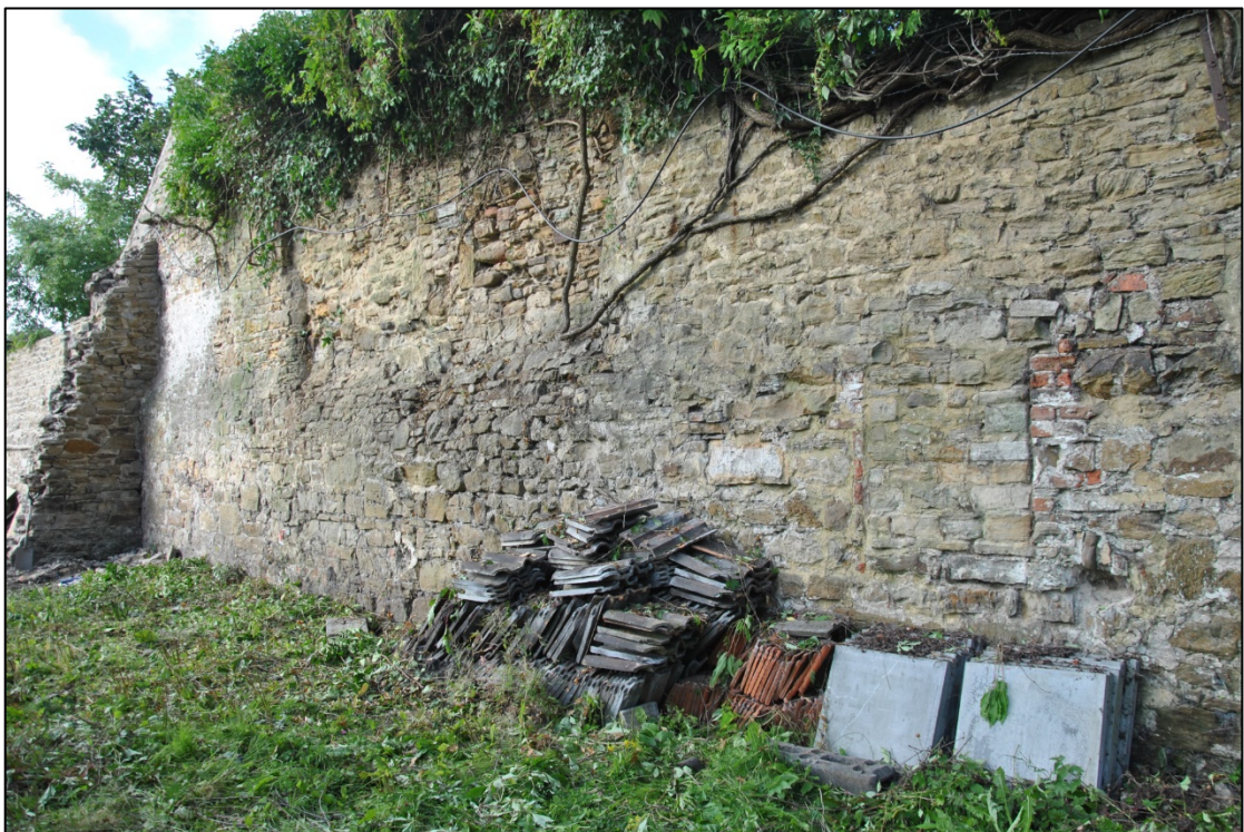
Photograph 10: The recessed section [5] with the blocked opening [6] near its right-hand end. The southernmost [8] of five square blocked openings can be seen at the right. At the far left, the sloping wall is partly demolished
