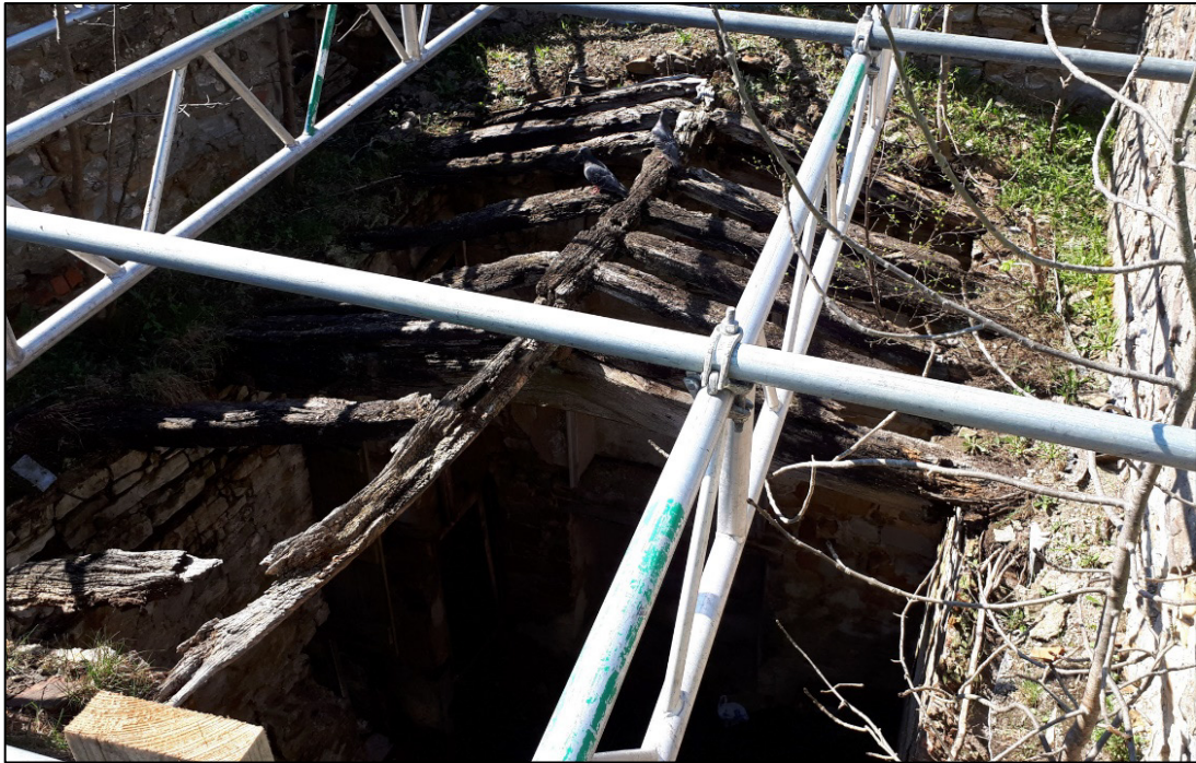
Photograph 17: The surviving roof timbers seen from the north-east corner of the building
