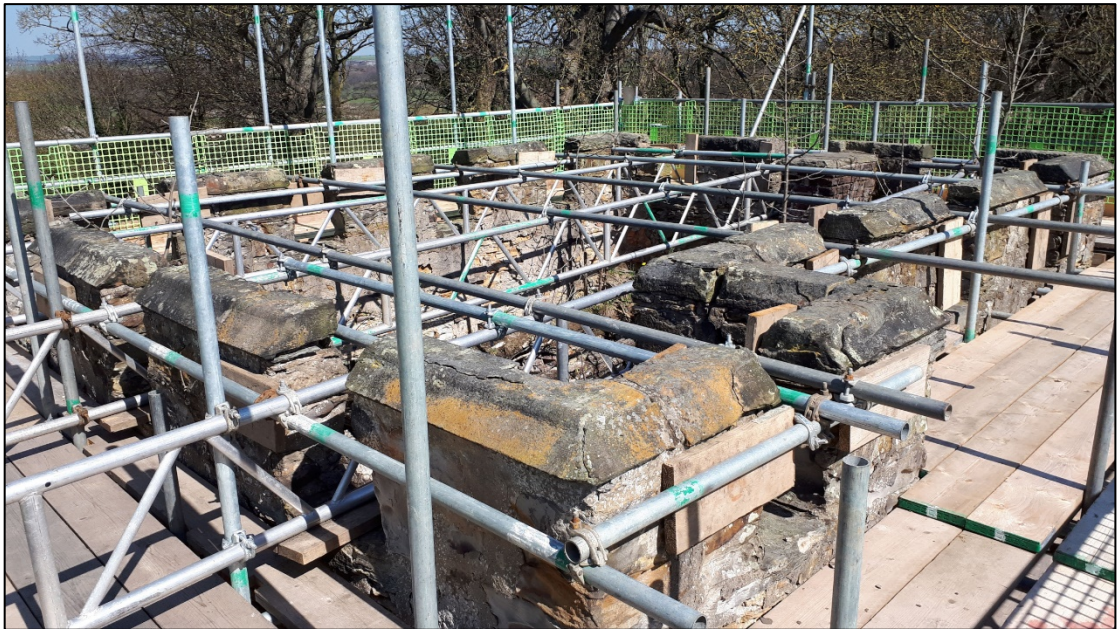
Photograph 16: Supporting scaffold in place around the tower's parapet at the start of the remedial work. A view looking north-east
