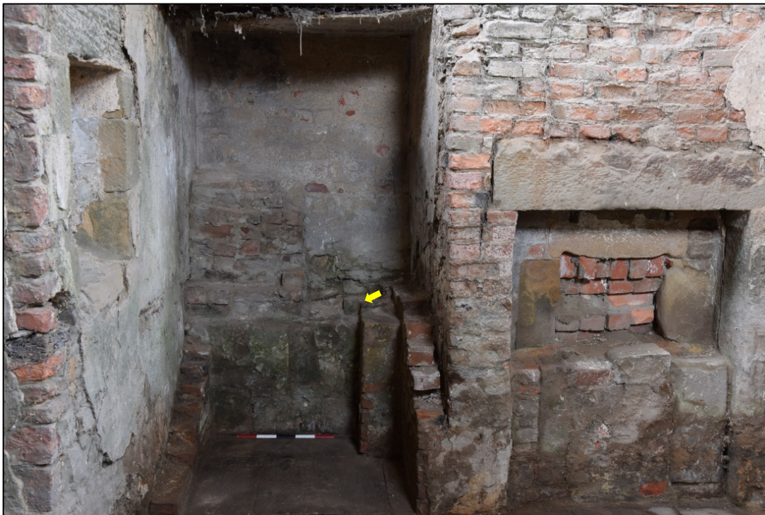
Photograph 36: The recess north of the ground-floor fireplace contains one rebated stone, arrowed, suggesting the this was an early doorway. The later brick and stone structure was built to support a copper
