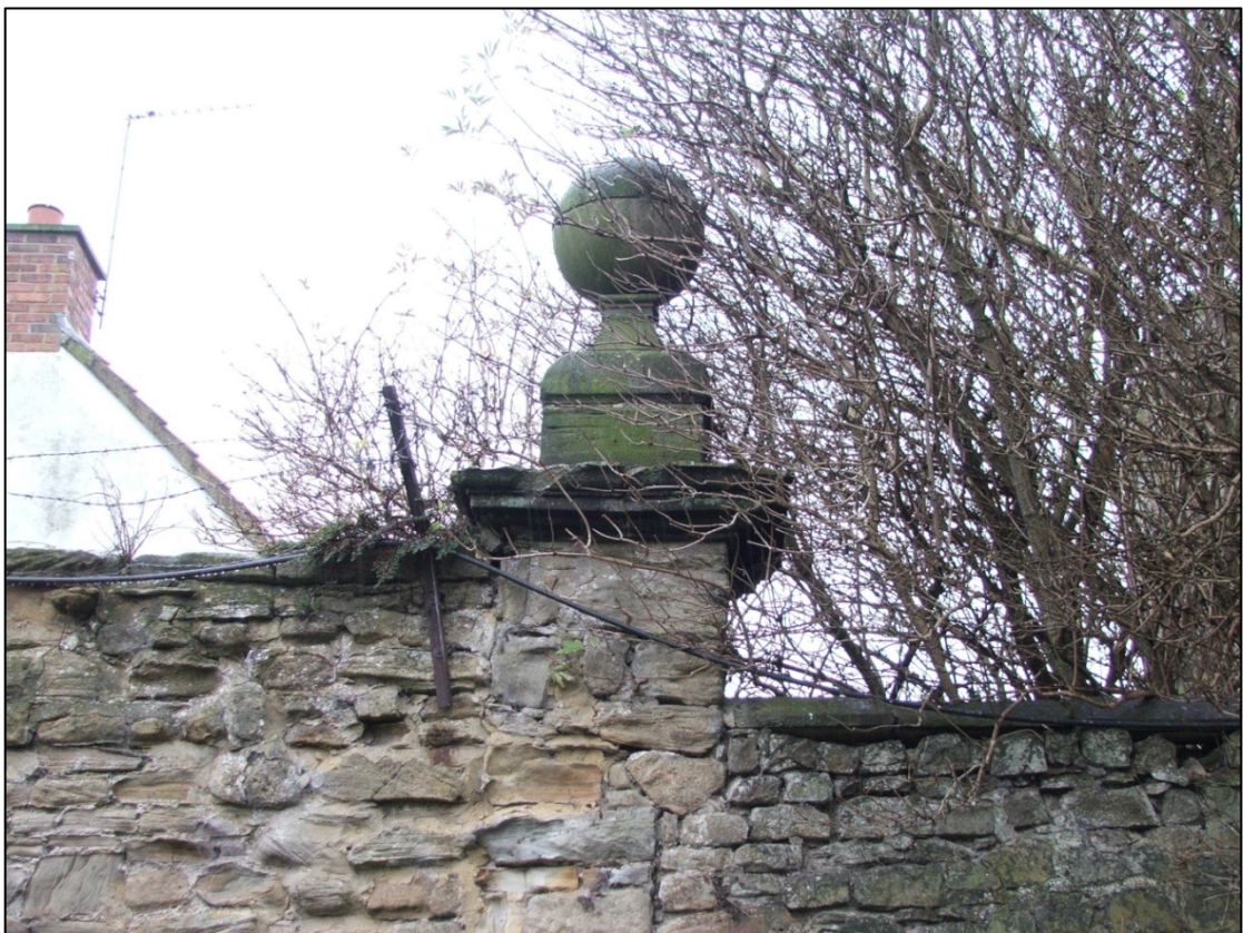
Photograph 14: The south finial of the gate beside the tower. In the centre, the straight joint between the wall and blocking steps to the right at the top of the rebate for the gate
