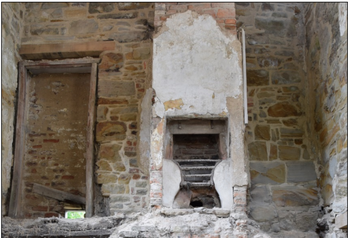
Photograph 38: Detail of the east wall on the first floor. The large stones to the right of the door frame suggest that there was a window here. On the right of the chimney, more large dressed blocks mark the putative fireplace
