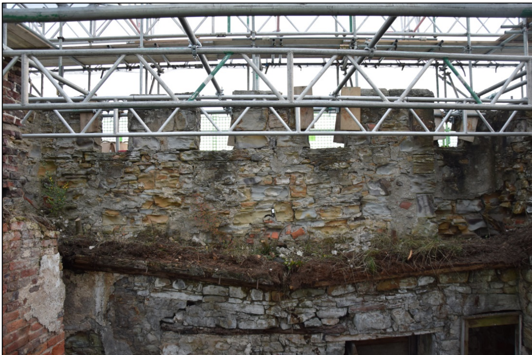
Photograph 28: The south wall. The severe deflection of the wall plate beams seems to have been caused in part by movement of masonry in the blocked opening under the decayed lintel at the bottom of the picture
