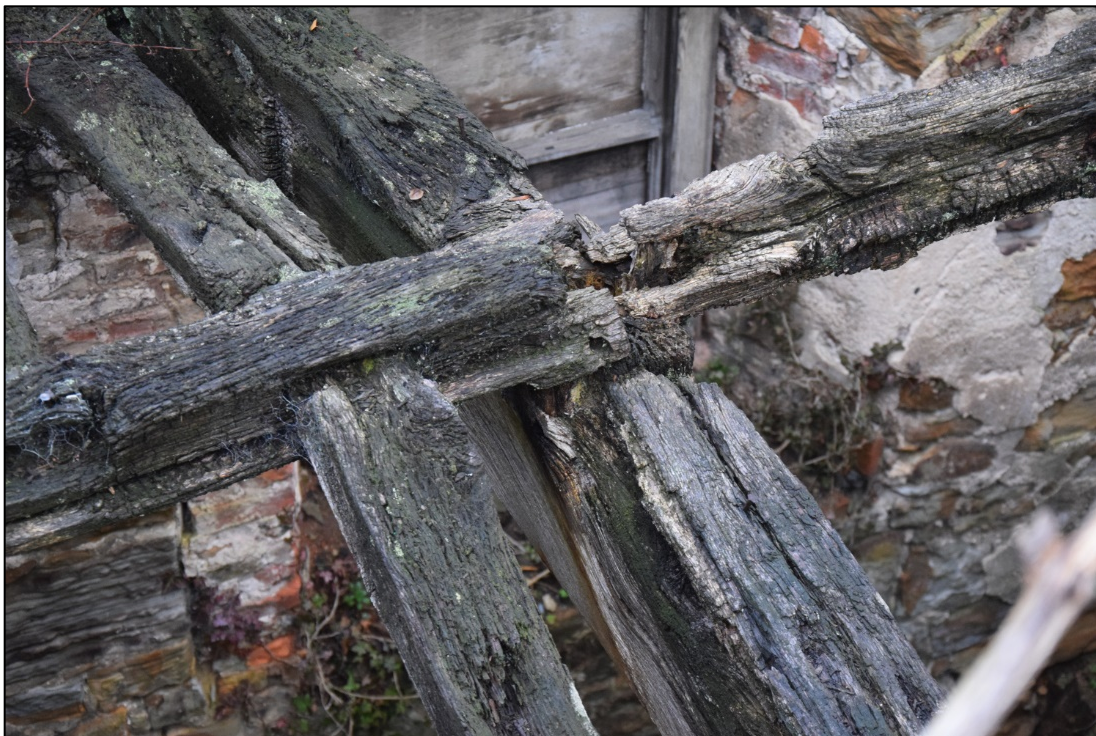
Photograph 22: The junction between the ridge beams (bottom left – top right) with the central tie beam; a pair of common rafters can be seen to the left
