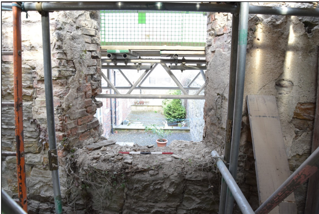
Photograph 30: North wall, first floor. Left of the left-hand brick jamb is the side of an older stone window
