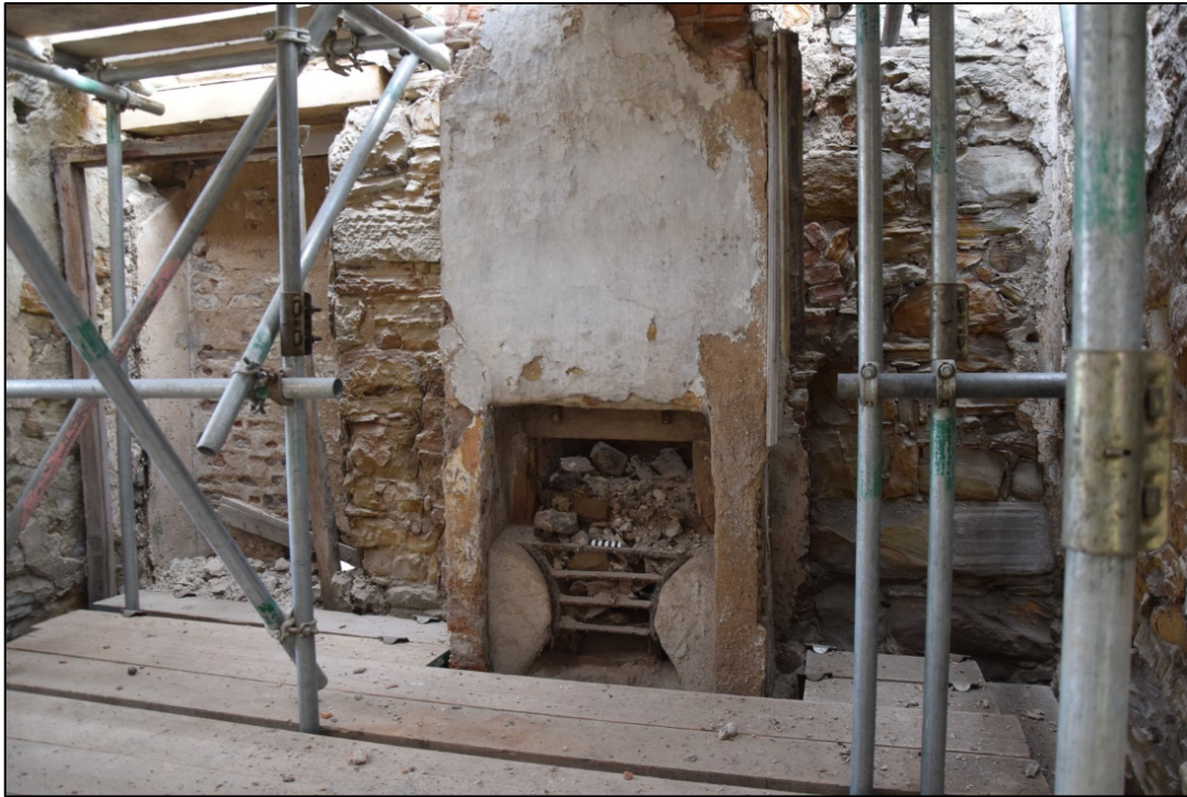
Photograph 35: The first-floor fireplace. There is a straight joint marked by plaster immediately right of the chimney breast; this may be what remains of an earlier fireplace
