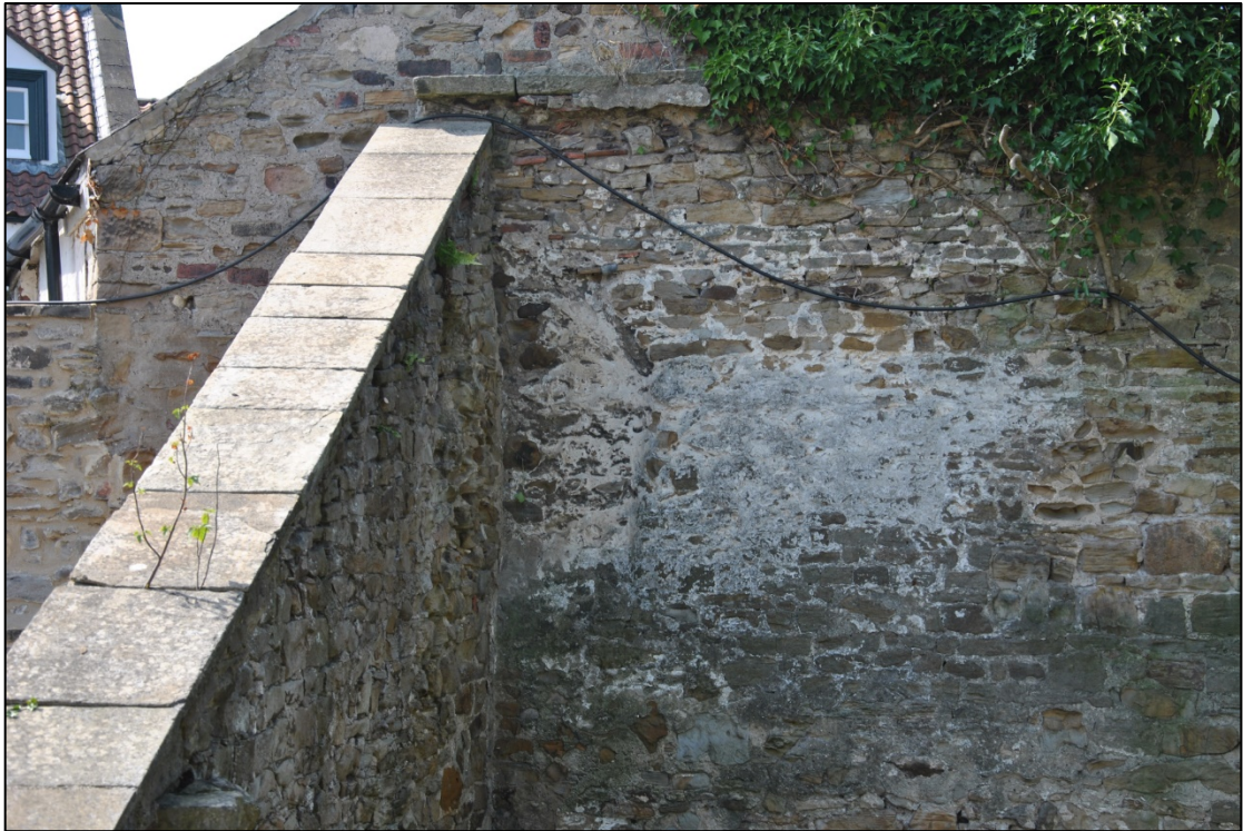
Photograph 9: The west wall and its junction with the gable of the neighbouring house. The possible blocked opening [3] is at the centre under a row of coping slabs and a few pantiles
