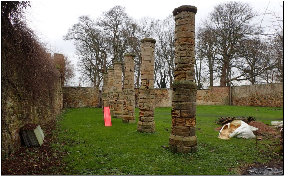
Photograph 5: The west court seen from the south-west corner, with the piers of the hay shed / coach house. The embattled parapet of the west mural tower can be seen, top left
