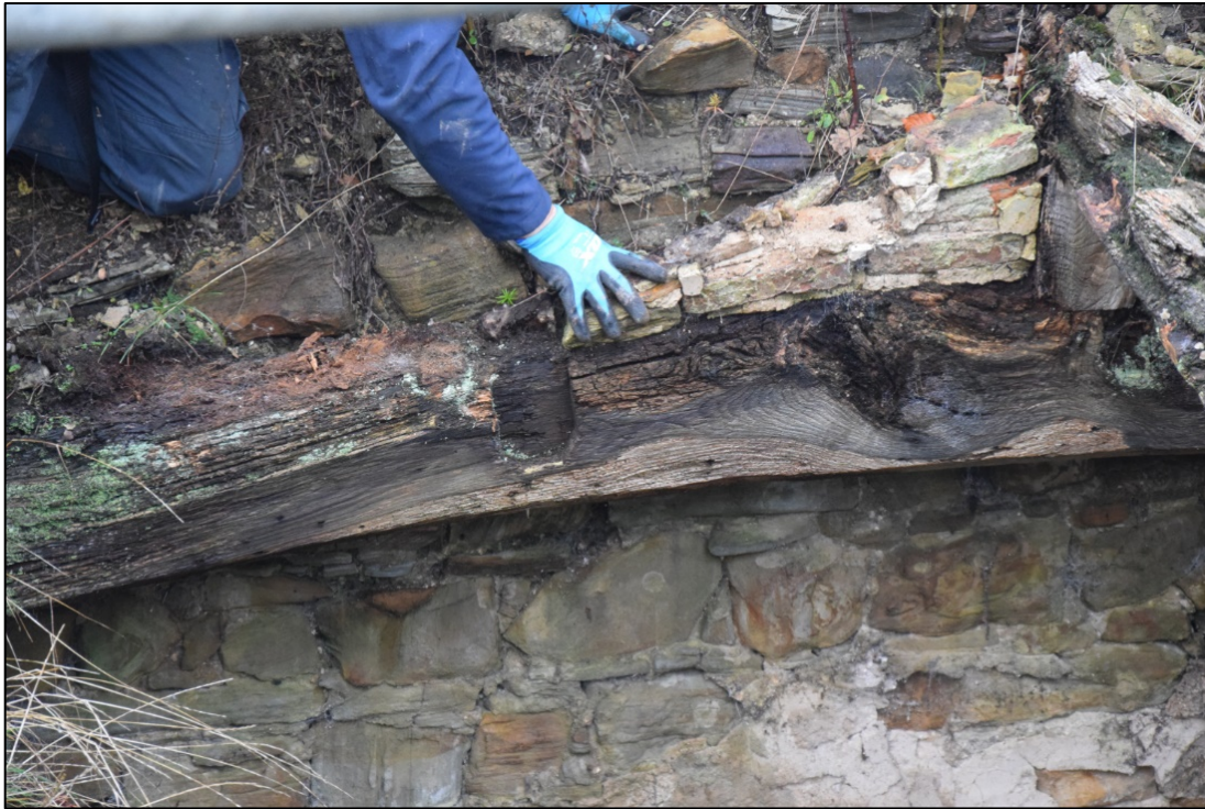
Photograph 19: The south limb of the western tie beam has a similar housing. The masonry that filled the space between the tie and the common rafter is being removed. At the top left, the ridge beam rests on a short vertical muntin
