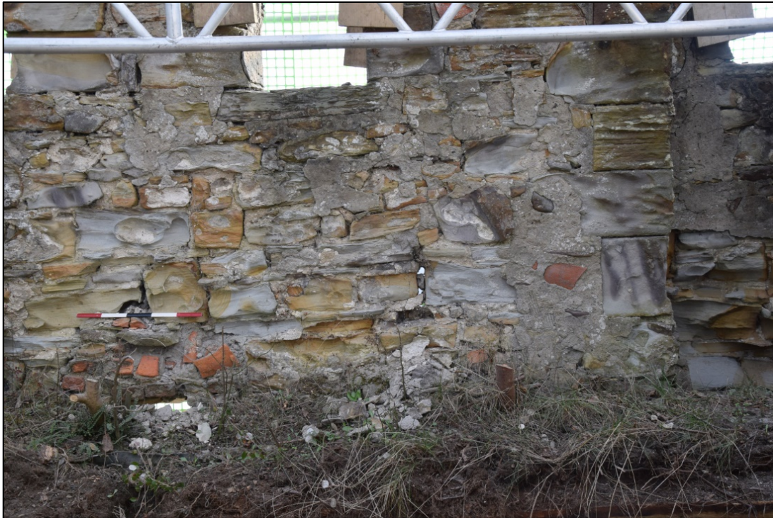
Photograph 27: Daylight is visible between the stones of the south parapet and there is another crude repair below the scale. Cement render covers the upper wall in the south block, at the extreme right
