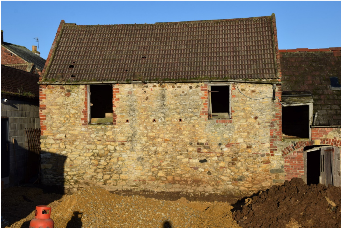
Photo 3: The face of the old byre and hayloft. The tall upper openings were used to pitch hay or straw from carts in the yard
