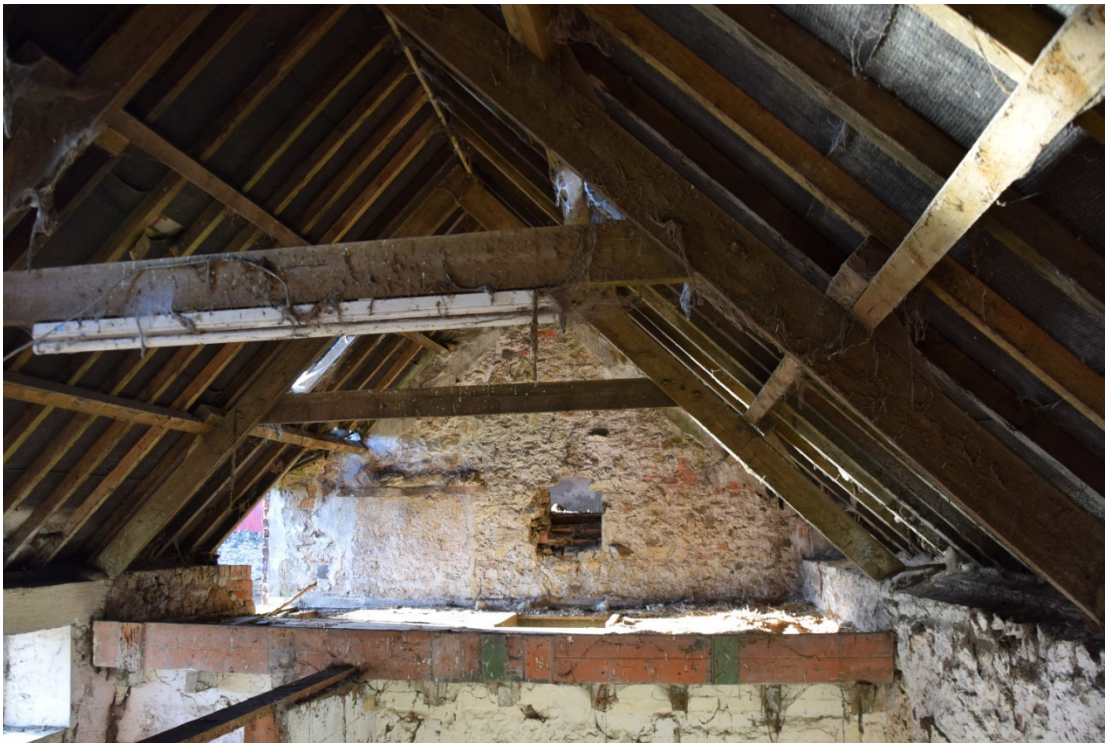
Photo 8 (below): The east end of the loft, seen from the adjoining barn. Note the blocked opening at the left, which extends below the hayloft floor
