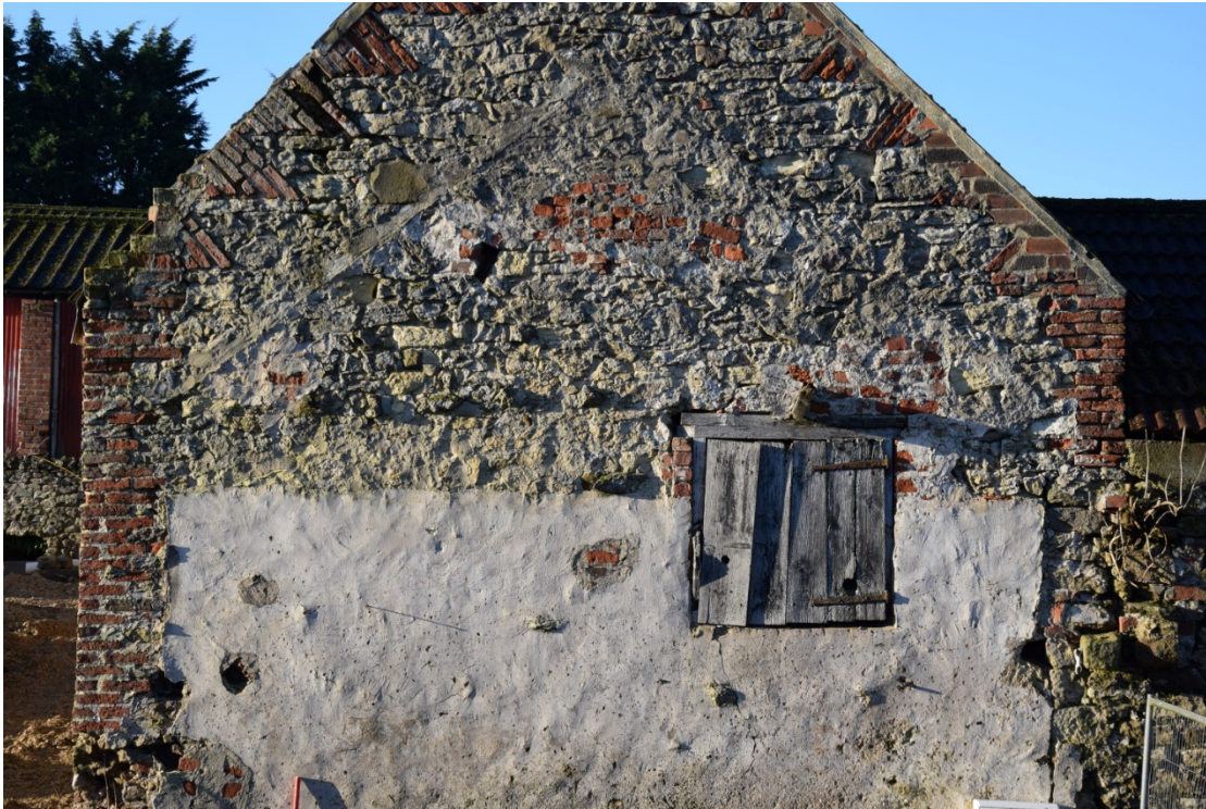
Photo 23: Detail of the east end, showing the roof line of the demolished third section above a blocked ventilator like that in Photo 19
