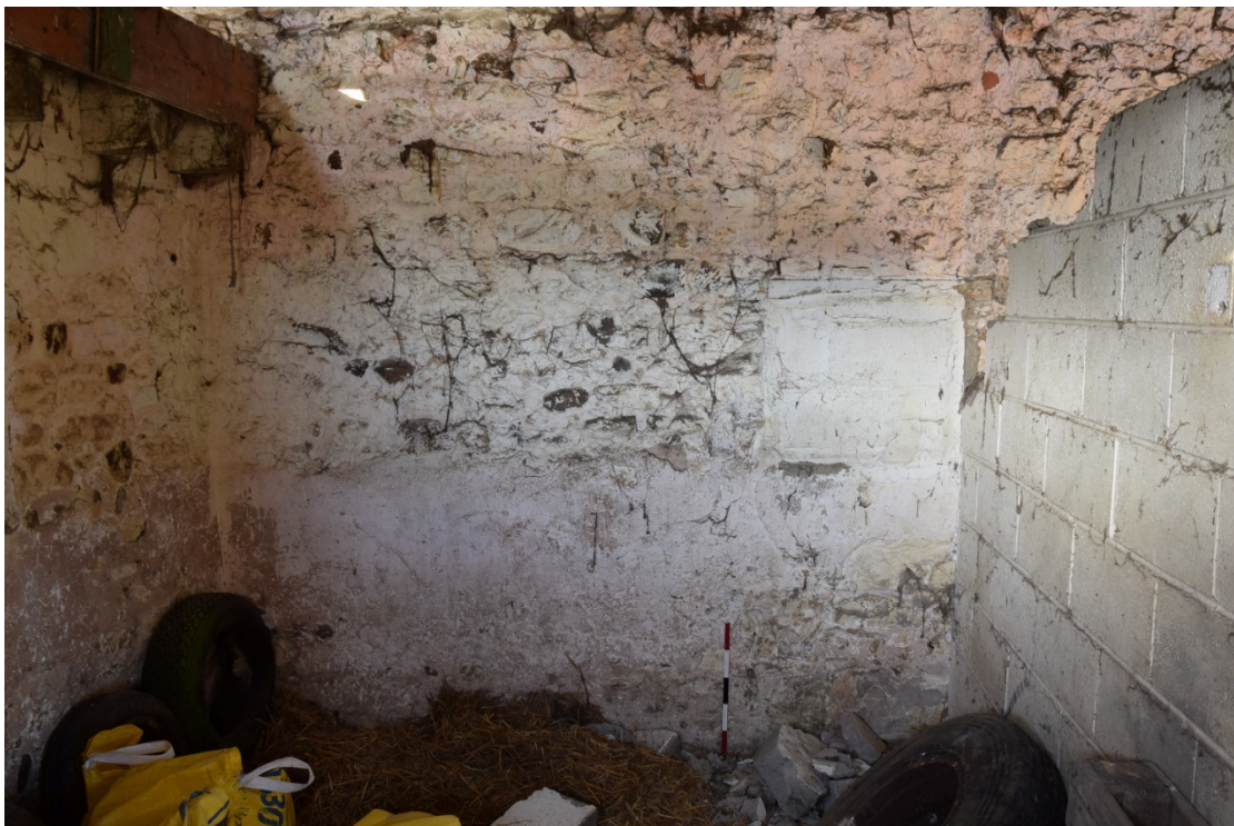
Photo 28: The western room in the barn, with a blocked opening in the north wall
