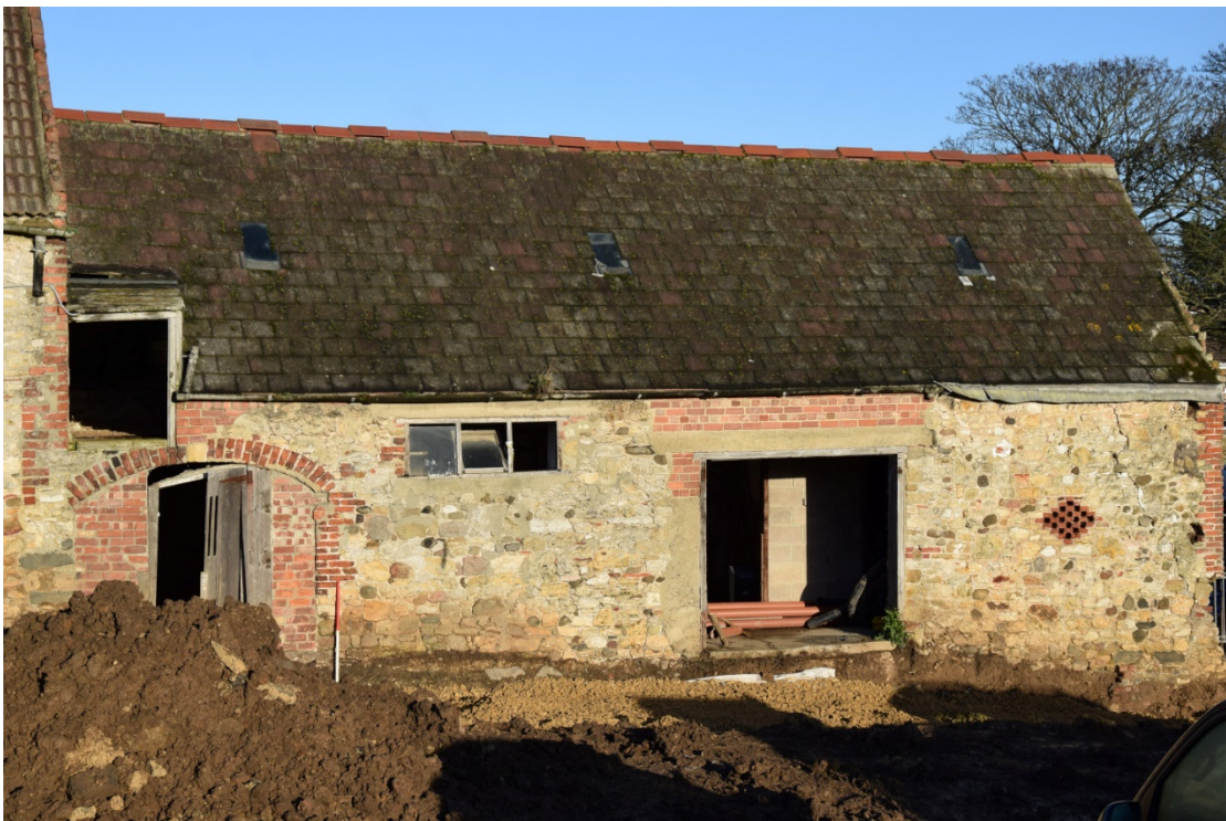
Photo 18: The barn seen from the south-west. The modern material of the roof is apparent here
