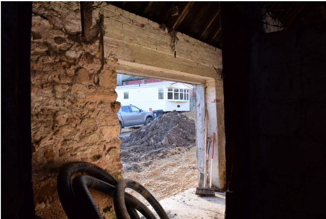
Photo 32 (below): Inside view of the large 1960s door in the south wall
