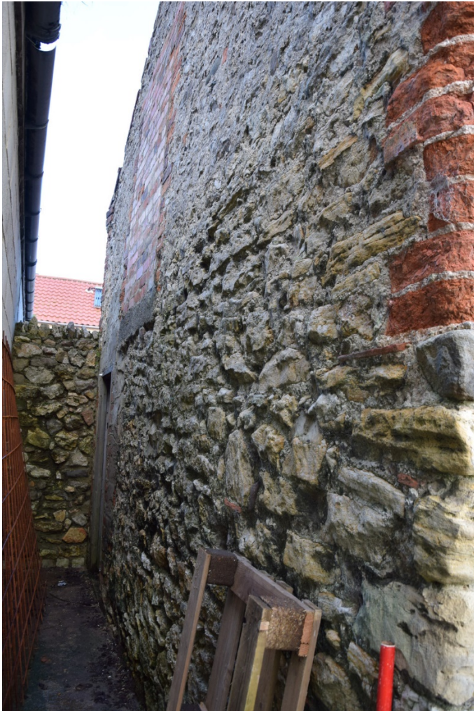
Photo 7 (left): The west end of the byre. A tall door to the loft is bricked up
