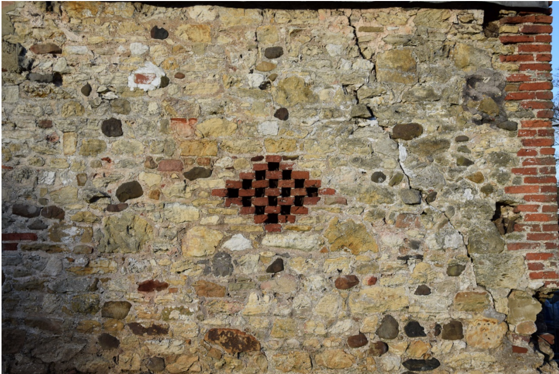
Photo 19: A large subsidence crack runs across the east end of the south face, above a brick ventilator
