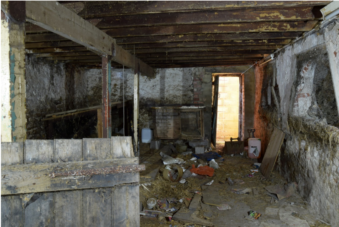
Photo 9: The byre, with steel I-beams supporting the main joist; at the left is a detached door from a stall. A view looking south-west
