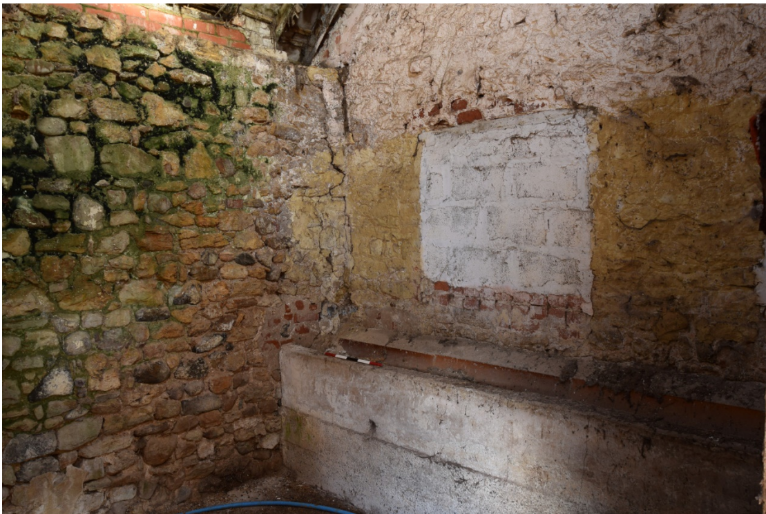
Photo 30: A modern trough runs across the east wall of the barn, below a blocked window
