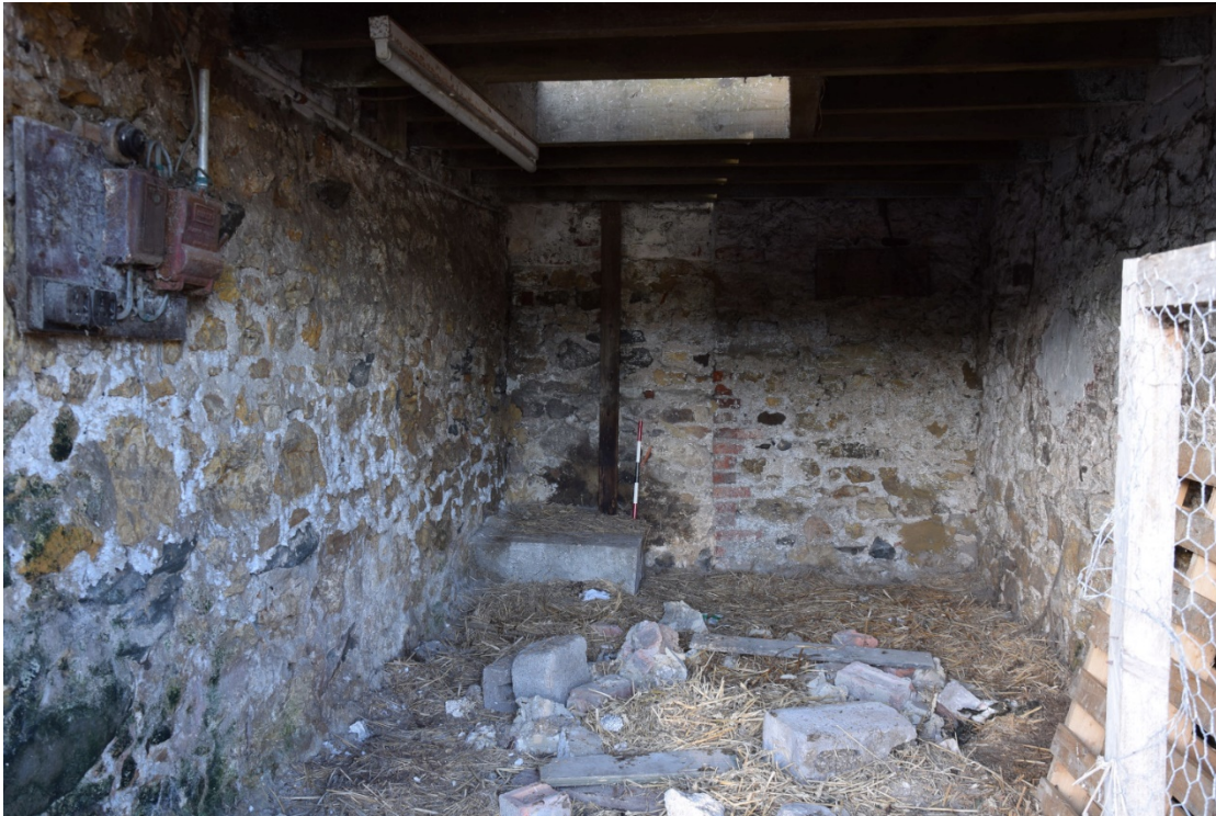
Photo 25: Looking north into the shed at the west end of the barn. Note the straight joint in the far wall
