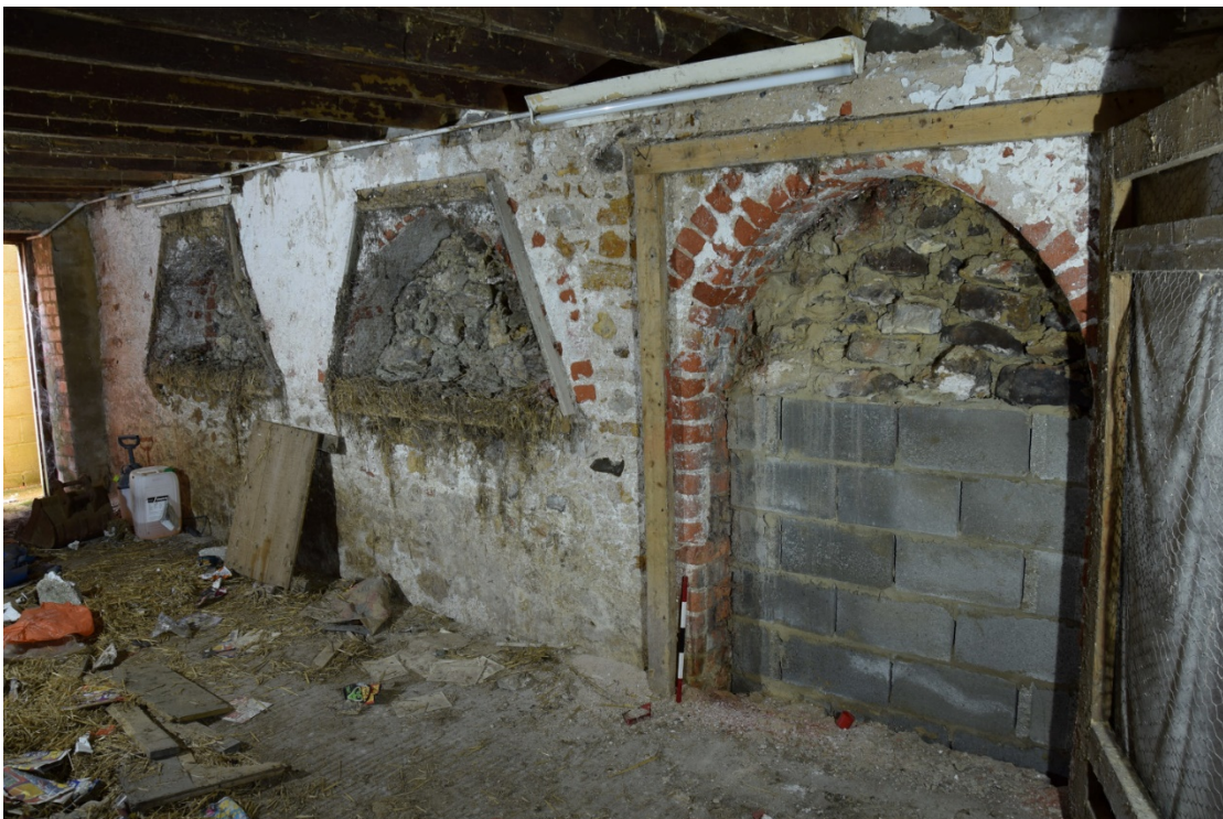
Photo 12: The north wall had two arched windows and a wide door from the yard, all now blocked up
