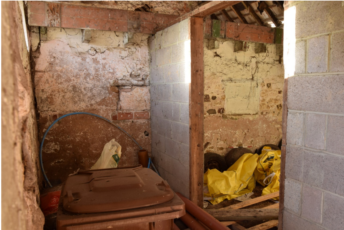
Photo 27: Two small blocked hatches in the wall between the shed and the main part of the old barn. A view looking north-west
