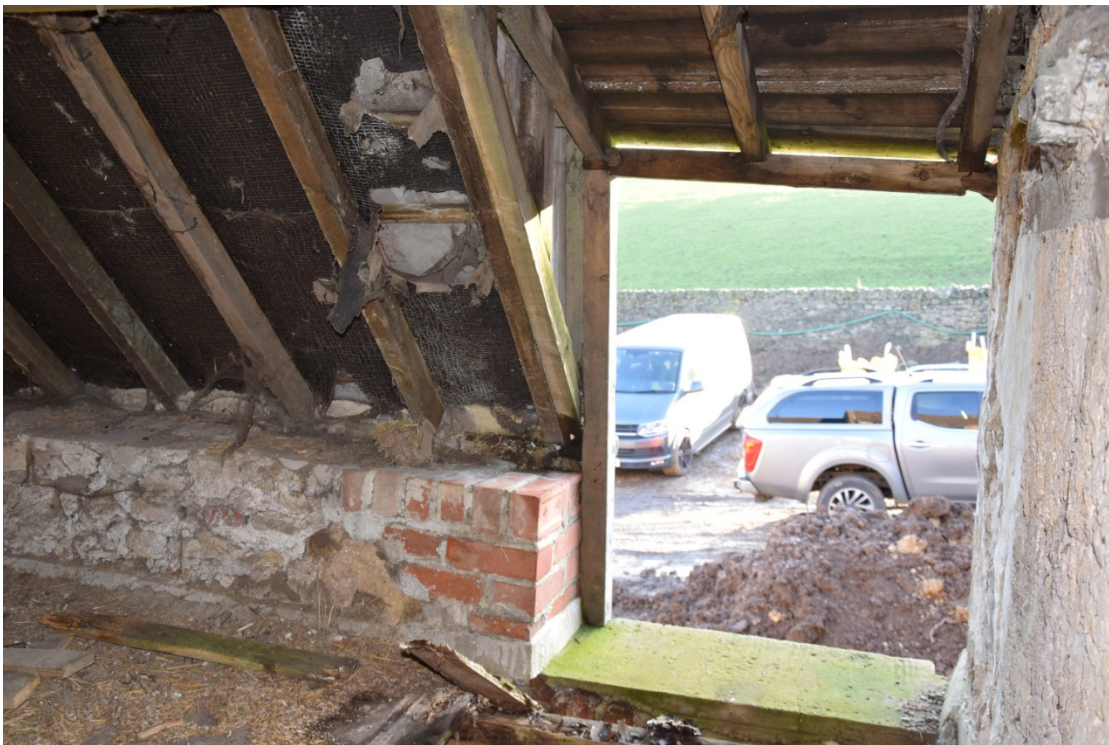
Photo 34: The modern pitching door at the south side of the small loft
