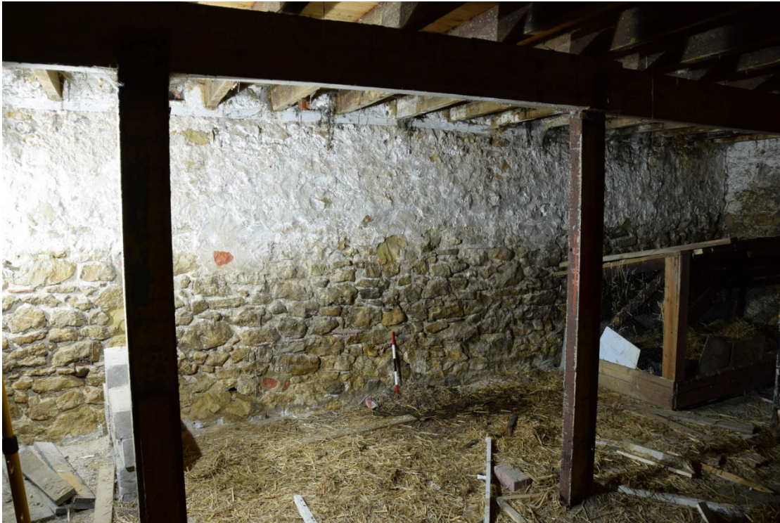
Photo 11: The south wall shows no trace of stall divisions and the ventilators between the joists are blocked up
