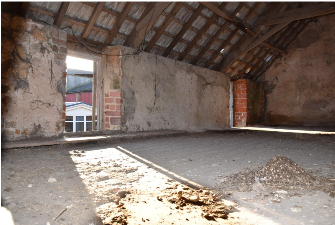
Photo 16: The larger pitching windows in the south wall have brick in their jambs
