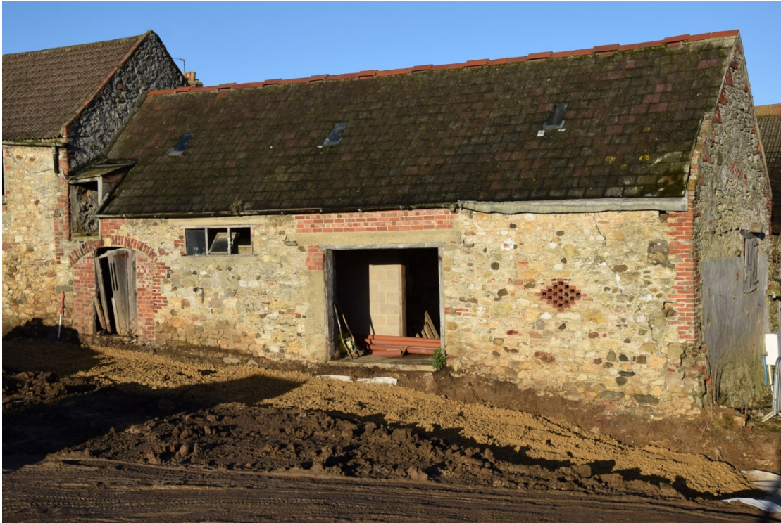
Photo 17: The old barn. The gin-gang joined this building where the big modern door is now
