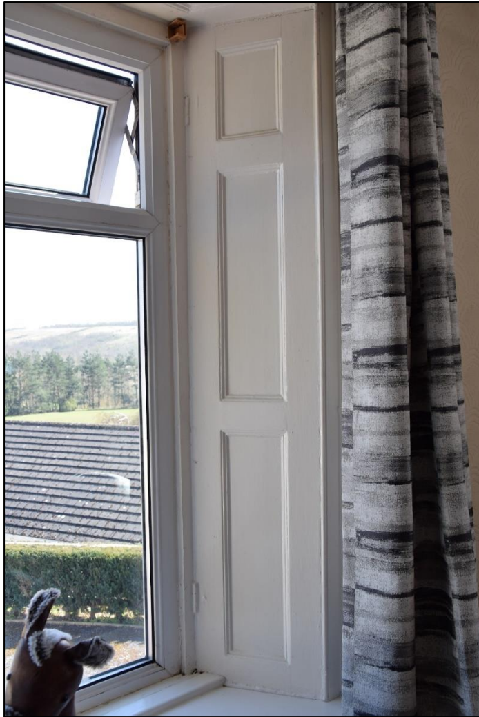
Photograph 29 (left): Hinges can be seen on the folding shutter of the east window in the sitting room
