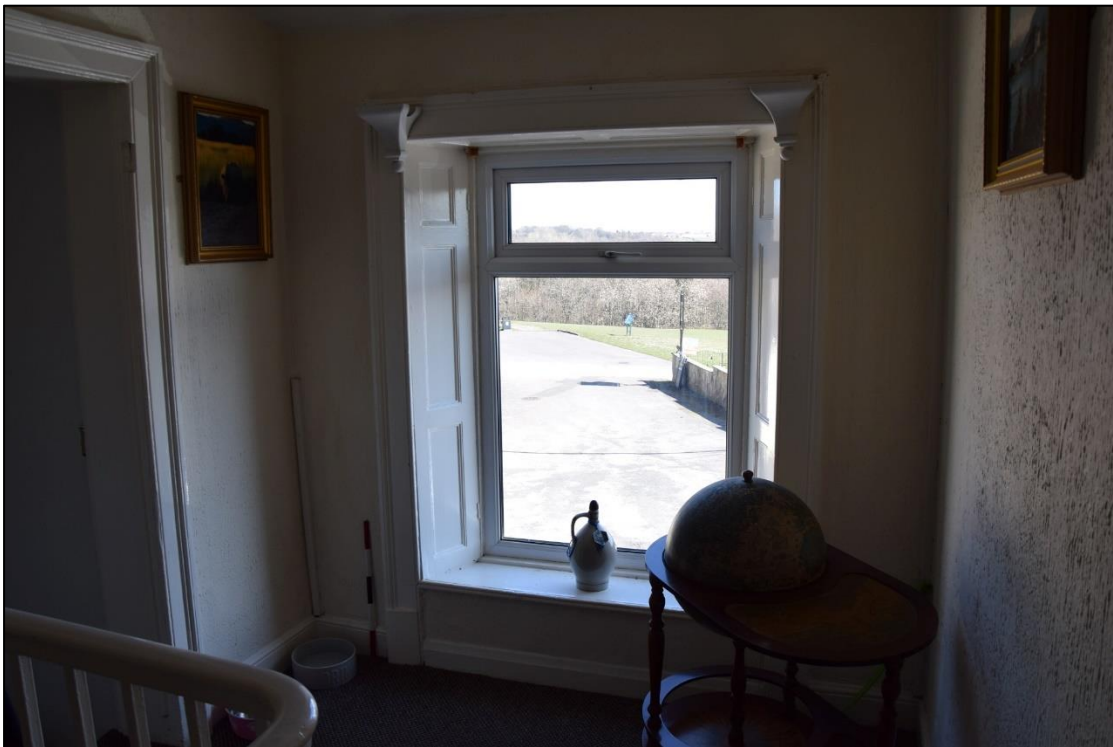
Photograph 26: The panelled window in the porch extension. The moulded brackets at the top corners are not original
