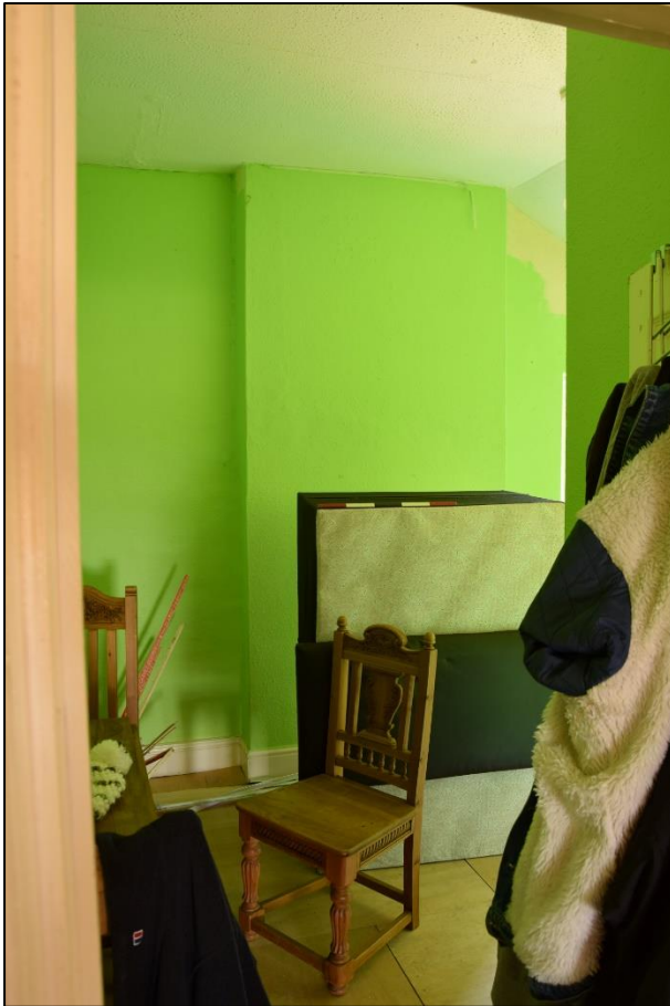
Photograph 33 (left): The altered back bedroom, seen from the door. The chimney breast has no fireplace. The darker green wall at the right is the corner of the inserted store room
