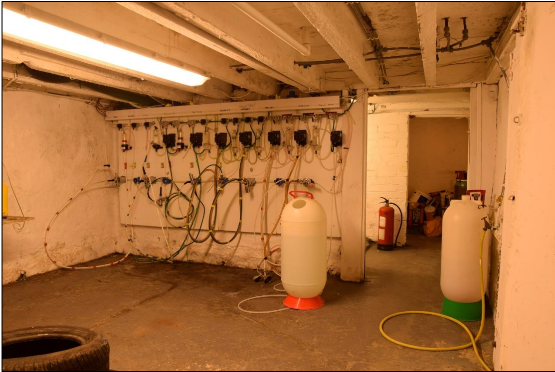
Photograph 37: A view looking north-west across the cellar. The staircase is behind the wall beside the fire extinguisher
