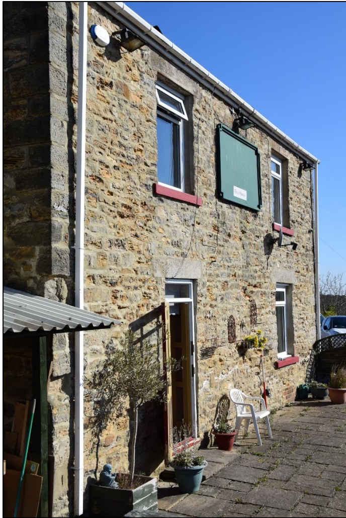
Photograph 7 (left): As elsewhere, the masonry and design of the south front is very simple. A view looking north-east
