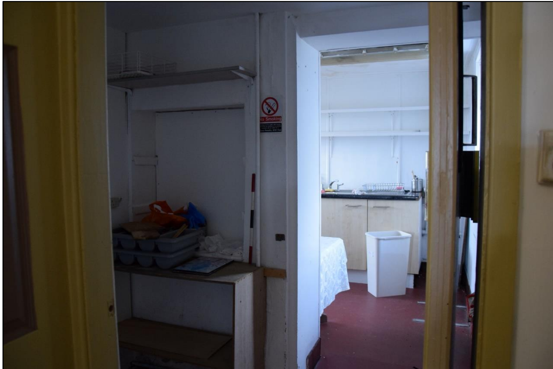
Photograph 21: A view from the bar across the rear passage into the kitchen
