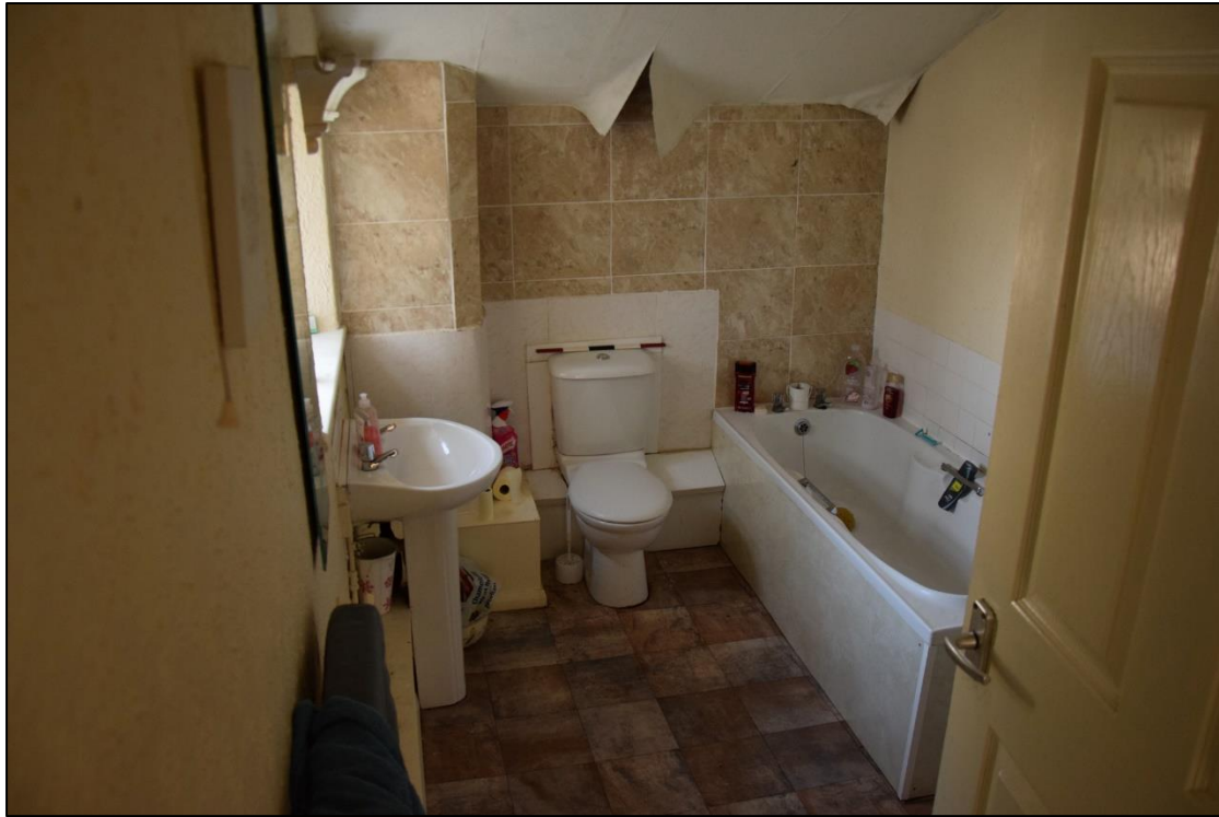
Photograph 35: The bathroom floor is well below that of the landing, where this photograph was taken from
