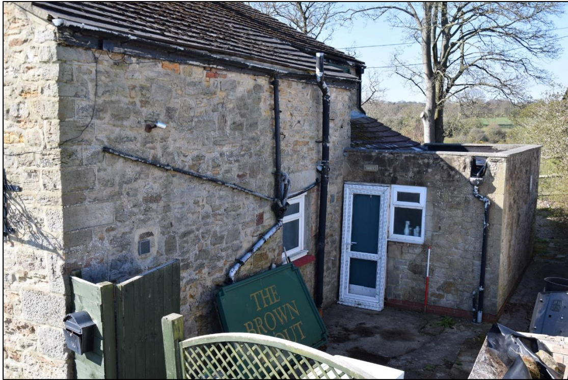
Photograph 11: The kitchen extension at the rear of the building runs up to the end of the old outshut
