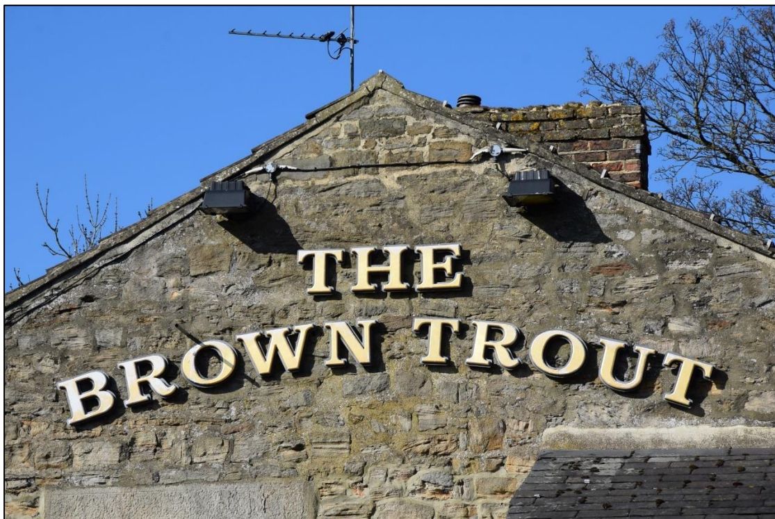
Photograph 4: The peak of the east gable has been rebuilt after the removal of a chimney stack
