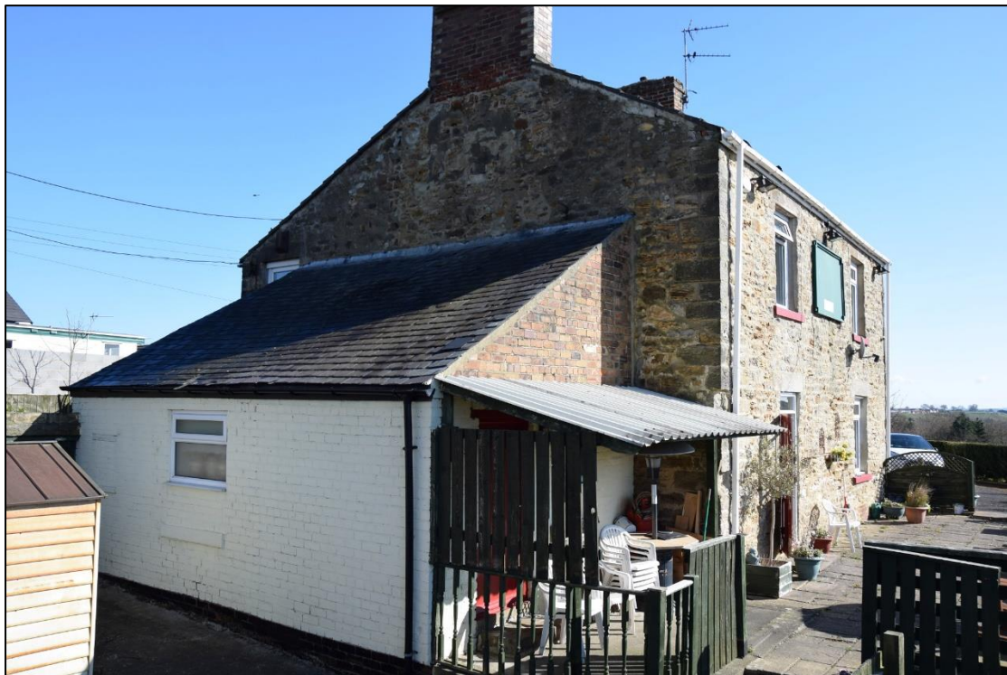
Photograph 8 (below): The brick-built games room at the west end of the building
