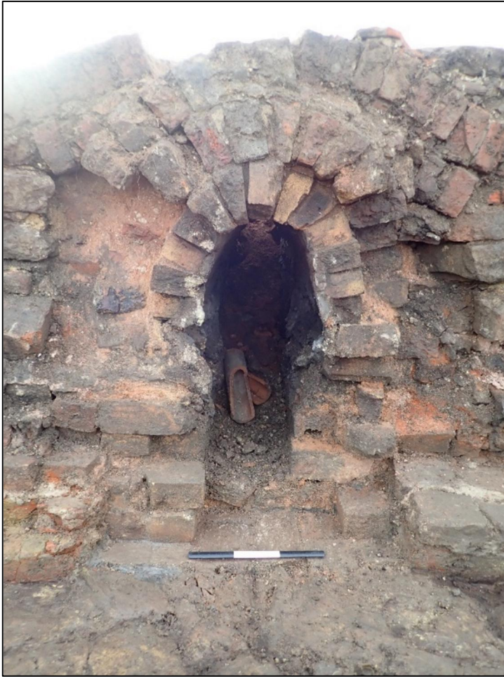
Photograph 11 (left): The central fire mouth in the northern furnace room shows several rings of brick in the arch. The shape is distorted by heat and movement of the structure. The scale divisions are 100mm long
