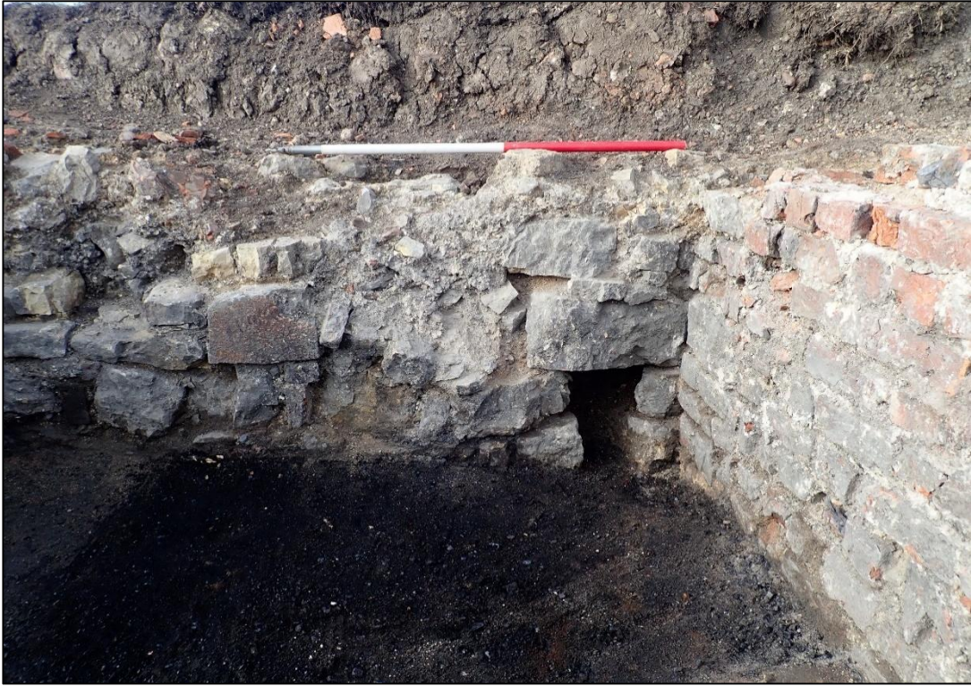
Photograph 27: The drain opening at the north-east corner of furnace room 57. A view looking north
