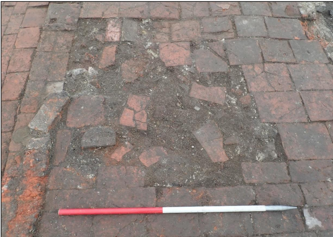
Photograph 36: The damaged floor of room A seen from the east, with the door at the top left
