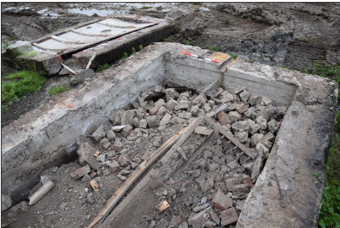
Photograph 10: The interior of the shelter, with the roof lying on the ground beyond it. Timber shuttering marks and coarse, unsorted aggregate can be seen on the inside faces of the walls
