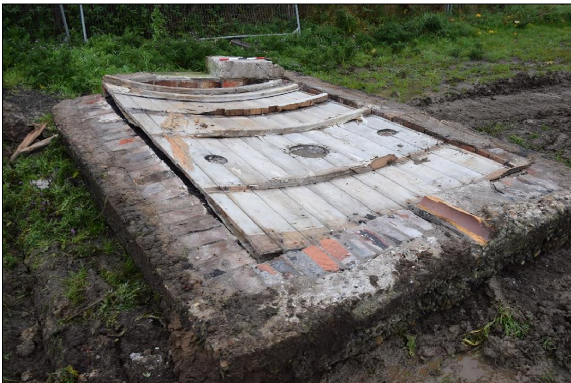
Photograph 12: The upturned roof of the shelter. A row of bricks runs around the inside of the concrete slab, which has broken away from the curved timber base along the left-hand side
