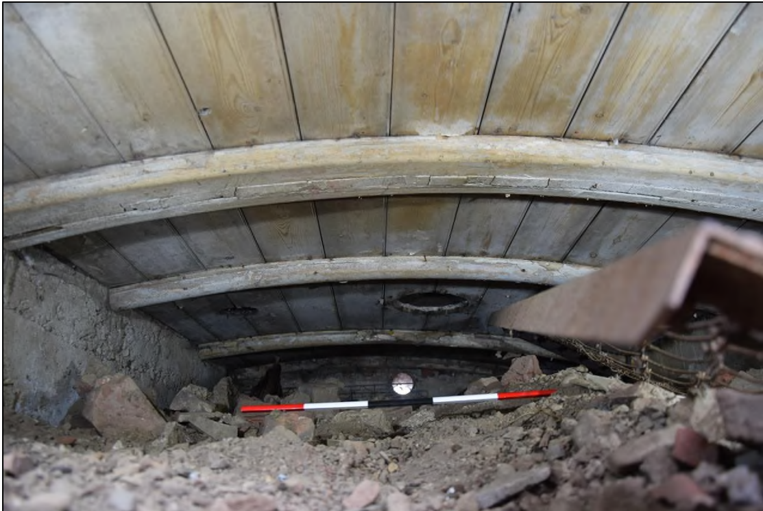
Photograph 9: Detail of the ribs and planking of the roof. Note the vertical boards sandwiched between two ribs, and two of the three flue holes in the timber further back
