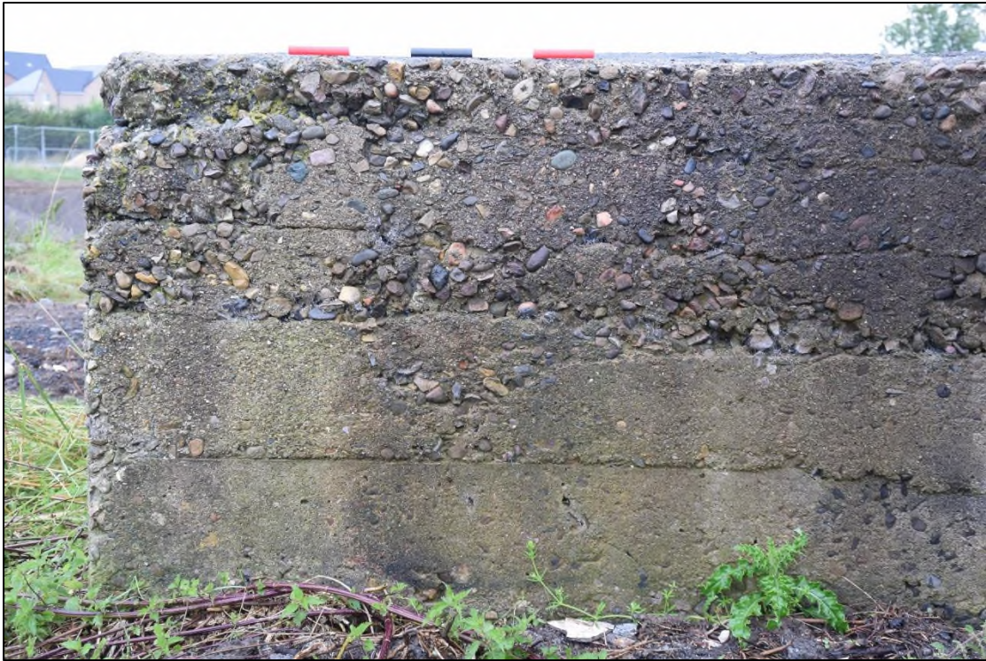
Photograph 5: Detail of the south-west corner, showing irregular shuttering marks and the coarse, poorly-sorted aggregate in the concrete
