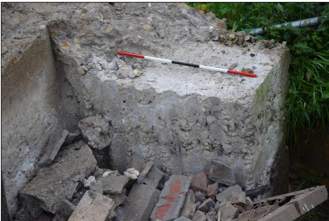
Photograph 6: The marks of corrugated iron sheet shuttering just inside the door of the shelter
