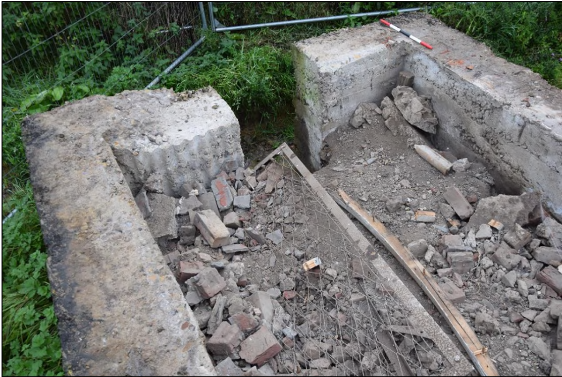
Photograph 11: The east end and the door after removal of the roof. The absence of any reinforcement is obvious here and in the previous picture
