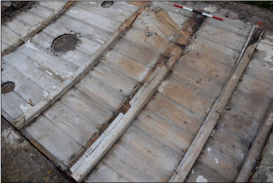
Photograph 13: Detail of the ribs and chimney or vent holes in the former guard's van roof. The thick rib at the centre incorporates the thick boards of the former partition
