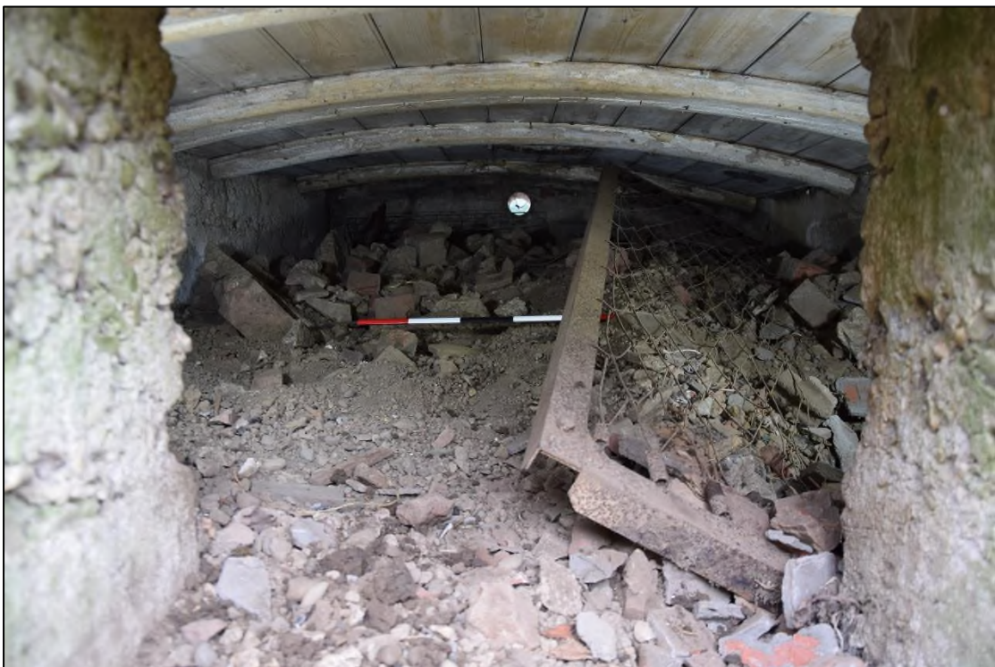
Photograph 8: A view looking into the shelter after the upper part of the door was cleared. The wooden railway van roof that supports the concrete is set slightly askew
