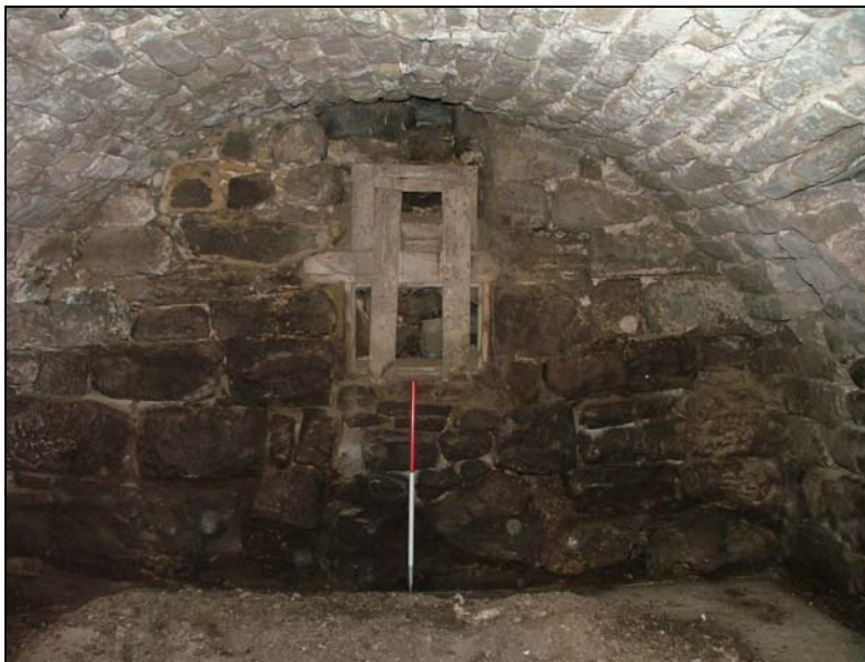
Figure 8 Interior view, northern wall, 1m scale. The panelling has been removed from the wall, and the wall cleaned, but the boarding remains on the void.
