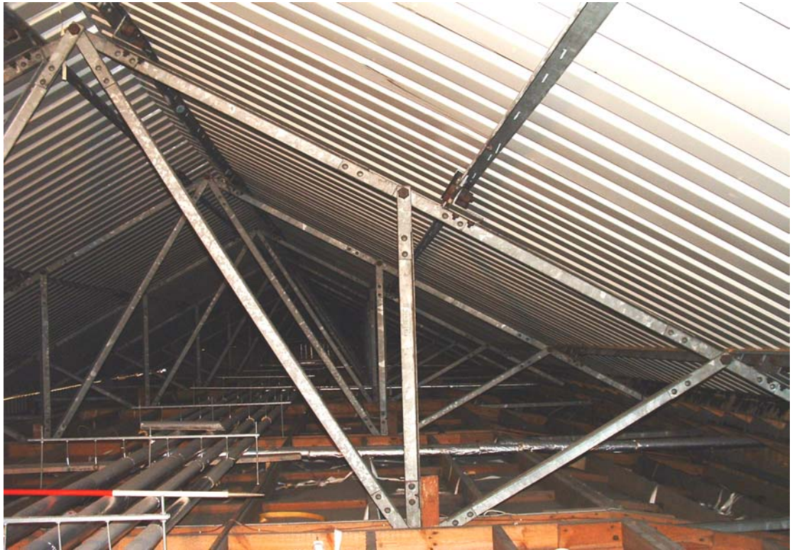
Figure 2 The eastern side of the roof truss, looking south-eastwards. The roofing sheets are fixed to light metal purlins bolted to the cleats; the trusses are fixed directly to the building's frame.
