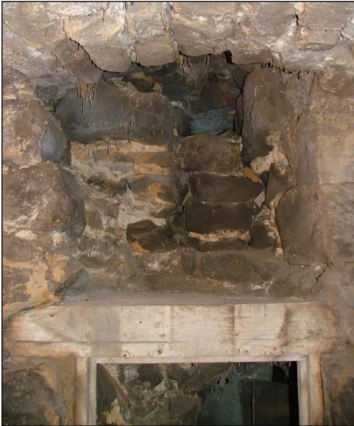
Figure 13 The north wall, after removal of the boards over the void. The sloping cast concrete above the horizontal beam is visible.
