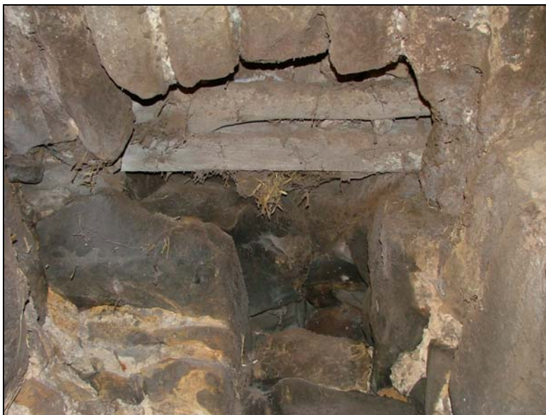
Figure 12 North wall, looking upwards into the void. A 'chimney' of collapse is visible at the bottom of the image, and several blocks that have fallen from the vault. The two beams appear to support a slab, possibly a repair to the floor above.
