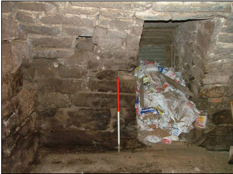
Figure 10 Interior view, eastern wall, 1m scale. Panelling has been removed and the area cleaned, but blocking remains in the disused doorway.
