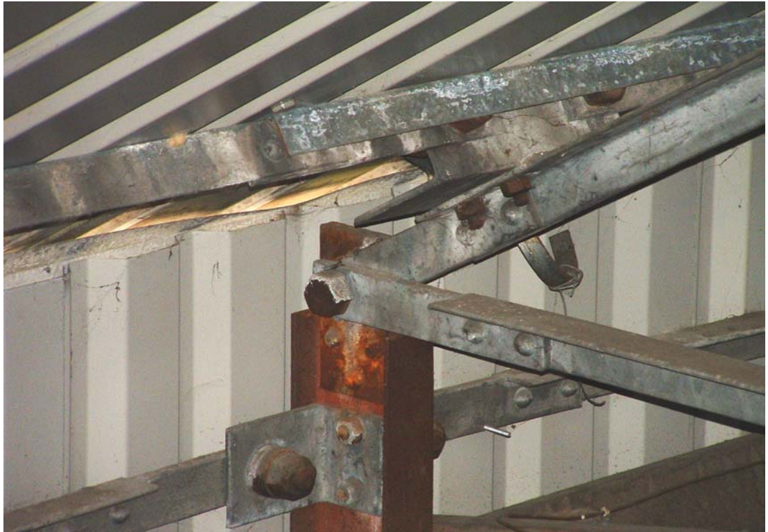
Figure 3 The connection between the roof truss and a steel upright on the south-west face of the building.
