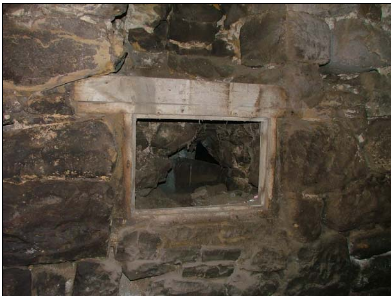
Figure 14 North wall. A close image of the wooden frame set into the stonework, directed through the void to the hole in the outer face of the wall. This illustrates the incline of the void, demonstrating the angle at which it passes through the wall.
