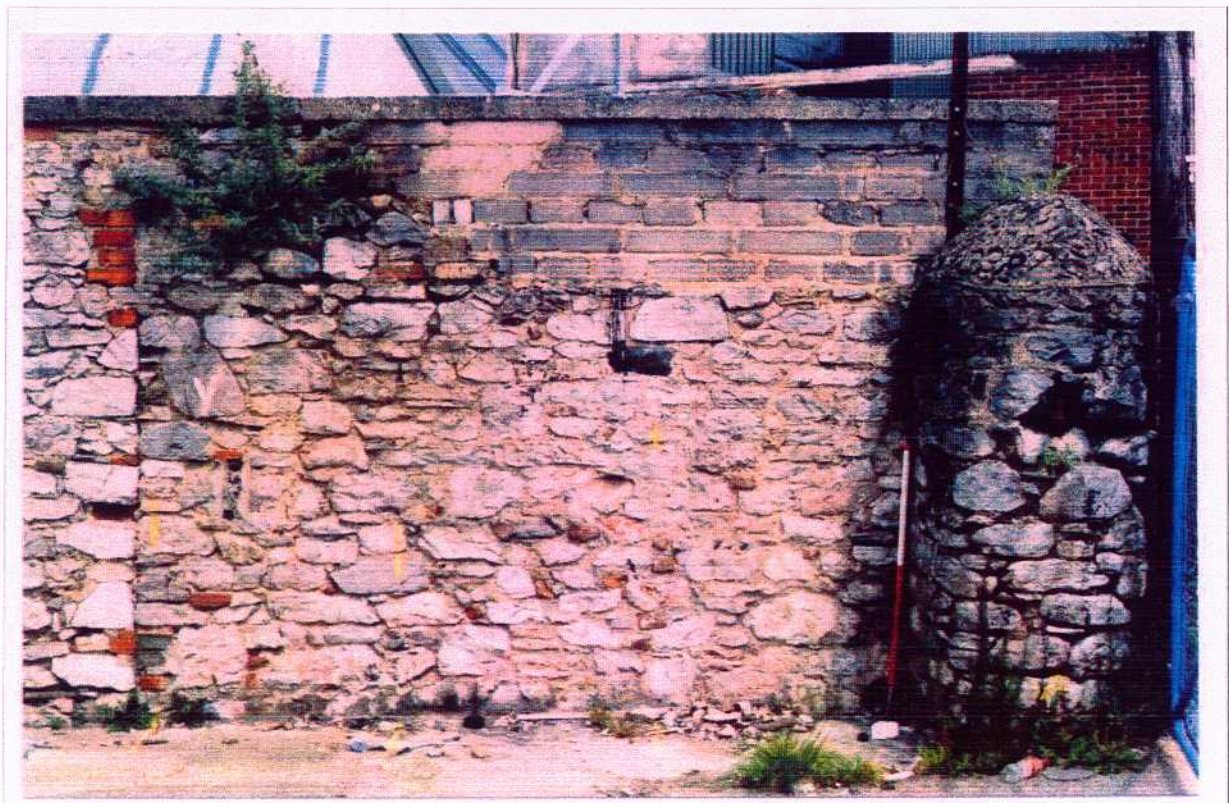
Figure 15. Structure 2. West-facing elevation of east wall, showing break with quoining and coped stub of southern wall.
