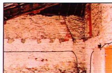
PLATE 17----- L/30/2005-29A-8405 DETAIL OF BLOCKED SOCKETS WITHIN BUILDING
