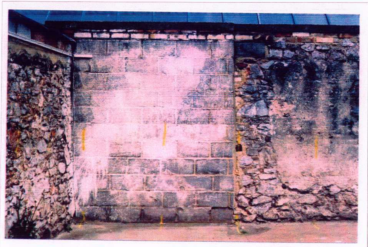
Figure 17. Structure 2. West-facing elevation of eastern wall, showing breeze-block stretch at north end.
