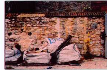
PLATE 13----- L/30/2005-29A-8413 VIEW OF BLOCKED ENTRANCE IN BOUNDARY WALL
