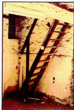
PLATE 1----- L/30/2005-5-8410 STAIR DETAIL WITH BLOCKED WINDOW
