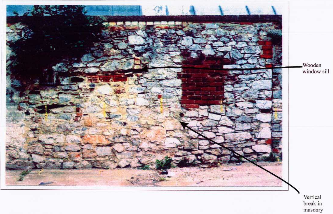
Figure 16. Structure 2. West-facing elevation of eastern wall showing blocked windows and masonry break.
