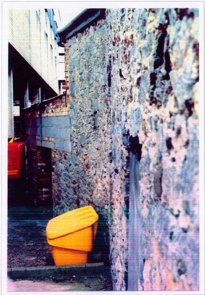
Figure 14. Junction of Structures 1 and 3, looking east. Partial new build with breeze-blocks is western end of Structure 1.
