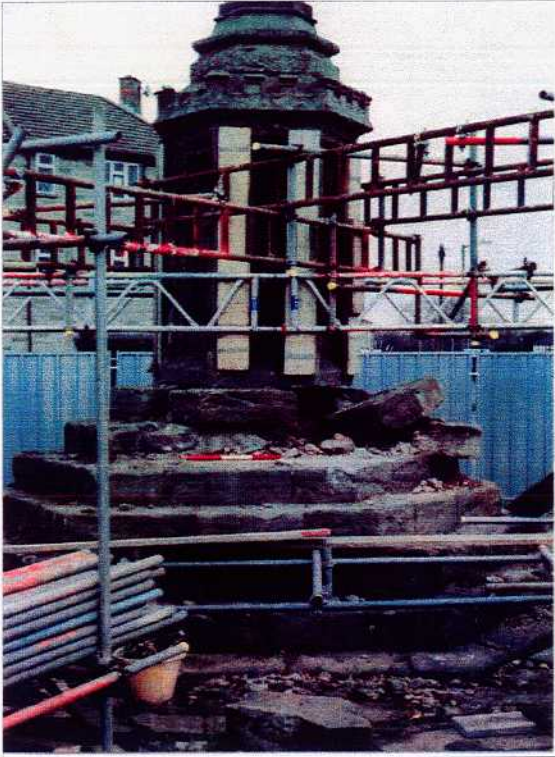
Plate 1, Damage to the monument steps resulting from the accident.
