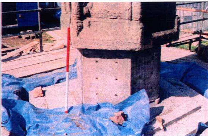
Plate 5, Cast concrete shaft with fixing/securing holes, on the bottom of the pediment, after being re-positioned on its new concrete pad.
