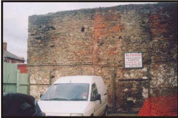
e. Wall on the line of City Wall to the north of Bastion House
