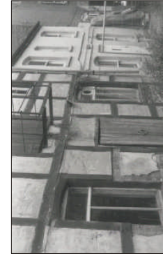
Plate 1. The granary and the cottage located to the rear (east) of number 13 South Street, as viewed from the east before work commenced on the site.
