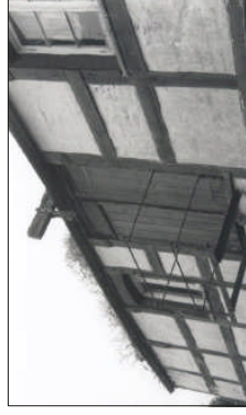
Plate 9. The granary balcony, pulley and double doors, 1st floor of the granary (the timber framing is a false cladding).
