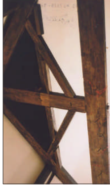
Plate 8. Truss in the bedroom of the cottage, bolted from below, raking struts lean out from the King post.
