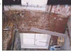
Plate 14. Original doorway between the granary and the cottage, north opening, the top of the arch has become flattened.
