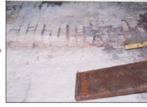
Plate 15. A step in the south wall between the granary and the lean to (east end), possibly tidied up after removal of a returning wall.
