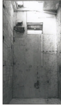
Plate 11. (Reverse of plate 6) the west wall of granary before the alterations were made, a straight joint was visible at the south (left) end of the elevation, the north end was obscured by plaster and paint.
