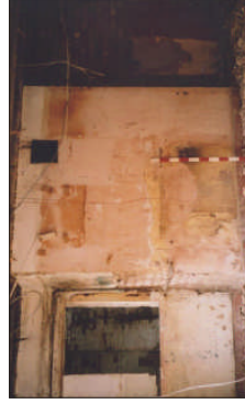
Plate 6. East wall of the cottage, prior to unblocking of the original doorways flanking the chimney breast.
