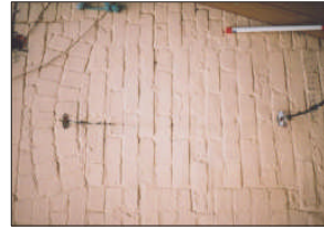
Plate 2. Blocked original doorway into the cottage (north face).
