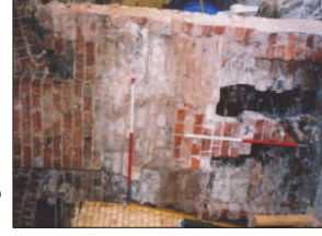
Plate 13. Central (much altered) chimney, flanked by openings between the granary and cottage.
