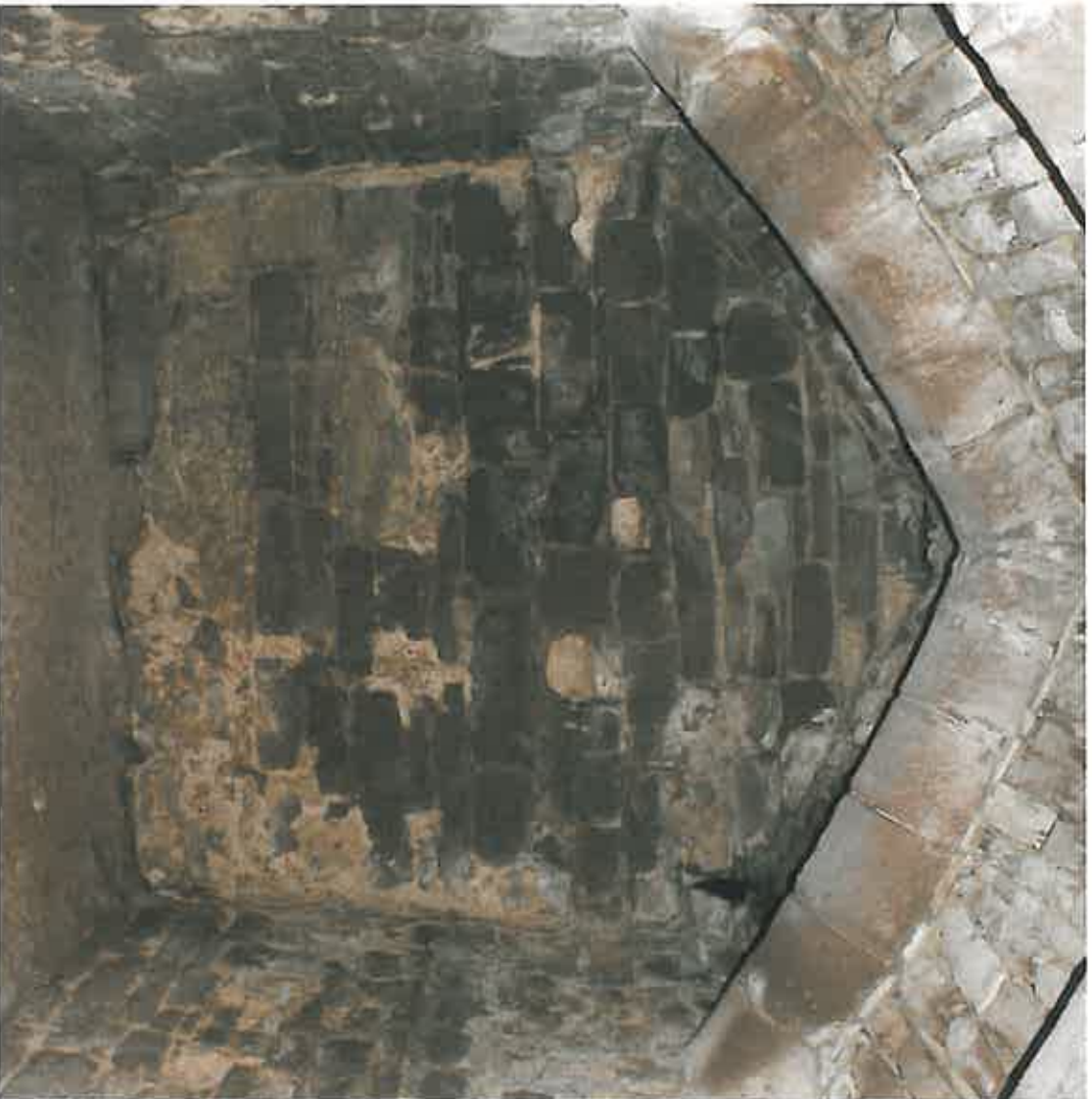
Plate 9. The rear wall of the dungeon with obvious signs of repair and maintenance
