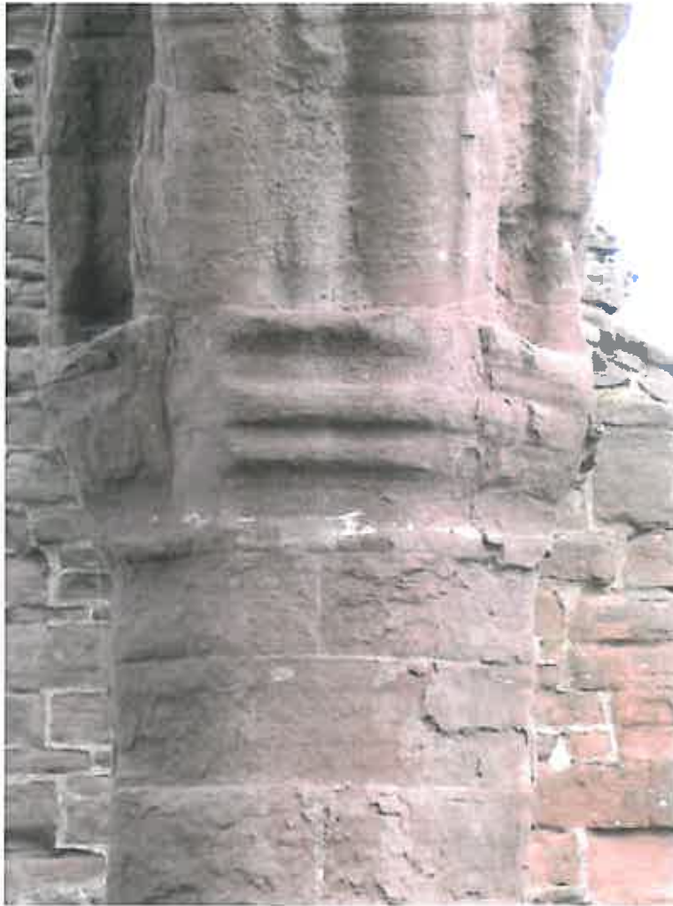
Plate 3. The effects of erosion on the pier capital
