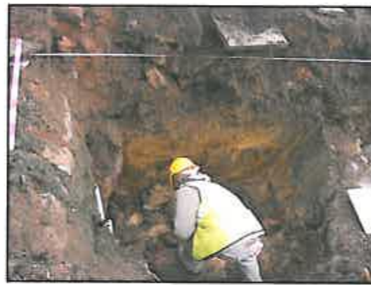
Plate 2, Trench 1, facing east, cleaning up rubble in the north end of the trench before cleaning the section for drawing.
