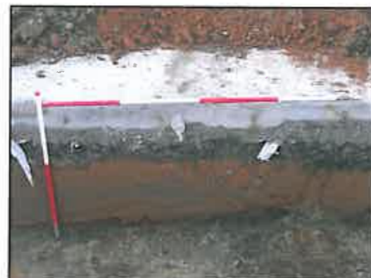
Plate 12, Trench 3, facing west, shows the thickness of the concrete surface, the scalpin sub base and the underlying red building sand used to fill and level the site before the bus station was built.
