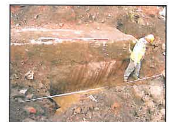
Plate 5, Trench 1, facing west. There are sheet pile impressions on this side of the concrete pile.
