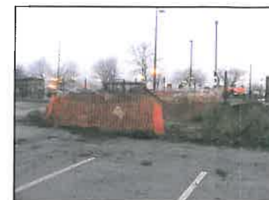
Plate 19, Trench 2, all the trenches were fenced off each evening until they were backfilled, which was done for the health and safety of the general public.
