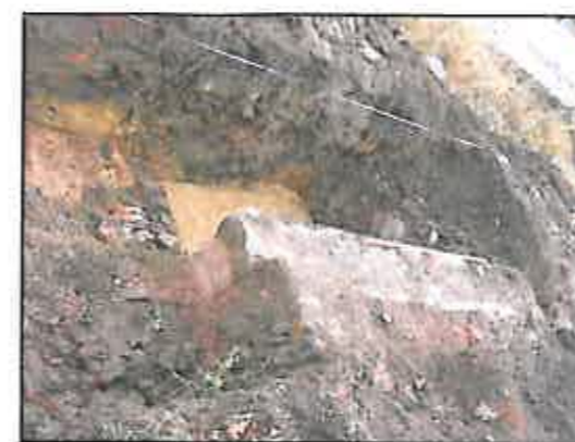
Plate 3, Trench 1, facing south-east, the concrete pile foundation is in the foreground, the area behind it is made ground overlying natural clay.
