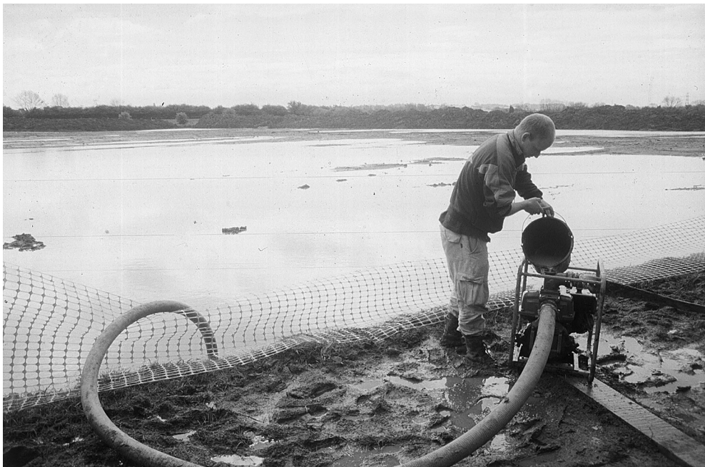
3 General view of flooded site
