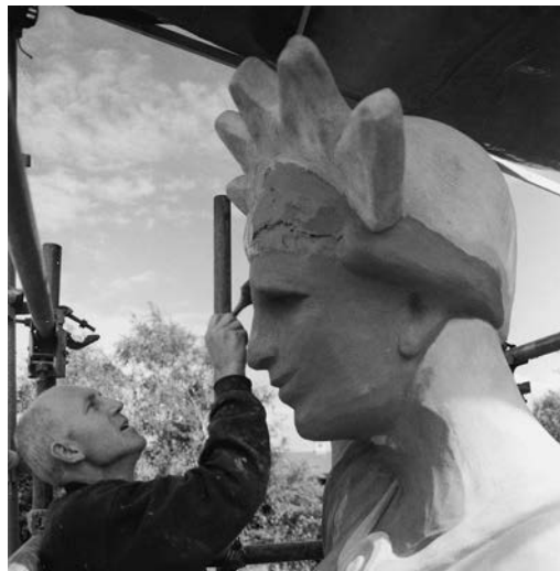
Fig. 9. The Liberty statue undergoing restoration work by Qadriga of Northwich, Cheshire, in 2004.
