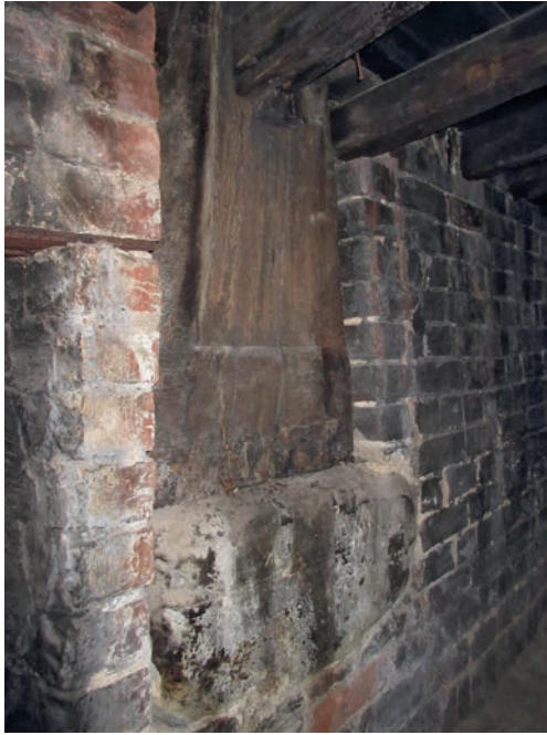
Fig. 14. Leicester Castle Hall; the foot of aisle post f, sitting on an inserted padstone, with horizontal step where the projecting base has been cut back. Image N Hill.
