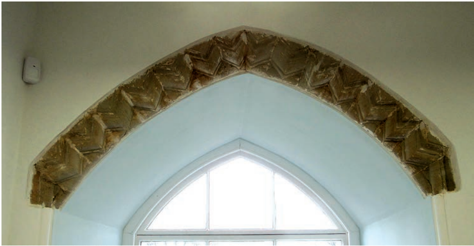
Fig. 17. Window to west elevation with pointed arch and chevron ornament. Image N Hill.
