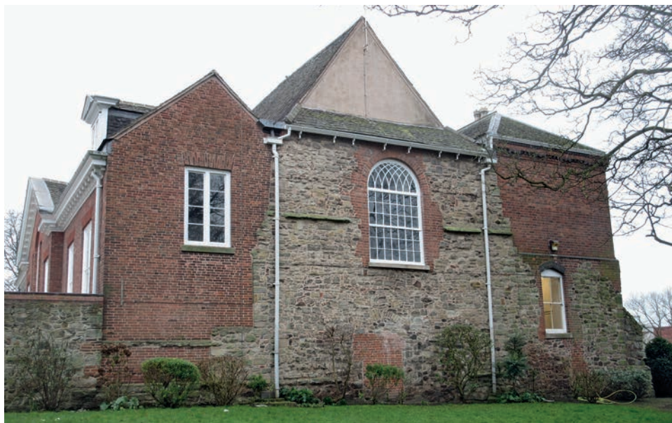
Fig. 19. The north gable. Note the projecting stone weathering to either side of the large window, indicating that an original building abutted against this wall. Image N Hill.
