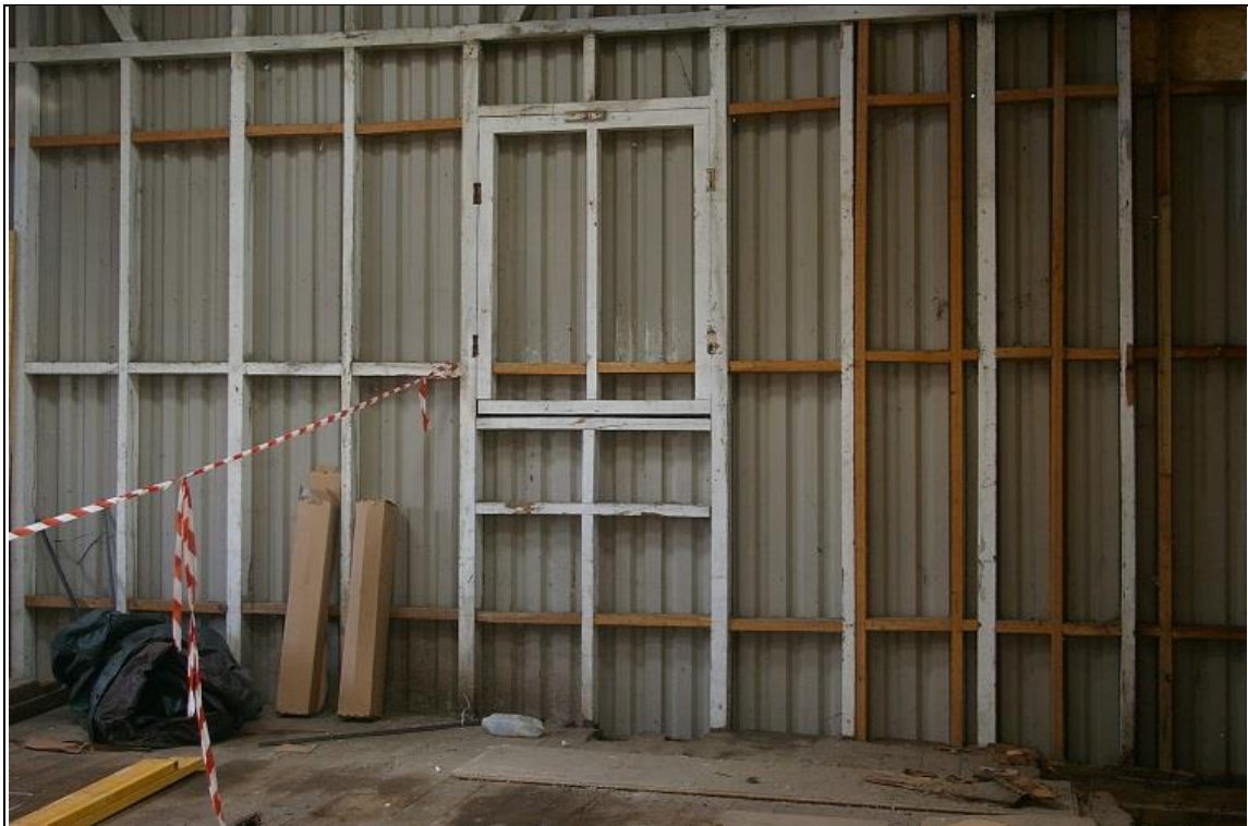
28. THE WINDOW IN THE SOUTH-EAST GABLE END WALL OF THE BUILDING, WITHIN THE TIMBER FRAME AT FIRST FLOOR; FROM THE WEST.
