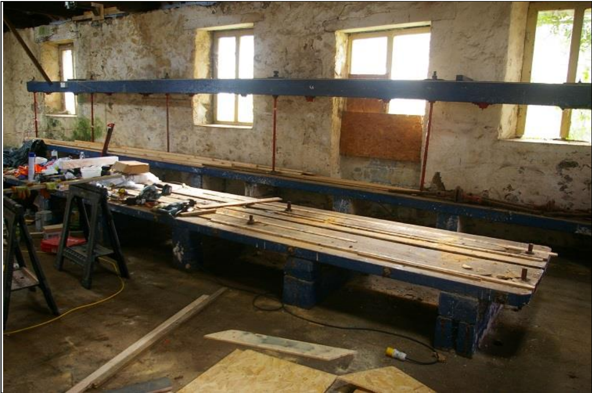
29. THE INTERNAL HEAVY TIMBER FRAMEWORK, ASSOCIATED WITH THE FISH CELLARS USE, AS IT CUTS ACROSS THE LOADING DOORS, FOR DRYING AND STORING EQUIPMENT; FROM THE NORTH.
