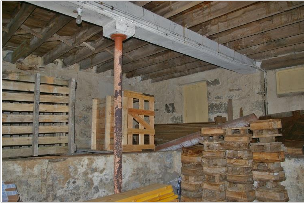
11. THE NORTH END OF THE GROUND FLOOR OF THE BUILDING, B1A – SHOWING OPENINGS AND CONCRETE FISH PITS AND TIMBER FRAME; FROM THE EAST.
