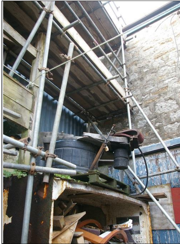
5. THE JOINT BETWEEN B1A AND B1B, SHOWING B1A ABUTS THE EARLIER STONE BUILDING; FROM THE EAST.
