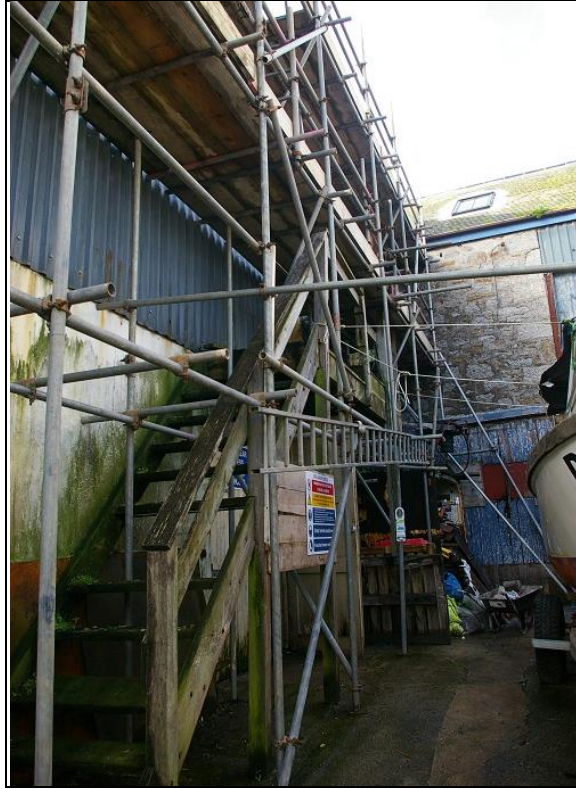
3. THE NORTH-EAST 'FRONT' OF THE BUILDING (2M SCALE), TIMBER-FRAMED EXTERNALLY CLAD IN MODERN CORRUGATED SHEETING; FROM THE EAST-SOUTH-EAST.
