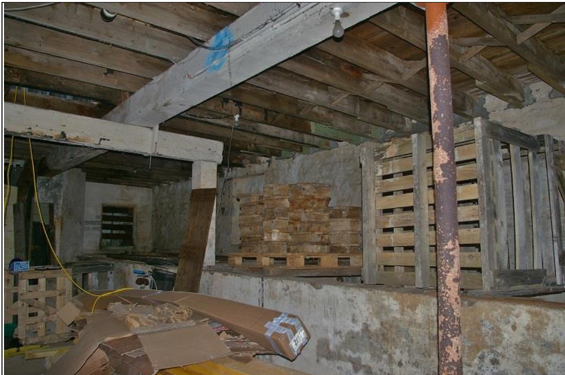
10. THE GROUND FLOOR INTERIOR - SHOWING MASSIVE FRAME, CARRIED ON CAST IRON COLUMN; FROM THE NORTH.
