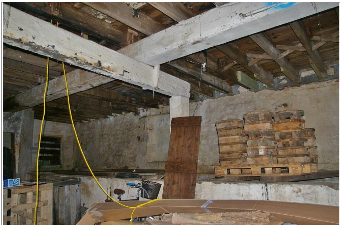
18. THE MASSIVE TIMBER FRAME WHICH CARRIES THE FIRST FLOOR; FORM THE NORTH.
