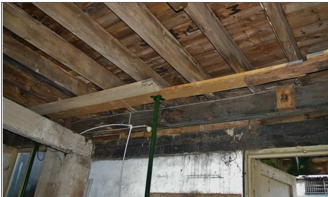
19. THE LARGE BEAM WHICH CARRIES THE TIMBER FRAME OF THE NORTH-EAST WALL - NOW SUPPORTED PARTLY ON A REPLACEMENT CONCRETE PIER; FROM THE SOUTH.
