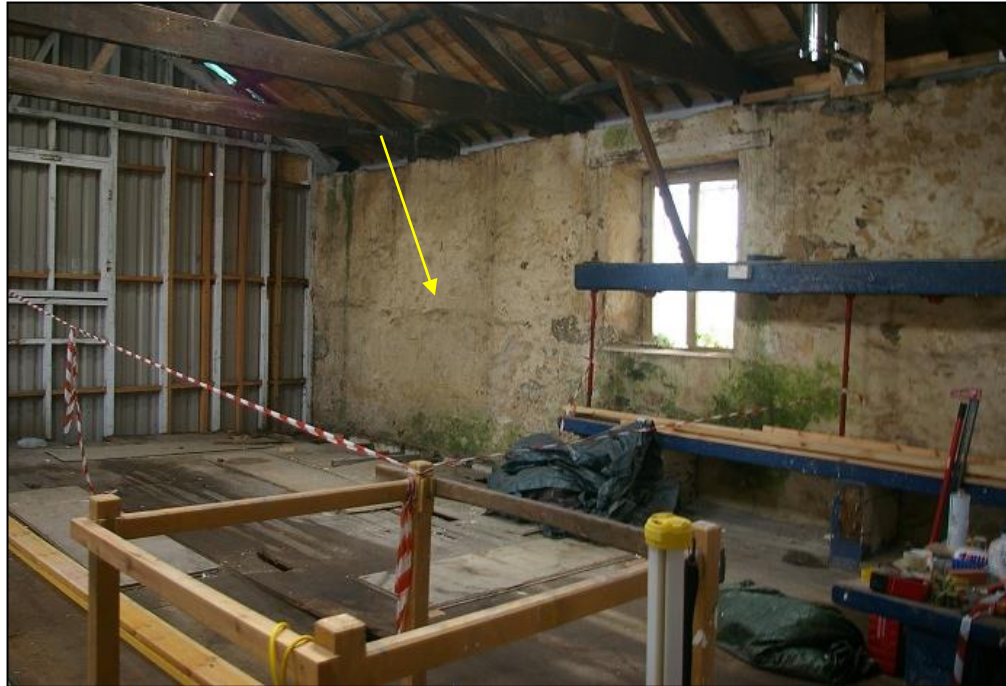
FIGURE 12: THE BUILD LINE ON THE LONG SOUTH-WEST WALL, SUGGESTING THE REUSE OF A RUINED STRUCTURE; FROM THE NORTH.
