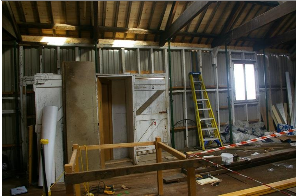
27. THE NORTH-EAST TIMBER FRAMED WALL OF THE BUILDING, SHOWING TWO DOORS – ONE BLOCKED BY THE TOILET; FROM THE WEST.
