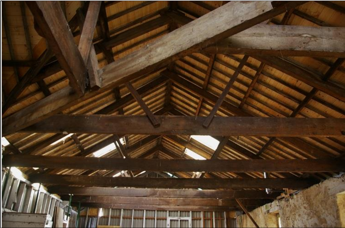
25. THE ROOF OF B1A, SHOWING LIGHTWEIGHT A-FRAMES WITH SIDE STRUTS; FROM THE NORTH-WEST.
