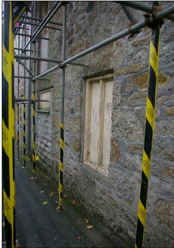
33. THE OPENINGS ON THE NORTH WEST FACADE OF B1A – SHOWING ITS RETAINED HISTORIC CHARACTER FROM THIS SIDE; FROM THE WEST.
