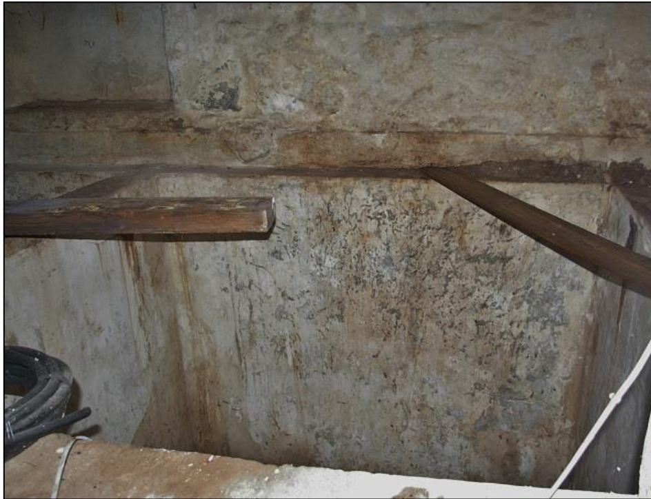
FIGURE 8: ONE OF THE RENDERED PITS FOR FISH ON THE GROUND FLOOR OF THE BUILDING; FROM THE NORTH-NORTH-EAST.
