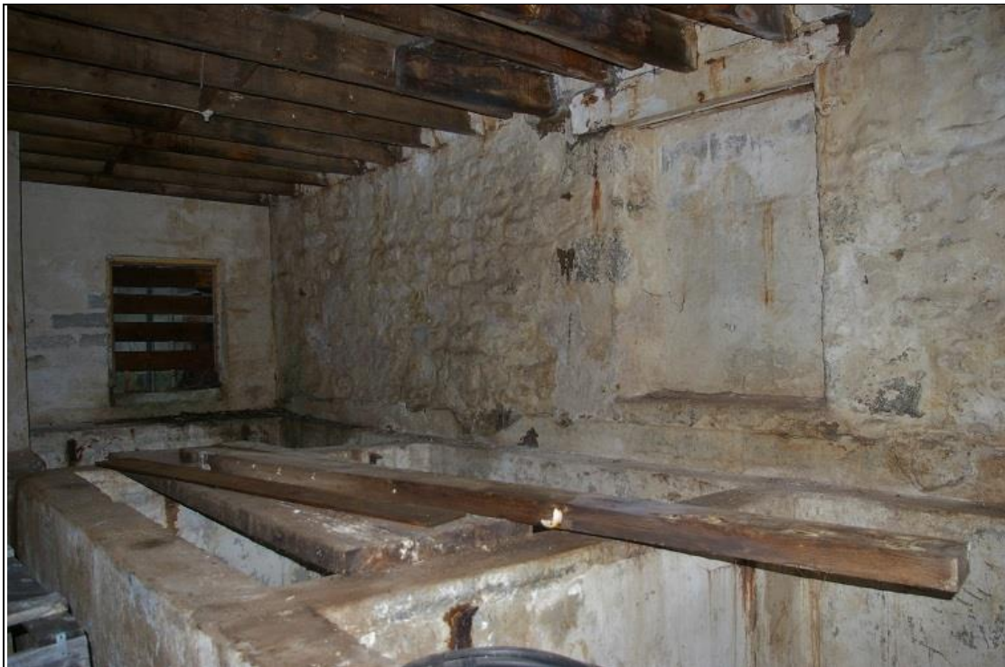
12. THE RELATIONSHIP BETWEEN THE LONG SOUTH-WEST STONE WALL - BLOCKED OPENINGS AND CONCRETE FISH PITS; FROM THE NORTH.
