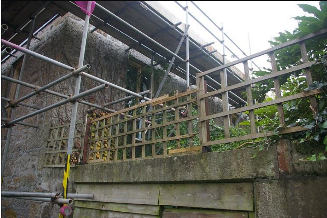
34. THE NORTH-WEST AND SOUTH-WEST STONE WALLS OF B1A – THE 1 ST PHASE OF THE BUILDING, WHEN IT ORIGINALLY EXTENDED B1B; FROM THE WEST.
