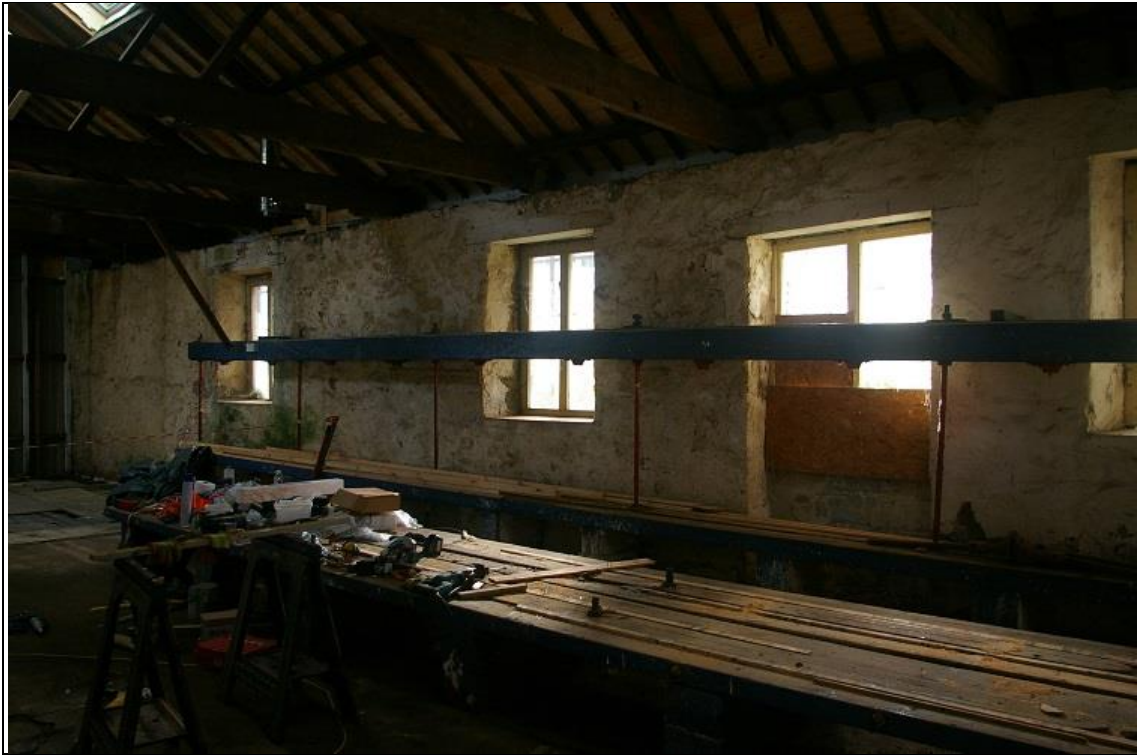
23. THE LONG SOUTH-WEST WALL - SHOWING CONSIDERABLE GAP BETWEEN THE OPENINGS - SUGGESTIVE OF STRUCTURAL PHASING; FROM THE NORTH.
