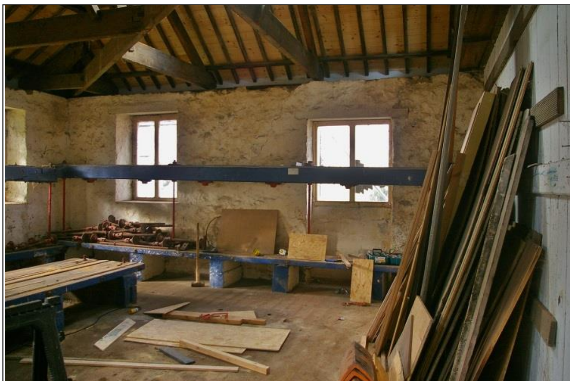
21. THE NORTH-WEST WALL OF THE BUILDING, WITH WINDOW AND BLOCKED LOADING DOOR, AT FIRST FLOOR; FROM THE EAST-SOUTH-EAST.
