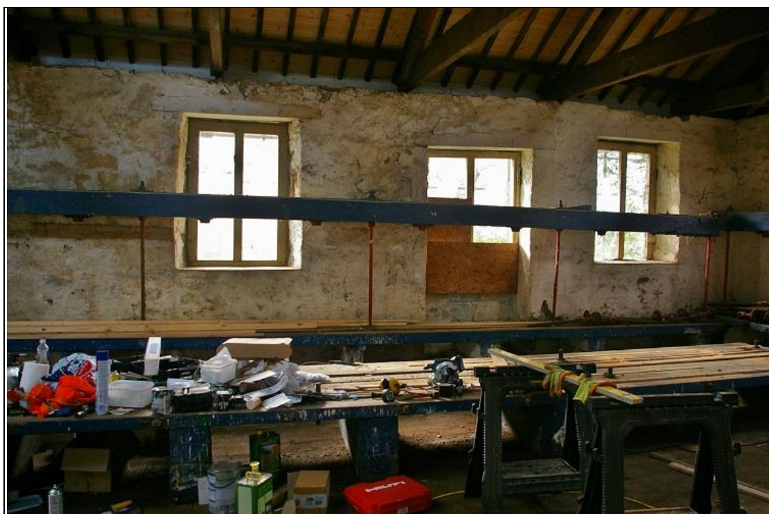
22. THE SOUTH-WEST WALL OF B1A, AT FIRST FLOOR - SHOWING ARRANGEMENT OF THREE OPENINGS AT THE 'NORTH' END - TWO WINDOWS FLANKING A NOW BLOCKED LOADING DOOR - SUGGESTING WAREHOUSE USE PREVIOUSLY; FROM THE EAST.
