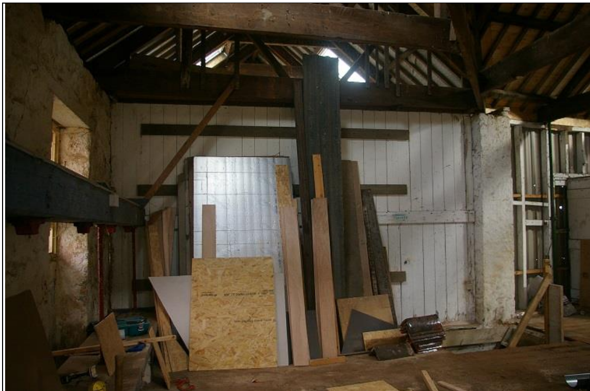
26. THE PARTITION WALL TO B1B – TIMBER PLANK BOARDING CARRIED ON HEAVY LEDGING BARS BETWEEN THE WALL AND GRANITE PIER; FROM THE WEST.
