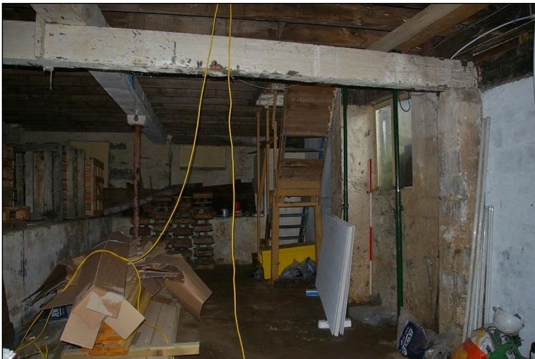
FIGURE 6: VIEW OF THE WAREHOUSE, WITH IN SITU RENDERED PITS (WITH 2M SCALE); FROM THE SOUTH-EAST.
