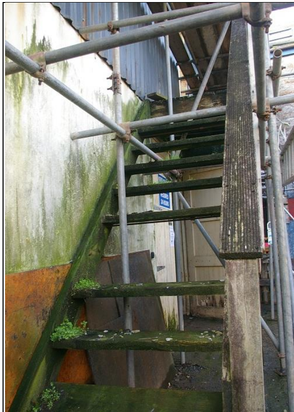
4. THE MODERN STAIRCASE ON THE NORTH-EAST FRONT OF THE BUILDING - NOW ROTTEN; FROM THE EAST.
