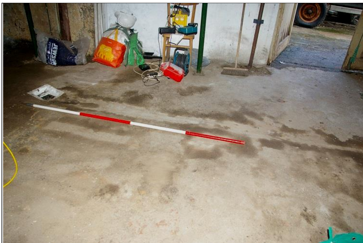
20. THE CONCRETE FLOOR OF THE BUILDING, WITH OFF-CENTRE DRAIN (2M SCALE); FROM THE SOUTH.
