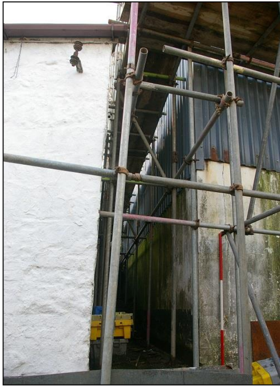
1. THE SOUTH-EAST GABLE END OF THE BUILDING (2M SCALE), WITH SMALL ALLEYWAY BETWEEN IT AND THE ADJACENT BUILDING; FROM THE EAST.
