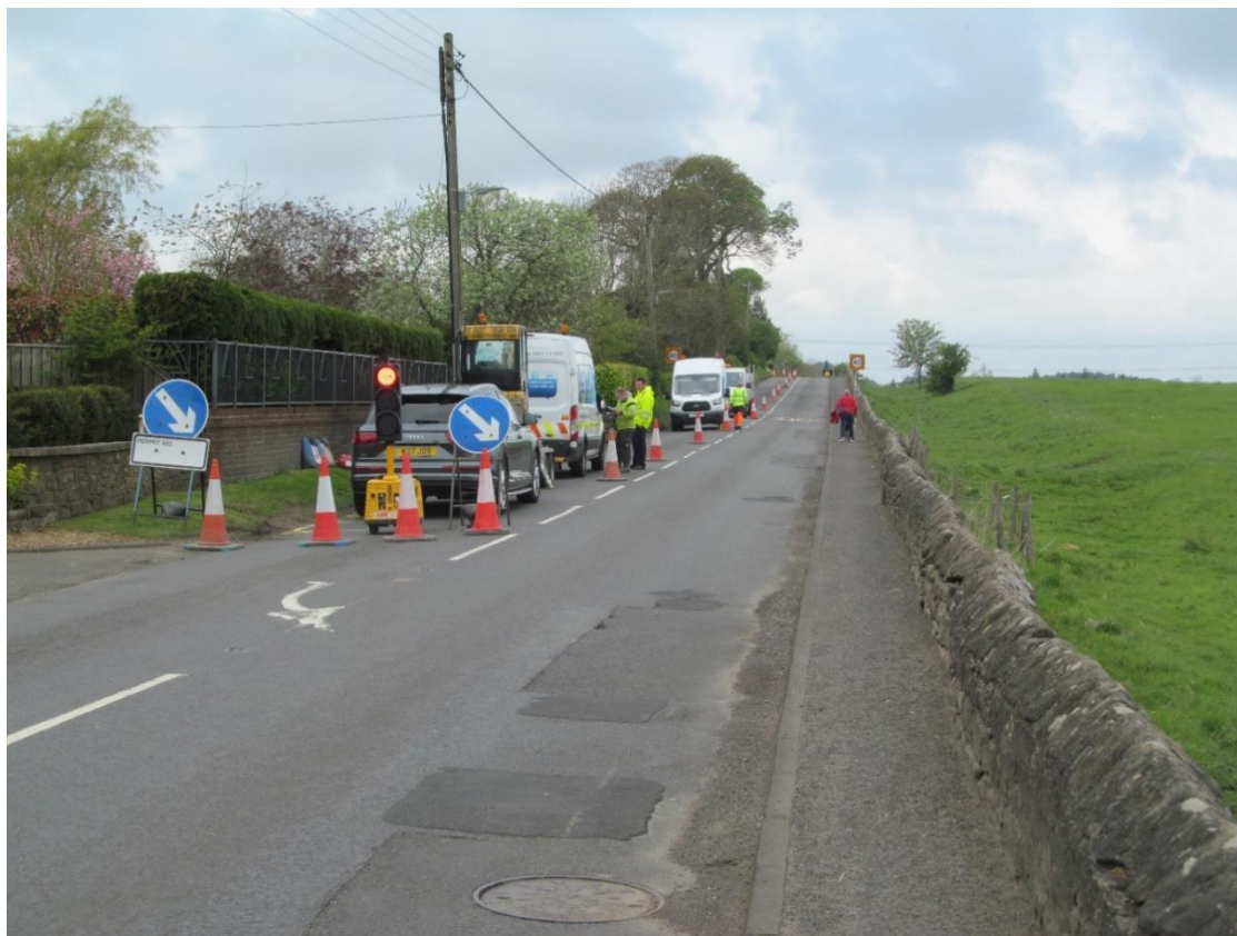
Figure 3: Pre-excavation view along Military Road from the eastern end of the excavation, looking west-south-west
