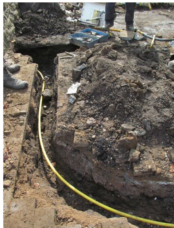
Figure 23: Post-excavation shot of northern half of the new gas pipe, looking east
