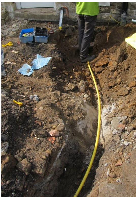
Figure 22: Post-excavation shot of southern half of the new gas pipe, looking south
