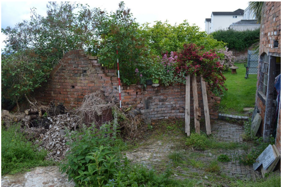
Plate 4: View west of surviving wall of former building and curved garden wall
