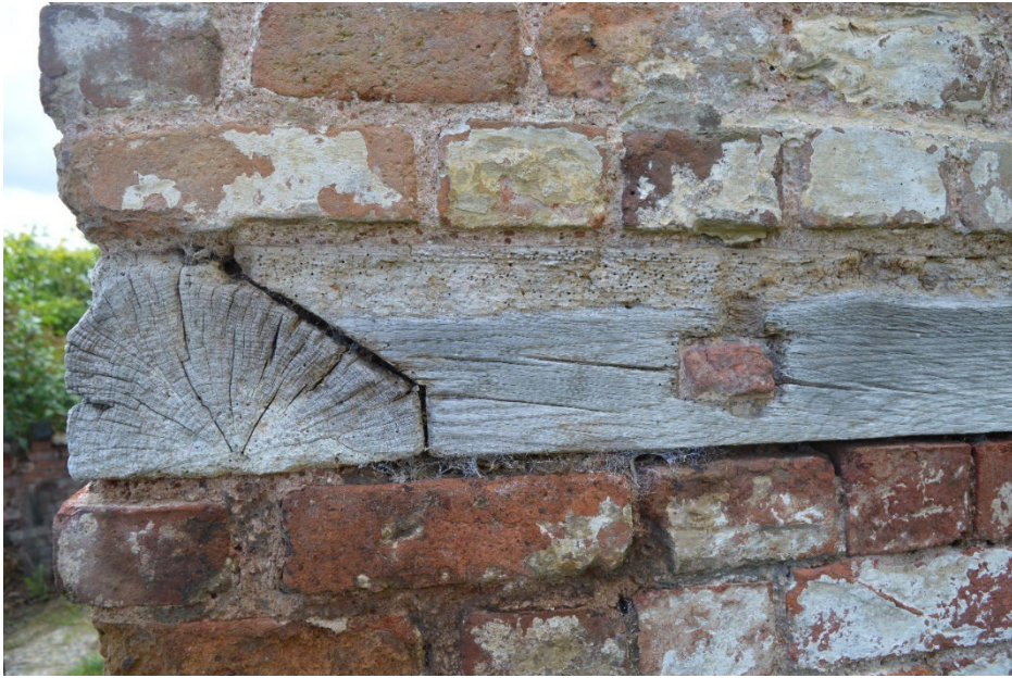
Plate 11: Joint between lintels on east and north elevations
