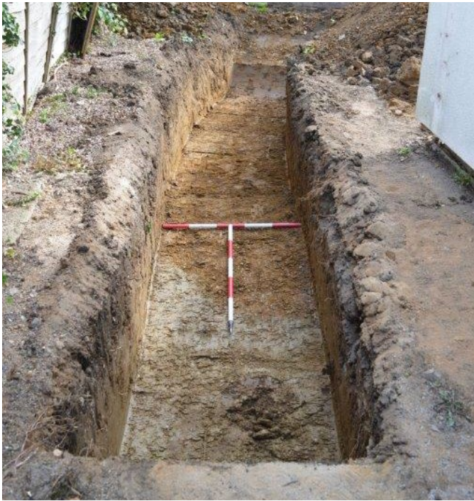
Plate 3: Trench 2 facing east (2m scales) with natural layer (203) in foreground and (204) further to the east
