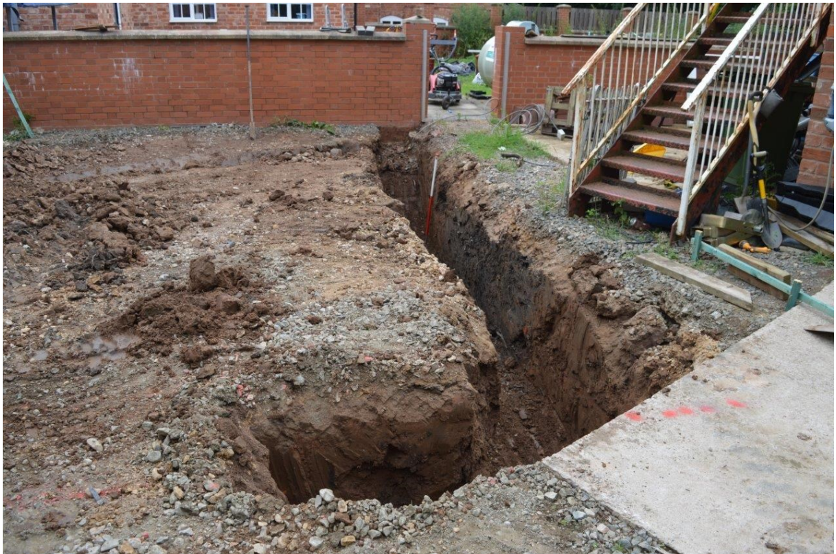
Plate 8. Trench 2 fully excavated, cut [204] to right of ranging rod, view north, scale 1m
