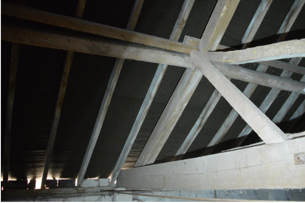
Plate 25. View south-east showing strengthened purlin in east pitch of hay loft roof
