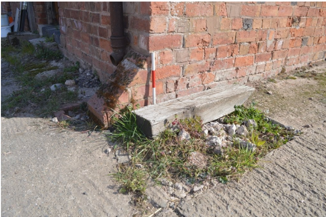
Plate 6. Low buttress at south-west corner of Stables Barn, view north-east, scale 0.3m
