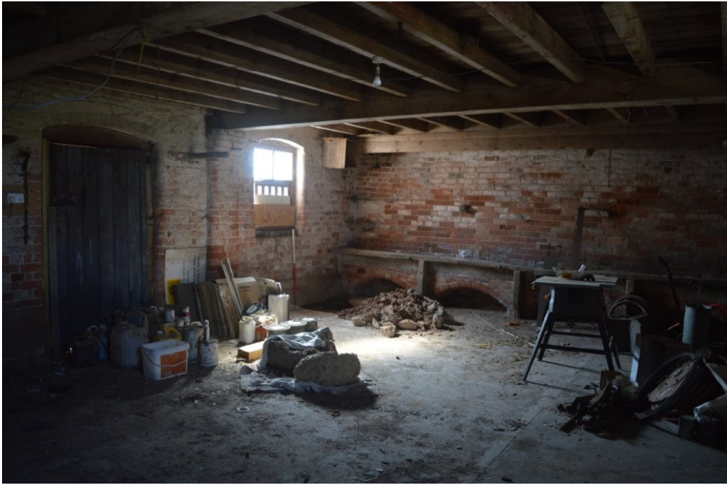
Plate 17. Stables on the ground floor of two storey section, view south-east, scale 1m
