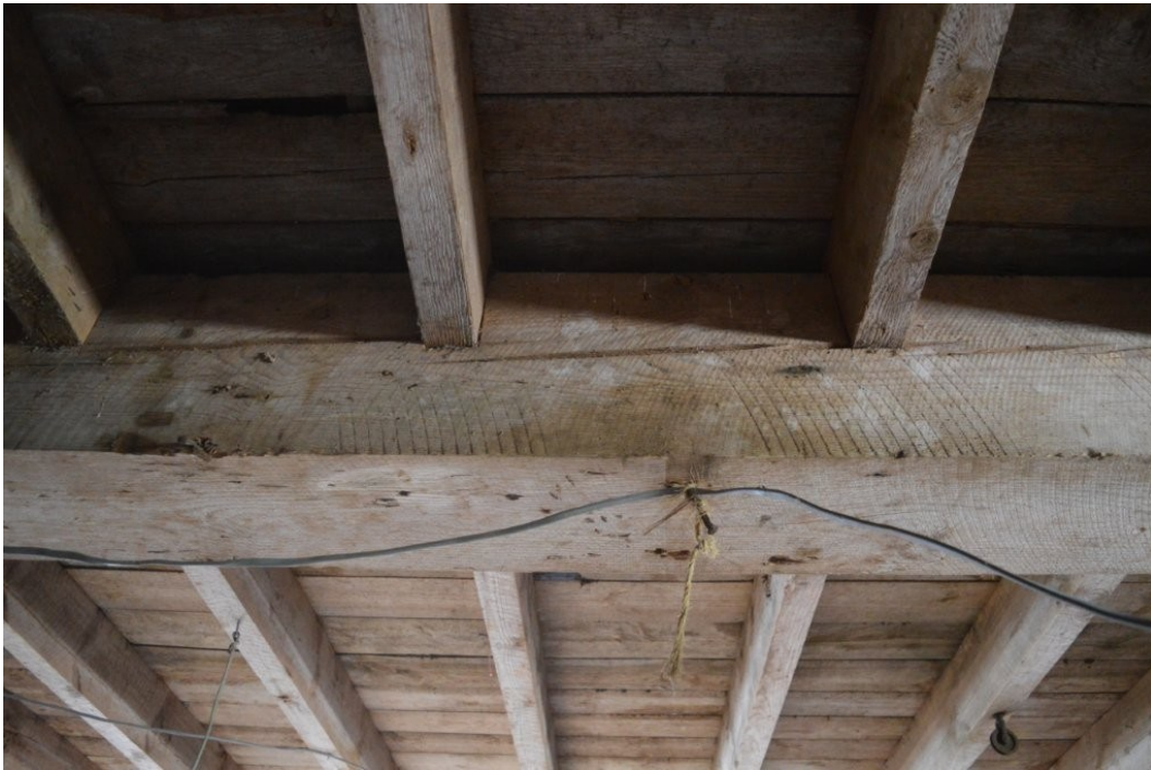
Plate 19. Circular saw marks on transverse beam above stables, view south
