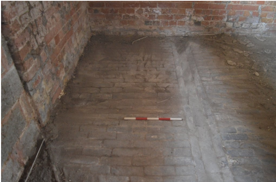
Plate 28. brick floor in eastern side of central section, view south, scale 0.5m
