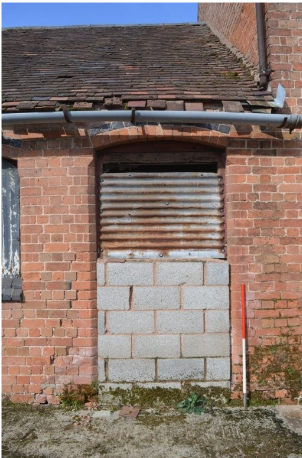
Plate 14. Partially blocked doorway in eastern elevation of Stables Barn, view west, scale 1m
