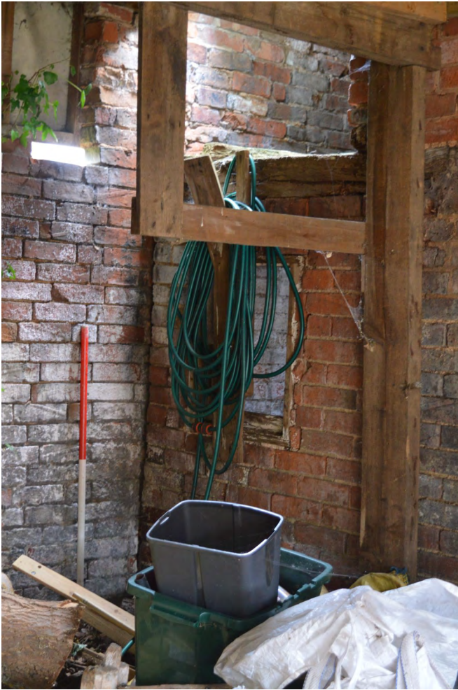
Plate 11. North-western corner of the added half bay, narrower at first floor level than ground floor level, view north-east
