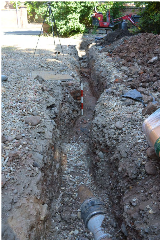
Plate 38. View east of foul pipe (107)
