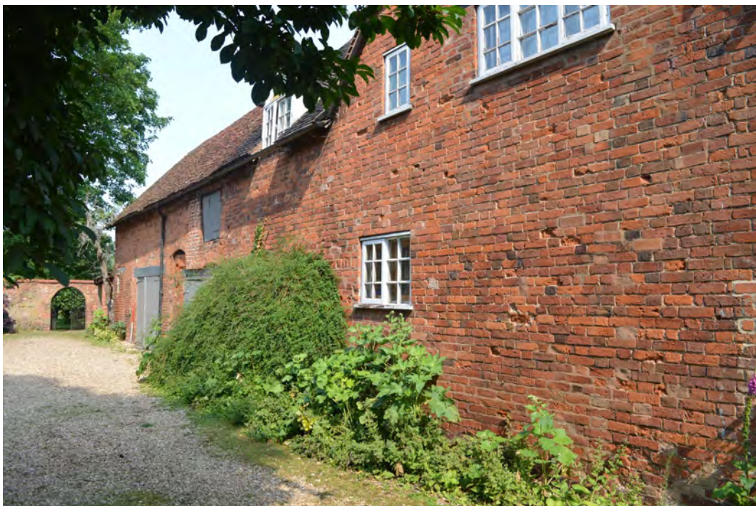
Plate 2. View north-north-west of former stable, with No. 43 High Street, Feckenham on the right hand side of the photograph
