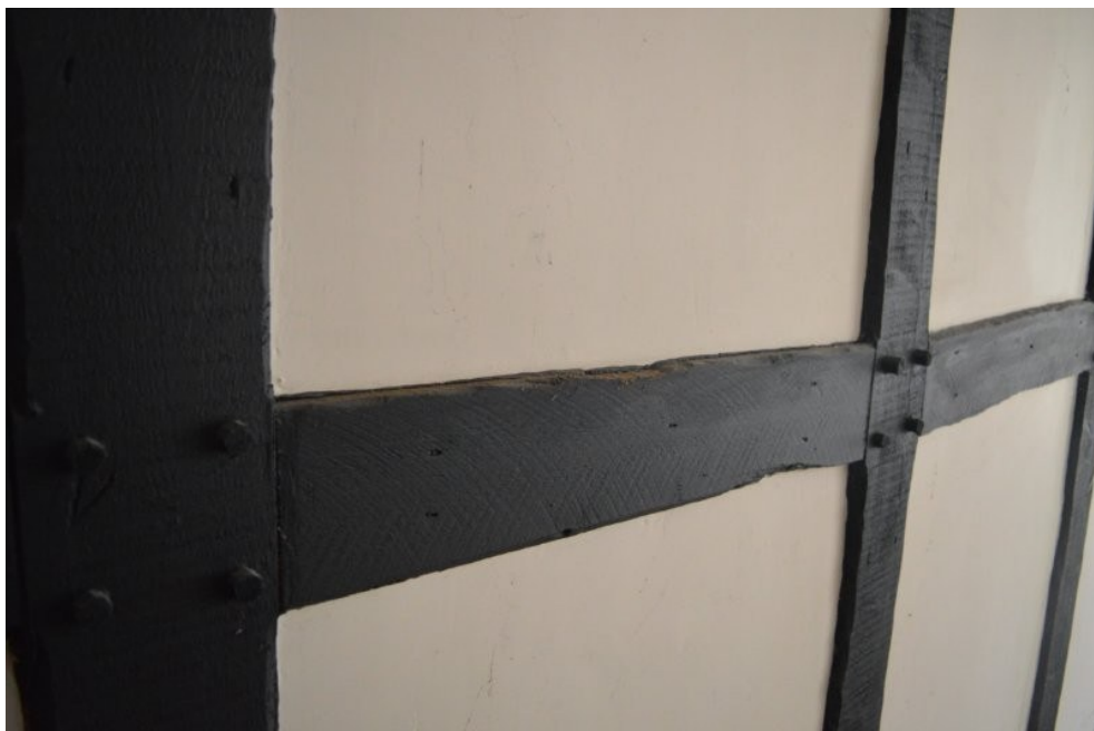
Plate 17. Differing saw marks in horizontal and vertical members
