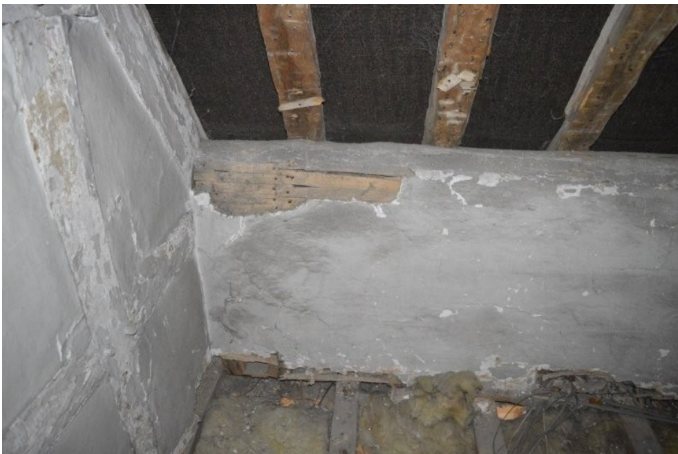
Plate 68. Lath and plastered section beneath lower purlin in space over northern rear extension
