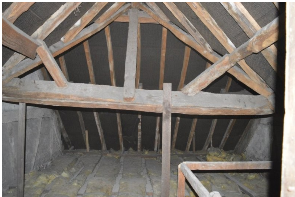
Plate 66. View west from rear extension into main axis of attic space. Note the angled struts supporting the purlins of the extension
