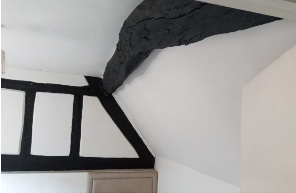
Plate 57. Bowed purlin in northern pitch of Room 18, view WNW
