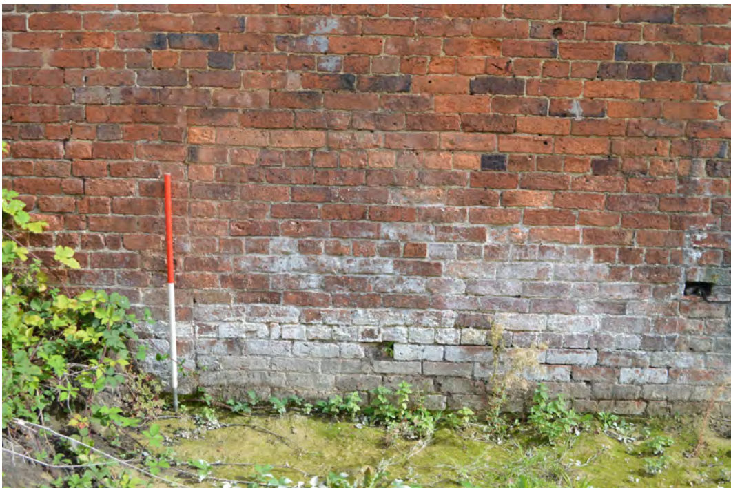
Plate 14. Brick joint in left of rear elevation
