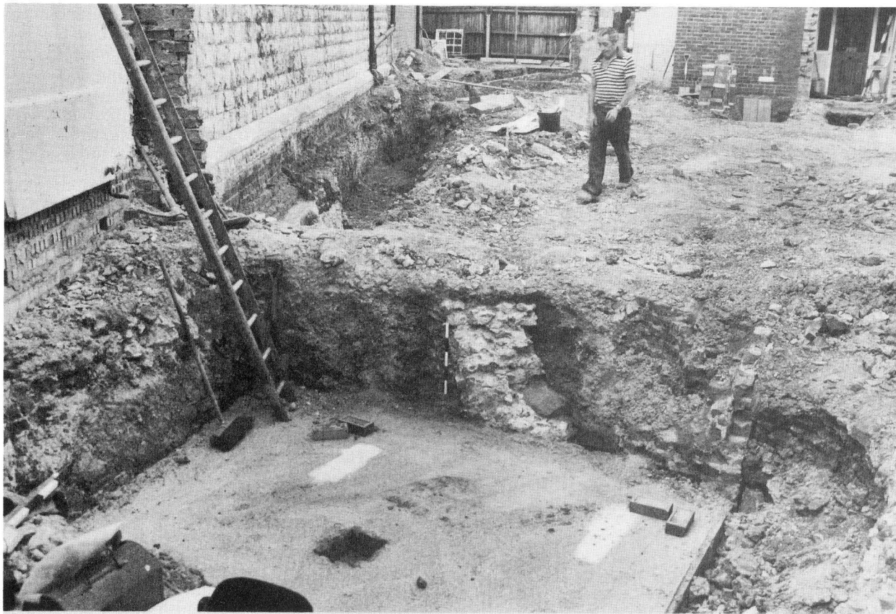
Fig. 1: View of the site, looking south, showing a wall of the cellar exposed in a contractor's excavation.
