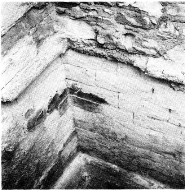
Fig. 2: the Wealden marble string course at the top of the plinth at the junction of the Bell Tower and the curtain.
