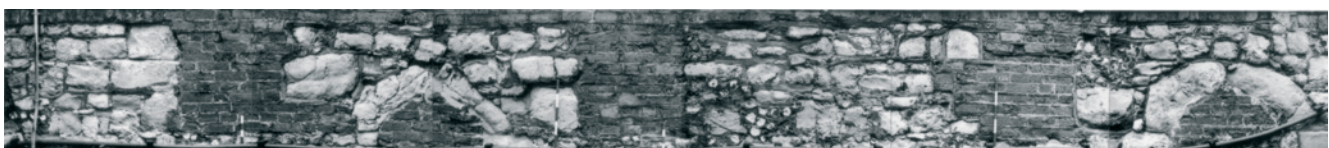
Fig. 5: composite photograph showing part of the blocked crenellations of Edward I's surviving in the Outer West Curtain Wall immediately south of Legge's Mount. The view shows the rear of the upper parts of these remarkable features and includes the arch of an arrow loop in one of the merlons (the upstanding part of the crenellations) (© author)
