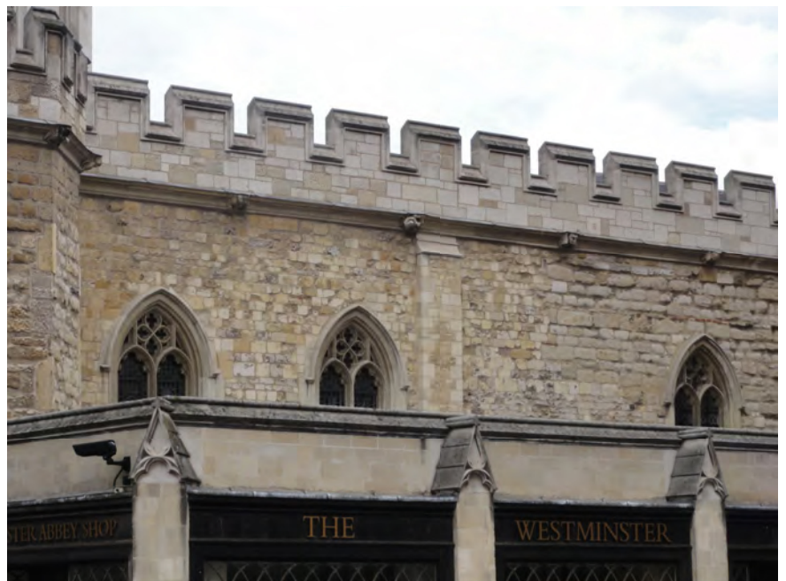
Fig. 3: west front of abbot's house showing the break in masonry between the Jerusalem Chamber and College Hall; the Kentish ragstone is visible (right)
