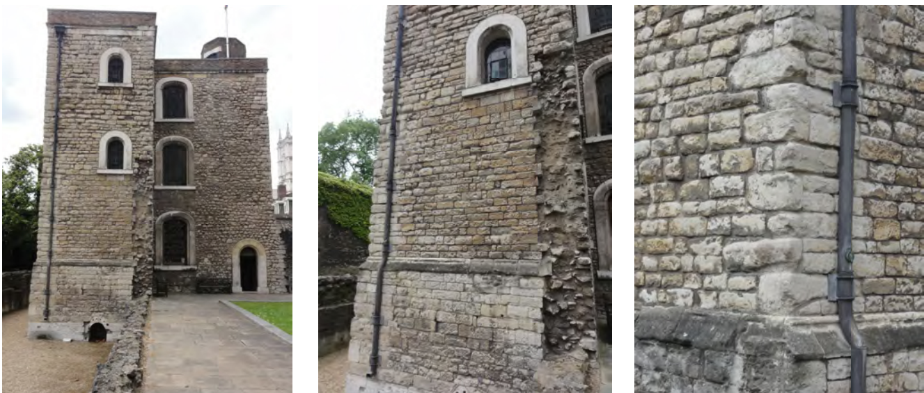
Fig. 1: the Jewel Tower, all the stone is Kentish ragstone, except the Portland stone window and door openings. View from the east (left); details of plinth and tower external face (centre) and details of the ragstone ashlar quoin and face on the north-west side (right).
