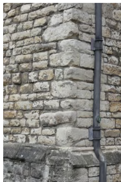
Detail of the Kentish ragstone ashlar quoin and face on the north-west side of the Jewel Tower, Westminster.
