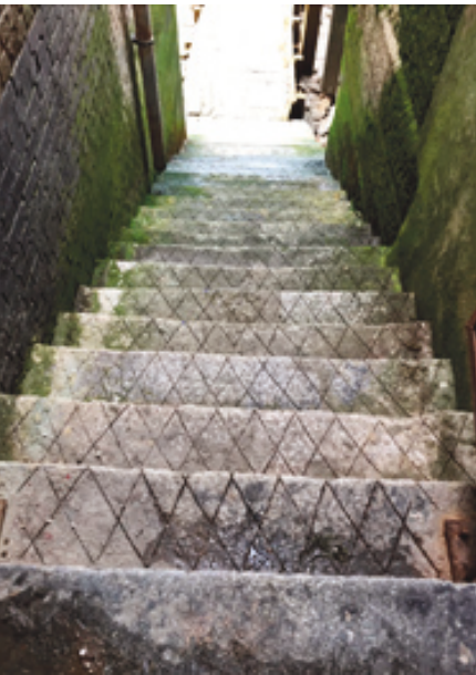
ABOVE: The steep Alderman Stairs running down to the causeway on the foreshore
