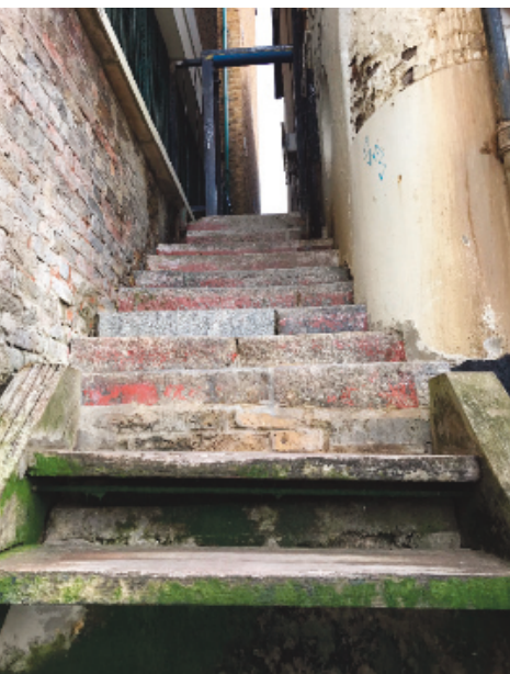
BELOW: Pelican Stairs in Wapping showing two phases of heightening of the river stair above the wooden steps
