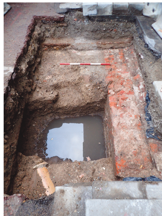
Fig 6: Trench 3, looking south-east, the early 18th-century wall can be seen along the right side of the trench continuing beyond the excavation, with a later 18th-century wall abutting it (1m scale)
