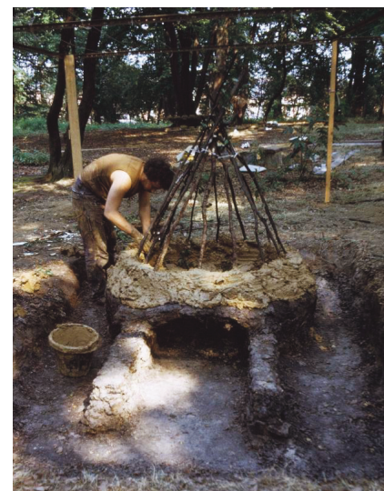
ABOVE Replica kiln construction in 1971, showing the structural use of coppice poles ABOVE LEFT One of the misshapen wasters from the excavation
