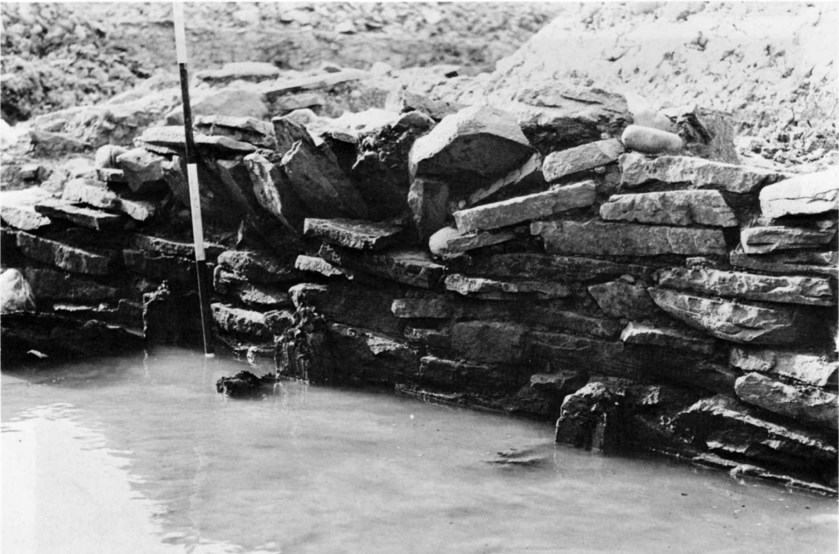
Plate IIIB. Damage caused to the secondary quay by the loosened joists of the stage, as the result of tidal action.
